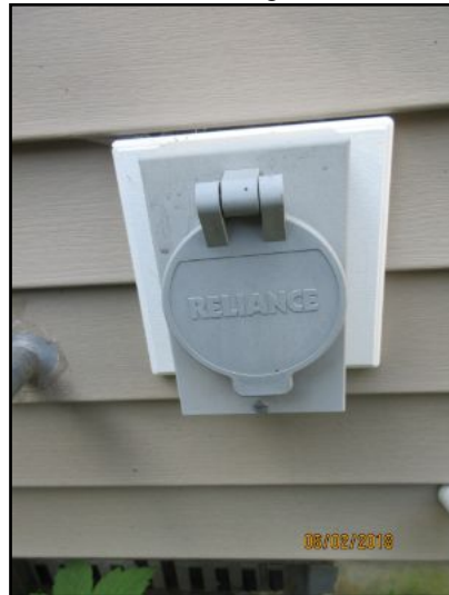
The home had provisions to connect a portable backup generator to provide the home with electricity when power is not available from public utilities. Inspection of backup generators and their electrical components lies beyond the scope of the General Home Inspection. The Inspector recommends that before the expiration of your Inspection Objection Deadline you have this backup system inspected by a qualified electrical contractor.
