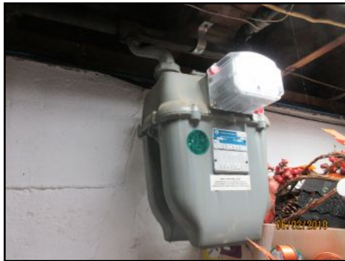
Public Gas Service: Meter, shutoff valve and vented regulator noted in basement.
