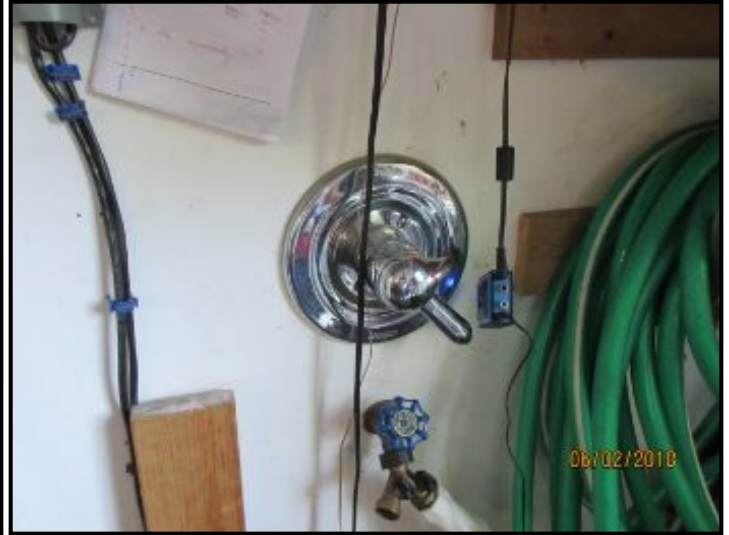
Hot/Cold mixing valve at garage hose bibb noted for washing cars.
