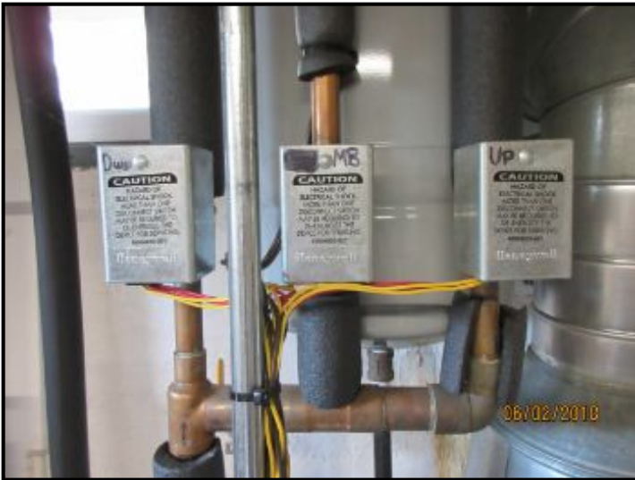
3-zone heating system noted.
