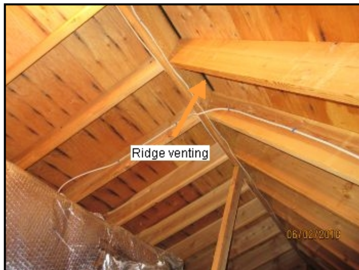
Ridge exhaust venting noted
