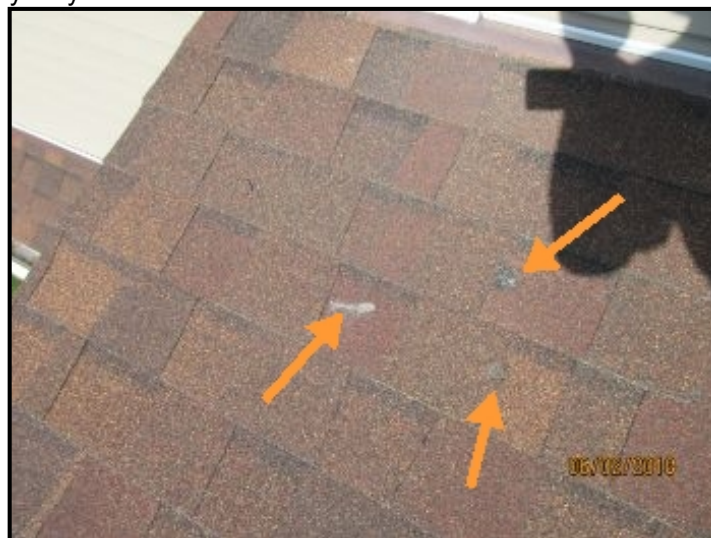
Beginning signs of minor wear and tear likely caused by walking on roof.
