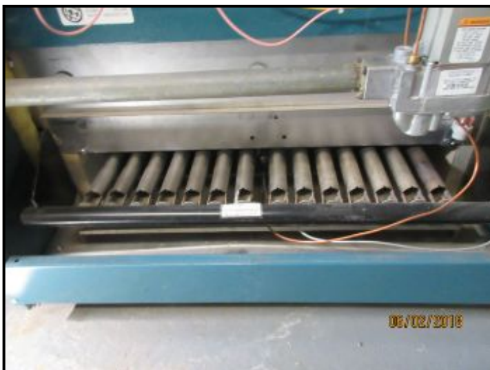
Burner fired by thermostat.
