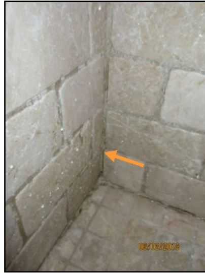
Shower wall corner grout (movement joint) is cracked. This is common; suggest replacing grout with matching silicone based sealant at corner movement joints.
