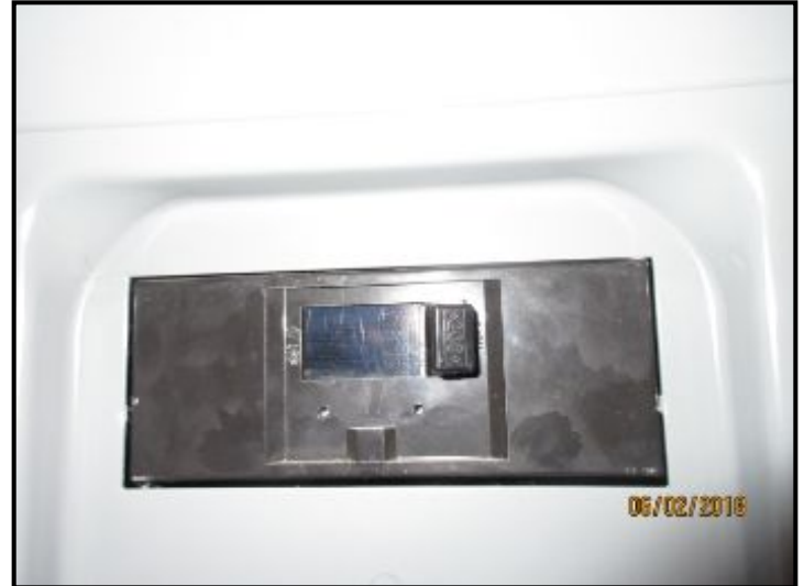
Main Disconnect: 200 amp main breaker serves the property.
