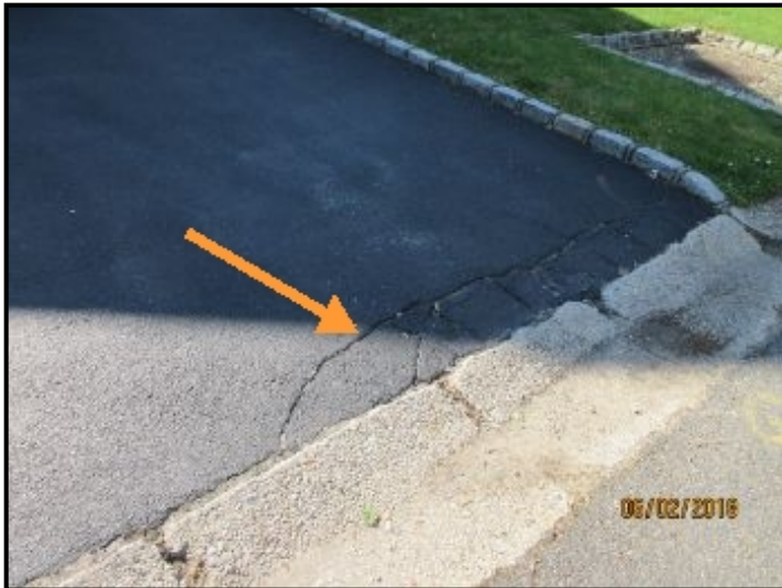
Moderate cracks in driveway near sidewalk noted. Seal cracks to prevent subsequent water entry and freeze-thaw damage.
