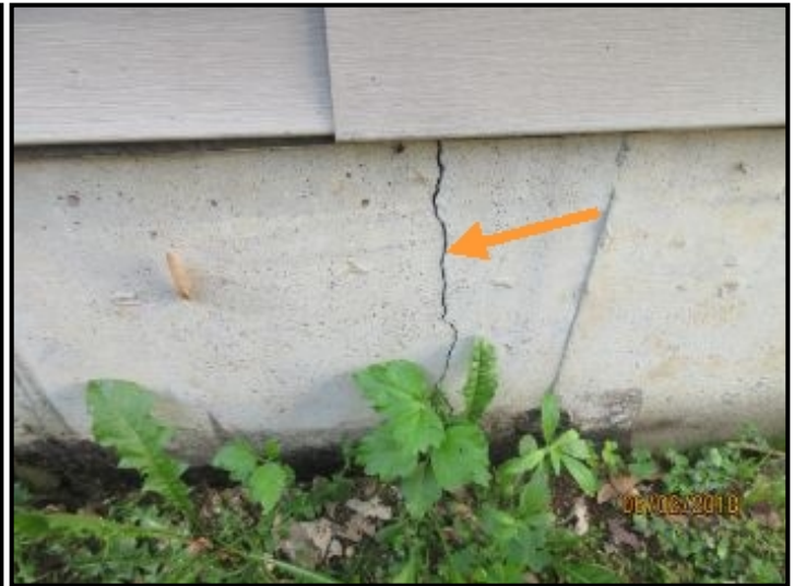
CRACKS: (1/4" or less) Cracks/Holes present in foundation wall / floor. Cracks that are less than 1/4" are not commonly regarded as being structurally significant. Recommend sealing the cracks with epoxy filler to prevent water infiltration, and monitor for further movement.
