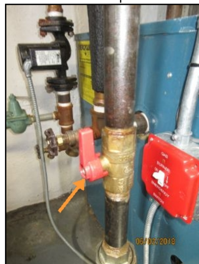
Gas supply shut-off valve located at furnace/ boiler.
