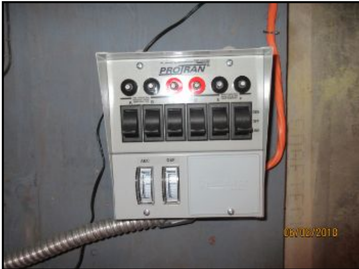
The home had provisions to connect a portable backup generator to provide the home with electricity when power is not available from public utilities. Inspection of backup generators and their electrical components lies beyond the scope of the General Home Inspection. The Inspector recommends that before the expiration of your Inspection Objection Deadline you have this backup system inspected by a qualified electrical contractor.
