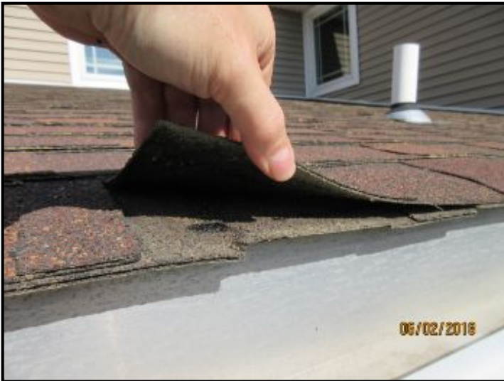
Two layers of asphalt shingles noted at lower roof.
