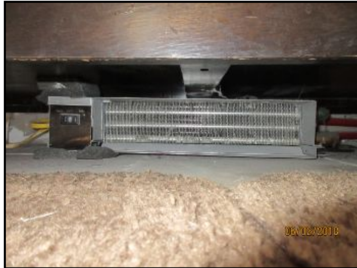
HVAC: Kick space heater noted
