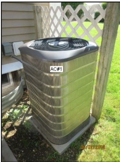
AC#1 Condenser: corresponding air handler located in crawlspace serves the 1st floor and basement.
