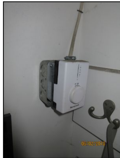
Unit Heater with thermostat noted in garage.
