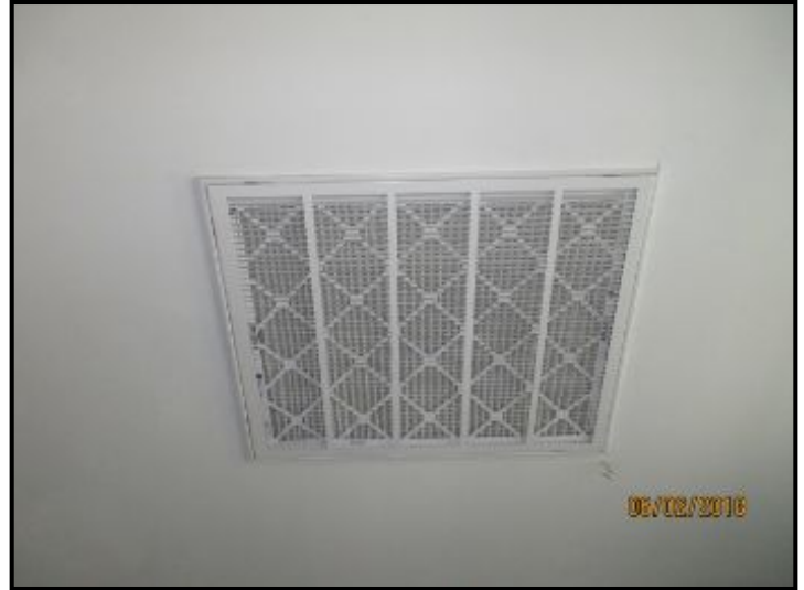
AC#2: Disposable filter located inside filter-grilles 2nd floor ceiling.
