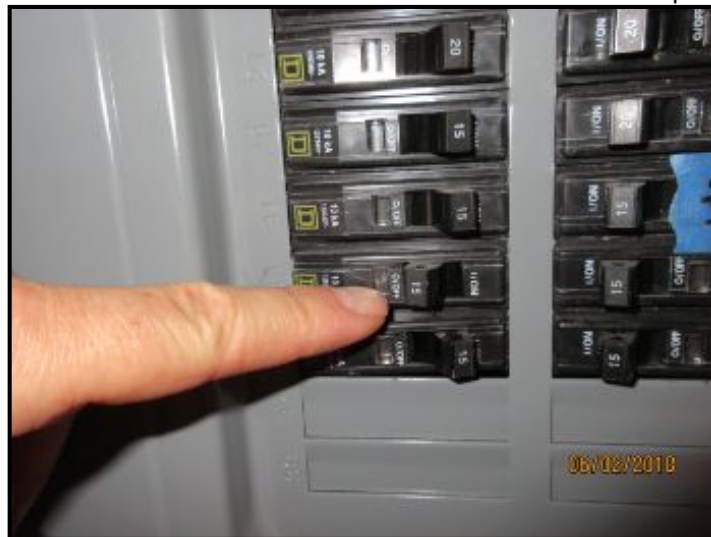
Main Panel: 1 - breaker in OFF position
