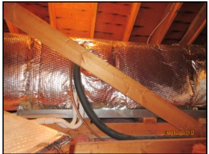
AC#@ Air handler located in attic operated via thermostat.
