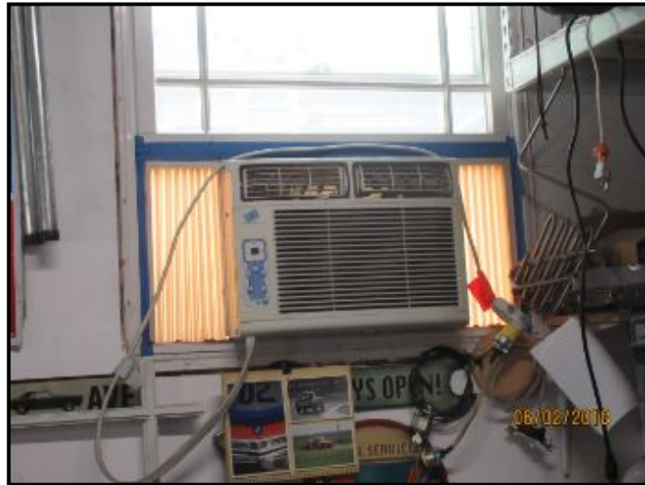
Window A/C unit not tested (exclusion).
