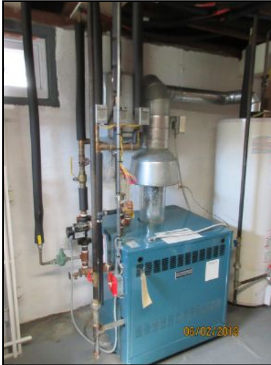
Burnham Gas-fired Forced Hot Water Boiler.
