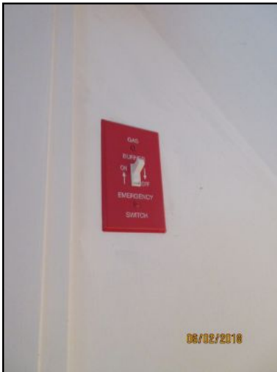
Remote Emergency Shut-off switch noted.
