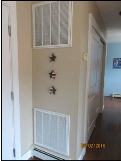
AC#1: Disposable filters located inside two filter-grilles at 1st floor hall wall.
