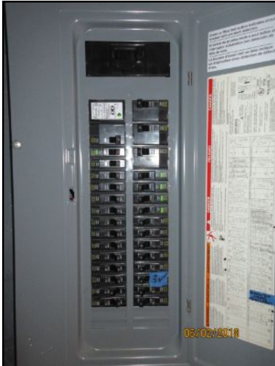
Main Panel (40 spaces): 4 - Spare circuit breaker space(s) noted.
