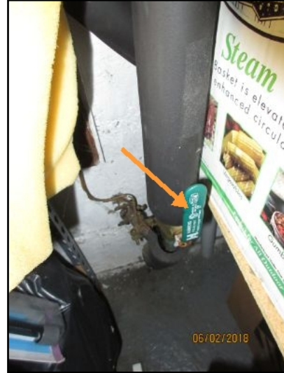
Main shutoff: Ball valve
