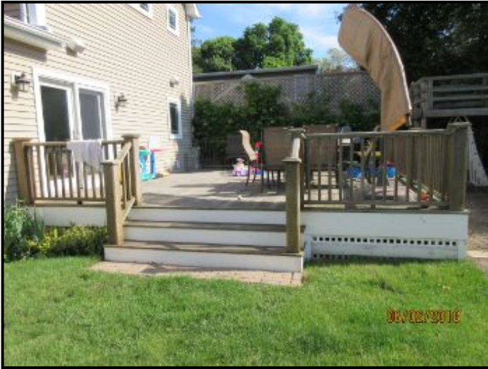
Recommend seller provide C.O. for the deck addition.
