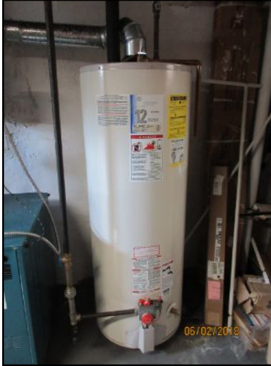
Water heater located in the basement. Gas, direct-fired water heater.
