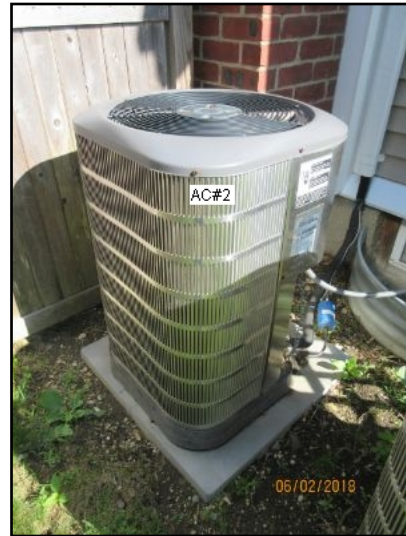
AC#2 Condenser: corresponding air handler located in attic serves the 2nd floor.
