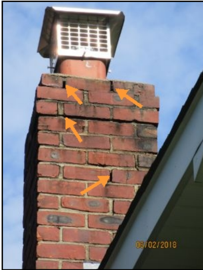
Chimney mortar joints show signs of deterioration. Recommend a mason to renew mortar joints; repointing as required to prevent further degradation.
