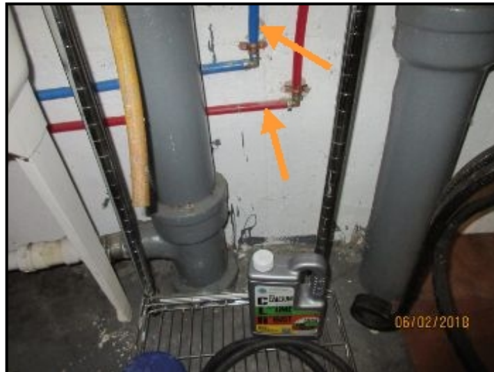
Supply Pipe Materials observed included PEX (cross-linked polyethylene) plastic tubing.
