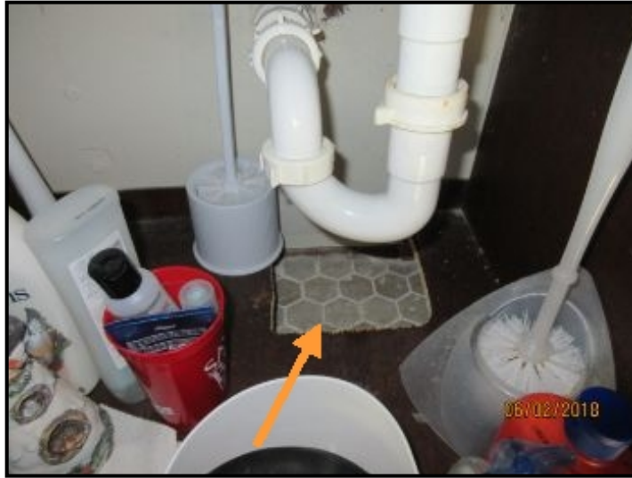
Vanity cabinet floor was cut out.
