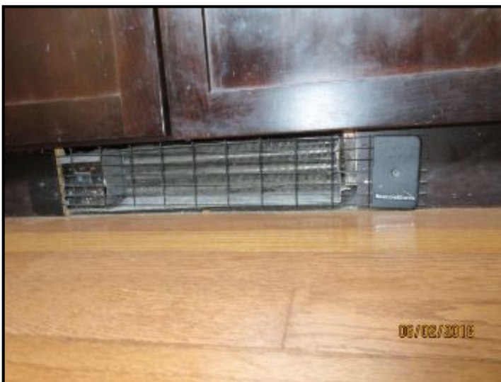
Kick space heater noted.
