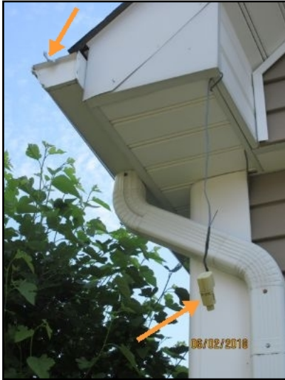
Sprinkler system rain sensor detached from gutter mount.
