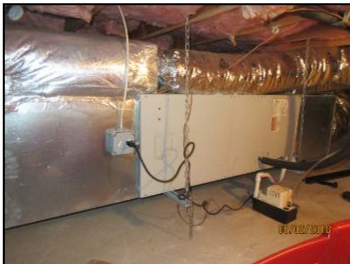
AC#1 Air handler located in crawlspace operating by means of the thermostat.
