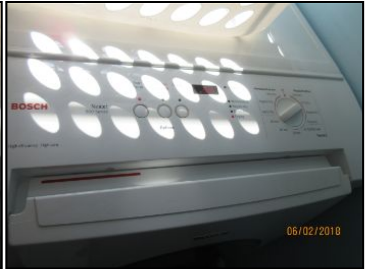
Gas dryer was operable. Estimated age of the Dryer is 1+ yrs.
