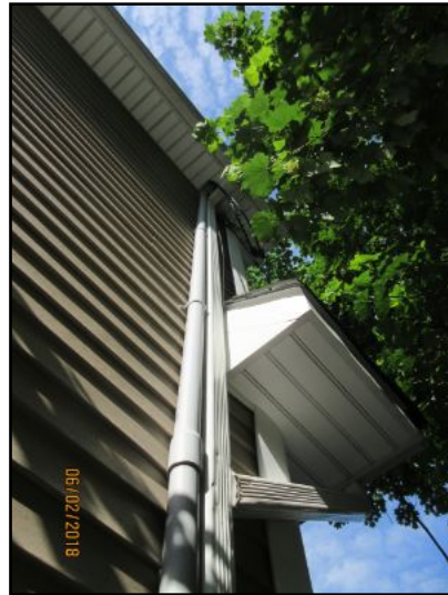
Tree branches in close proximity to electrical service drop cable, recommend trimming back tree branches.
