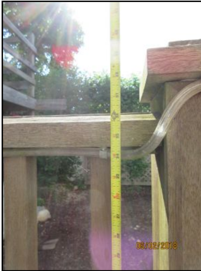
Guardrails meet the 36" min. height requirement.
