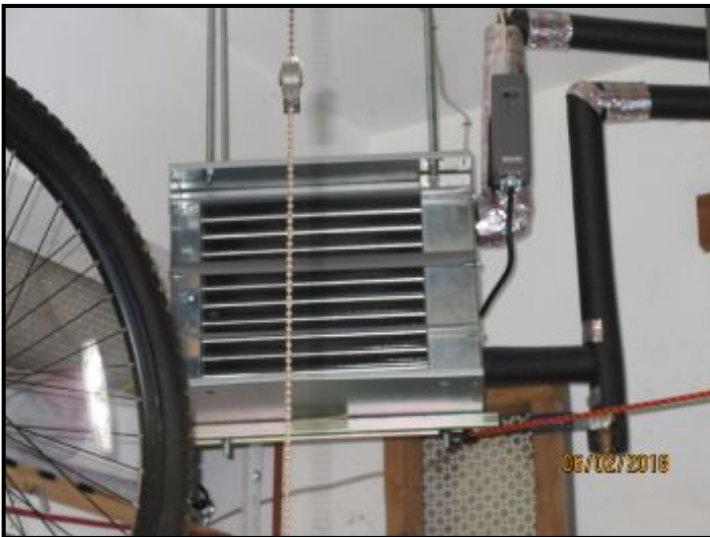
Unit Heater with thermostat noted in garage.
