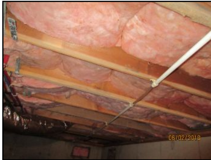
Unfinished fiberglass batts noted in joist cavities and perimeter joist bays.
