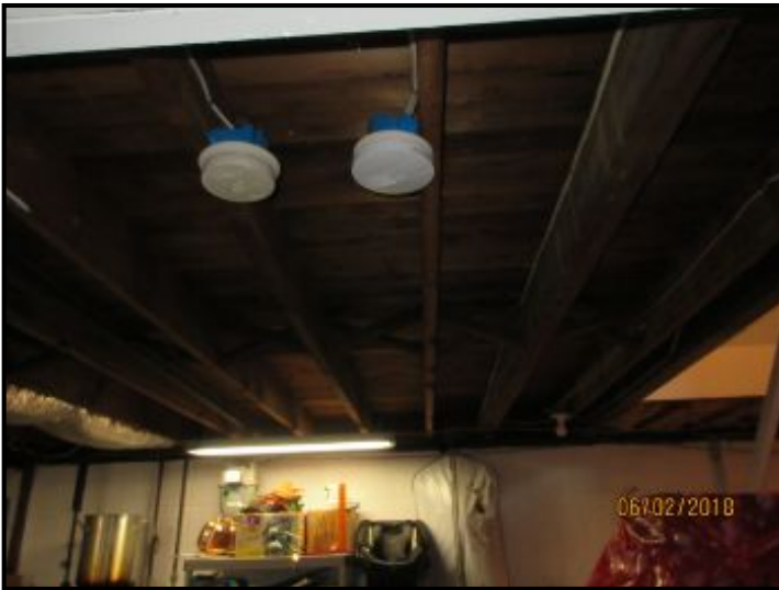
Smoke and CO detectors noted in basement.
