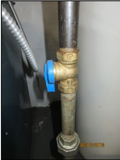
Gas supply shut-off valve noted at water heater
