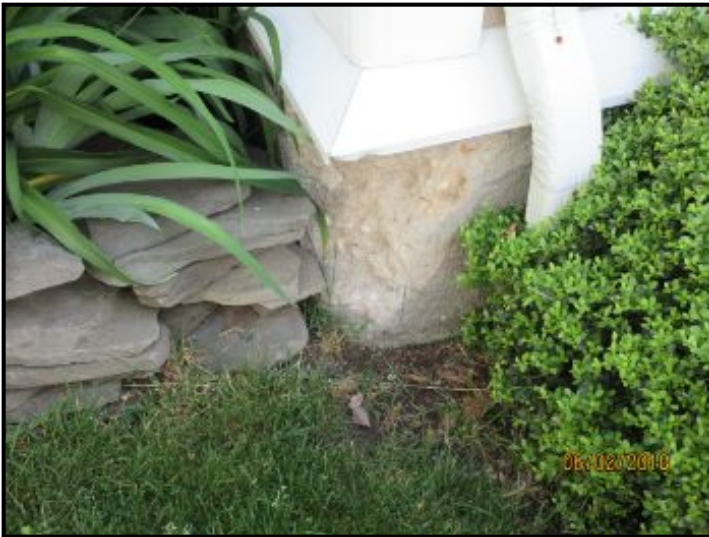
Cracked off piece of foundation front corner is cosmetic only.
