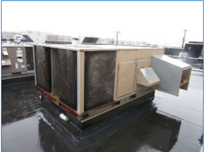
HVAC#1A mostly serves the front and larger portion of the suite.
