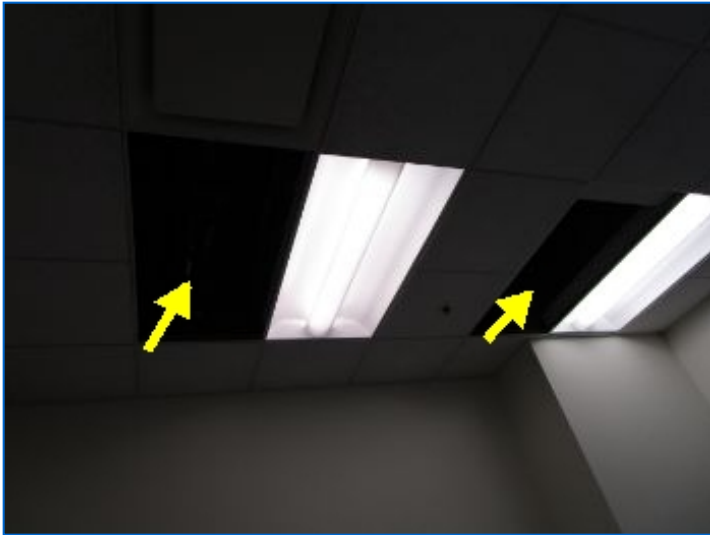
Ceiling tiles found removed.
