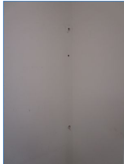
General cosmetic misc. repairs/finishes needed.
