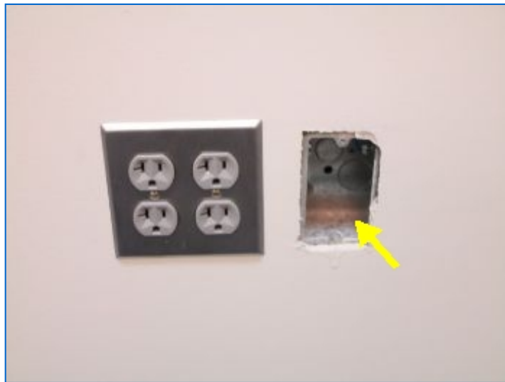
Unused electrical box noted.
