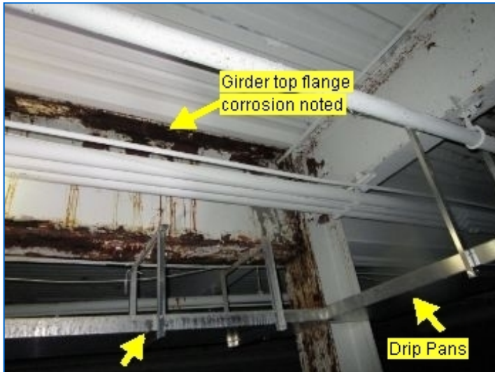
Steel girder corrosion at top flange noted. Drip pans used as a secondary band-aid repair.
