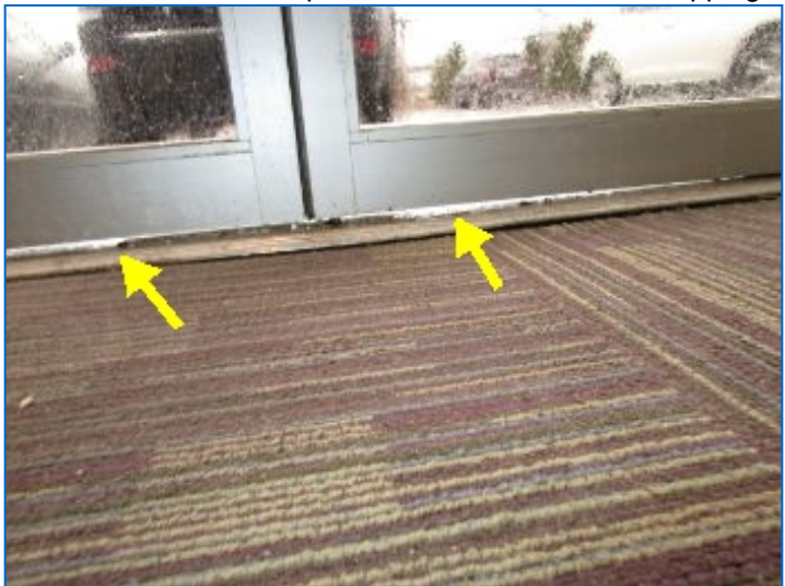
Aluminum storefront entrance was functional, with the exception of deteriorated weatherstripping observed along bottom of doors that allowed splashing raindrops to infiltrate beneath the doors. Replace deteriorated weatherstripping.
