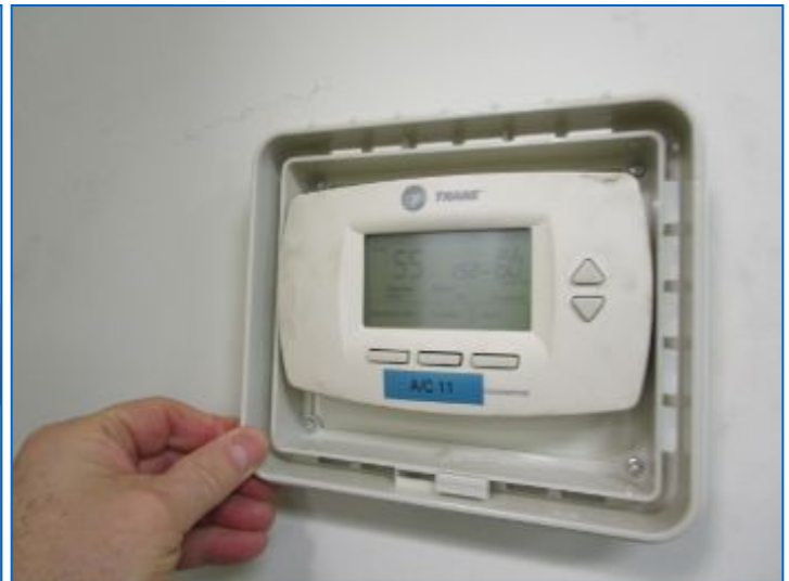
Security cover for Room #6 thermostat was missing.
