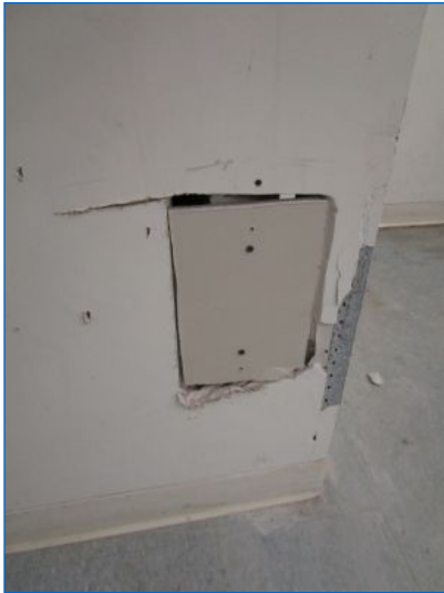
Shoddy and unfinished wall repair resulting from apparent installation of a roof drain riser pipe inside closet of the adjacent room.
