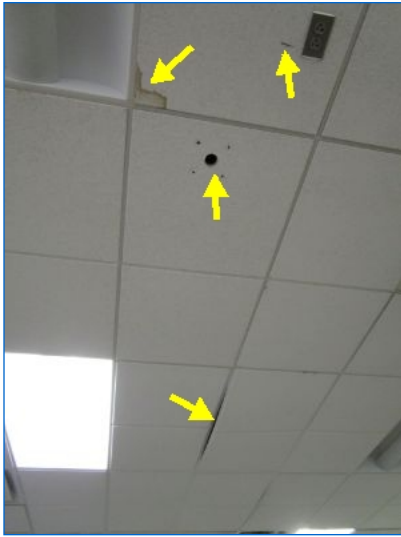
Some cosmetic stains and minor damages were observed at ceiling tiles in various places.
