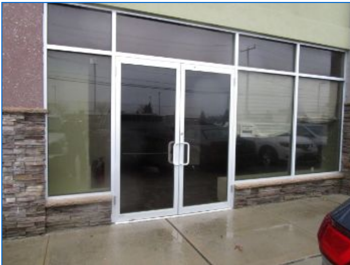
Aluminum storefront entrance was functional, with the exception of deteriorated weatherstripping observed along bottom of doors that allowed splashing raindrops to infiltrate beneath the doors. Replace deteriorated weatherstripping.
