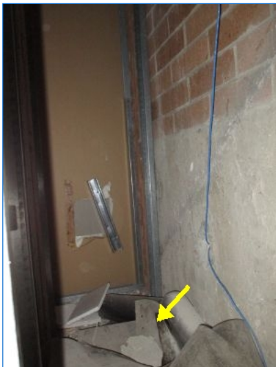
Construction debris noted inside wall cavity at northeast corner of the suite.
