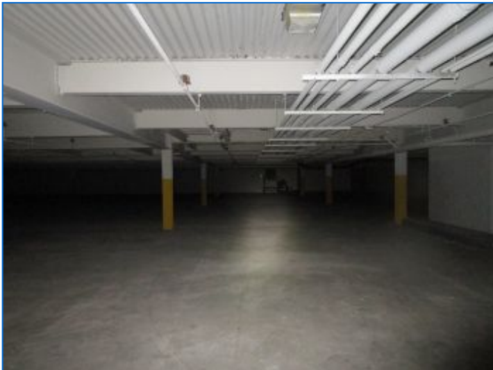
Structural conditions beneath the major portion of the office suite were satisfactory.
