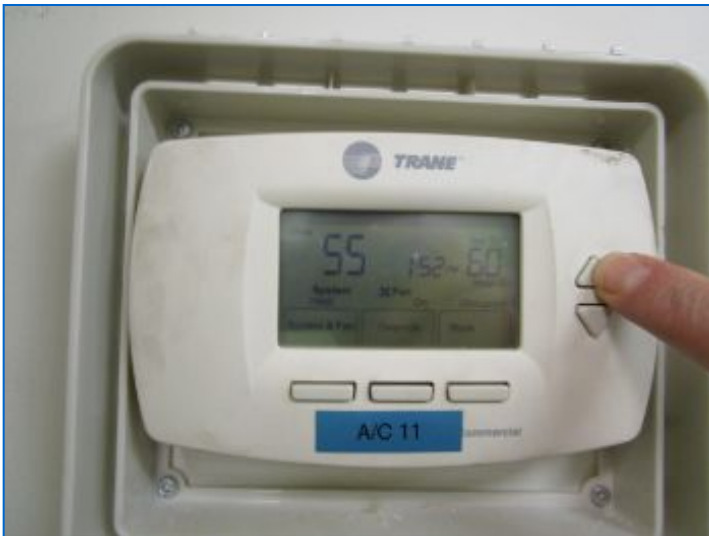
Digital Programmable type thermostat noted in Room #6; Heating & Cooling ; appeared functional. HVAC unit's fan ran but heating mode did not function due to gas being turned off.
