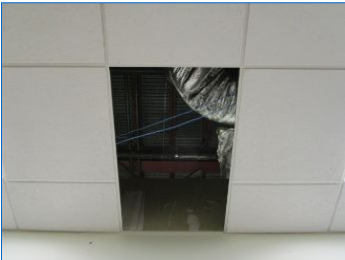
Ceiling tiles found removed.
