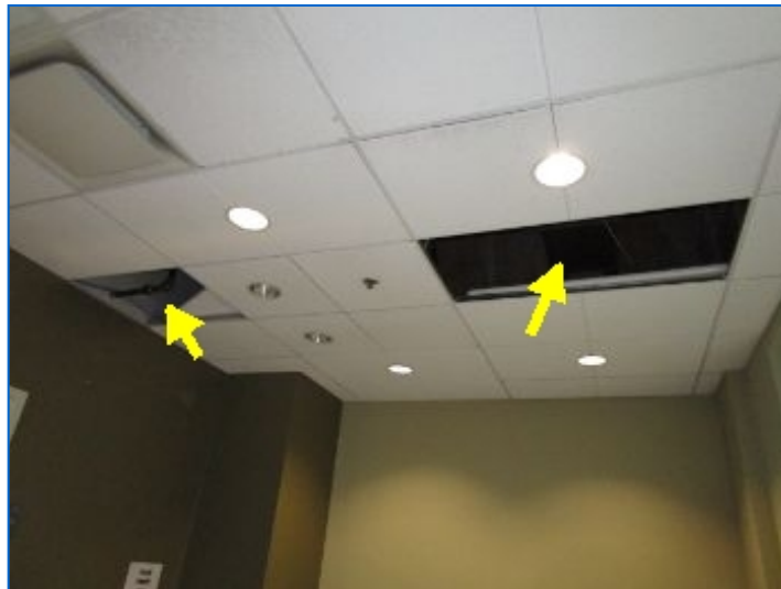
Ceiling tiles found removed.
