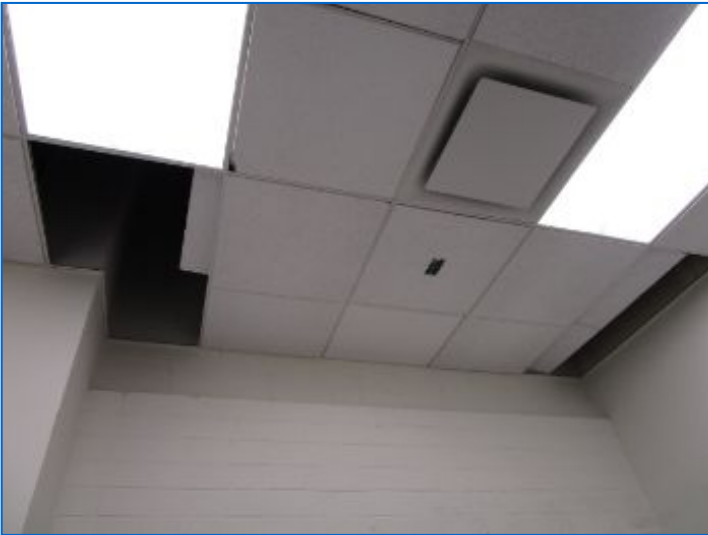
Ceiling tiles found removed.
