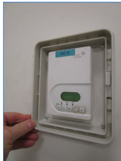
Security cover for Room #7 thermostat was missing.
