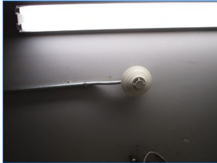
Electrical Closet: Maintain functioning Smoke and Carbon Monoxide detectors at required locations.
