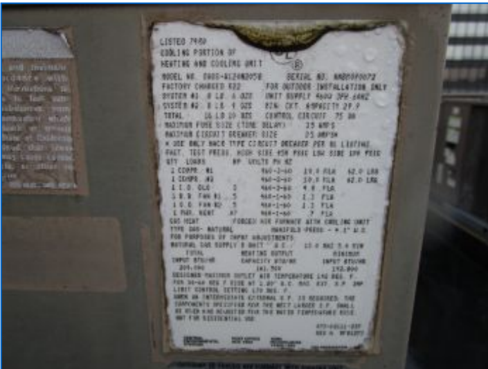
HVAC#1A York HVAC Unit data plate/serial no. indicates a Cooling capacity of 10 Tons, a Heating capacity of 161,500 Btu/hr, and a manufacture date of 8/1993, (26.3 yrs old). HVAC#1A has Exceeded its designed life expectancy. Anticipate replacing this HVAC equipment.
