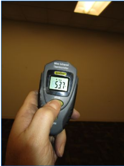
HVAC unit heating sections were not enabled due to gas valves being shut off.
