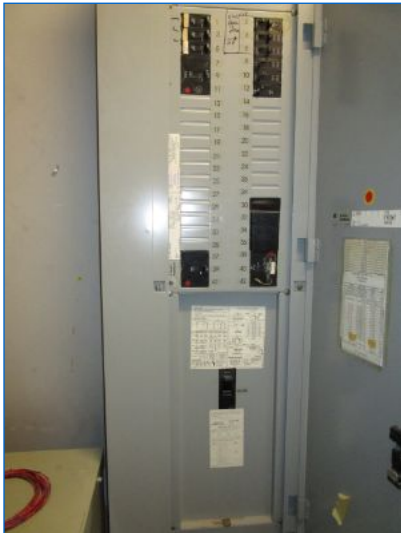
Main Panel# PP2: 42 circuit breaker spaces; 24 spare breaker spaces noted; 3 breakers were in the Off position.
