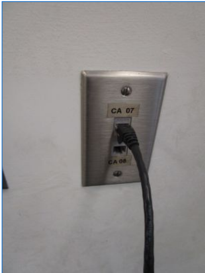
IT jacks noted in office spaces throughout.
