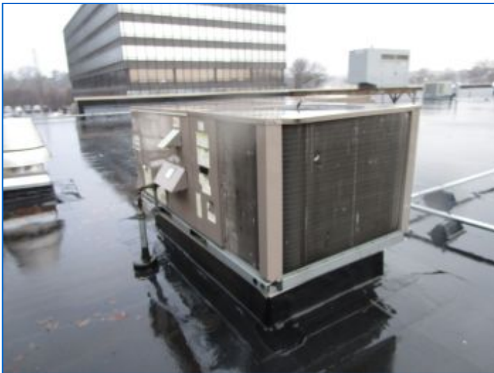
HVAC#1B mostly serves the rear and smaller portion of the suite.
