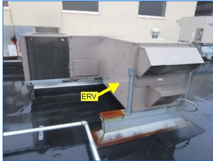
HVAC#1B Unit with Energy Recovery Ventilator (ERV) add-on.
