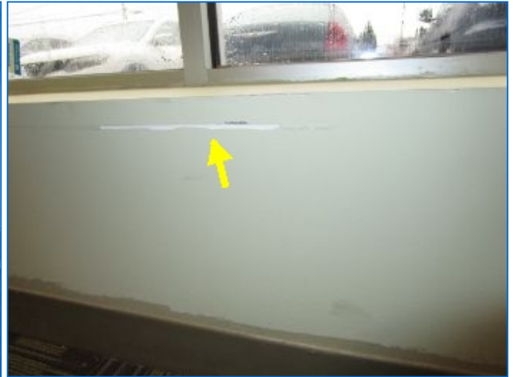
Cosmetic repair suggested for sill wall.
