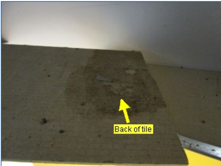
Water stains noted at ceiling tiles in Room #8; The areas were dry at the time of the inspection. Suggest cosmetic repairs and monitor for recurrence. Refer to Roof heading for related comment.
