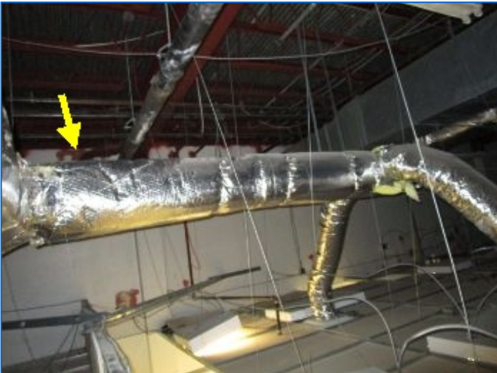
HVAC#1B Supply ductwork (looking south).
