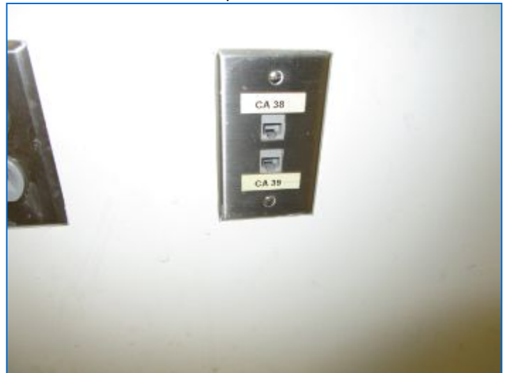
IT jacks noted in office spaces throughout.
