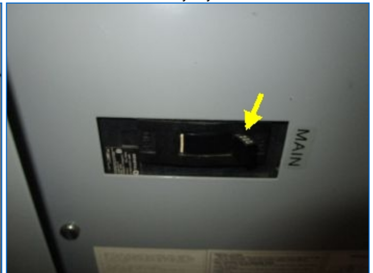
Main Panel# RP2 Disconnect: 200 amp main breaker serves the property.
