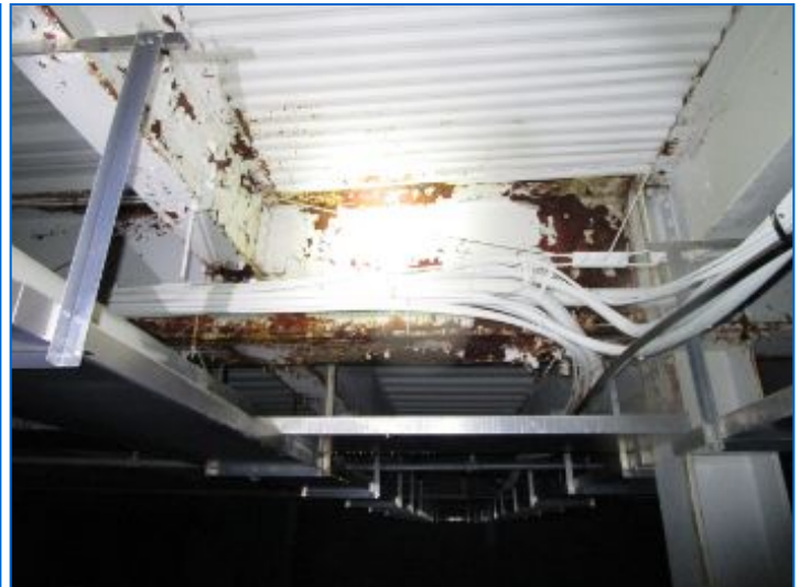
Steel girder corrosion at top flange noted. Drip pans used as a secondary band-aid repair.
