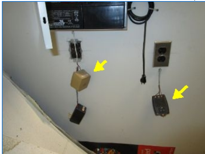
Smoke/Fire/Security panels deactivated in electrical closet. Confer with seller for installation/maintenance contractor information to ensure proper operation prior to close.
