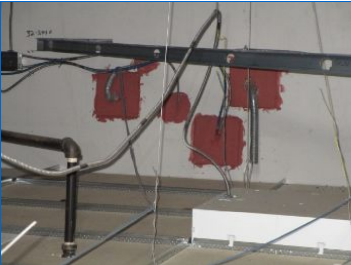
Repairs noted at fire barrier wall above hung ceiling separating the adjacent office suite.
