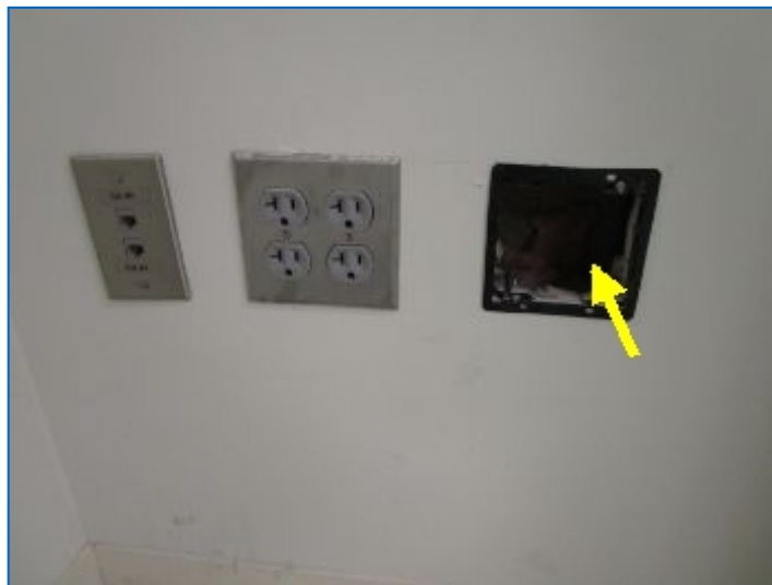
Opening in wall resulting from a damaged electrical box.
