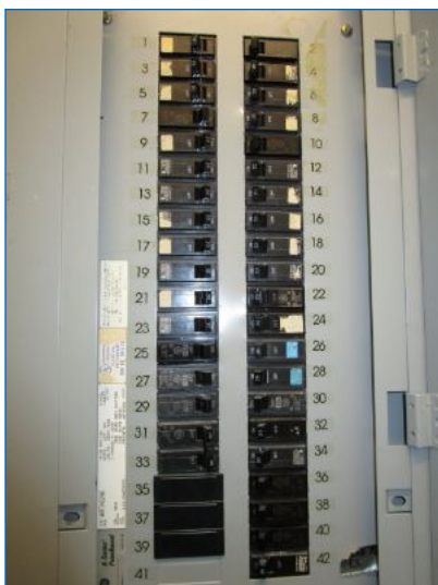
Main Panel# RP2: 42 circuit breaker spaces; 4 spare breaker spaces noted; 3 breakers were in the Off position.
