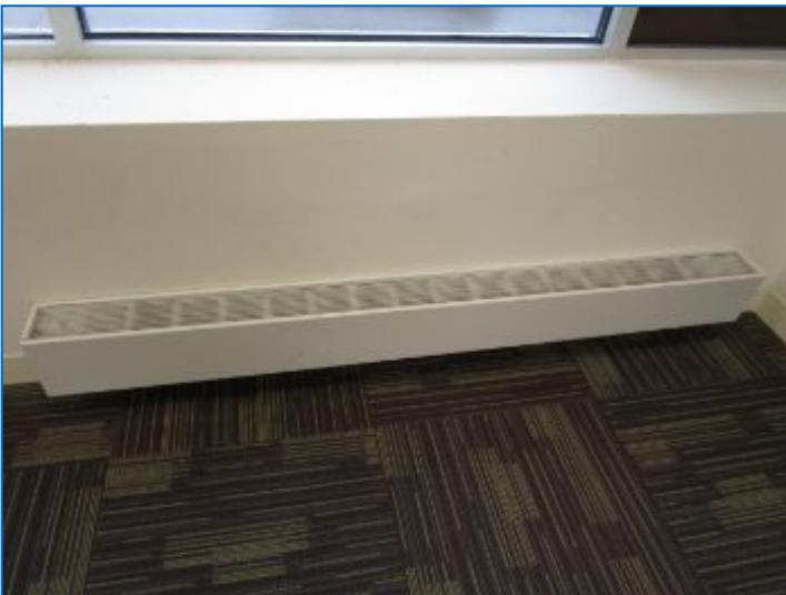
Electric Baseboard Heater located at front wall had no apparent on/off/temperature control switch and was apparently shut off at time of inspection. Refer to Electrical-Main Panel/s heading.
