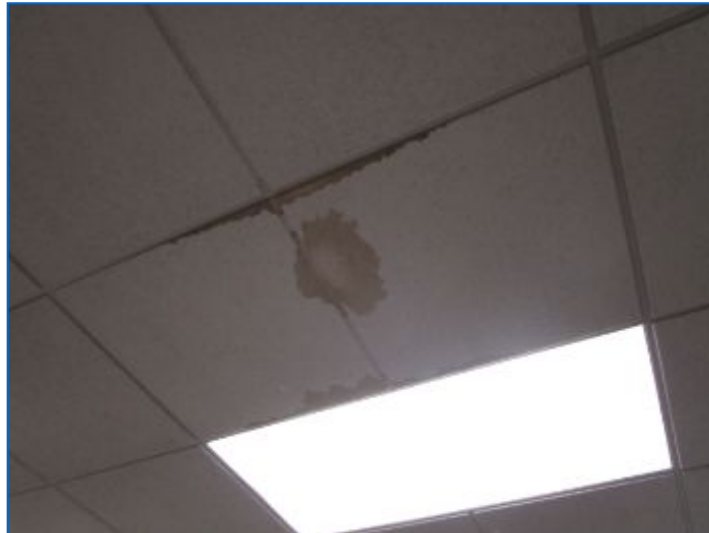
Moisture stains at ceiling tested dry at time of inspection; apparently from a past plumbing/sprinkler pipe leak that perhaps occurred during past construction activity. Replace damaged ceiling tiles and monitor.
