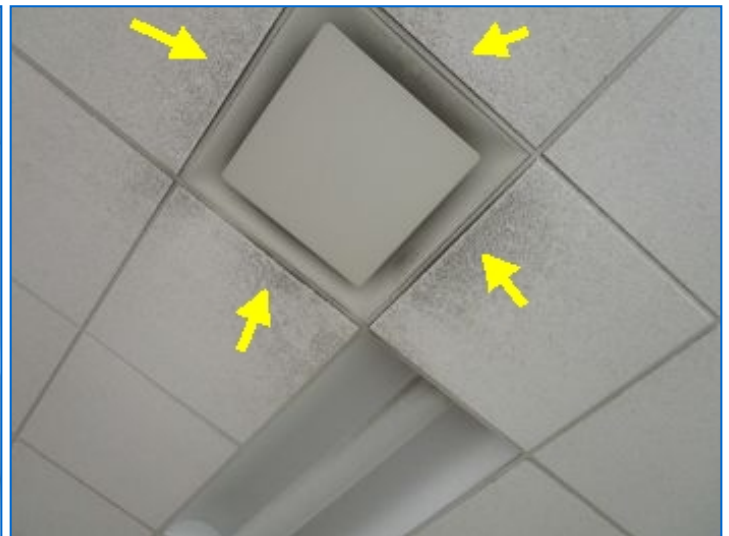
Cosmetic stains observed at ceiling tiles at HVAC outlet indicates a lack of HVAC unit maintenance.
