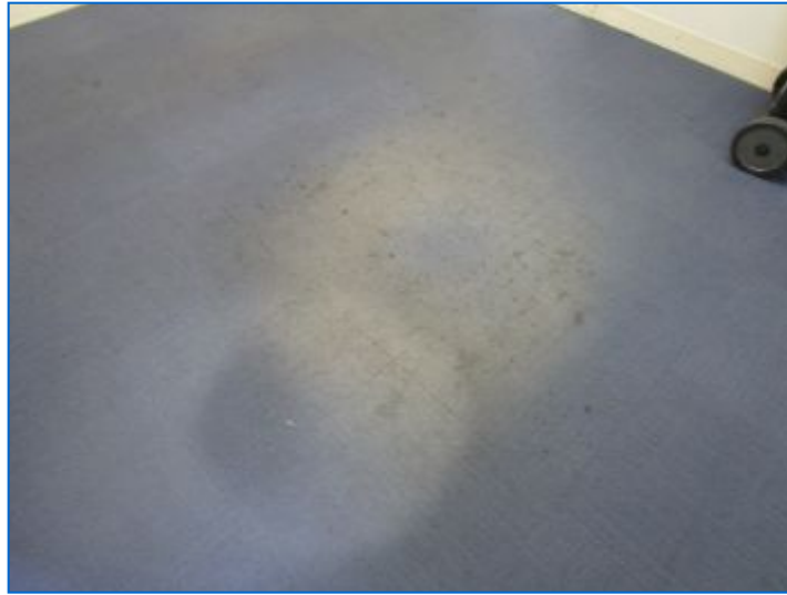
Cosmetic damage and wear at carpeted floor; typical throughout carpeted office areas.
