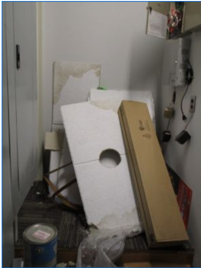
Construction debris noted in electrical closet.
