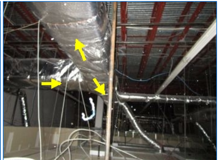
HVAC#1A Supply ductwork.
