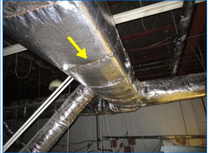
HVAC#1B Supply ductwork (looking south).
