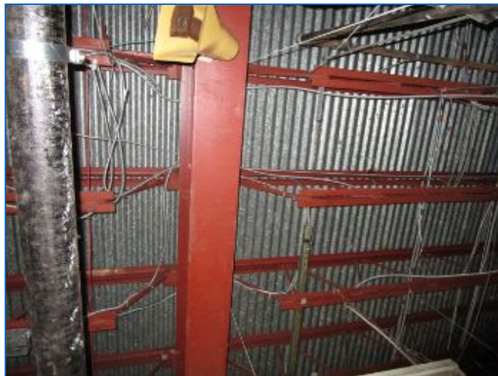
Steel columns, girders, bar joists supporting steel Q deck with poured concrete floor slab above i.e., 2nd floor above.
