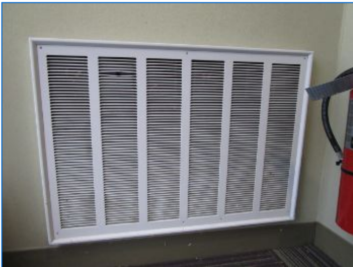
Electric Unit Heater located at wall in entryway had no apparent on/off/temperature control switch and was apparently shut off at time of inspection. Refer to Electrical-Main Panel/s heading.
