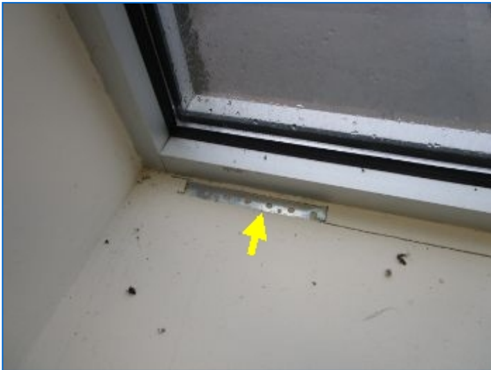
General cosmetic misc. repairs/finishes needed.
