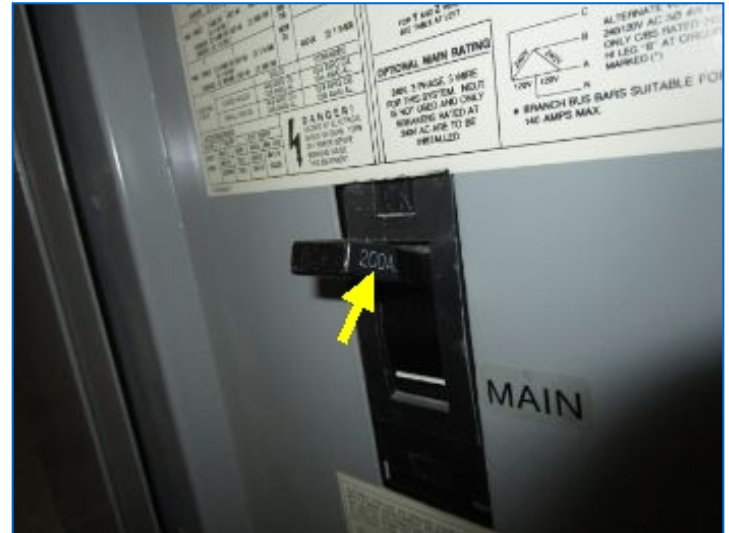
Main Panel# PP2 Disconnect: 200 amp main breaker serves the property.
