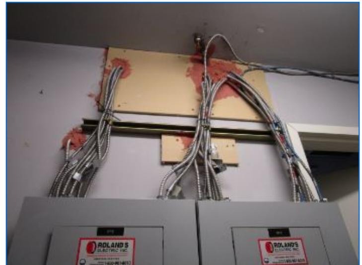
Distribution wiring observed consisted of copper, metallic armored cable.
