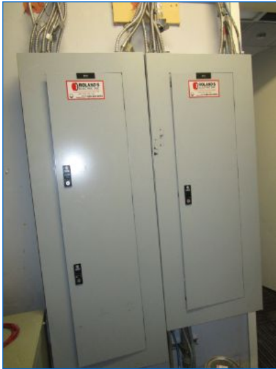
Two (2) Main Electric Panels located in Electrical Closet at front.
