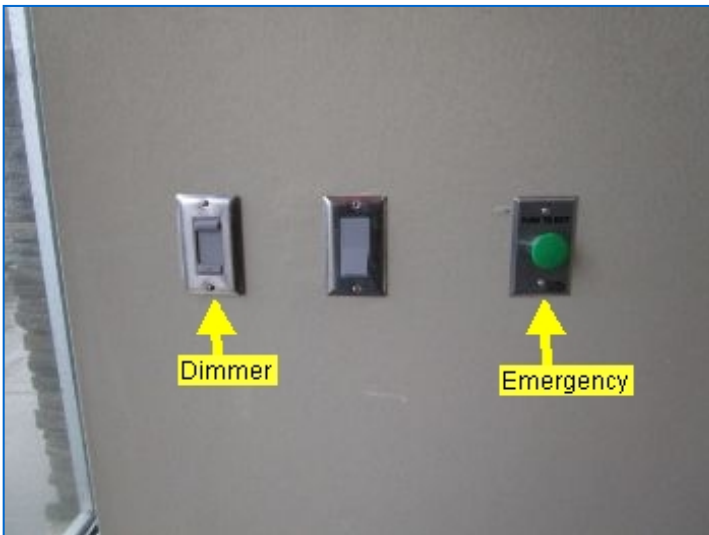
Dimmer switch and emergency door release button perhaps showed no apparent purpose at time of inspection. Confer with seller for functionality.
