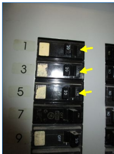
Main Panel# RP2 breakers labeled "#1 Conv. Rec", "#3 Microwave" and "#5 Microwave" were in the Off position. The Inspector was unable to detect the locations of these Off circuits within the rooms.
