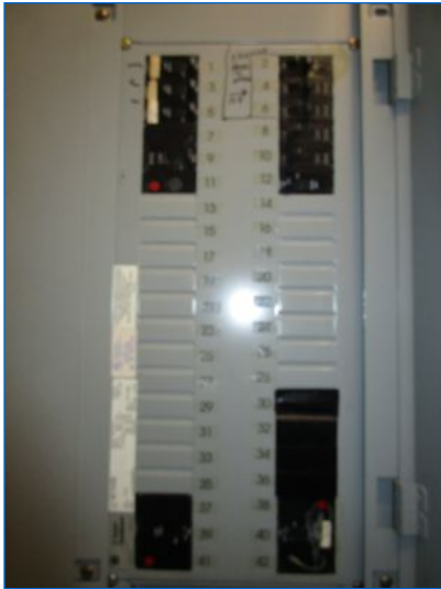
Main Panel# PP2: 42 circuit breaker spaces; 24 spare breaker spaces noted; 3 breakers were in the Off position.
