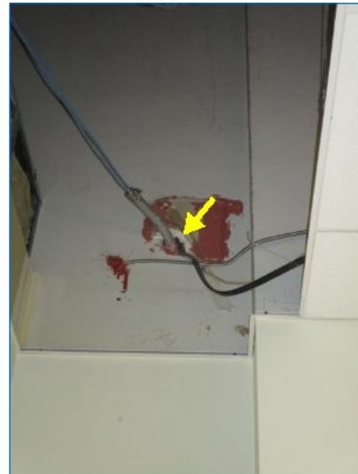
Inadequate fire-stopping noted at some penetrations through fire-rated barriers at suite border walls.
