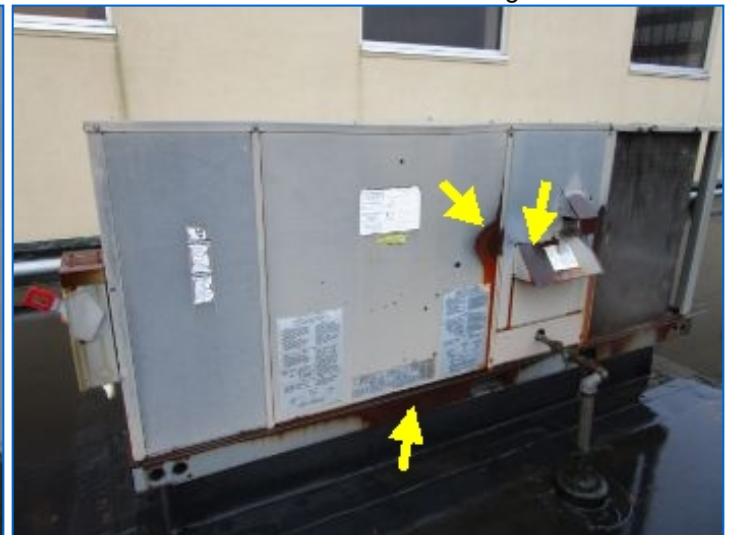
HVAC#1A is the older unit; showed signs of rust at cabinet and frame.
