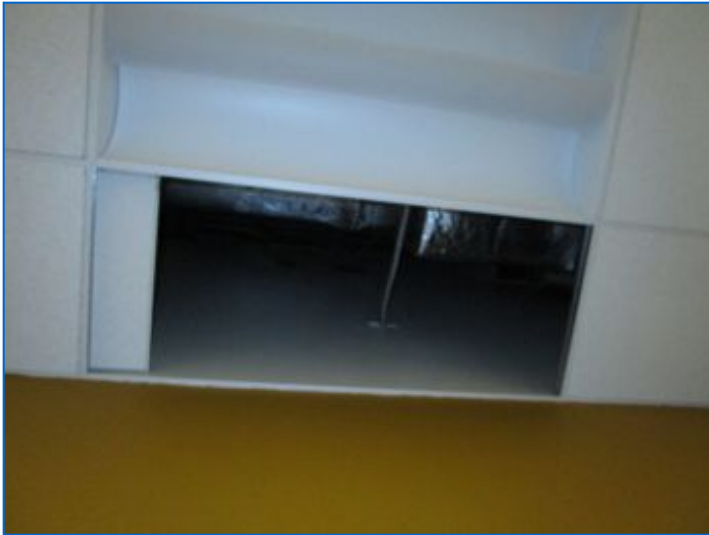
Ceiling tile found removed.
