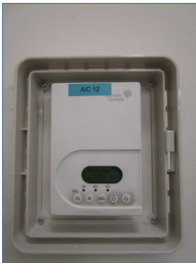
Digital Programmable type thermostat noted in Room #7; Heating & Cooling ; appeared functional. HVAC unit's fan ran but heating mode did not function due to gas being turned off.
