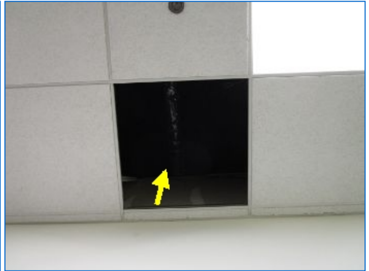
Ceiling tiles found removed.
