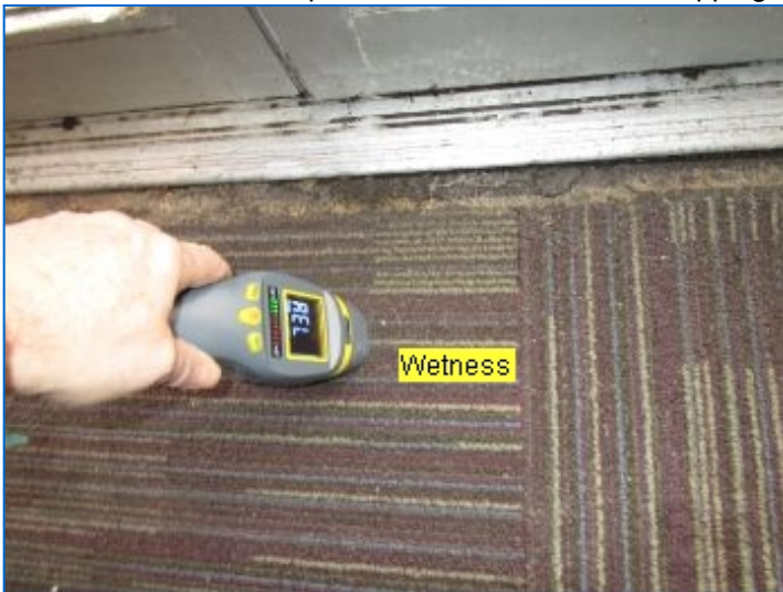
Aluminum storefront entrance was functional, with the exception of deteriorated weatherstripping observed along bottom of doors that allowed splashing raindrops to infiltrate beneath the doors. Replace deteriorated weatherstripping.
