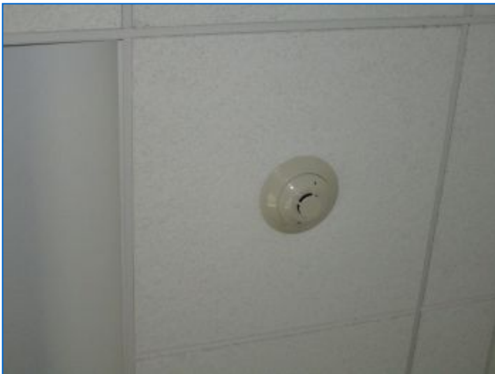
LIFE SAFETY: Maintain functioning Smoke and Carbon Monoxide detectors at the recommended locations.
