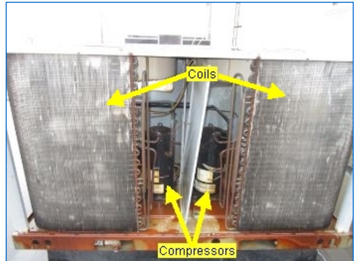
HVAC#1A: Access panel for compressor section was removed at time of inspection. Recommend inquiry as to what the status is of the cooling section of this unit; appears as if that ongoing access/service to the compressor section was needed. Condenser coil aluminum: some fins are bent and dirty; this will reduce performance and efficiency of the system. Recommend a qualified HVAC professional comb fins straight and clean coil to improve cooling system performance and efficiency. Refer to Service Recommendation heading.
