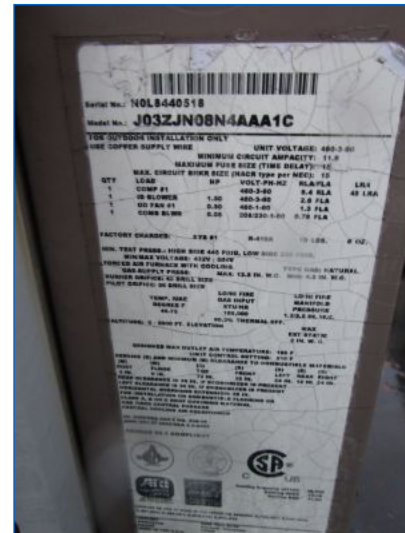
HVAC#1B Johnson Controls HVAC Unit data plate/serial no. indicates a Cooling capacity of 3 Tons, a Heating capacity of 100,000 Btu/hr, and a manufacture date of 10/2008, (10.2 yrs old).
