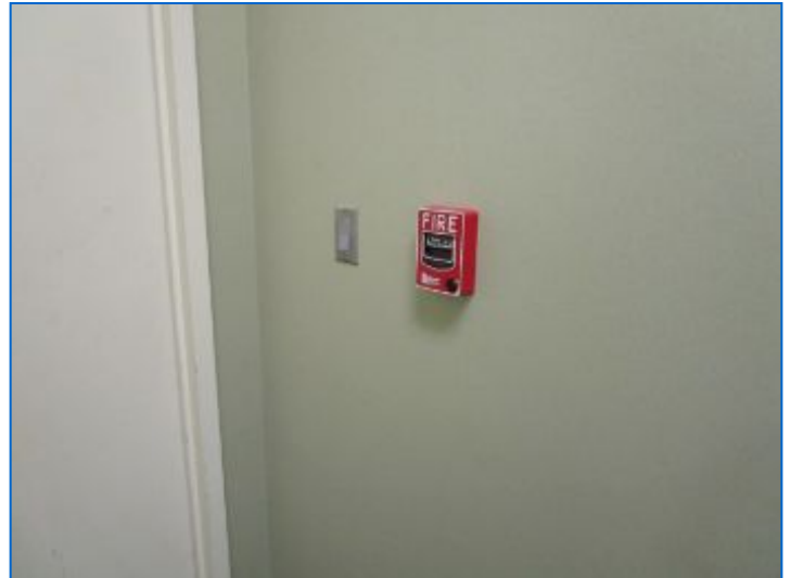
Fire alarm pull station noted.
