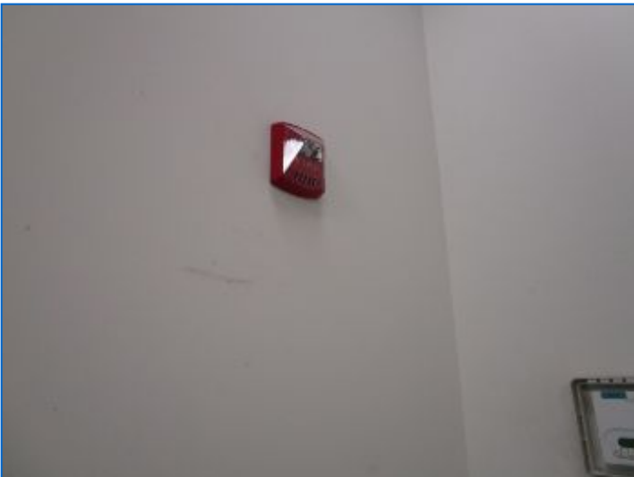
Fire alarm pull station noted.
