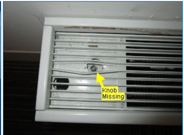
Electric Baseboard Heater located at front wall had no apparent on/off/temperature control switch and was apparently shut off at time of inspection. Refer to Electrical-Main Panel/s heading.
