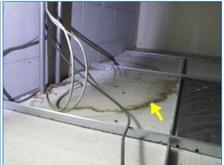
Water stains noted at ceiling tiles in Room #8; The areas were dry at the time of the inspection. Suggest cosmetic repairs and monitor for recurrence. Refer to Roof heading for related comment.
