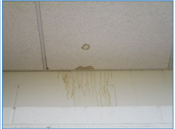
Water stains noted at ceiling tiles in Room #8; The areas were dry at the time of the inspection. Suggest cosmetic repairs and monitor for recurrence. Refer to Roof heading for related comment.
