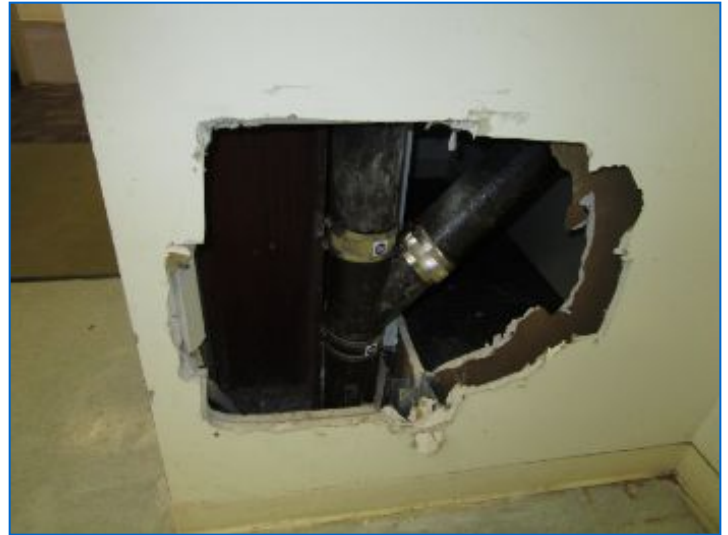
Wall repairs needed resulting from apparent installation of a roof drain riser pipe inside closet of the adjacent room.
