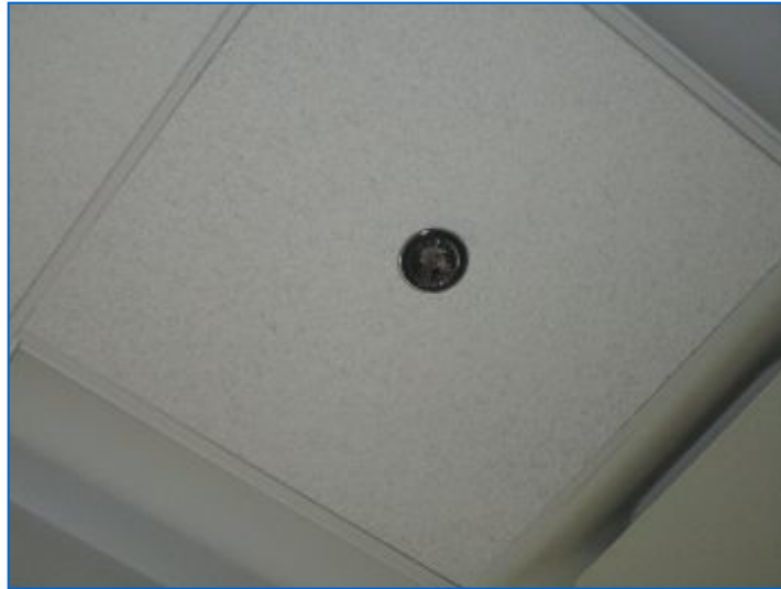
The office sweet is sprinklered.
