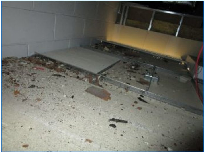
Some construction debris noted above ceiling tiles.
