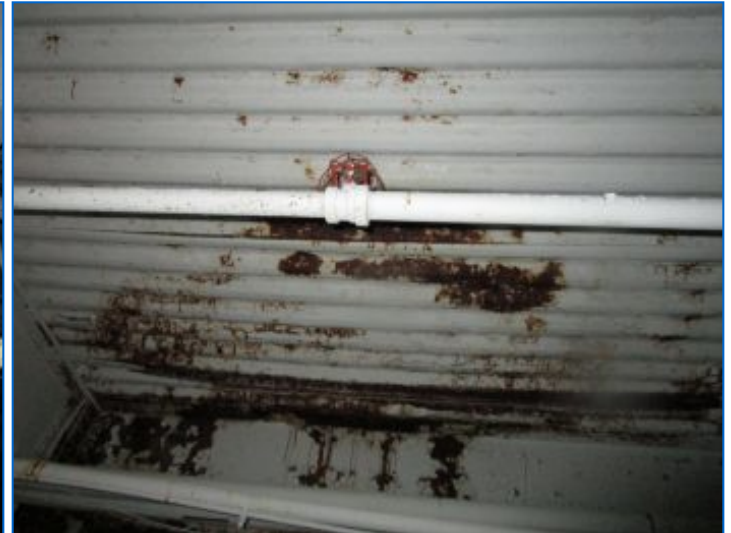
Water penetrating expansion joints in the concrete sidewalk and cracks in the asphalt parking area have penetrated the structural concrete base causing leaks and corrosion observed at few locations in the steel Q decking at the parking garage roof structure below the sidewalk/parking areas. This leaking and corrosion of the steel Q decking should be mitigated as soon as possible to prevent continued structural deterioration. Refer to related comments.
