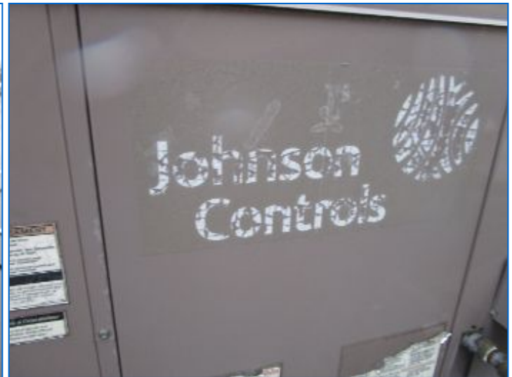
HVAC#1B: Johnson Controls HVAC Unit.
