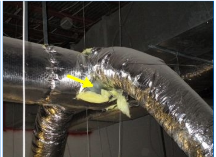
Insulation detached from HVAC#1B supply ductwork; recommend repairing insulation.
