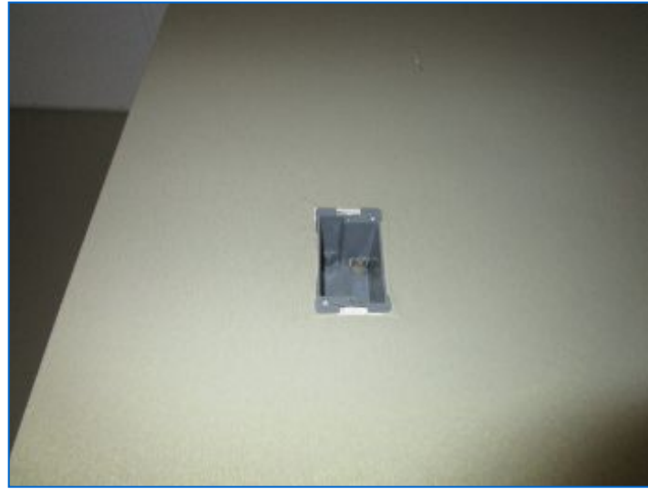
Unused electrical/cable box noted at wall in entryway.
