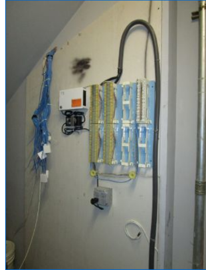
IT cables and telecom terminals noted in electrical closet.
