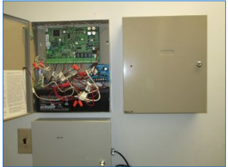
Smoke/Fire/Security panels noted in electrical closet. Confer with seller for installation/maintenance contractor information to ensure proper operation prior to close.
