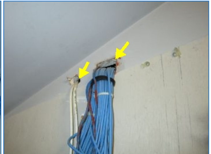
Inadequate fire-stopping noted at some penetrations through fire-rated barriers at suite border walls.
