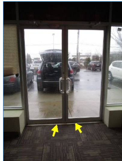
Aluminum storefront entrance was functional, with the exception of deteriorated weatherstripping observed along bottom of doors that allowed splashing raindrops to infiltrate beneath the doors. Replace deteriorated weatherstripping.
