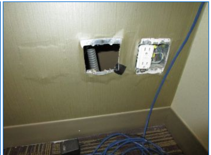
Entryway/Recep: Cosmetic damages at wall and electrical box cover missing. Repairs are recommended to eliminate shock/electrocution hazard.
