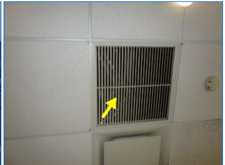
HVAC return grille to ceiling plenum noted.
