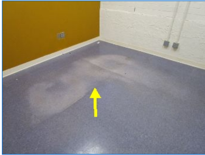
Worn VCT flooring.
