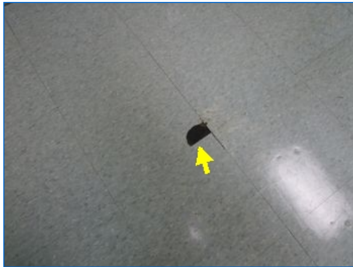
VCT flooring damage noted.
