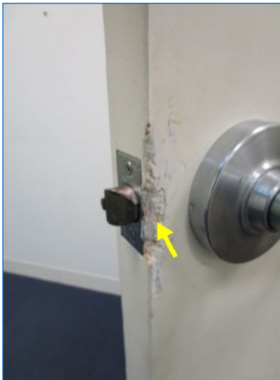
Cosmetic damage noted near door latch.
