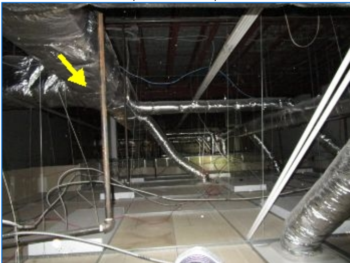
HVAC#1A Supply ductwork (looking towards the front).
