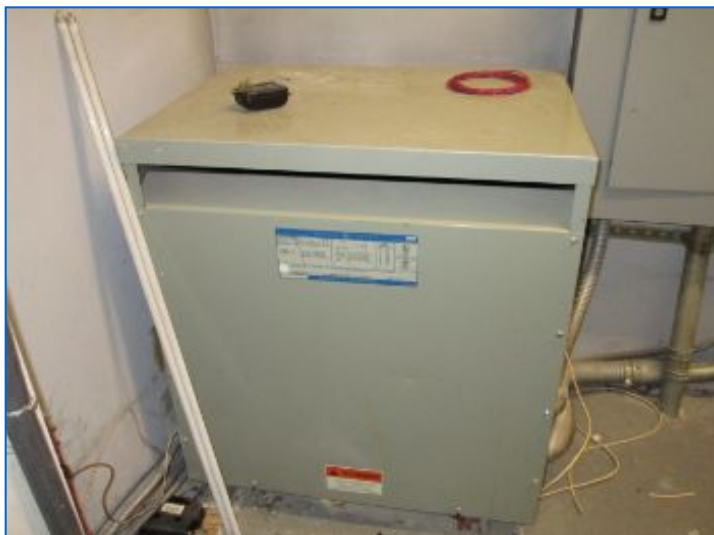
A 75 KVA Step-down transformer in the electric closet reduces the 480 volt power to 208/120 volt power as needed to serve the office suite.
