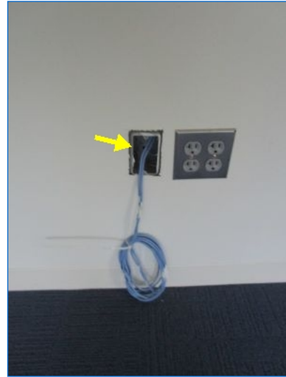
Uncovered IT cable box noted.
