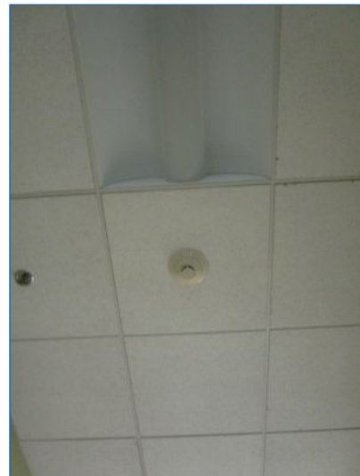
LIFE SAFETY: Maintain functioning Smoke and Carbon Monoxide detectors at the recommended locations.
