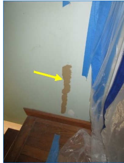
Drywall surface damage caused by masking tape. Recommend wall repairs.
