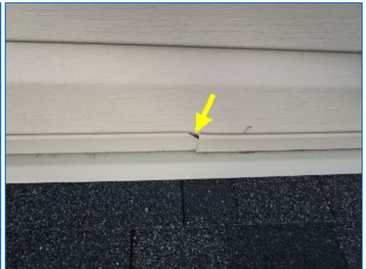
Some signs of sloppy trim work noted at rear dormer.
