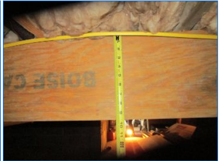
Main Floor Structure: Wood triple 2x10 main beams supported by steel posts in conc., 2x8 Joists 16" O.C. (w/cross braces), Plywood floor boards.
