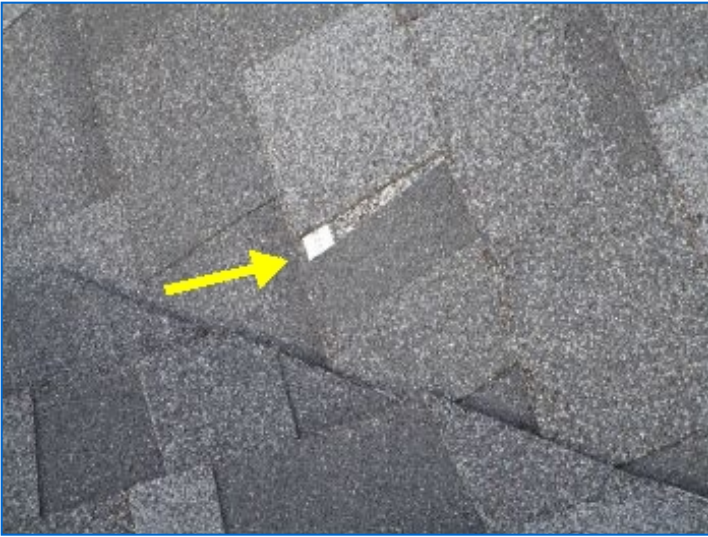
Signs of inferior workmanship by roofers.
