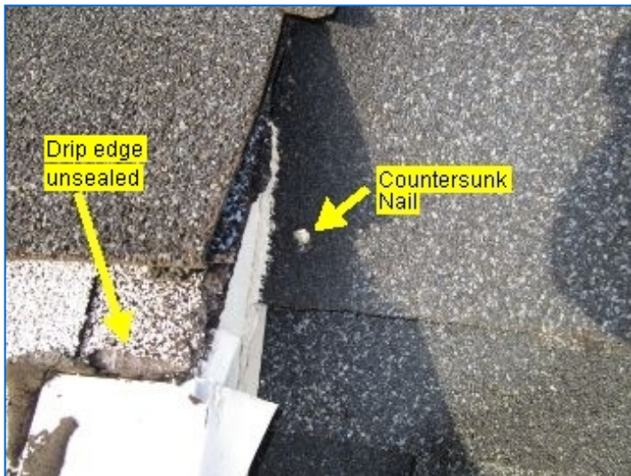
Signs of inferior workmanship by roofers. Conditions that can lead to water intrusion noted. The Inspector recommends review by a qualified roofing contractor to provide remedial improvements and warranty workmanship for the roof. Exposed and countersunk nail heads at roofing material. Recommend sealing all fastener heads.
