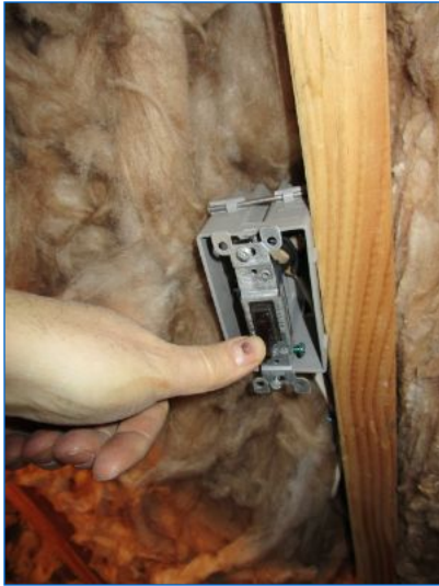
Proper lighting and GFCI type receptacles were not installed in the crawlspace. Recommend licensed electrician provide lighting and GFCI receptacle provisions.
