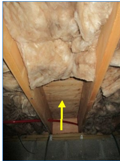
Batt insulation was observed to be hanging/missing at a few joist cavity locations. Recommend restoring missing/hanging insulation and securing in place using insulation support wires.
