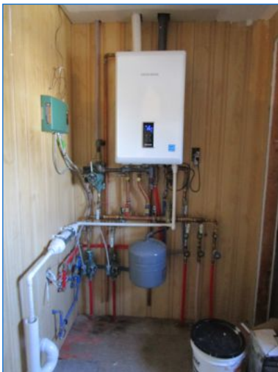
Heater Type: Gas-fired, Combination Tankless Boiler & Water Heater (CBWH); Manufactured by Navien.
