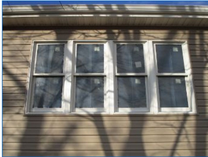
All window screens were missing. Contractor to provide.
