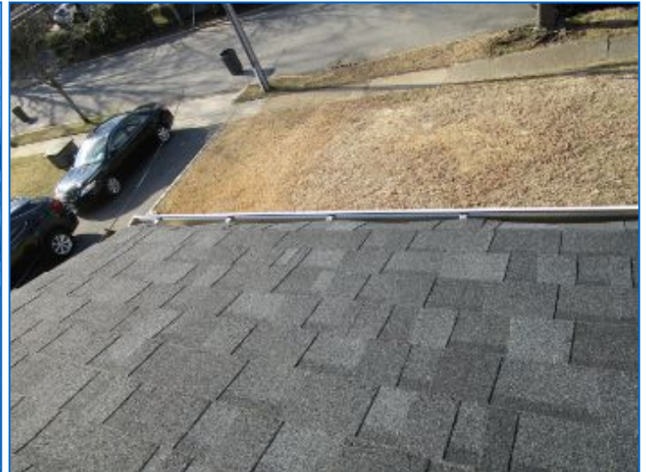
Shingles extended to far over gutter which may affect proper gutter drainage; recommend corrective action.
