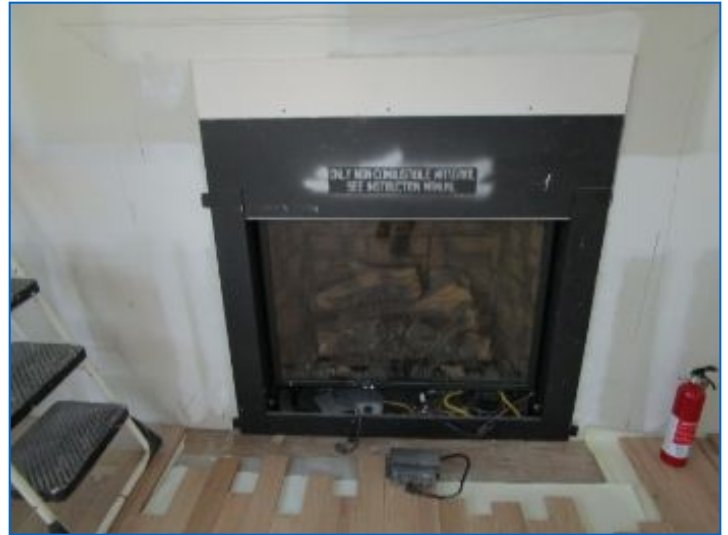
Gas fireplace surround/mantle, stone hearth and manufacturer approved startup of fireplace was yet to be completed.
