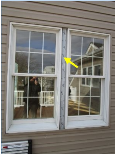
Missing trim noted at mullion.
