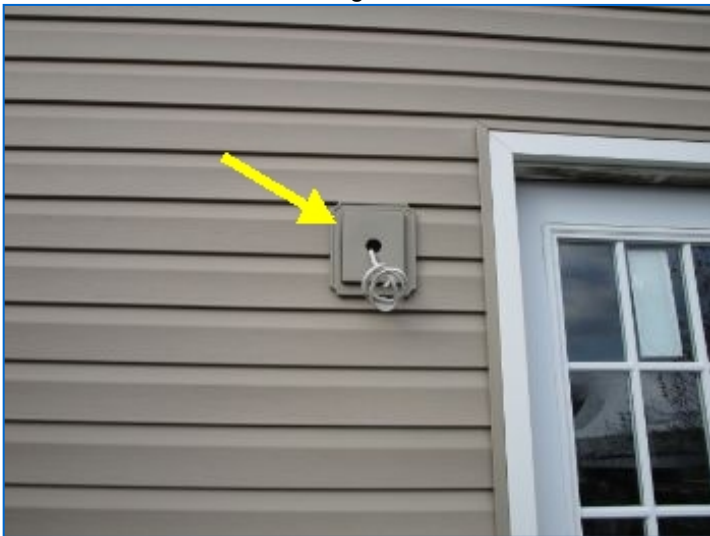
Exterior light fixture not installed at east facing wall leaving exposed wires that can potentially become energized.
