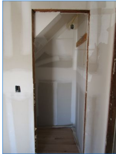
Doors, door/window hardware, baseboard, casings, sills, moldings/trim, transitions, receptacles, switches, lighting, baseboard enclosure parts, finishes, etc. were not yet installed.
