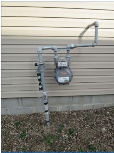
Gas service elevated pressure pipe was not vertical; possibly stressing the pipe. This is not typical of gas company installations. Recommend asking National grid to review installation and coordinate corrective action with contractor.
