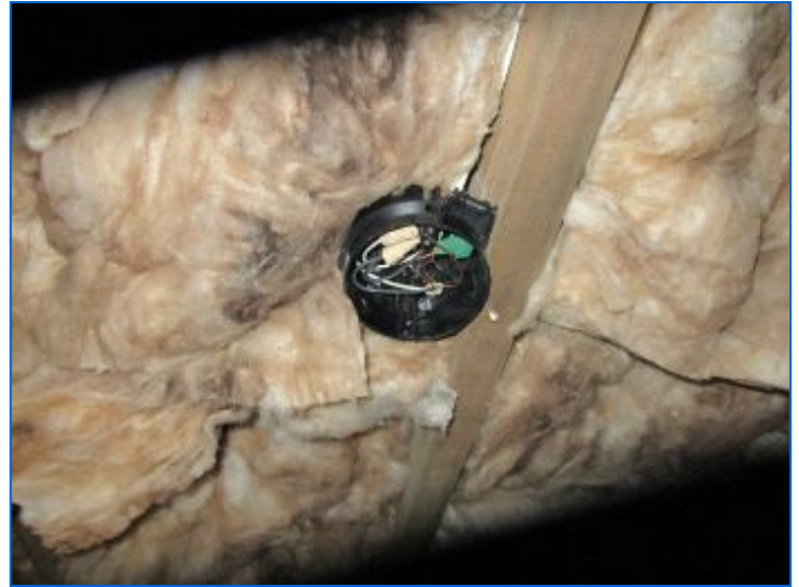
Open junction boxes were observed, which is a safety concern. Recommend installing proper covers, as needed for safety.
