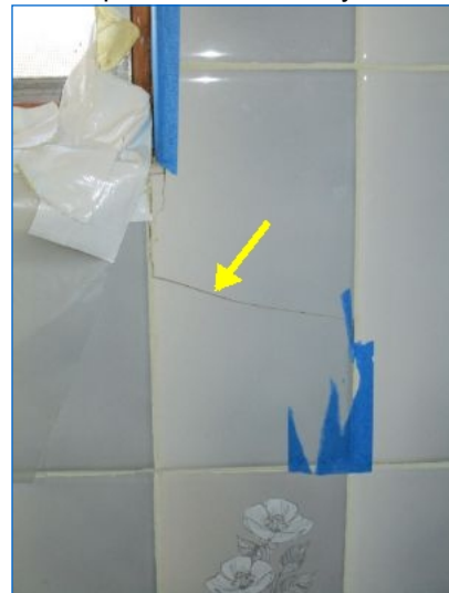
Cracked tile at outer wall noted to have been caused by the structure elevation. Tile and grout repairs recommended around window to prevent water entry.
