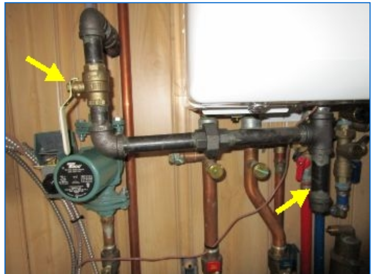
Gas shut-off valve and drip leg located at boiler.
