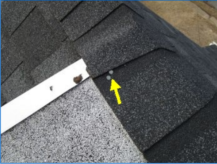
Exposed and countersunk nail heads at roofing material. Recommend sealing all fastener heads.
