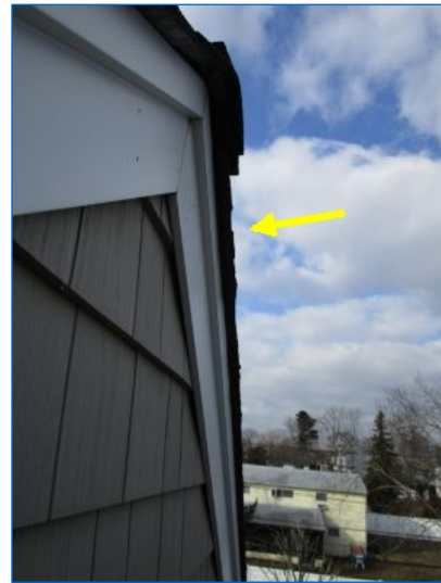
Signs of inferior workmanship by roofers. Jagged shingle cut/damaged edges. The Inspector recommends review by a qualified roofing contractor to provide remedial improvements and warranty workmanship for the roof.
