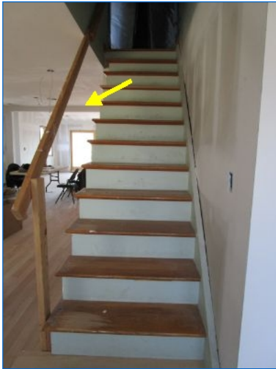
A compliant handrail was not installed.
