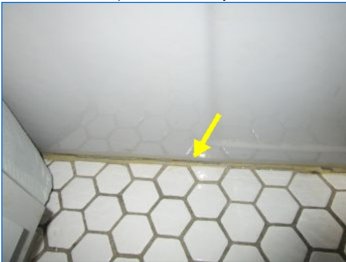
Cracked grout at floor-tub joint noted to have been caused by the structure elevation. Grout repairs recommended to prevent water entry.
