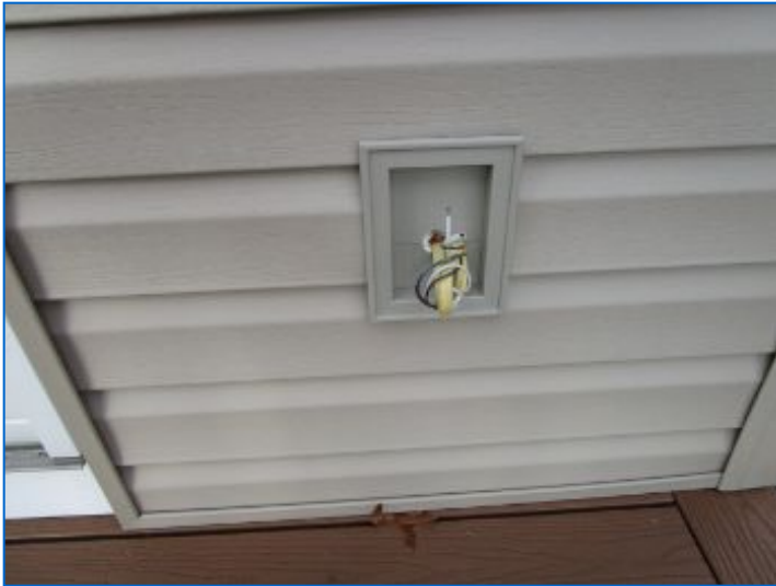
Exterior GFCI type receptacles were not installed at east side (2 places) leaving exposed wires that can potentially become energized.
