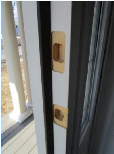
Front door hardware was missing.
