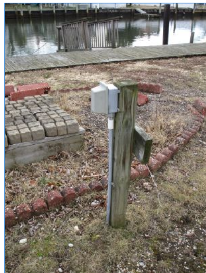
Underground electrical work was incomplete at east side and dock area.
