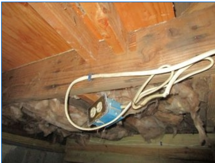
Proper GFCI type receptacles were not installed in the crawlspace. Recommend licensed electrician provide GFCI receptacle provisions.
