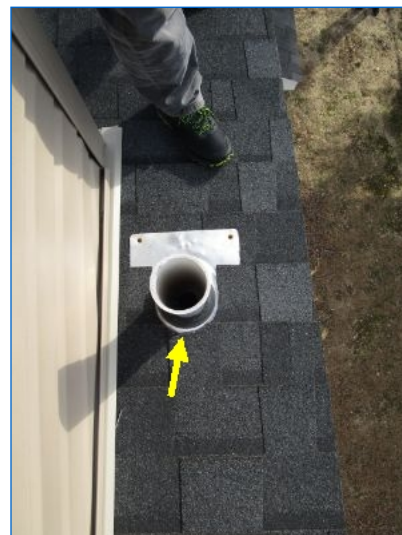
Due to the low-slope roof where plumbing vent penetrates roof the Inspector recommends sealing around shingle cut to ensure that no snow/ice/water intrusion occurs at this south side location.
