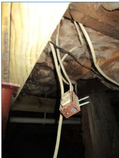
Hanging, uncovered receptacle box should be mounted to the structure and covered using a listed cover.
