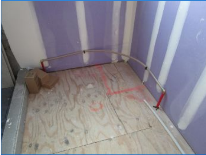
Floor tile, baseboard heat, door/window hardware, casings, sills, baseboard, moldings/trim, transitions, GFCI/receptacles, switches, lighting, exhaust fan, cabinets/counters, plumbing fixtures, accessories, grab bars, finishes, etc. were not installed.
