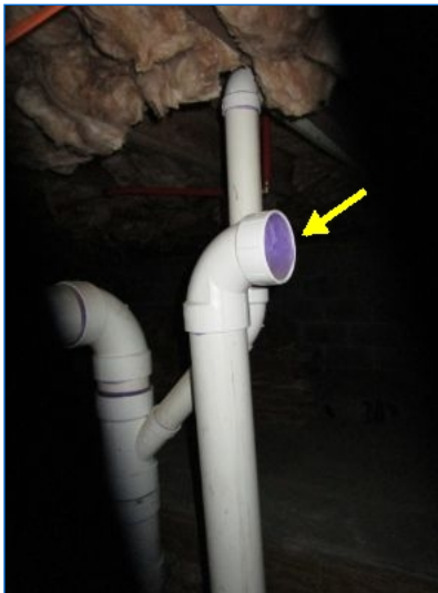
DWV pipe for proposed bathroom; unfinished plumbing work noted for the 1st floor (kitchen and bathroom).
