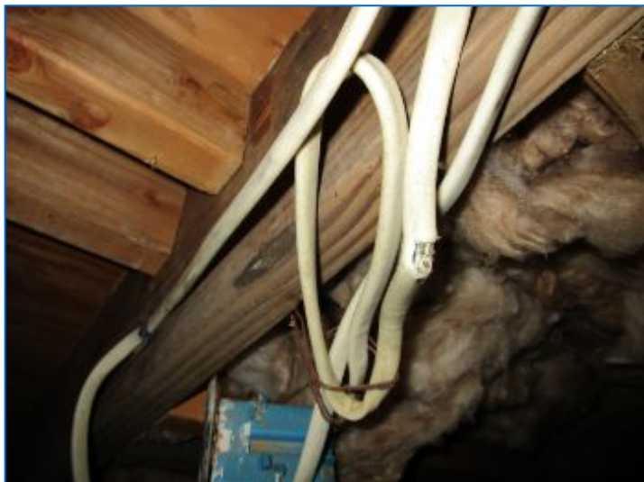
Damaged cable with potentially live electrical wires exposed to touch in the crawlspace; electric shock and short circuit hazard. Defective wires should be removed and replaced by a licensed electrician.
