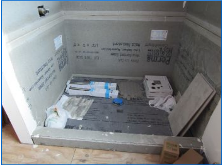
Shower tile work, plumbing/fixtures, wall accessories, grab bar, enclosure, lighting, finishes, etc. were not installed.
