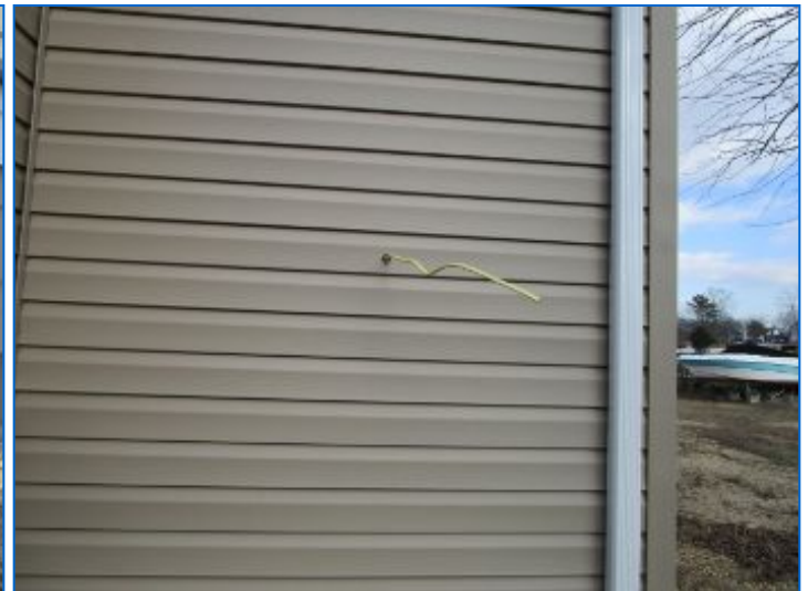
Exterior fixture/device not installed at south-facing wall leaving exposed wires.
