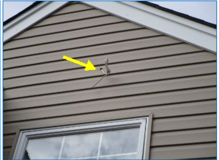
Exterior light fixture not installed at east facing wall leaving exposed wires that can potentially become energized.
