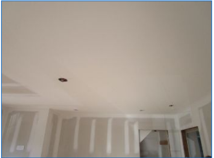
Doors, door/window hardware, baseboard, casings, sills, moldings/trim, transitions, receptacles, switches, lighting, baseboard enclosure parts, finishes, etc. were not yet installed.
