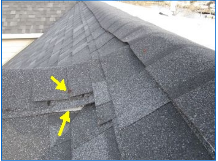
Some shingles damaged; improper nails used; undercut shingles; shoddy repairs noted Recommend proper repairs by a licensed qualified roofing contractor.
