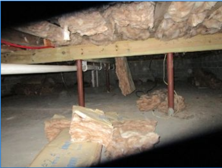
Main Floor Structure: Wood triple 2x10 main beams supported by steel posts in conc., 2x8 Joists 16" O.C. (w/cross braces), Plywood floor boards.
