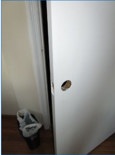
Door hardware noted as missing.
