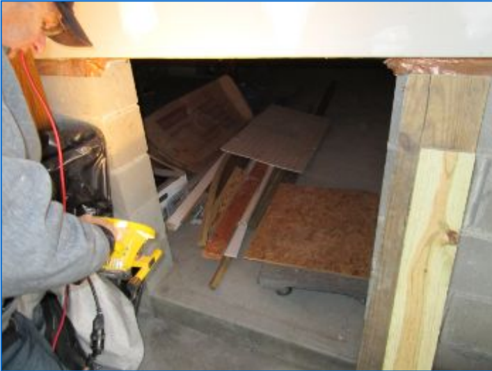
Crawlspace access door was missing. Recommend a proper door be installed.
