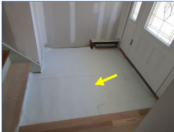
Entryway flooring was not installed.
