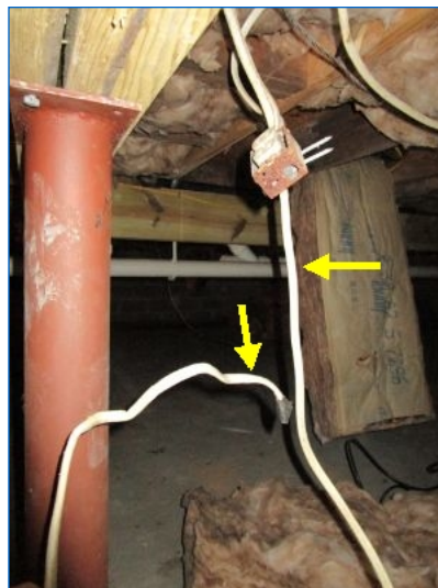
Potentially abandoned wiring visible in the crawlspace should be evaluated by a qualified electrical contractor to determine whether any wiring is still energized. Improperly terminated, energized wiring is a shock/electrocution hazard.
