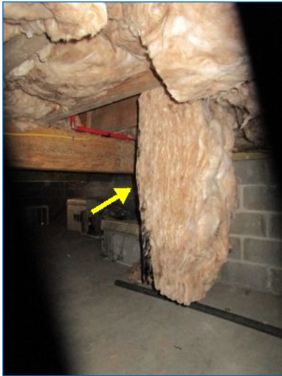
Batt insulation was observed to be hanging/missing at a few joist cavity locations. Recommend restoring missing/hanging insulation and securing in place using insulation support wires.
