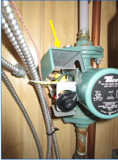
Circulator terminal box cover was open; exposed wires, contractor to close box.
