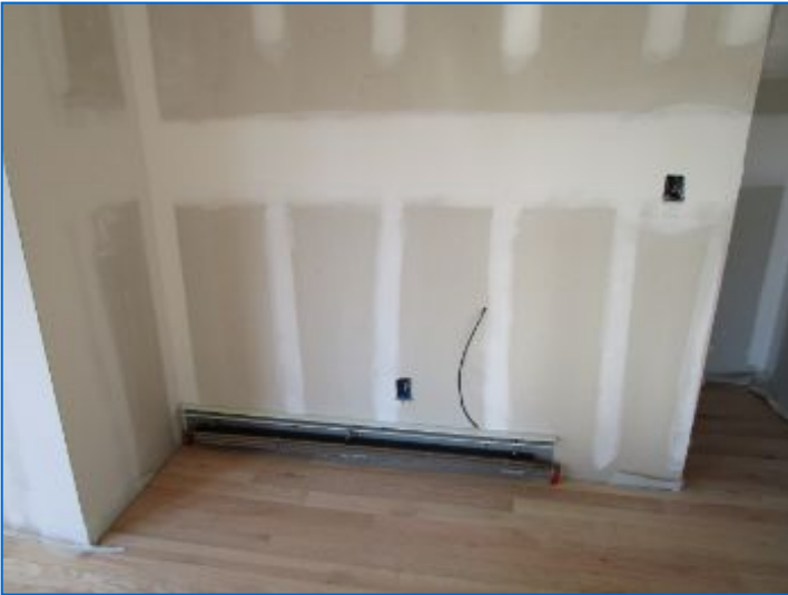
Doors, door/window hardware, baseboard, casings, sills, moldings/trim, transitions, receptacles, switches, lighting, baseboard enclosure parts, finishes, etc. were not yet installed.
