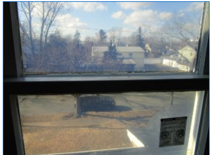
Front window hardware noted missing.
