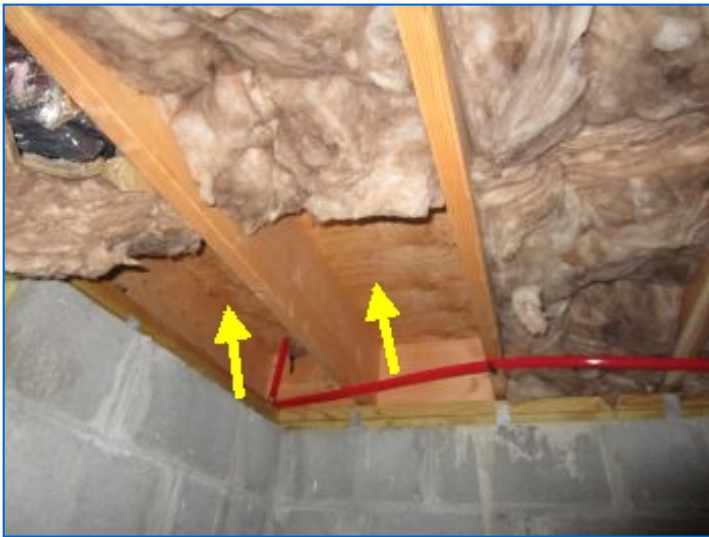
Batt insulation was observed to be hanging/missing at a few joist cavity locations. Recommend restoring missing/hanging insulation and securing in place using insulation support wires.
