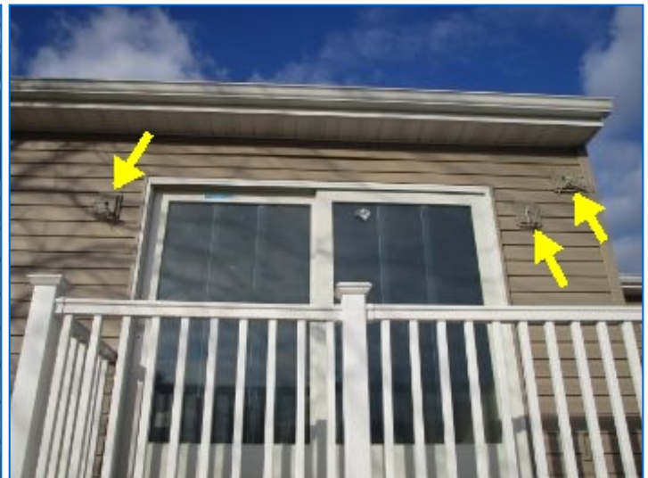
Exterior light fixtures not installed at three mounting bases at the east wall, leaving exposed wires that can potentially become energized.
