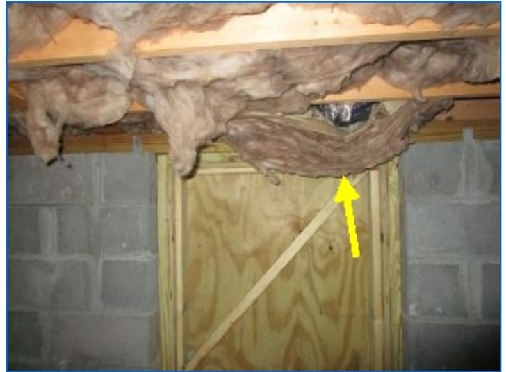
Batt insulation was observed to be hanging/missing at a few joist cavity locations. Recommend restoring missing/hanging insulation and securing in place using insulation support wires.
