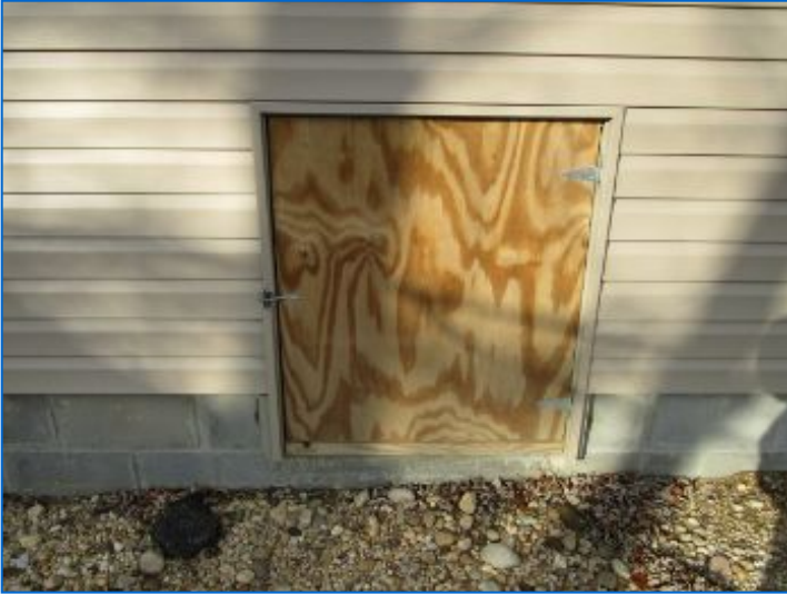
Exterior door for crawlspace not finished or secured. Recommend contractor provide a properly finished and lockable access door.
