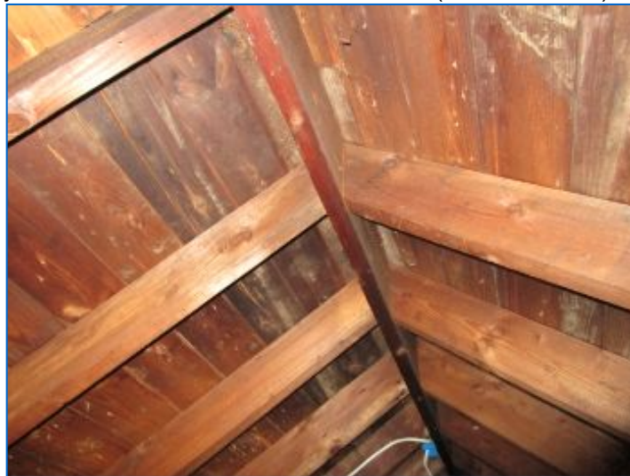
Roof Structure: 2x6 Rafters 16" O.C., 2x8 ridge beam, T&G and plywood roof boards.
