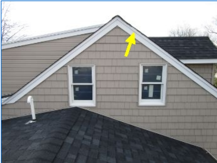
Signs of inferior workmanship by roofers. Jagged shingle cut/damaged edges.
