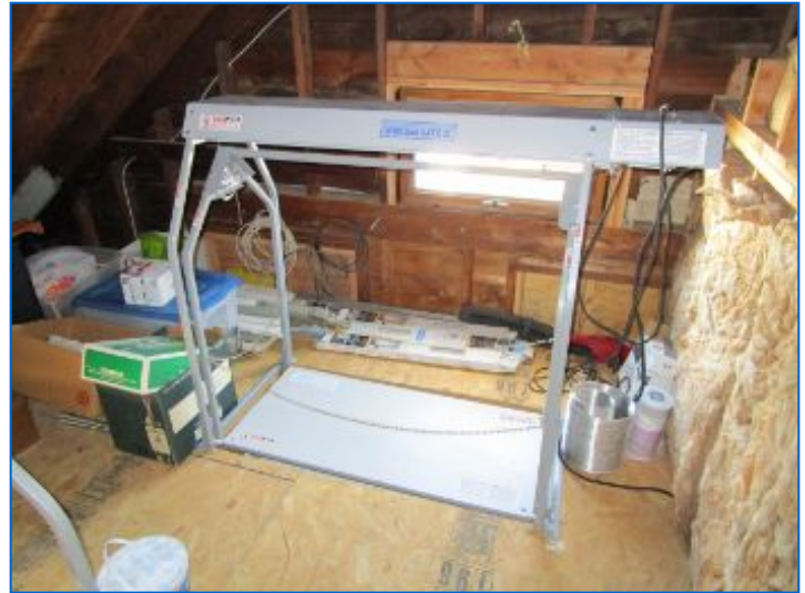
Attic storage lift did not have a dedicated outlet installed.
