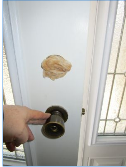
Front door hardware was missing.
