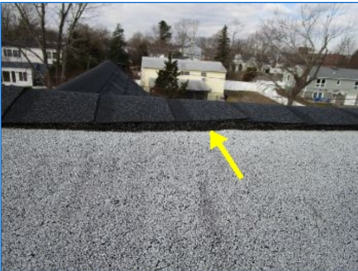
Ridge cap shingle overlap appeared too little at ridge vent and low-slope roof interface (potential water intrusion).
