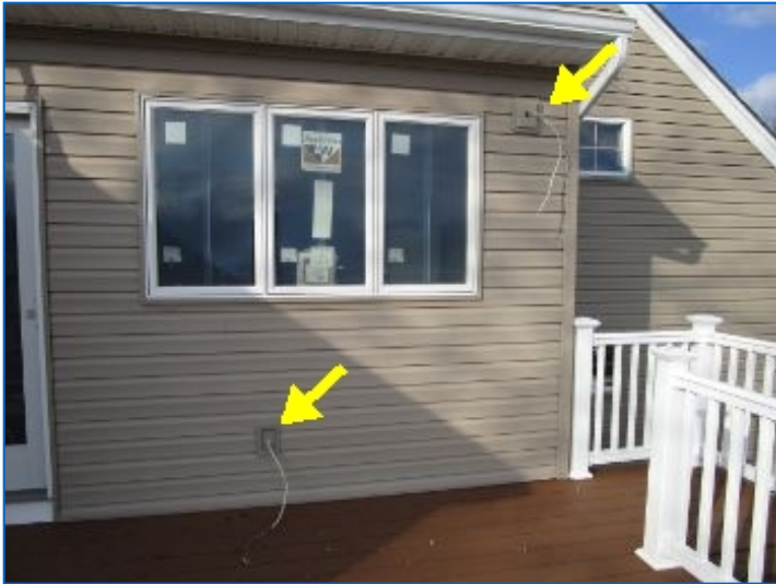
Exterior two light fixtures not installed at east facing wall leaving exposed wires that can potentially become energized.
