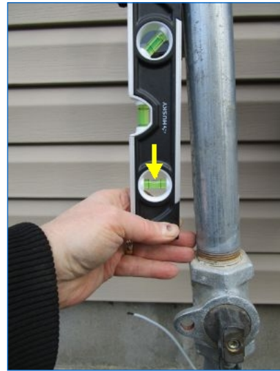
Gas service elevated pressure pipe was not vertical; possibly stressing the pipe. This is not typical of gas company installations. Recommend asking National grid to review installation and coordinate corrective action with contractor.
