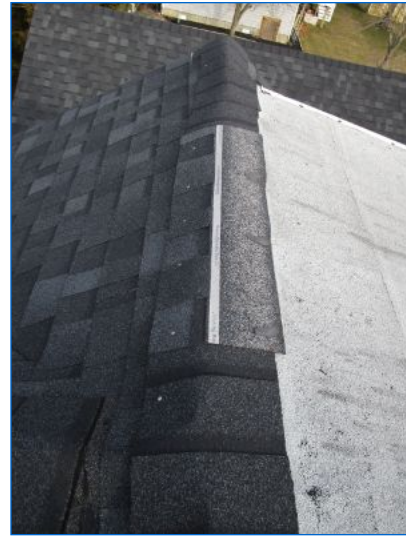
Signs of inferior workmanship by roofers. Conditions that can lead to water intrusion noted. The Inspector recommends review by a qualified roofing contractor to provide remedial improvements and warranty workmanship for the roof.
