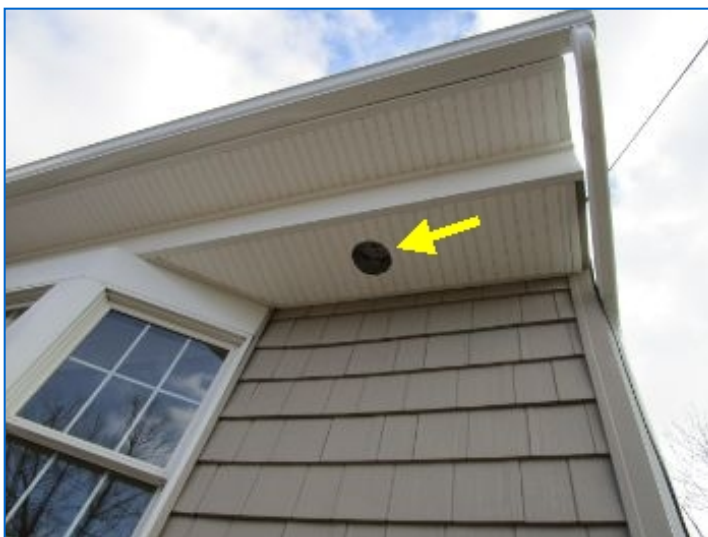
Exterior recessed can trim rings and bulbs not installed at front porch.
