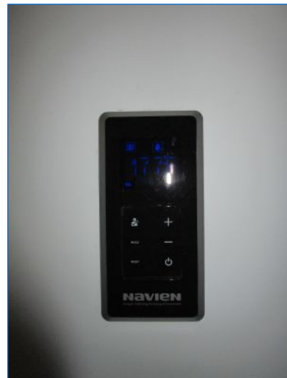
Heating Equipment located in Garage area was operable; delivering 177F supply water temperature.
