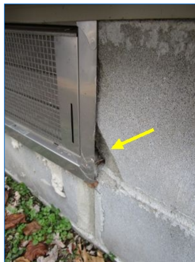
Damaged concrete block at flood opening at rear of garage. Suggest concrete repair.
