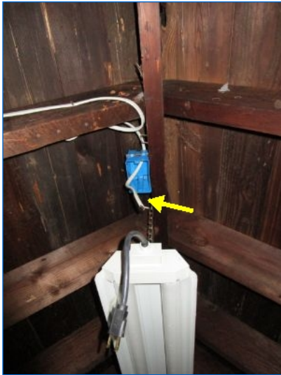
Incomplete electrical for attic lighting noted.
