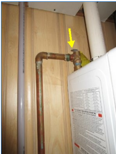
TPR (Temperature Pressure Relief) valve and discharge pipe show no deficiencies.
