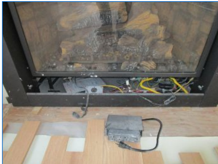
Gas fireplace surround/mantle, stone hearth and manufacturer approved startup of fireplace was yet to be completed.
