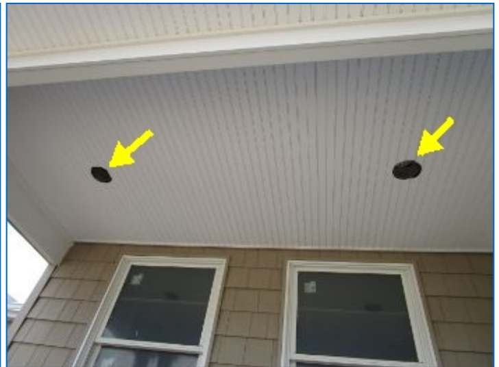
Exterior recessed can trim rings and bulbs not installed at front porch.
