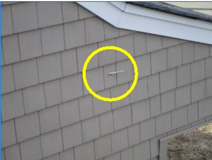
Exterior fixture/device not installed at north-facing wall leaving exposed wires.
