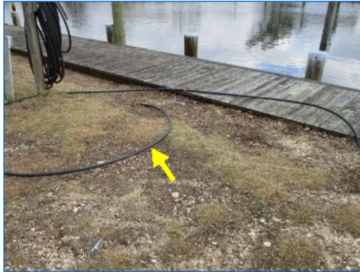
Underground water supply work was incomplete at east side/dock area.
