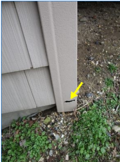
Cracked/damaged vinyl corner trim noted.
