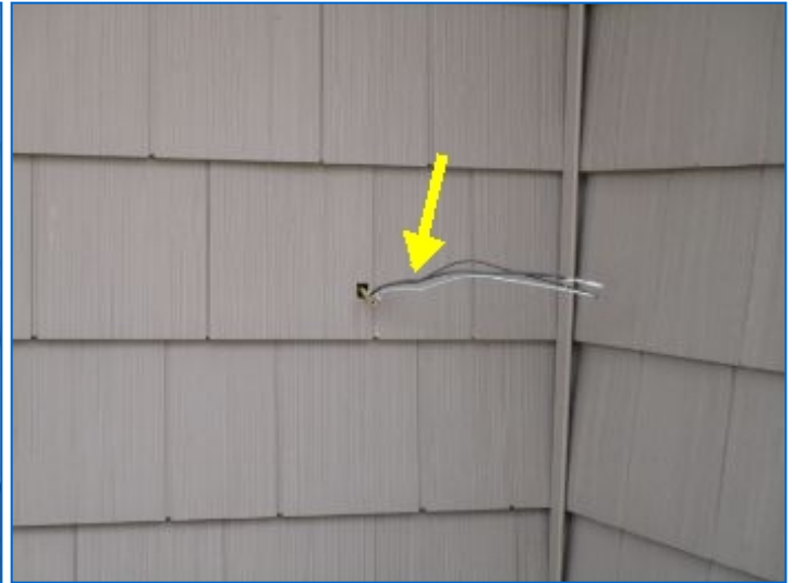
Exterior GFCI type receptacles were not installed at front leaving exposed wires that can potentially become energized.
