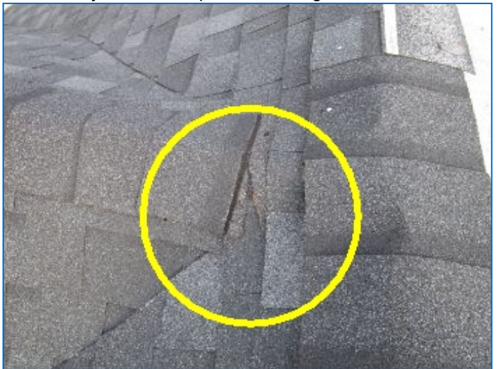
Some shingles damaged; improper nails used; undercut shingles; shoddy repairs noted Recommend proper repairs by a licensed qualified roofing contractor.
