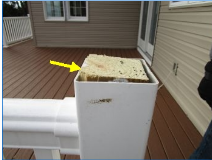
Post cap did not fit properly due to over extended wood post.
