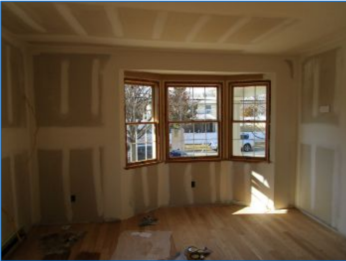
Doors, door/window hardware, baseboard, casings, sills, moldings/trim, transitions, receptacles, switches, lighting, baseboard enclosure parts, finishes, etc. were not yet installed.
