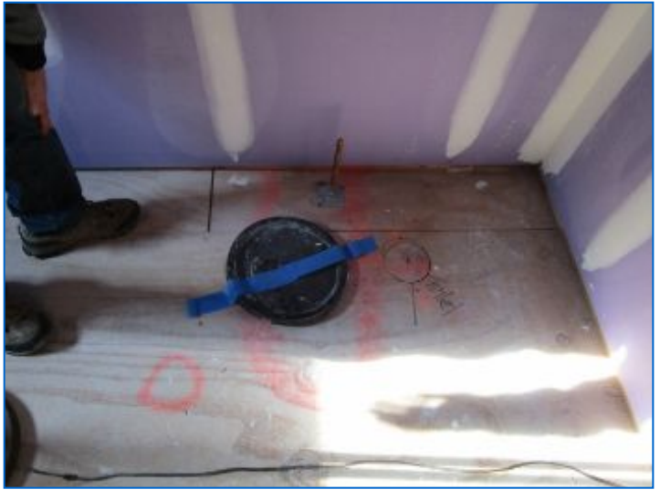
Floor tile, baseboard heat, door/window hardware, casings, sills, baseboard, moldings/trim, transitions, GFCI/receptacles, switches, lighting, exhaust fan, cabinets/counters, plumbing fixtures, accessories, grab bars, finishes, etc. were not installed.
