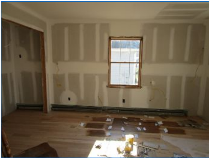
Doors, door/window hardware, baseboard, casings, sills, moldings/trim, transitions, receptacles, switches, lighting, baseboard enclosure parts, finishes, etc. were not yet installed.
