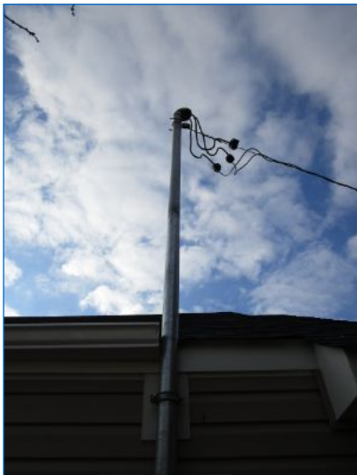
Overhead electrical service drop and riser showed no major system safety or function concerns at time of inspection.
