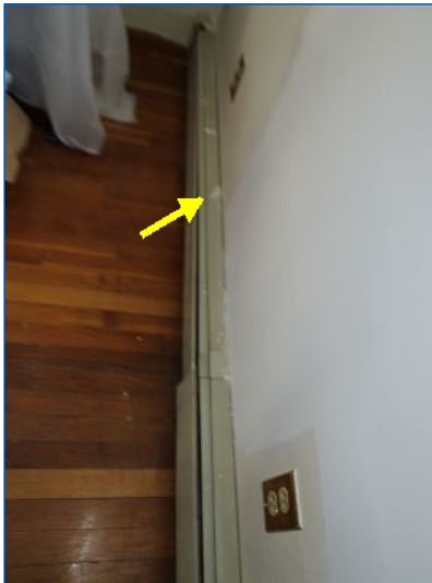
Contractor is responsible to clean up all spackle/paint drippings.
