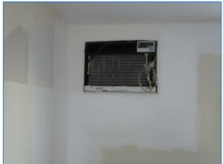
A/C front cover was missing/broken and needs replacement for proper operation.
