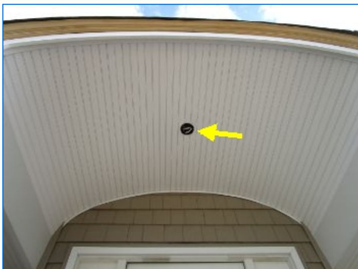
Exterior light fixture not installed at front porch.
