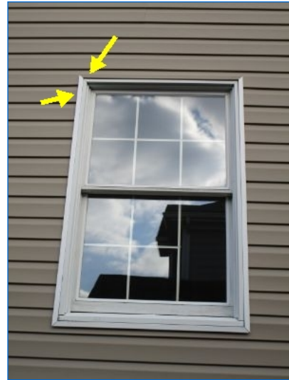
Color mismatched at south facing window trim. Other window trim is tan.
