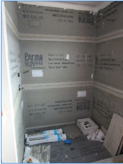
Shower tile work, plumbing/fixtures, wall accessories, grab bar, enclosure, lighting, finishes, etc. were not installed.
