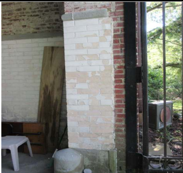
IMG_1178.JPG Glazed brick with glazed surface damaged and missing.
