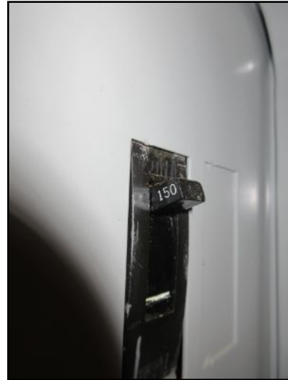
Main Panel #2 Main Disconnect: 150 amp main breaker serves Part of the property.
