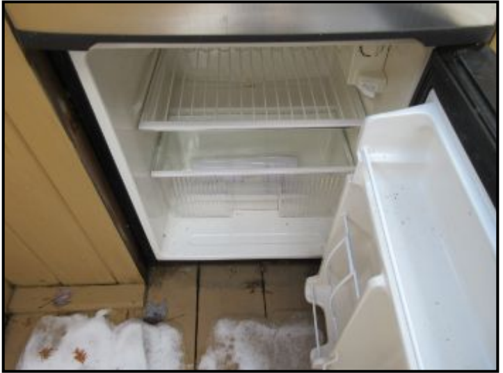
Mini-fridge at barbecue station was not powered/operating; appeared fairly new and unused. Recommend requesting seller to confirm the completion of mini-fridge installation.
