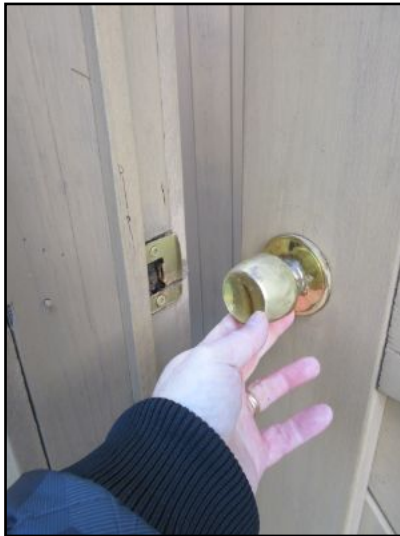
Door at outdoor shower did not latch; suggest hardware repair.
