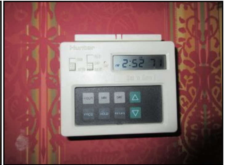
Digital Programmable type thermostat noted in Master bedroom.
