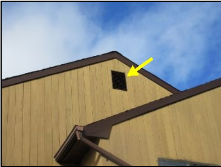
Gable-end louver vent(s) noted for attic ventilation.
