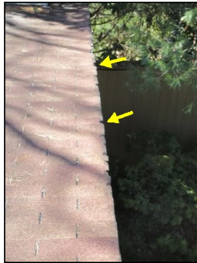
Signs of past shingle damage caused by tree branches abrading shingle edges.
