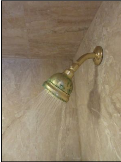
Shower head had water deposits/stains.
