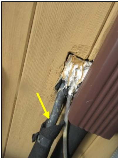
AC#1 Outdoor refrigerant pipe insulation is deteriorated/missing at outdoor condenser. Recommend replacing outdoor deteriorated/missing insulation for the larger suction line.
