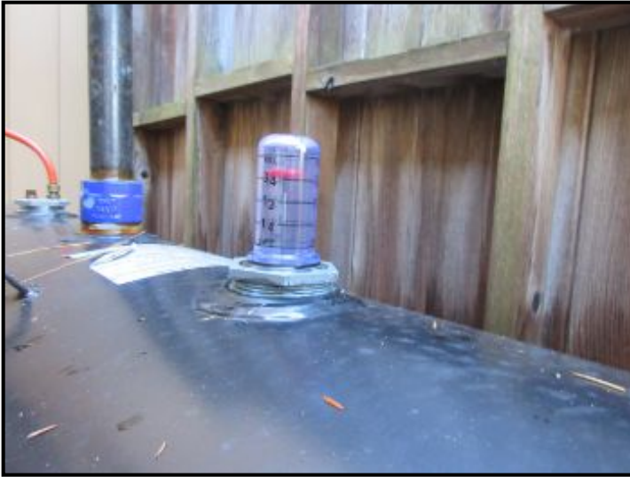
Oil tank gauge indicated the tank was approx. 3/4 full at time of inspection.
