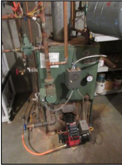
Oil-fired Heating Equipment located in Basement was operable.
