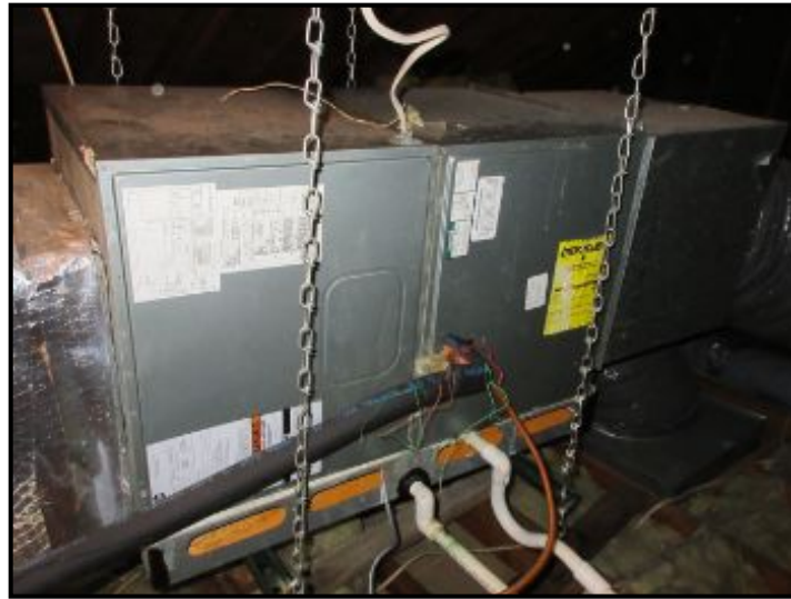
Central Air Handler (A/C#1) located in Attic.
