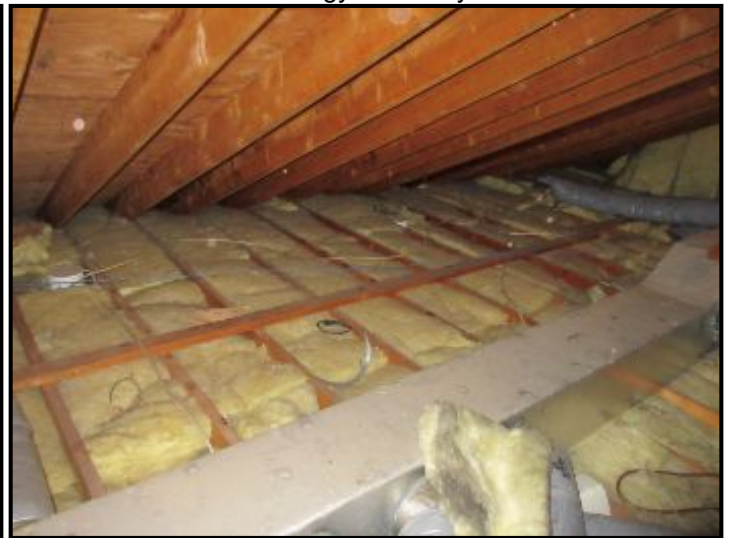
Installed in joist cavities.
