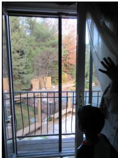
Sliding screen has damage at bottom at master bedroom balcony. Suggest screen repair.
