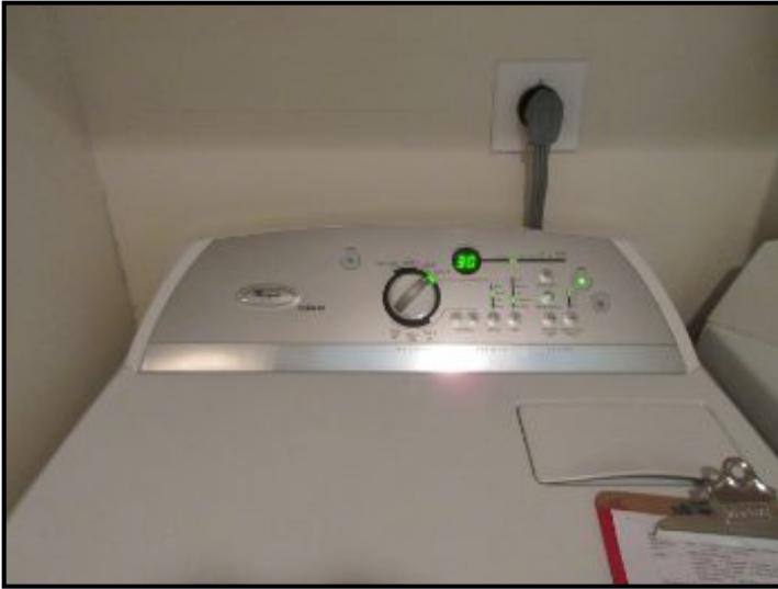
Electric dryer was operable. Estimated age of the dryer is 5+ yrs.
