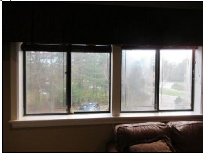
Condensation visible in the double-pane glazing of windows in the Den (2nd floor) indicated a loss of thermal integrity.
