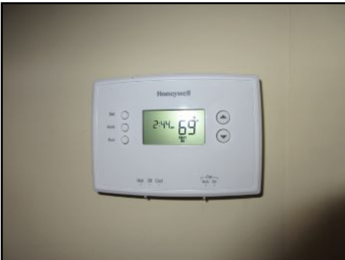
Digital Programmable type thermostat noted in Basement.
