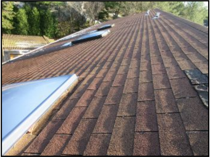
At the time of the inspection, asphalt composition shingles covering the roof of this home appeared to be at or near the end of their useful lives.
