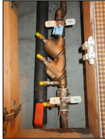
Backflow preventer for sprinkler system noted.
