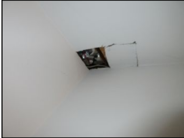
2nd floor, front eave storage space: Unrepaired opening in ceiling.
