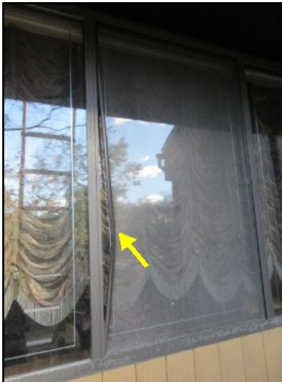
Damaged screen observed at the Front of the home.
