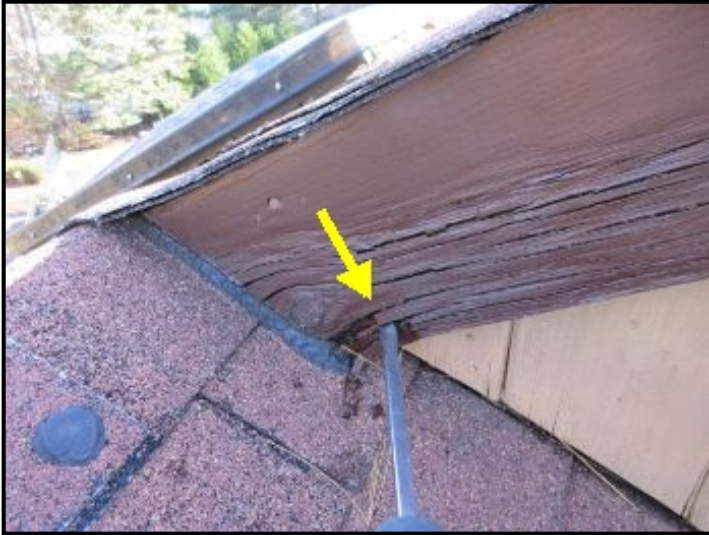
Wood deterioration noted at barge boards (north). Recommend replacement of deteriorated barge boards at time of roofing replacement.
