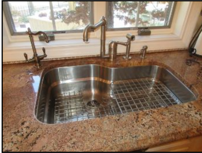
Faucets operated normally at time of inspection.
