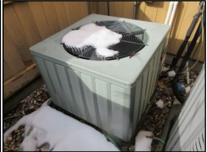
AC#1 Condenser: corresponding Air Handler located in the Attic serves the 1st floor & Basement.
