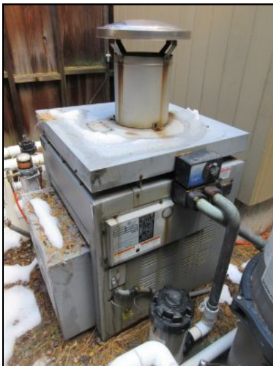
Oil-fired Pool heater generally appeared to be in serviceable condition at the time of the inspection, however was shut-down, winterized and could not be tested at time of inspection.
