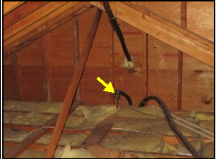
Unused set of A/C refrigerant piping noted.
