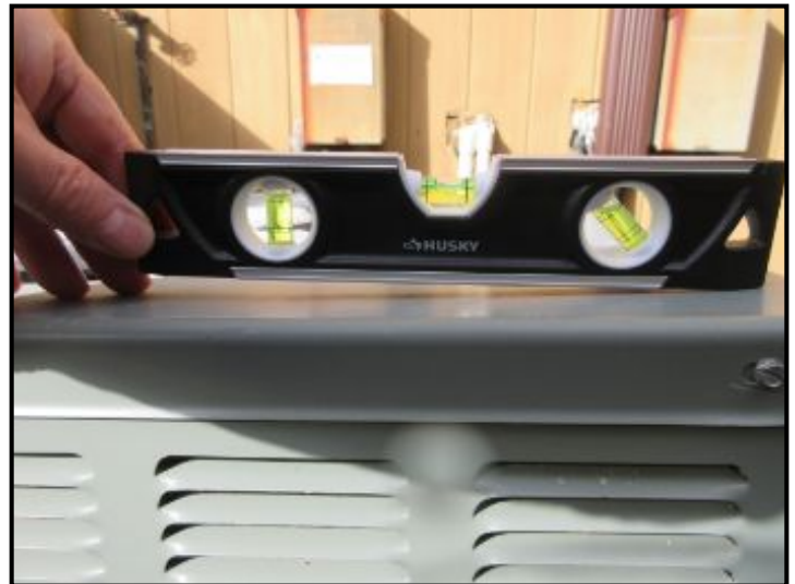
AC#1 condenser is not level; this may shorten motor life. Suggest leveling mounting pad or unit itself.
