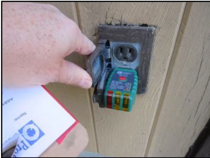
No Power at Non-GFCI type receptacle/s at time of inspection. Recommend having seller locate source / restore power prior to close.
