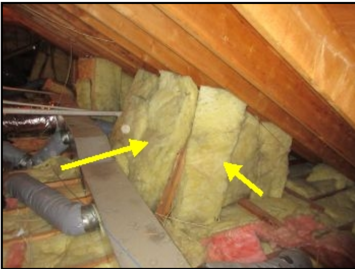
Installed in wall cavities of vaulted ceiling areas.
