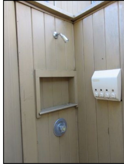
Outdoor shower was turned off at time of inspection (winterized perhaps); unable to test.
