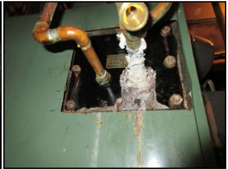
Unit's general condition indicates that it has reached its designed life expectancy. Consider replacement. We make no warranty, guarantee or estimation as to the remaining useful life of this unit.
