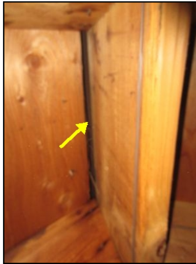
Ridge exhaust venting noted at north end of attic.
