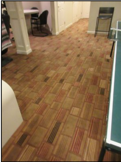
Limitation: Concrete floor slab was Mostly concealed by Floor Covering; unable to fully inspect floor slab.
