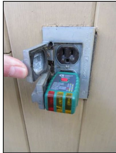
No power at GFCI type receptacle/s at time of inspection. Recommend having seller locate source / restore power prior to close.
