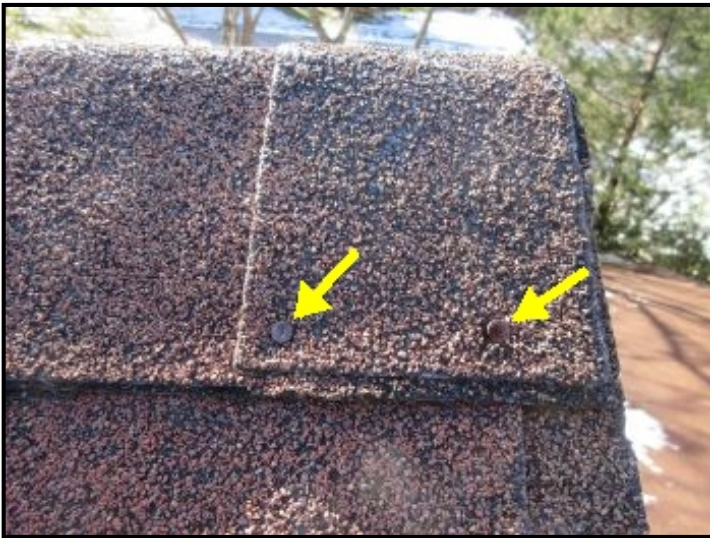
Exposed nail heads on roofing material. Recommend sealing all fastener heads.
