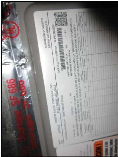
AC#2 Rheem Air Handling Unit data plate/serial no. indicates a cooling capacity of 4 tons, and a manufacture date of 5/2015, (3.6 yrs old).
