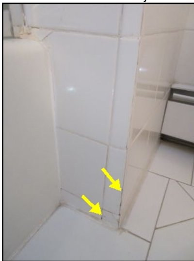
Wall tile damaged, grout cracked/missing; suggest tile and grout repair/s.
