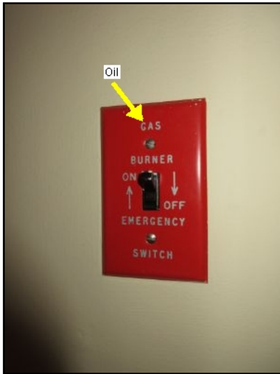
Oil Burner: Remote Emergency Shut-off switch noted.
