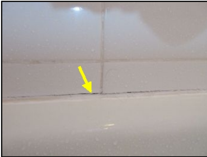
Tub perimeter grout (movement joint) is cracked/missing. Suggest replacing grout with matching silicone based sealant at movement joints.
