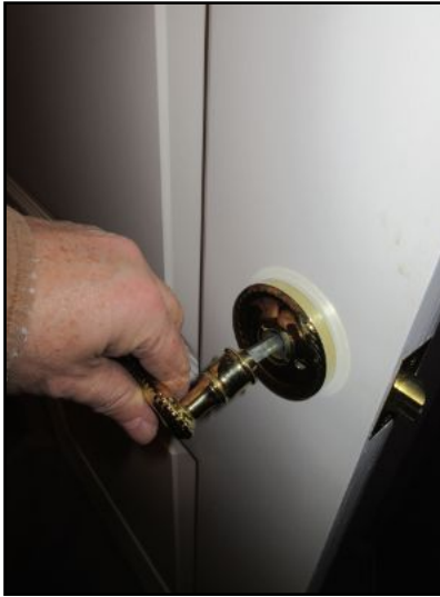
Door lever minor repair needed for Bedroom (2nd floor, rear).
