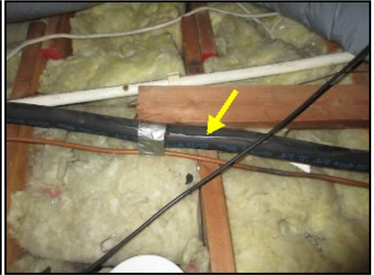
Refrigerant pipe insulation not covering entire pipe in attic space where condensation can form and drip onto insulation. Recommend HVAC technician review conditions and make any corrective repairs.
