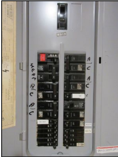
Main Panel #2: 20 circuit breaker spaces; 0 spare breaker space(s) noted.
