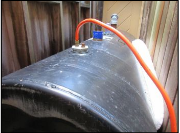
Above ground fuel oil tank currently dedicated to the pool heater.
