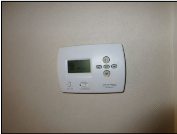
Digital Programmable type thermostat noted in Hallway (2nd floor).
