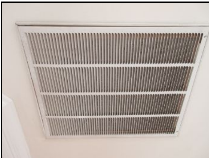
AC#1: Disposable filter located in filter-grille at Hallway (2nd floor) ceiling.
