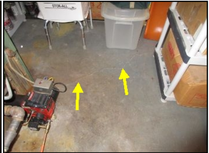
Common shrinkage/settlement cracks observed in concrete floor slab; these may leak at some point.
