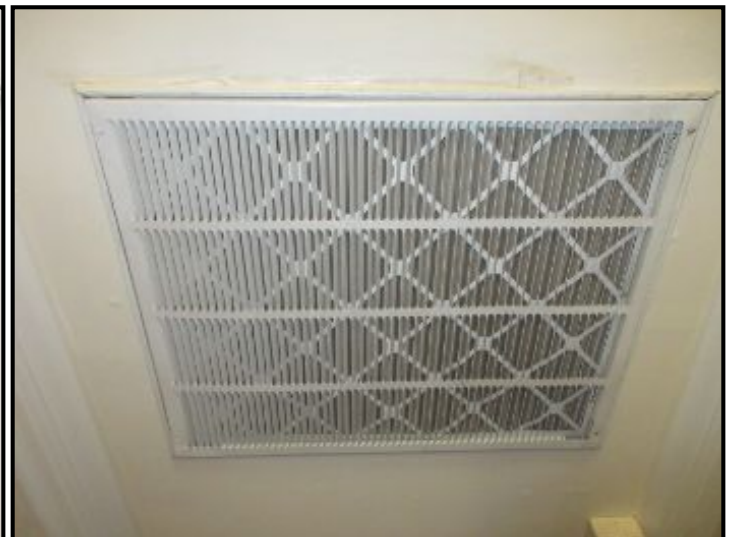
AC#2: Disposable filter located in filter-grille at Hallway (2nd floor) ceiling.
