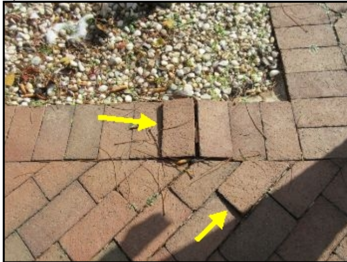
Uneven settlement of brick walkway noted. Monitor and/or repair to prevent potential trip hazard from developing.
