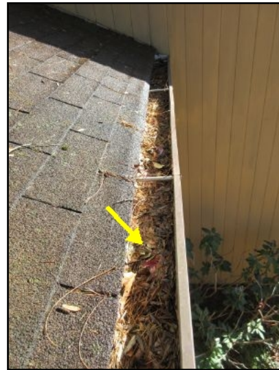
MAINTENANCE: Keep gutters cleared of organic debris to prevent downspouts from being clogged, causing overflow and ice damming at gutters; ensure that all downspouts have extensions to carry water away from the foundation.
