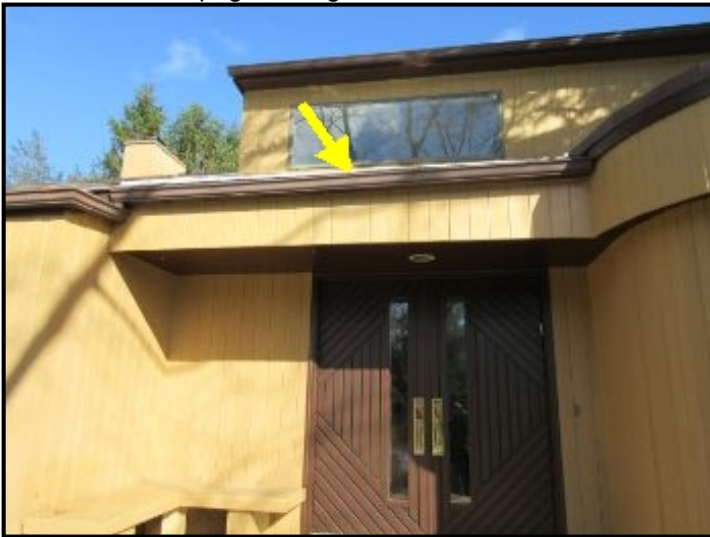
Front gutter clogged with debris prevented proper drainage (overflow) at time of inspection
