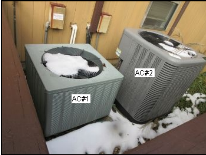
Multiple Central A/C split-systems, each with outdoor condenser and Ducted indoor air handler.
