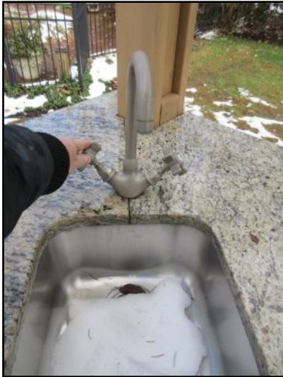
Bar sink turned off; winterized; unable to test.
