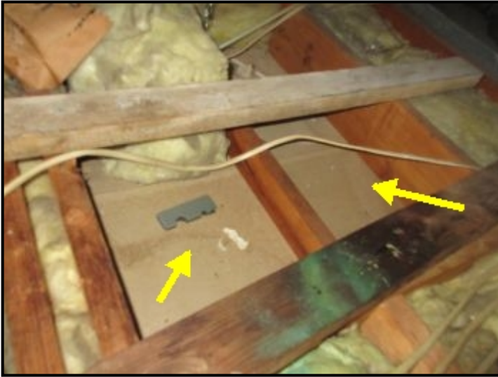
Insulation is missing in some sections of the attic floor.
