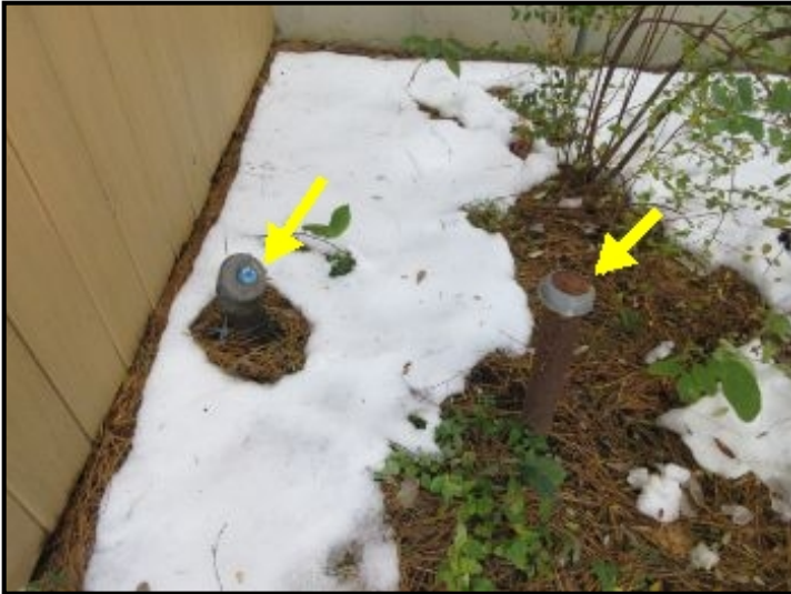
Oil tank fill/vent pipes emerging from the ground at the North side of the house; underground oil tank in use.
