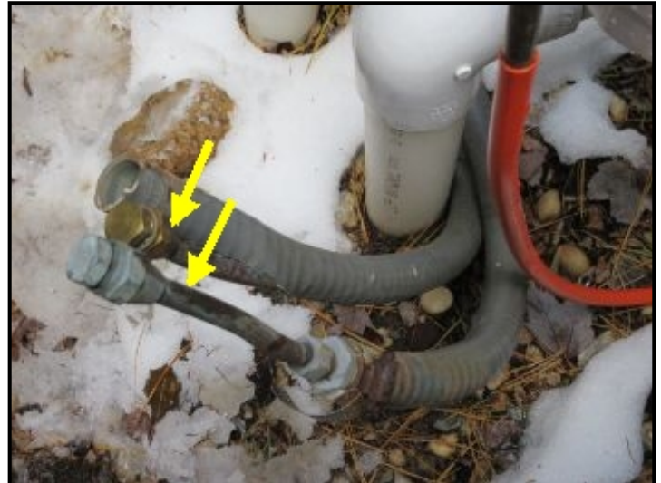
Abandoned oil supply lines from underground oil tank,
