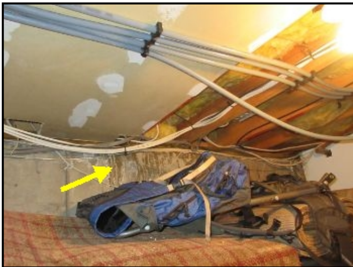
Signs of Past moisture intrusion was observed in the form of stains at the east-side, bare section of the foundation wall.
