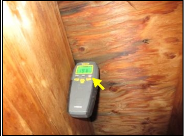
Moisture penetration noted at south end roof boards. Roof cover replacement is recommended.
