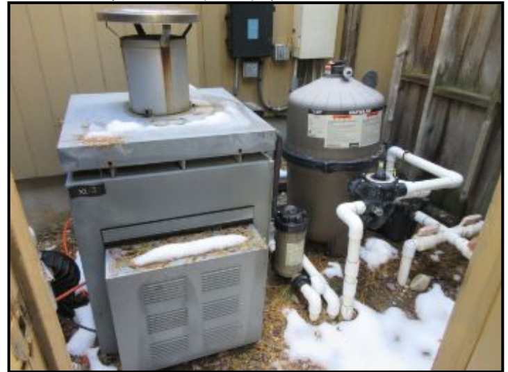
Pool heater, filter, pump/s and piping were winterized; unable to test.
