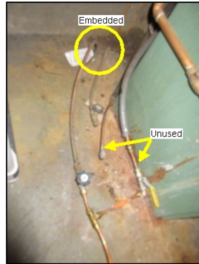
Oil lines (from underground oil tank) embedded in concrete slab is not in compliance with current standards. Installation of above slab line/s recommended in order to reduce possibility of corrosion. Unused oil lines (for pool heater) noted in basement due to new above ground tank installation.
