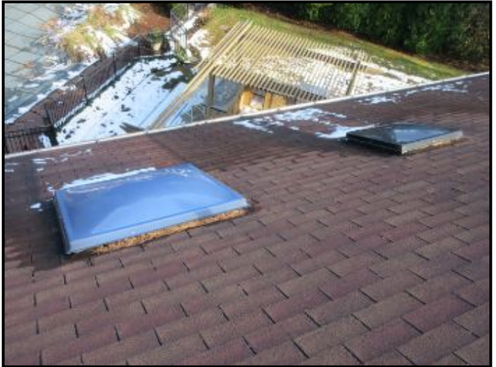
Skylight flashings covered with organic debris; suggest qualified roofing contractor ensure proper seal around skylight/s until roof cover is replaced.
