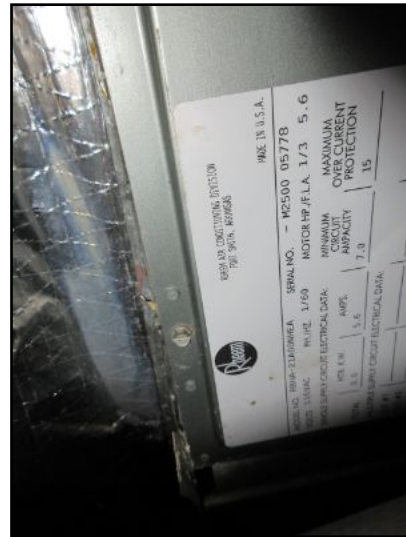
AC#1 Rheem Air Handling Unit data plate/serial no. indicates a cooling capacity of 3 tons, and a manufacture date of 6/2000, (18.5 yrs old).
