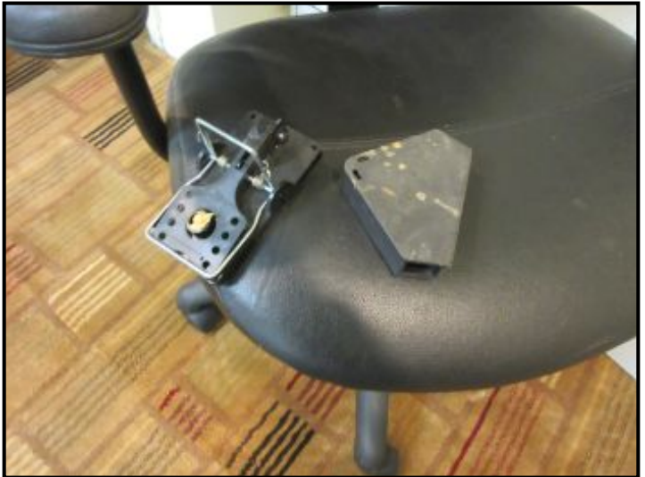
Mouse trap and bait station noted above hung ceiling.
