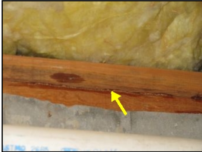
Past termite activity noted at Sill plate at West wall of Basement. Refer to NPMA-33 report.
