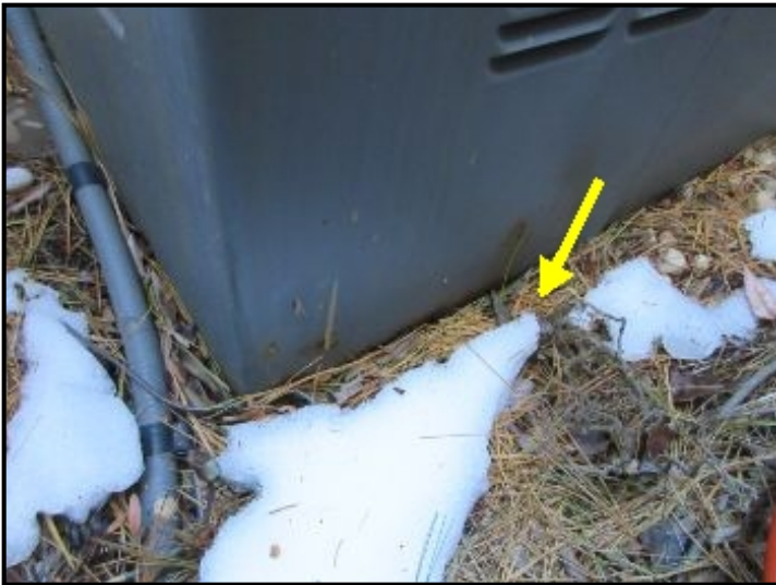
Recommend lowering soil level to prevent contact with pool heater metal casing to prolong the life of the unit.
