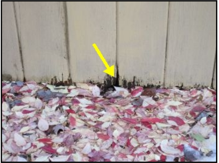
Wood fence shows signs of deterioration; wood in contact with earth. Recommend lowering soil level to prevent wood contact with earth.
