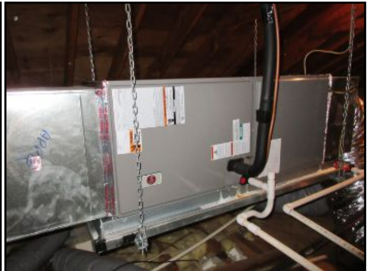
Central Air Handler (A/C#2) located in Attic.
