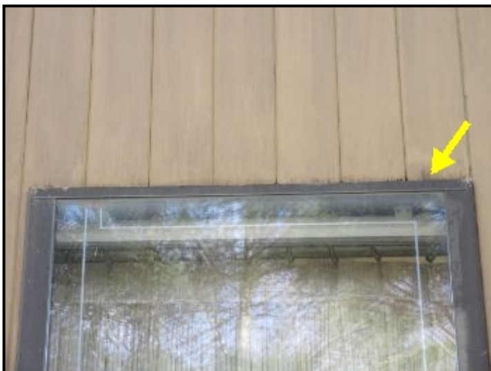
Signs of some siding deterioration along drip edge above original aluminum frame windows due to a lack of sealant here.
