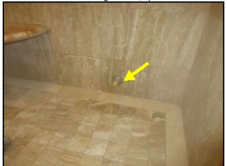
Shower steam generator; operable.
