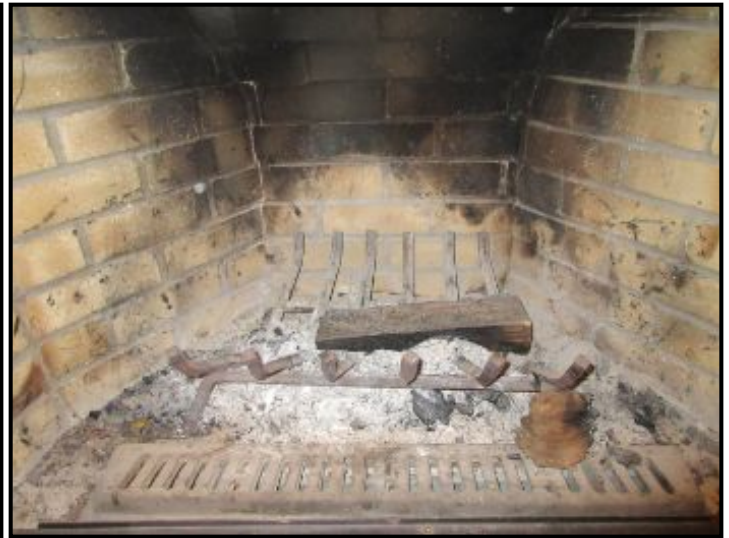
Masonry fireplace noted. Appeared in serviceable condition.
