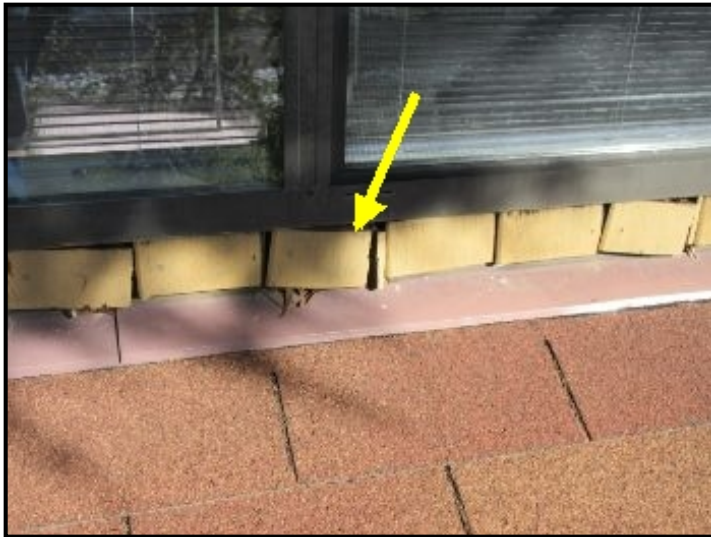
Small pieces of siding not properly secured to wall sheathing at flashing; recommend qualified contractor provide corrective repair.
