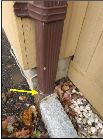
Downspout extension missing at South side. Recommend extending downspout/s 4 ft minimum where possible to divert run-off away from the structure to prevent water seepage through foundation walls.
