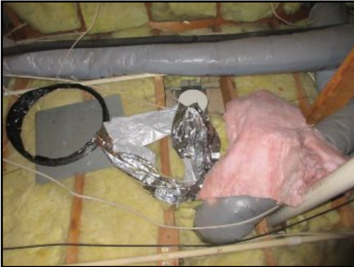
Debris observed in attic left behind from past construction activities. Suggest removing debris. in order to move more safely through attic space.
