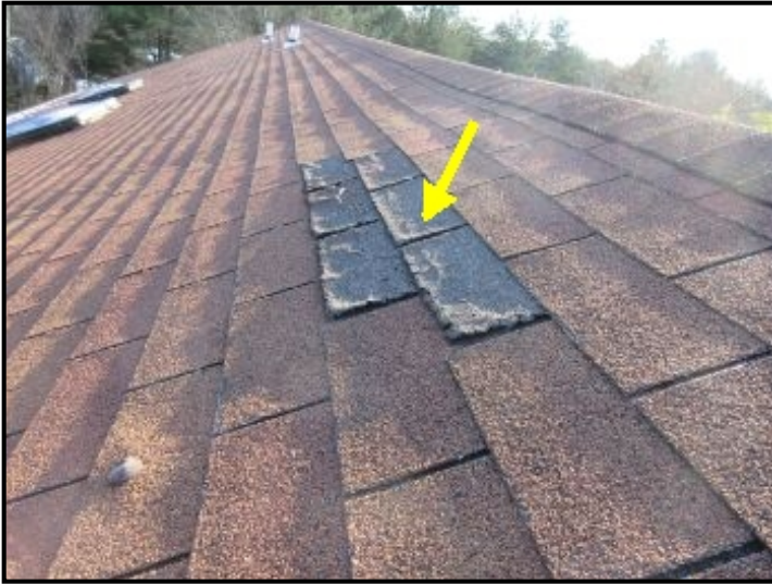
Past roof repair noted.
