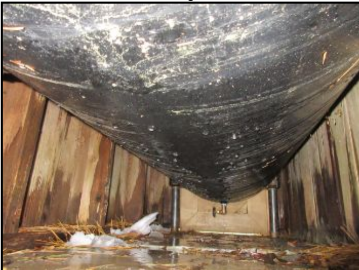
Newer above ground oil tank showed no signs of leakage.
