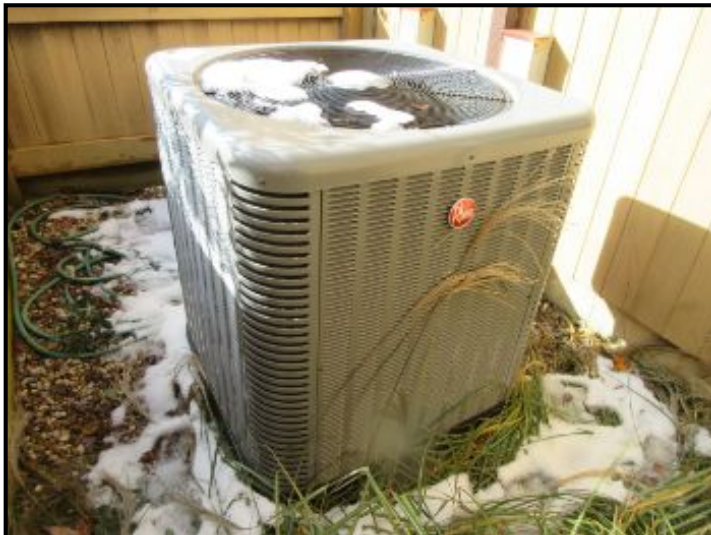
AC#2 Condenser: corresponding Air Handler located in the Attic serves the 2nd floor.
