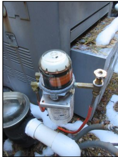
Oil shut-off valve and filter located at burner.
