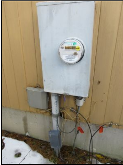
Underground service lateral; 120/240 volts. No major system safety or function concerns noted at time of inspection.
