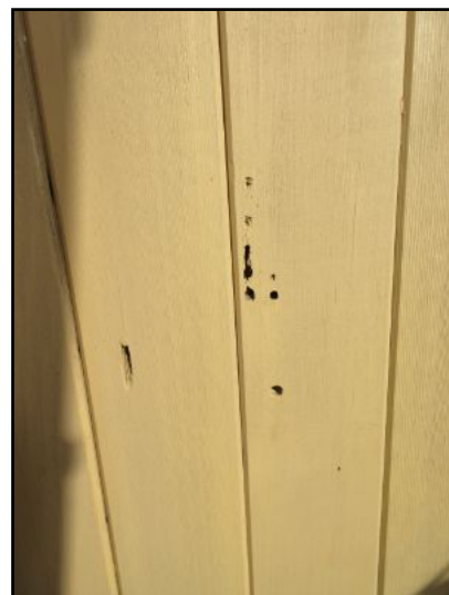
Small holes in front siding below dining room window; appears to be past damage that was since painted over. Not from termites. Cedar siding holes like these are usually the result of woodpeckers foraging for insects.
