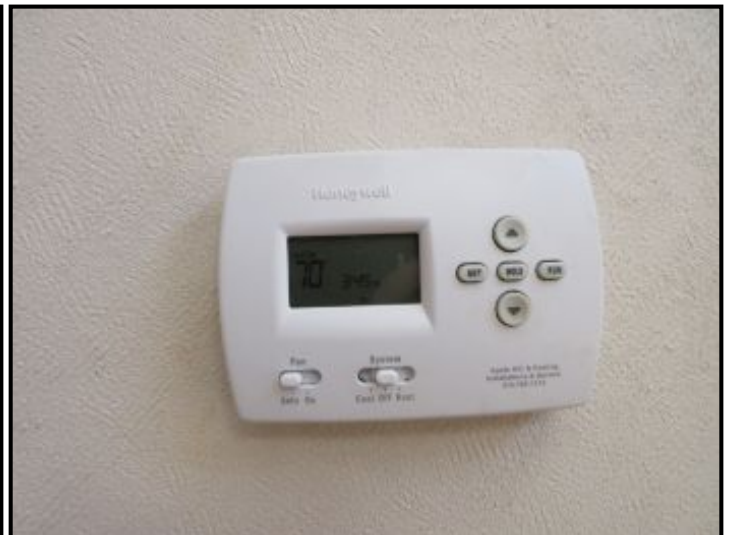
Digital Programmable type thermostat noted in Kitchen/general area.
