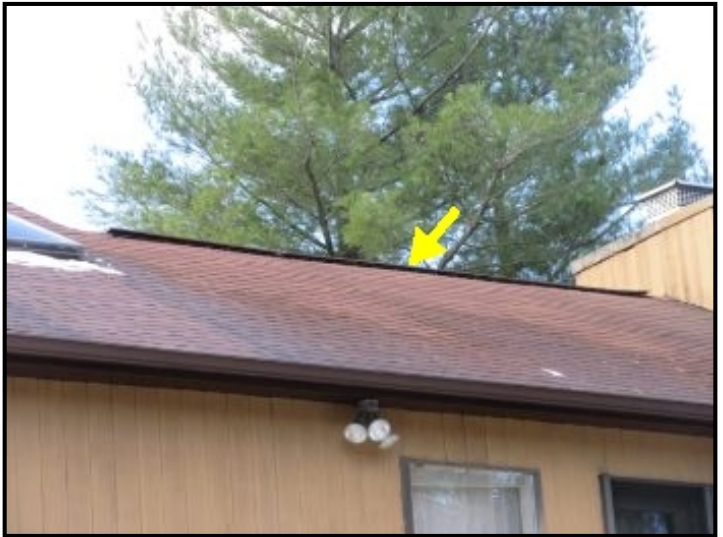
Ridge exhaust venting noted for north attic ventilation.
