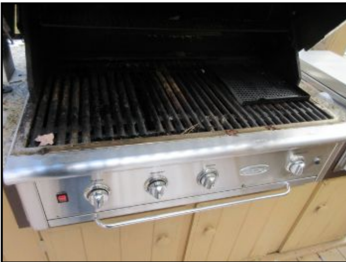
Barbecue left burner did not light via igniter; suggest maintenance be performed to verify all burner operation.
