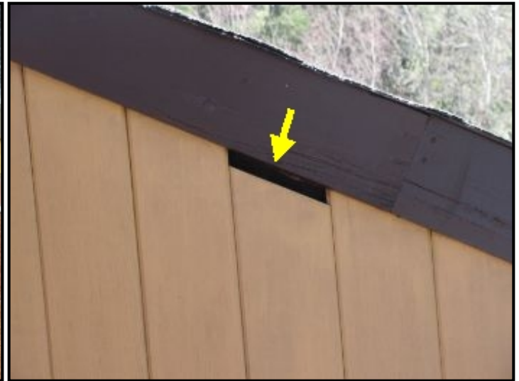
Gap noted at siding in front, facing north; recommend qualified contractor provide corrective repair to prevent water entry.
