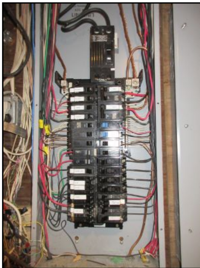
Main panel interior checked.
