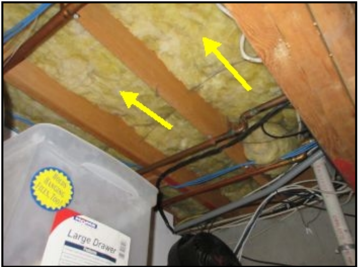
Limitation: Insulation cover at Floor boards, joists, band joists and sill plates; unable to fully inspect main floor structure.
