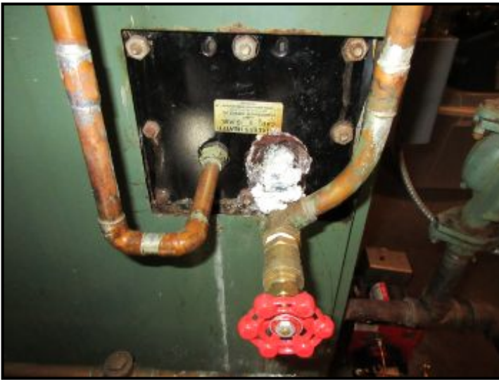
Diversified Heat Transfer manufactured tankless water heater data plate/serial no. did not reveal the manufacture date of the unit. We estimate the unit to be approximately 15+ yrs old.
