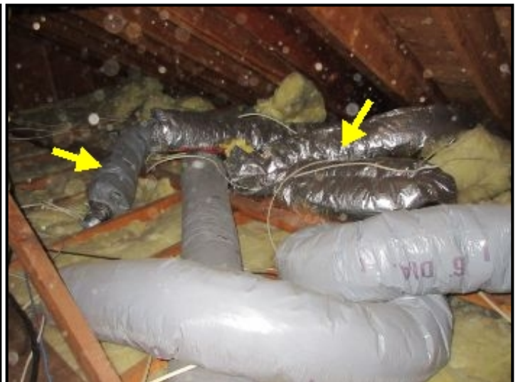
Debris/unused ducts observed in attic left behind from past construction activities. Suggest removing debris. in order to move more safely through attic space.
