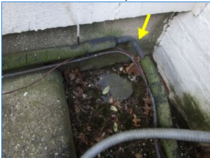
AC#3 outdoor refrigerant pipe insulation was deteriorated/missing at outdoor condenser. Recommend replacing outdoor deteriorated/missing insulation for the larger suction line.
