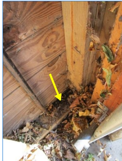
Moderate to severe moisture damage noted at sill plates at all walls of the garage.
