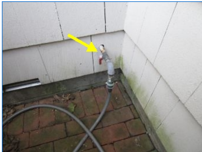
Gas line connection for barbecue.
