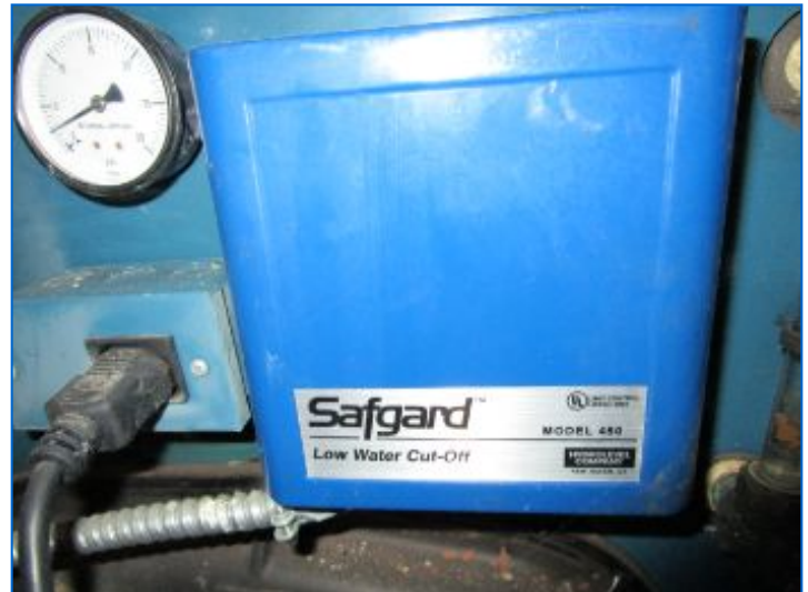
Low water cut-off noted.
