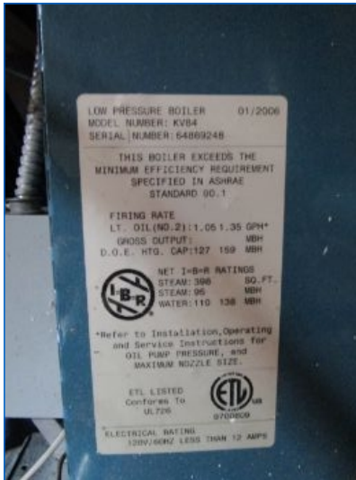
Boiler data plate/serial no. indicates a nominal steam heating capacity of 95,000 Btu/hr, and a manufacture date of 1/2006, (12 yrs old).
