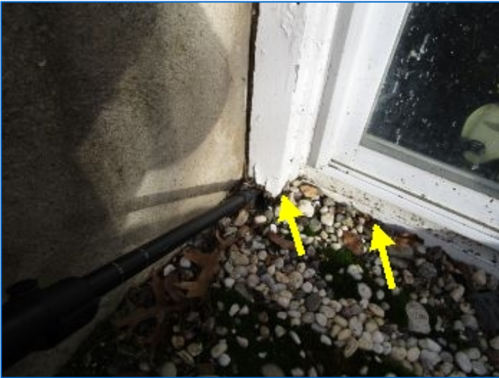
Basement window wood frames in contact with soil showed signs of moisture damage at South side (2 locations). Recommend lowering soil level 6 inches below wood frames and provide top layer of gravel. Repair moisture damaged sections of frames.
