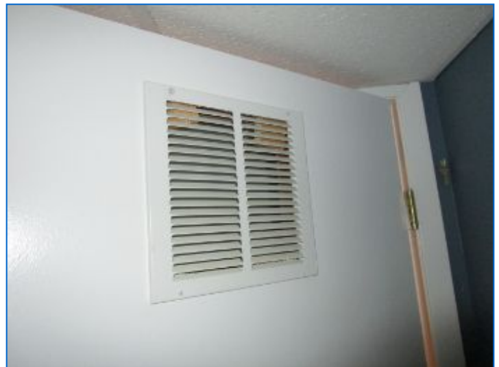
Boiler room door exterior grille was blanked off by sheet metal cover. See Combustion Air Venting notation.
