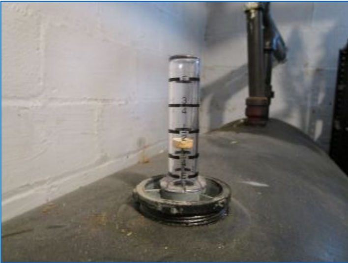
Oil tank gauge indicated the tank was approx. 1/3 full at time of inspection.
