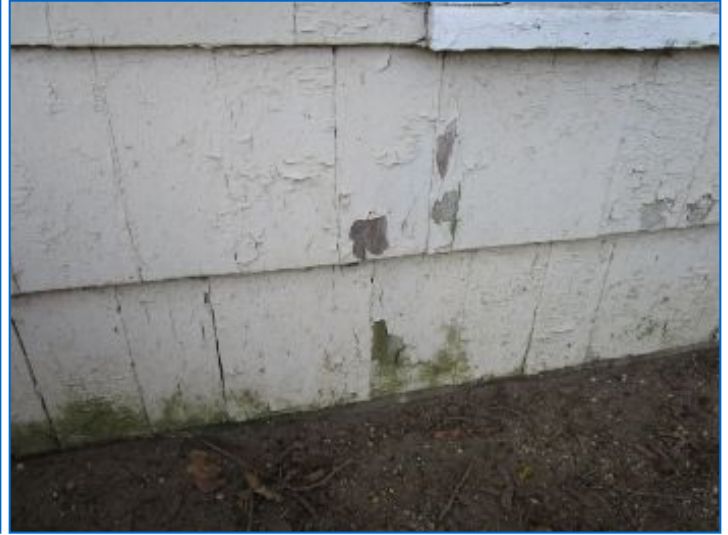
Wood siding covering the exterior walls of the garage had areas of peeling paint exposing the wood siding beneath. Paint should be maintained in good condition to help prevent damage to wood siding from sun and moisture.
