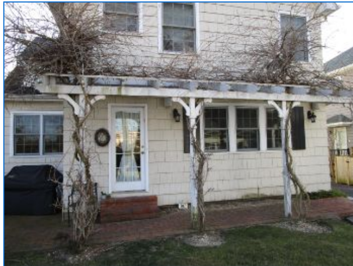
Vines can grow aggressively and can damage siding/finishes and provide a pathway for insects. We recommend cutting back from the structure.
