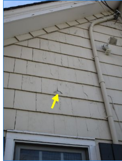
Wood siding covering the exterior walls of the home had areas of peeling paint revealing the white paint layer beneath. Paint should be maintained in good condition to help prevent damage to wood siding from sun and moisture.
