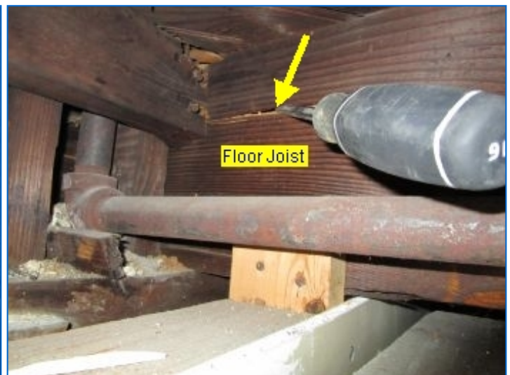
Signs of past termite damage was observed at floor joists, band joist and blocking above basement office at south wall above office in basement. Floor joist repairs were noted. Refer to NPMA-33 Report.
