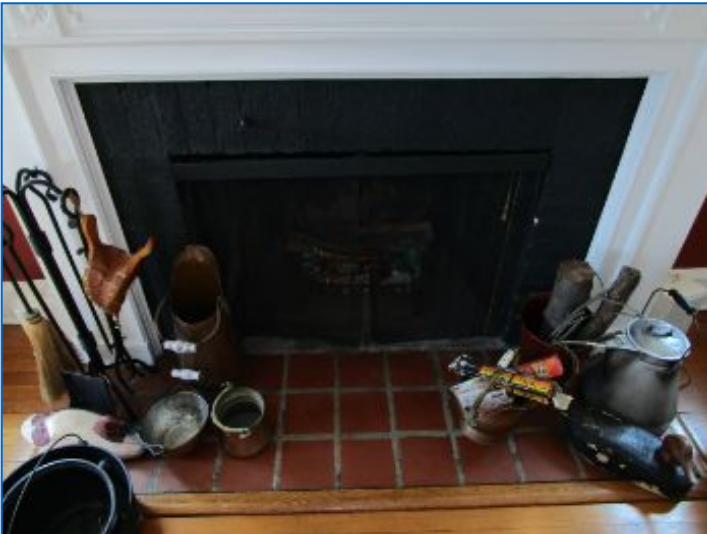
Wood burning fireplace in Living room on 1st floor. Fireplace enclosure was functional.
