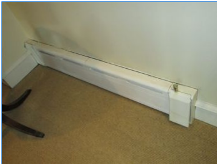
Baseboard cast iron radiators noted
