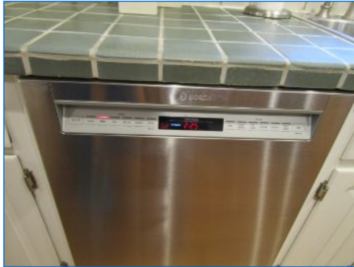
Dishwasher was operable at time of inspection.
