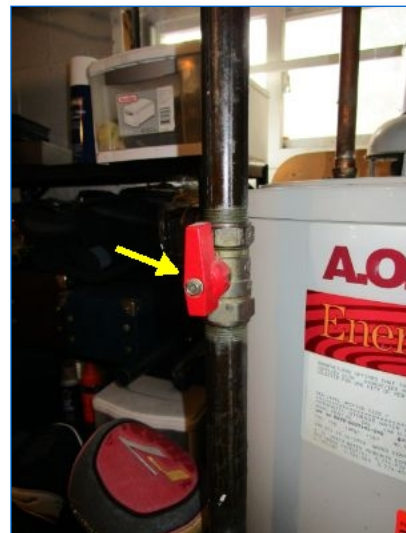
Gas supply shut-off valve and drip leg noted at water heater
