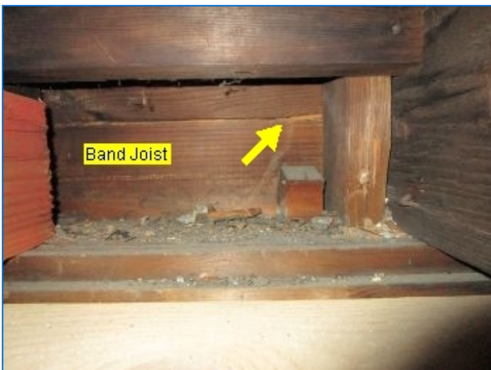
Signs of past termite damage was observed at floor joists, band joist and blocking above basement office at south wall above office in basement. Floor joist repairs were noted. Refer to NPMA-33 Report.
