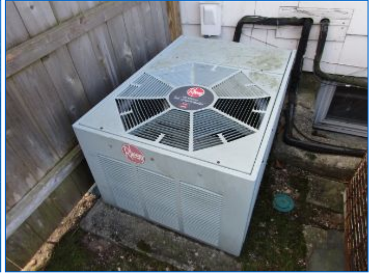
AC#1 Condenser; corresponding Air Handler located in the Attic serves a portion of the home. Refer to Thermostat section.
