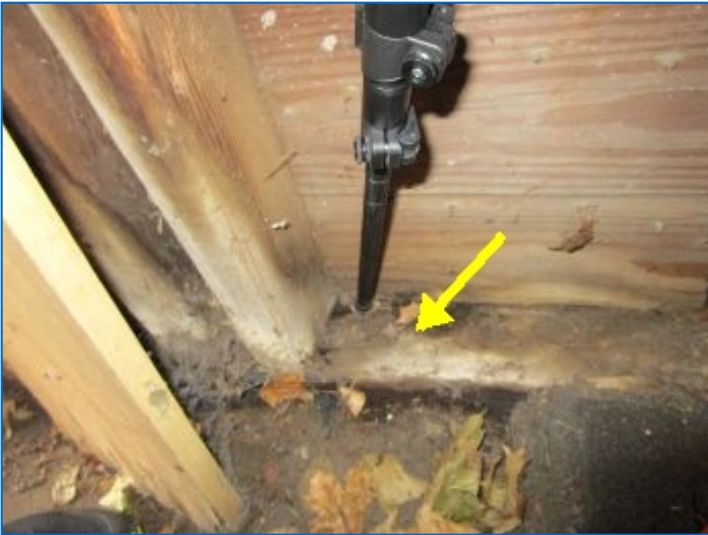
Moderate to severe moisture damage noted at sill plates at all walls of the garage.
