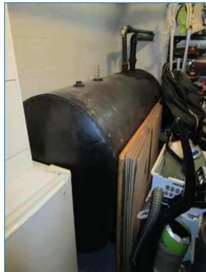
Oil tank located at the basement level.
