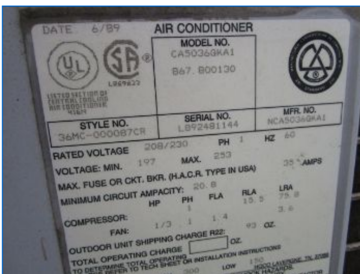
AC#2 Kenmore Condensing Unit data plate/serial no. indicates a cooling capacity of 3 tons, and a manufacture date of 6/1989, (29.5 yrs old).
