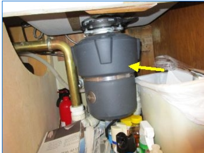
Disposal unit was operable.
