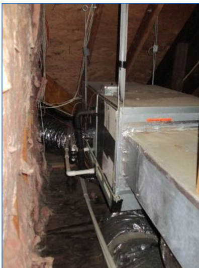
One of three air handlers located in attic eave space serves one of the three cooling zones.
