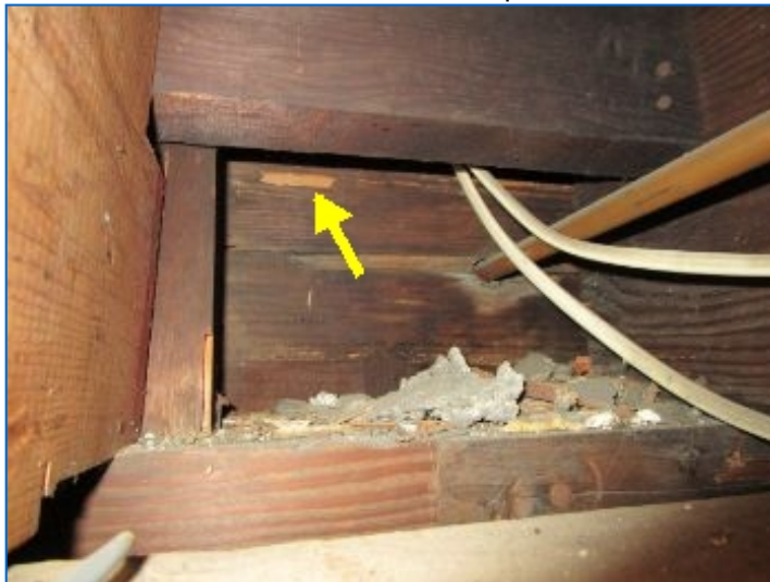
Signs of past termite damage was observed at floor joists, band joist and blocking above basement office at south wall above office in basement. Floor joist repairs were noted (2 places). Refer to NPMA-33 Report.
