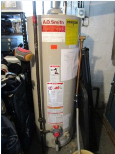
Gas, direct-fired water heater was operable.
