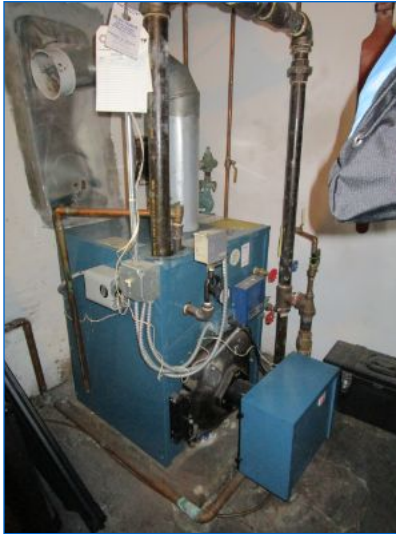
Heating Equipment located in Basement was operable.
