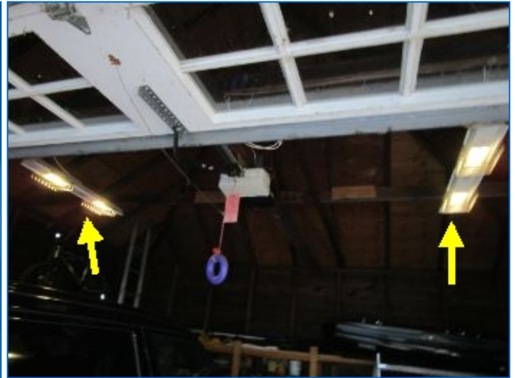
Light fixtures were operable.
