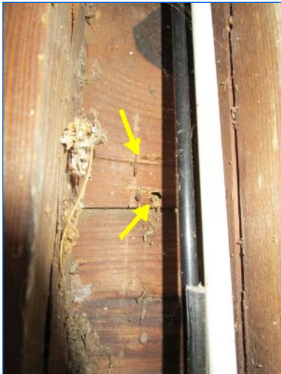
Past Termite damage observed at wall boards at North and South front areas of garage.
