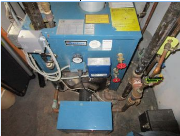
Service Tag Missing. Recommend annual inspection/maintenance be performed by a licensed HVAC contractor to ensure safe and efficient operation.
