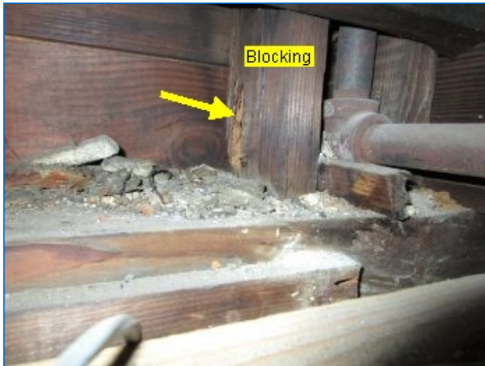
Signs of past termite damage was observed at floor joists, band joist and blocking above basement office at south wall above office in basement. Floor joist repairs were noted. Refer to NPMA-33 Report.
