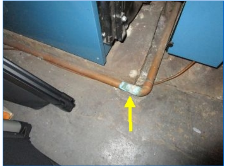
Deposits observed at heating pipe fittings; a sign of past leakage.
