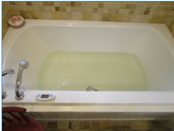
Whirlpool pump was operable at time of inspection.
