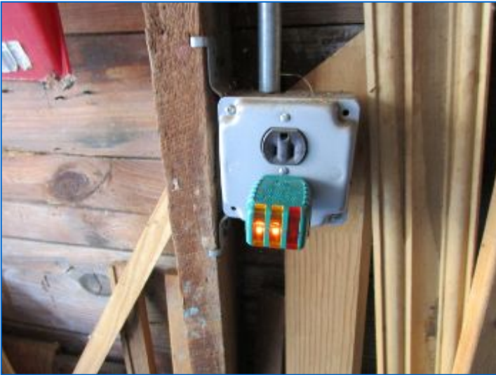
Inside receptacle/s were not GFCI protected. Recommend updating to GFCI protected receptacles. Refer to Electrical section.
