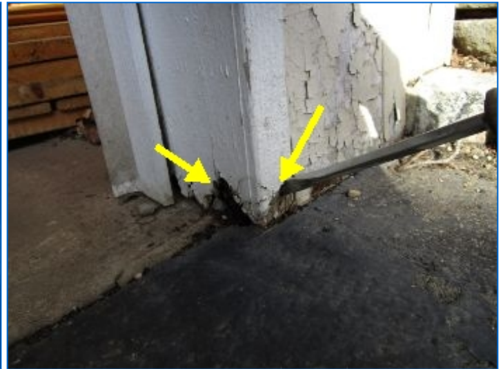
Vehicle door Jamb/s deteriorated (water damage).
