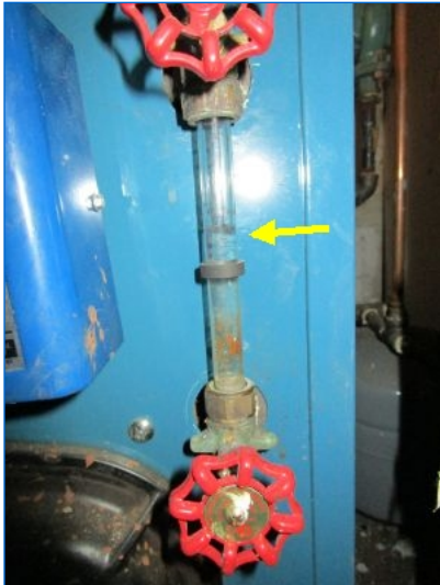
Check steam boiler water level periodically to ensure safe operation.
