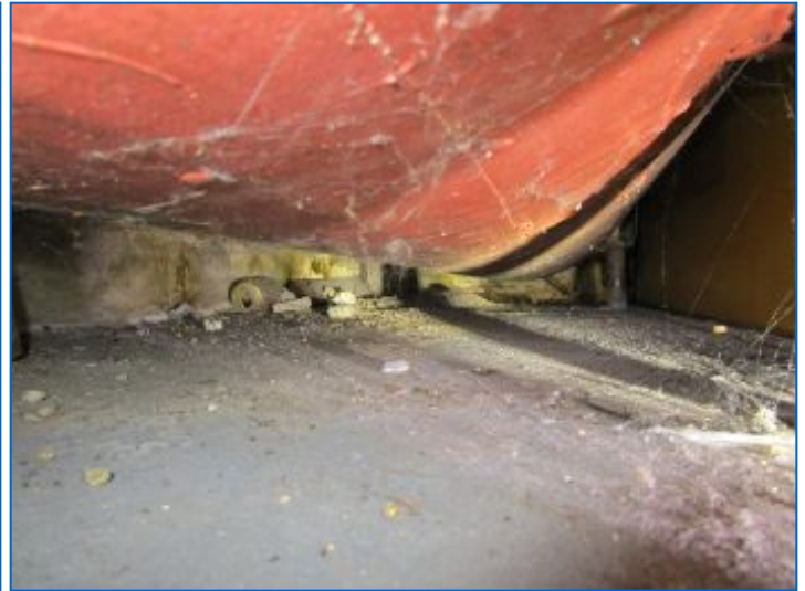
Oil tank showed no apparent signs of leakage at the visible portions of tank at time of inspection.
