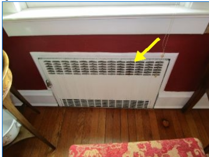
Heat distribution type/s included Radiators (cast iron).
