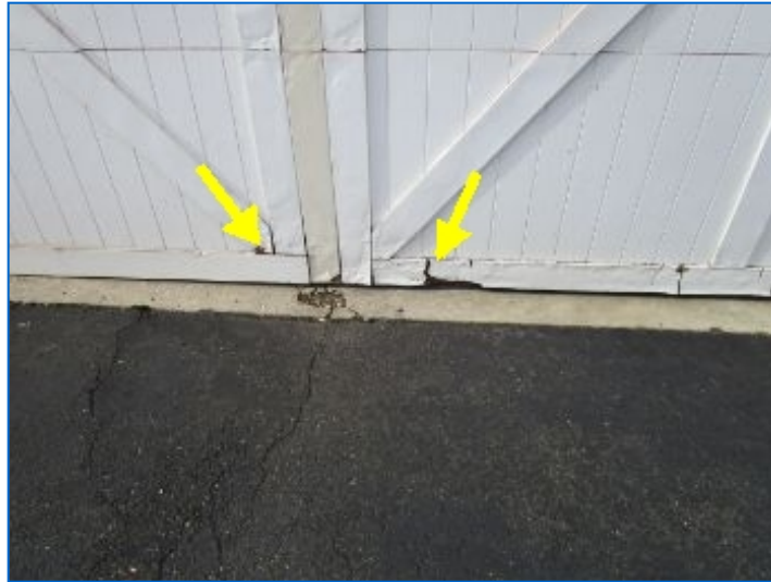
Rotted wood at bottom of sectional roll-up door. Recommend repairing damaged areas.
