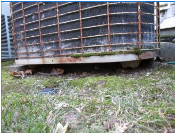
AC#2 Outdoor condenser coil aluminum fins were bent and dirty; this will reduce performance and efficiency of the system. A qualified HVAC professional can comb fins straight and clean coil to improve A/C system performance and efficiency.
