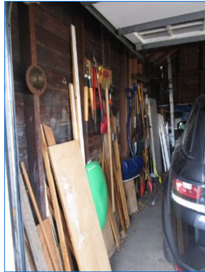
Limitation: Shelving & stored items limited visual access of garage walls/structure; unable to fully inspect.
