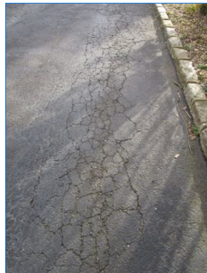
The asphalt driveway had moderate surface deterioration and displacement. The Inspector recommends that before the expiration of your Inspection Objection Deadline you consult with a qualified contractor to discuss options and costs for repair or replacement.
