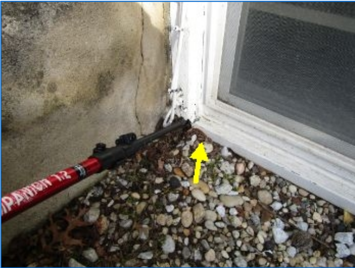
Basement window wood frames in contact with soil showed signs of moisture damage at South side. Recommend lowering soil level 6 inches below wood frames and provide top layer of gravel.
