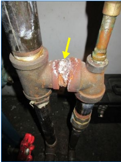
Deposits observed at heating pipe fittings; a sign of past leakage.
