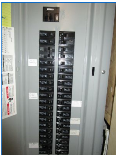
Main Panel: 40 circuit breaker spaces; 0 spare breaker space(s) noted.
