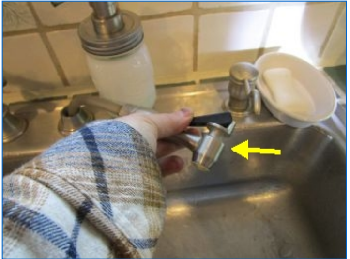
The spray wand at the kitchen sink was inoperable.
