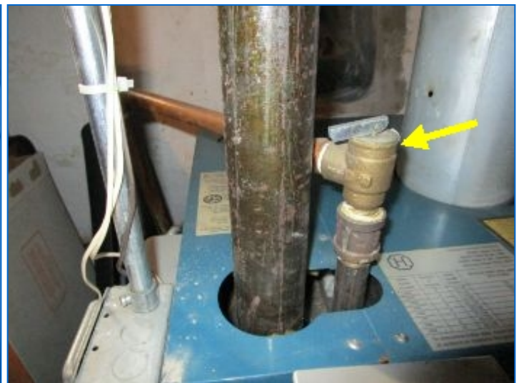
TPR (Temperature Pressure Relief) valve and discharge pipe show no deficiencies.
