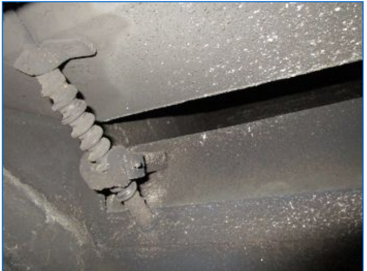
Damper was operable; opened and closed several times.
