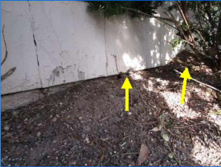
Wood siding covering exterior walls of the home was in contact with soil at front planting bed. This condition will result in deterioration of these areas from wood decay unless these areas are re-graded to provide clearance between wood and soil.
