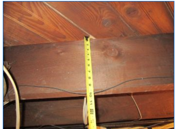
Main Floor Structure: Wood main beam supported by steel lally columns, 2x10 Joists 16" O.C., T&G floor boards.
