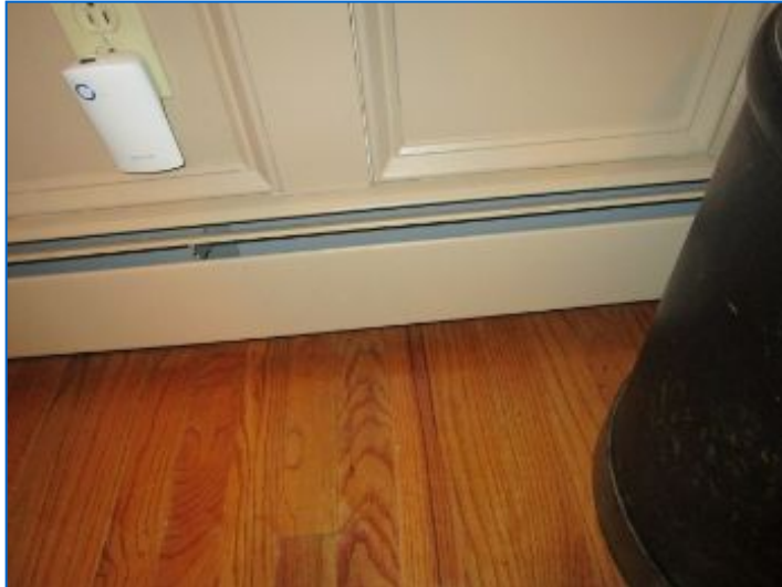
Baseboard convectors noted (hydronic heating zone).
