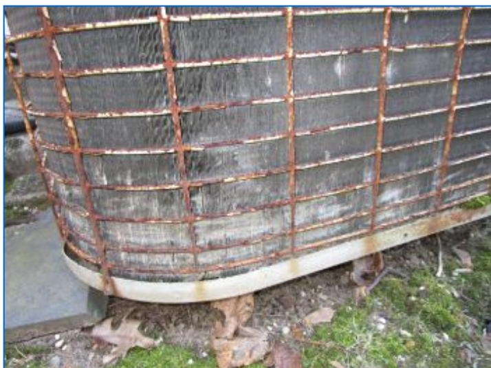
AC#2 Outdoor condenser coil aluminum fins were bent and dirty; this will reduce performance and efficiency of the system. A qualified HVAC professional can comb fins straight and clean coil to improve A/C system performance and efficiency.
