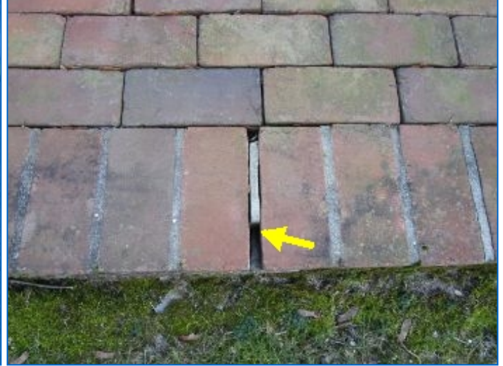
Patio was in functional condition. Minor mortar repairs suggested at border brick.
