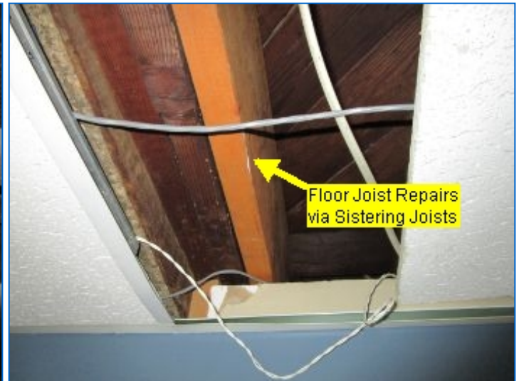
Signs of past termite damage was observed at floor joists, band joist and blocking above basement office at south wall above office in basement. Floor joist repairs were noted (2 places). Refer to NPMA-33 Report.
