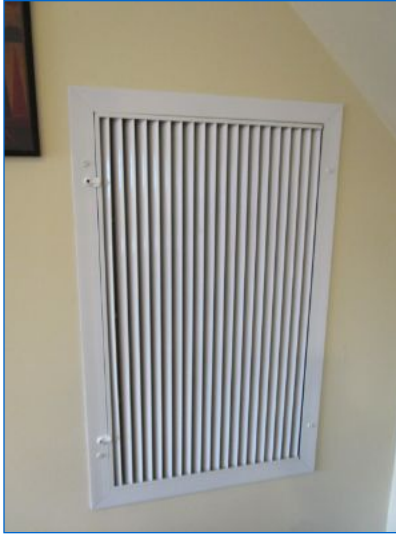
AC#3: Disposable filter located in filter-grille at Attic wall.
