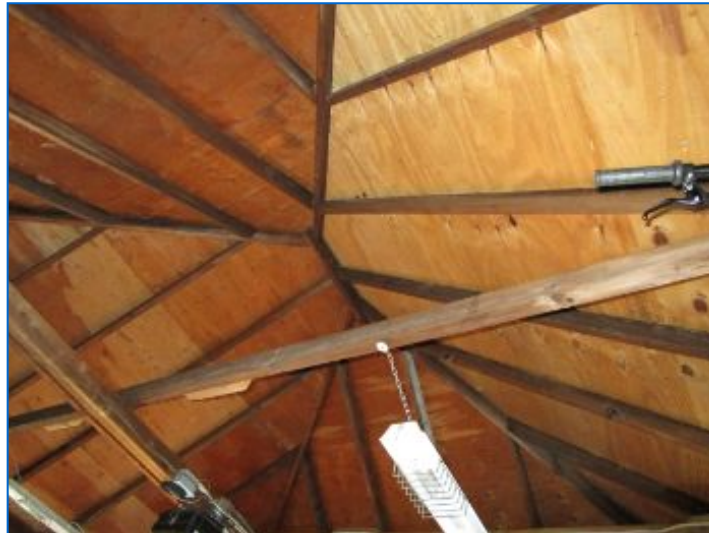
Garage roof boards were apparently replaced when the roof shingles were replaced.
