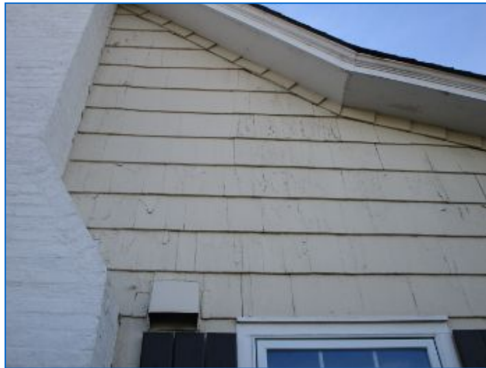
Wood siding covering the exterior walls of the home had areas of peeling paint revealing the white paint layer beneath. Paint should be maintained in good condition to help prevent damage to wood siding from sun and moisture. The Inspector suggests that before the expiration of your Inspection Objection Deadline you consult with a qualified contractor to gain an idea of options and costs for repainting.
