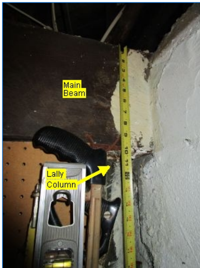
Main Floor Structure: Wood main beam supported by steel lally columns, 2x10 Joists 16" O.C., T&G floor boards.
