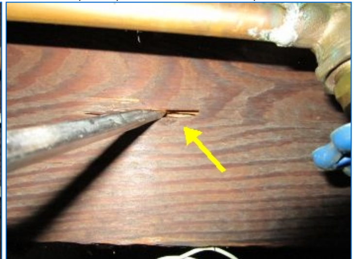
Signs of past termite damage was observed at floor joists, band joist and blocking above basement office at south wall above office in basement. Floor joist repairs were noted (2 places). Refer to NPMA-33 Report.
