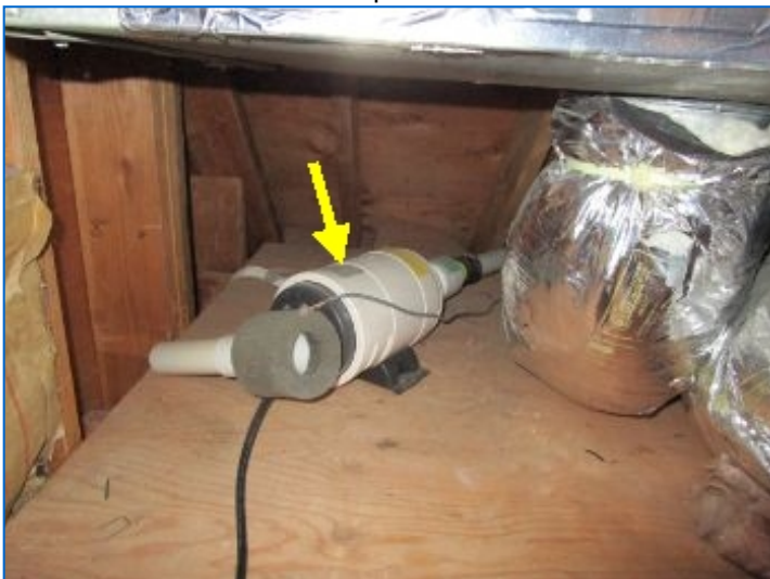
Air pump located in attic eave space; for master bath whirlpool.
