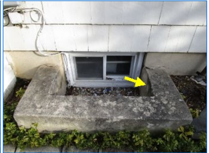
Poured concrete window wells noted at south side. Suggest covers or steel grates for small child fall protection.
