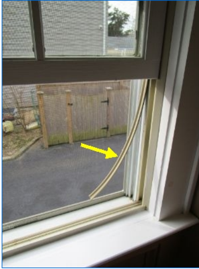
Weather stripping detached at double-hung window.
