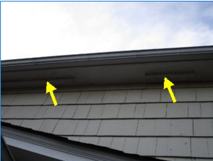
Under eave soffit inlet vents noted for attic ventilation.
