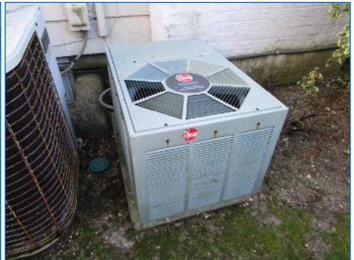
AC#3 Condenser; corresponding Air Handler located in the Attic serves a portion of the home. Refer to Thermostat section.
