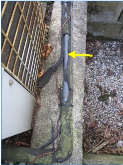
AC#2 outdoor refrigerant pipe insulation was deteriorated/missing at outdoor condenser. Recommend replacing outdoor deteriorated/missing insulation for the larger suction line.
