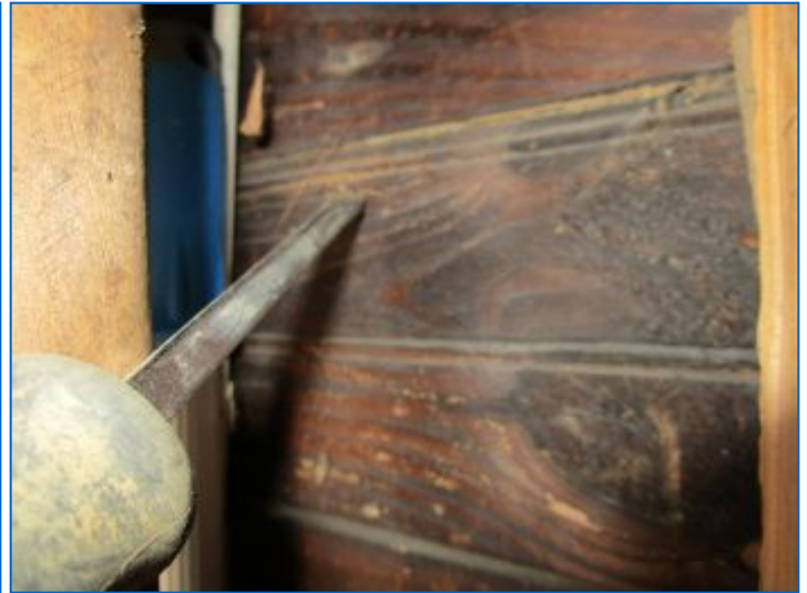
Past Termite damage observed at wall boards at North and South front areas of garage.
