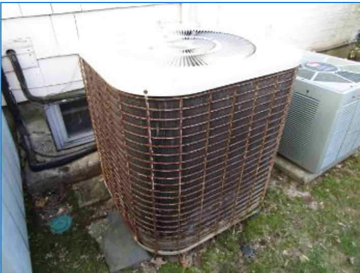
AC#2 Condenser; corresponding Air Handler located in the Attic serves a portion of the home. Refer to Thermostat section.
