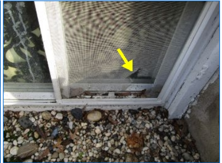
Torn screen noted at south basement window.
