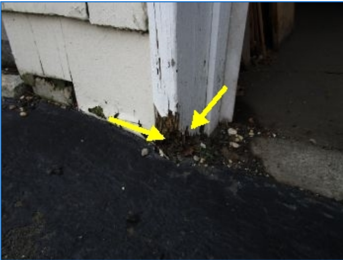
Vehicle door Jamb/s deteriorated (water damage).
