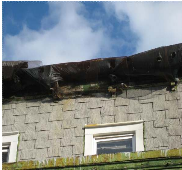
IMG_2466.JPG Rear facias and soffits at roof levels are deteriorated with some of the old-style architectural cornices missing and damaged.
