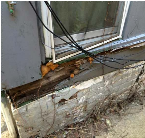
IMG_0866.JPG Wood trim at rear windows is badly deteriorated.
