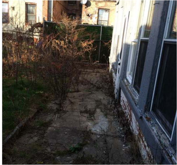
IMG_0896.JPG Backyard concrete area is cracked.
