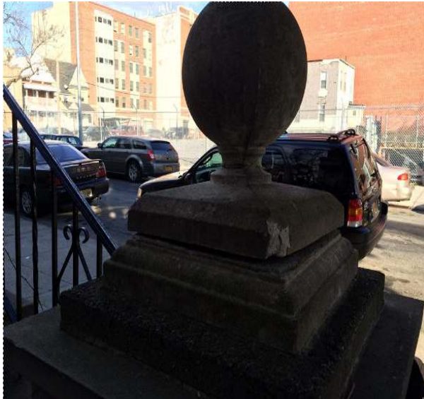
IMG_0849.JPG Concrete ball ornament on masonry column in front yard is loose and can fall.
