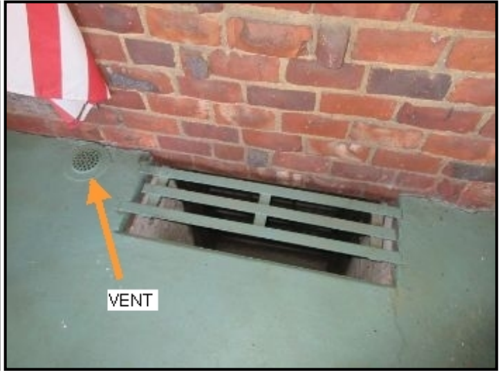
Waste Pipe Exit located at the rear of the house. Whole-house trap with vent connection at basement north wall.
