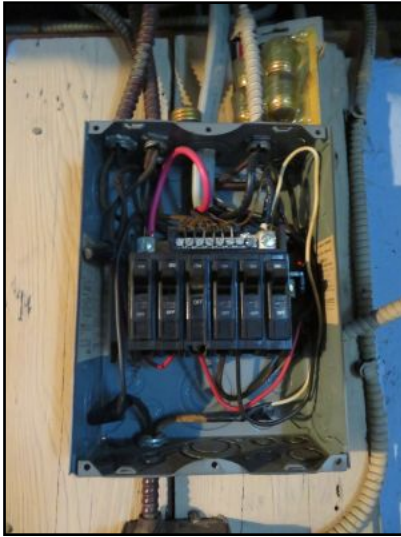
No major system safety or function concerns noted at time of inspection at sub panel box.
