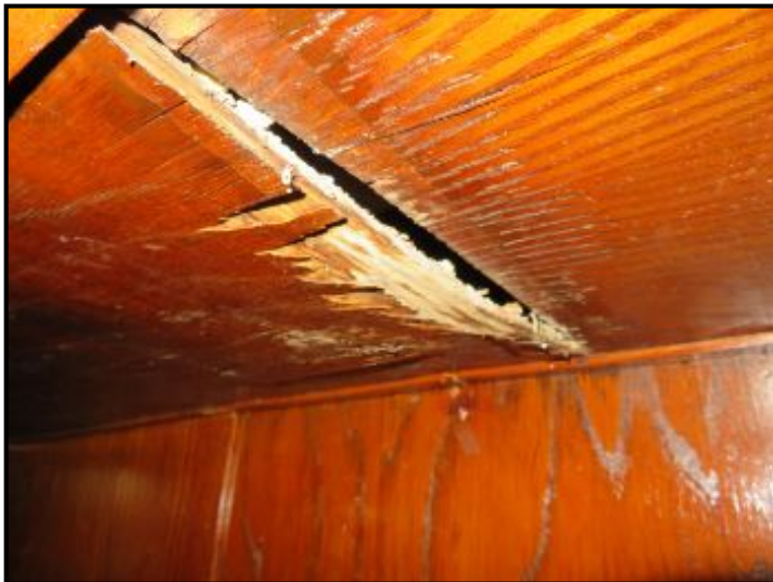
Water damage observed at basement ceiling caused by either past plumbing leaks. Suggest monitoring for recurrence and repair as necessary.
