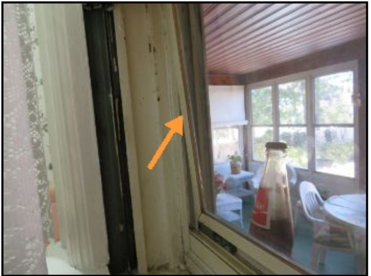
Outer window sash off track.
