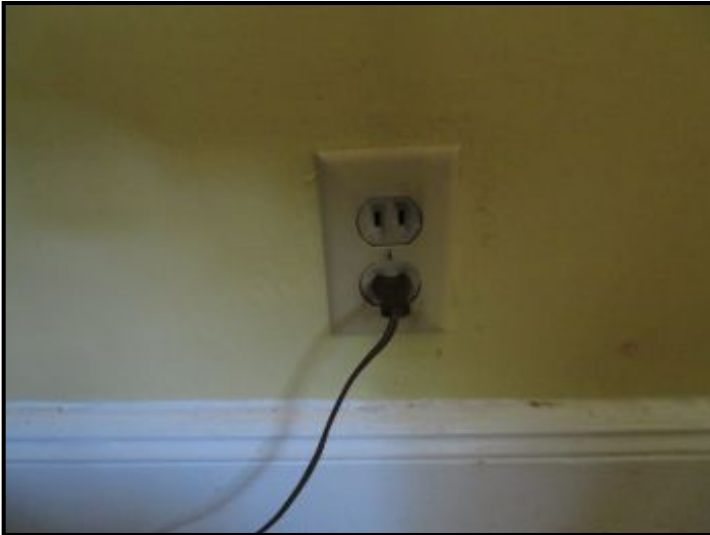
Existing electrical outlets are the older ungrounded 2-prong type. Suggest electrician install grounded 3-prong outlets.
