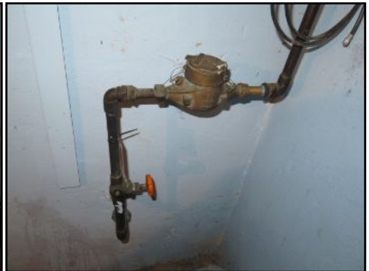
Water Service Entrance: 3/4" Lead pipe, meter and shut-off valves. Recommend having licensed electrician ensure that proper ground is installed.
