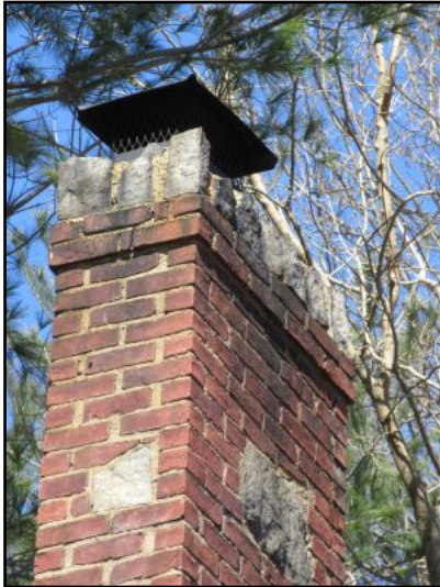
Combined fireplace and furnace chimney brick enclosure noted.
