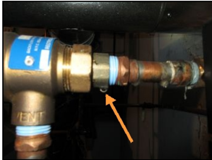
Drip leak observed at boiler check valve connection. Repair needed.
