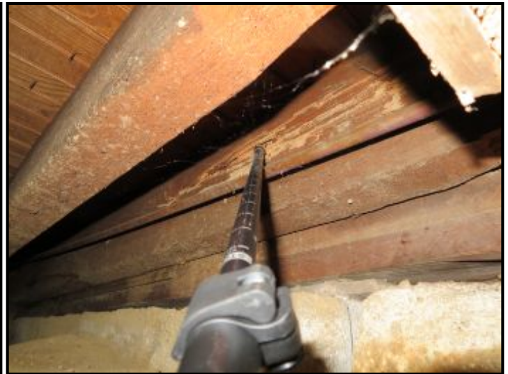
Extensive termite damage and activity noted at joists in crawlspace along east foundation wall.
