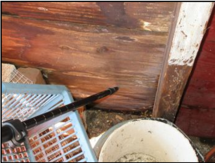
Decay of wall boards and studs noted.
