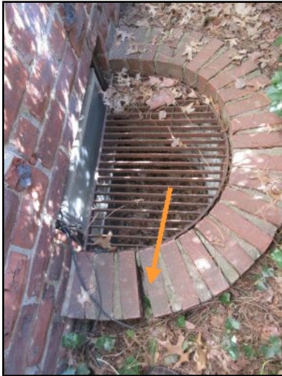
Mortar damage noted at window wells. Repair and ensure gratings are secure.
