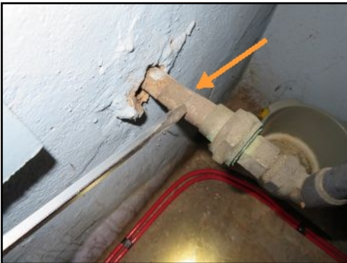
Water Service Entrance: 3/4" Lead pipe noted.
