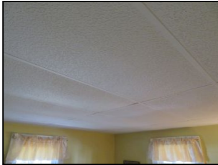
Hung ceiling noted in sitting room
