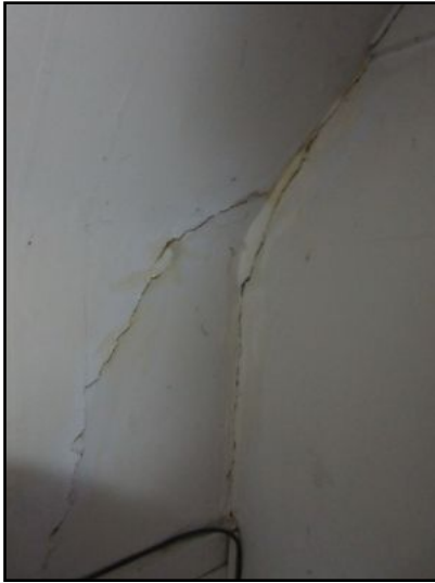
Cosmetic damage in west bedroom closet caused by structural settlement and subsequent neglect.
