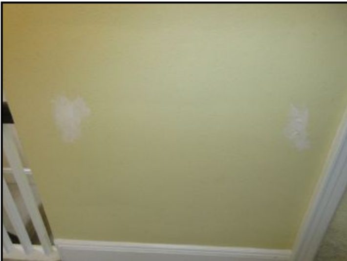
Unfinished wall repairs observed at stairway walls.
