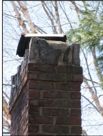
Boiler chimney flue liner was not visually accessible. Recommend chimney contractor check to see if a s.s. chimney liner was installed at time of the boiler update. Combined chimney requires a flue liner for boiler. Chimney crown cement not visible from ground. Suggest chimney contractor inspect further to ensure there's no water intrusion here.
