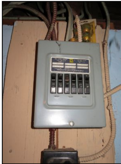
Sub Panel in Boiler Room.
