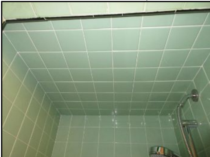
Light needed in stall shower.
