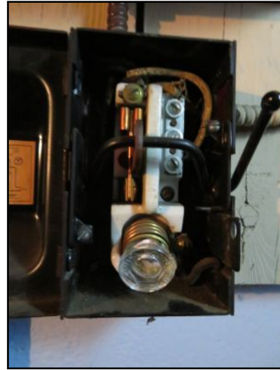
Old type fused disconnect switch noted.
