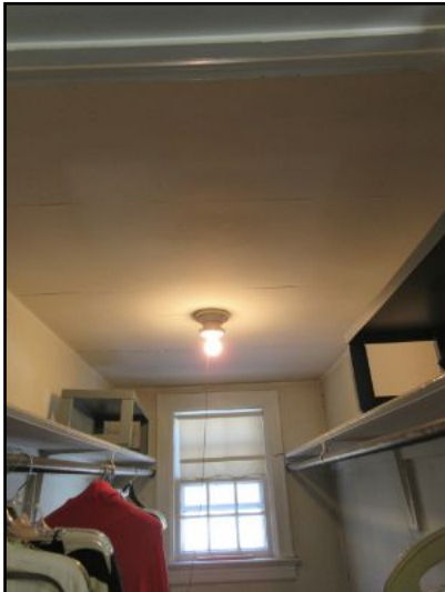
Wall paper painted over at walk-in closet.
