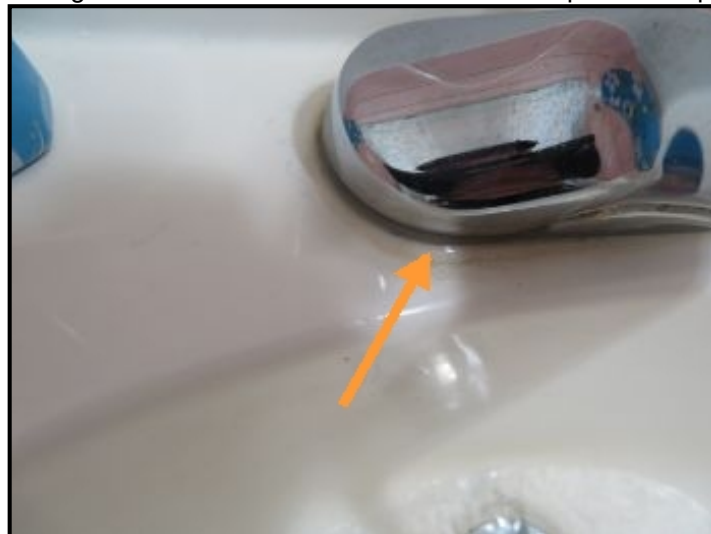
Sink faucet leaks at base; recommend faucet repair or replacement.
