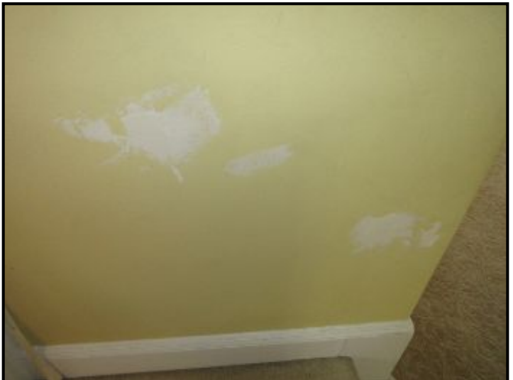
Unfinished wall repairs observed at stairway walls.
