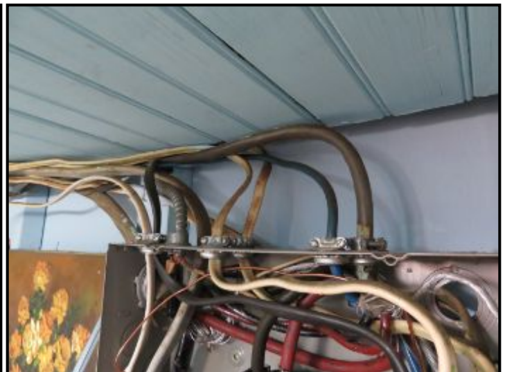
Various wire types noted
