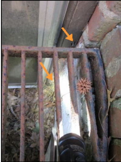
Deterioration of wooden frames noted. In the inspectors opinion the windows/frames are near the end of their useful life.
