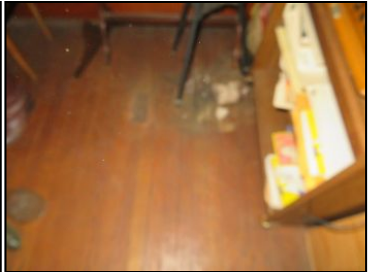
Basement hardwood floor showed signs of past water damage.
