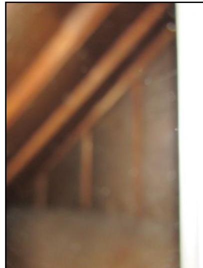
Installed in rafter cavities. Loose fill insulation noted.
