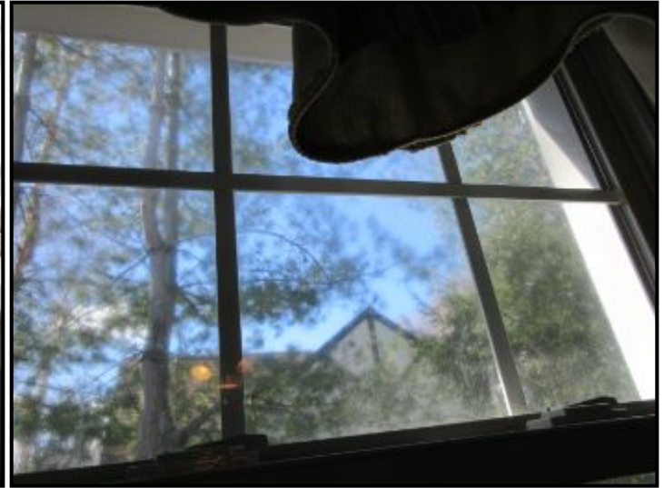
Fog/condensation observed in thermopane window at west bedroom. This is an indication of a failed seal. Recommend review for repair or replacement as necessary.
