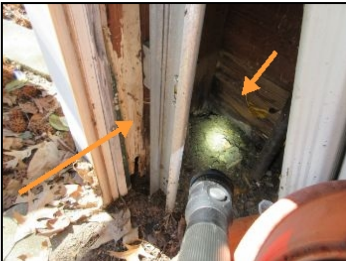
Termite damage noted at garage door jamb. Refer to NPMA-33 report form.
