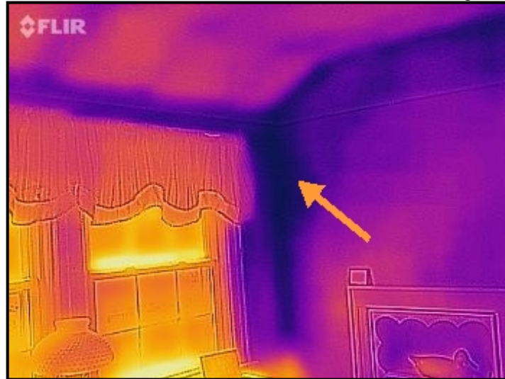
Deficient insulation noted at west bedroom corner wall.
