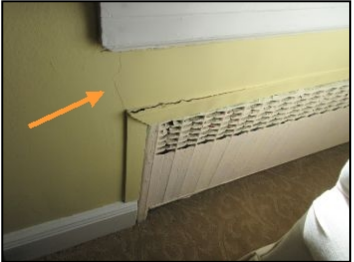
Signs of past water penetration/damage at living room window below window.
