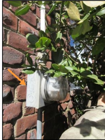
Meter box and riser not properly attached to the house. Recommend licensed electrician to repair.
