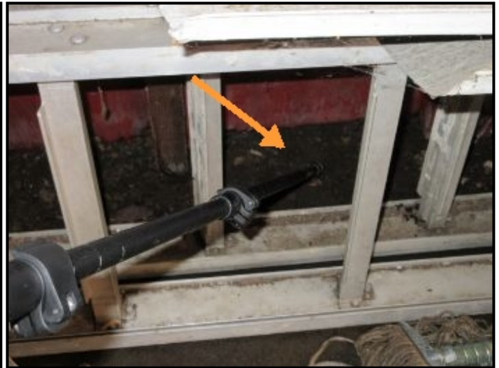
Wood to soil contact at east wall is an invitation to termites.
