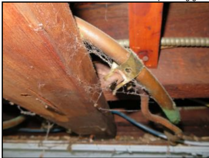
Water piping in laundry room grounding observed. Recommend having licensed electrician ensure that proper plumbing grounding is installed.
