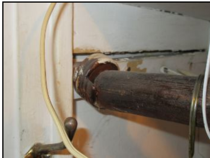
Older clothes hanger rod not long enough; possible wall movement had occurred from structural settlement.
