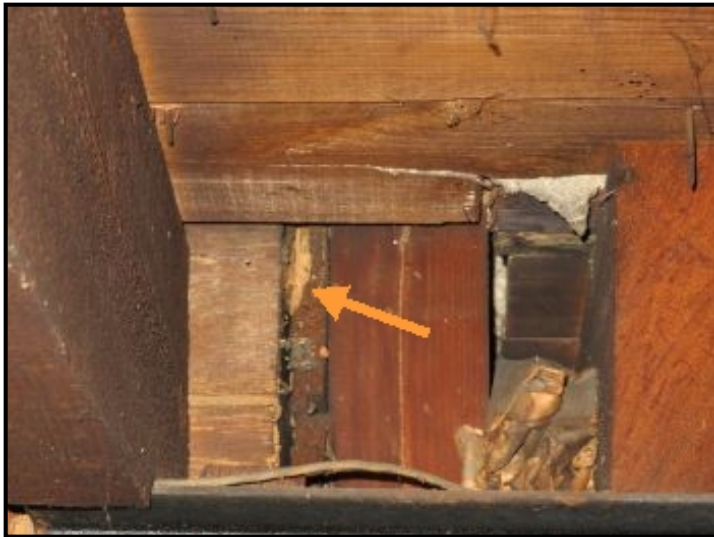
Termite damage noted at vertical studs located in boiler room at north foundation walls. Refer to NPMA-33 report.
