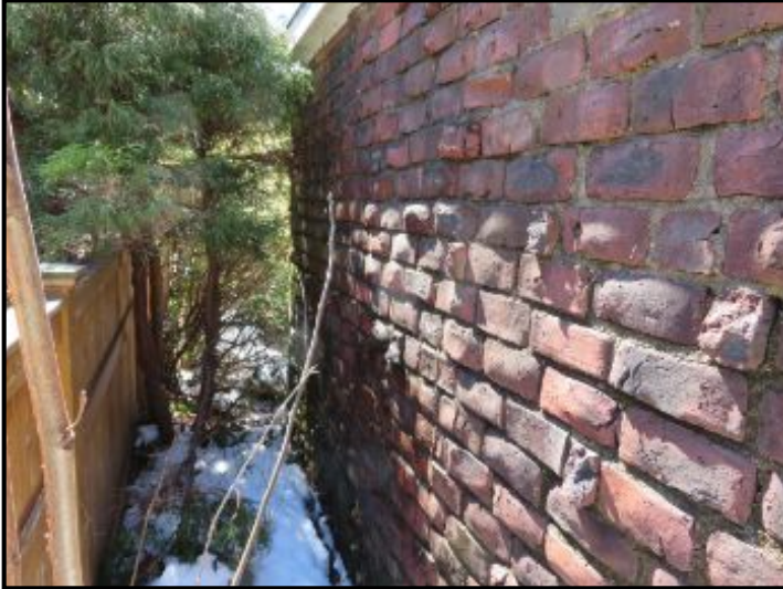
Distorted bricks observed at garage walls.
