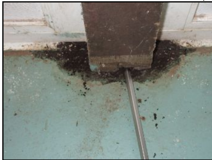
Water damage at base of porch roof posts (2 plcs). Recommend replacing decayed wood.
