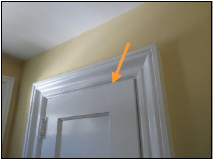
Door binds against frame; Does not close properly.
