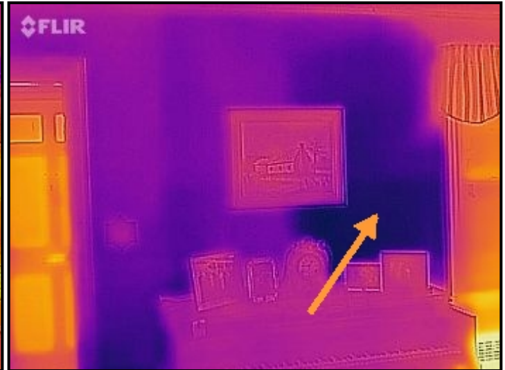
Darker (cooler) area at living room south wall indicates a lack of insulation. Suggest adding blown-in loose fill type insulation.
