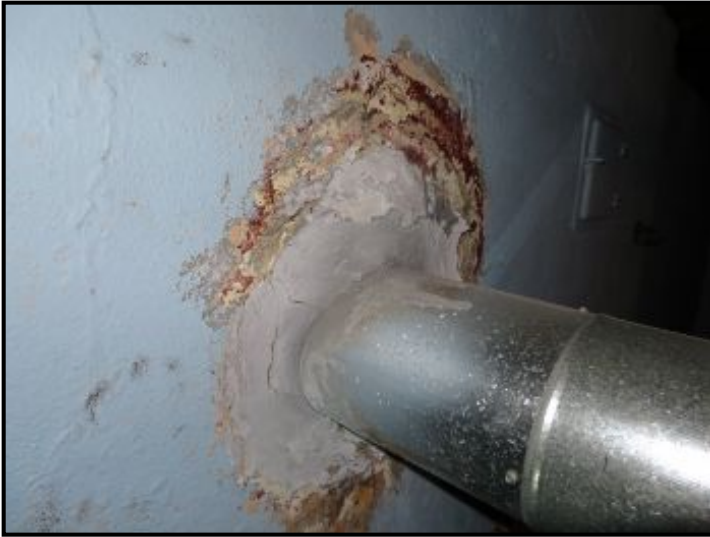
Maintain sealed connection between equipment vent pipe and chimney wall.
