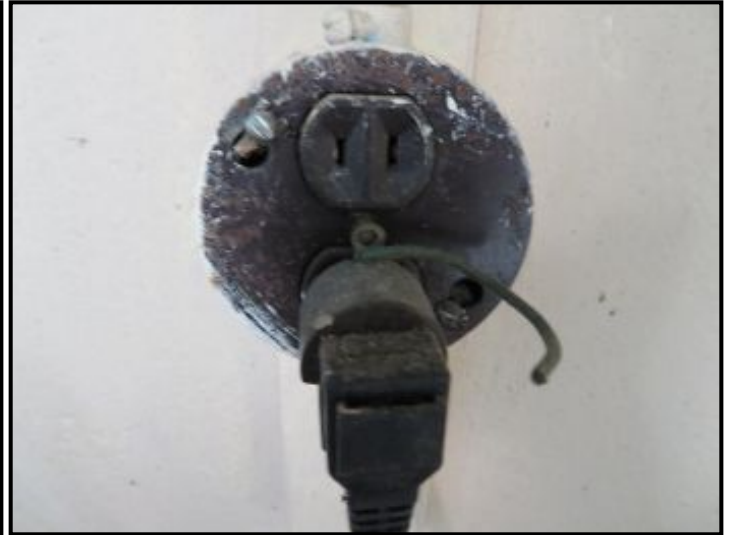
Laundry receptacle is not GFCI protected. Refer to Electrical section.
