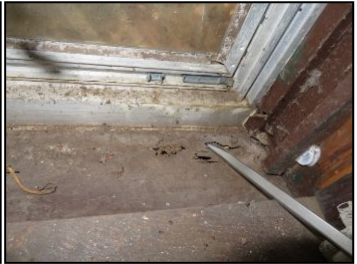
Deterioration of wooden sills and frames noted. Replacement may be necessary at some point.
