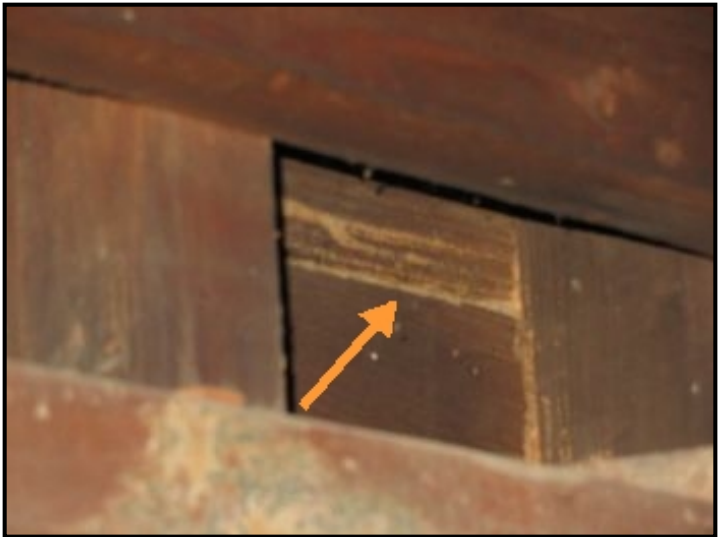
Termite damage and activity noted at west wall in boiler. Refer to NPMA-33 report form.
