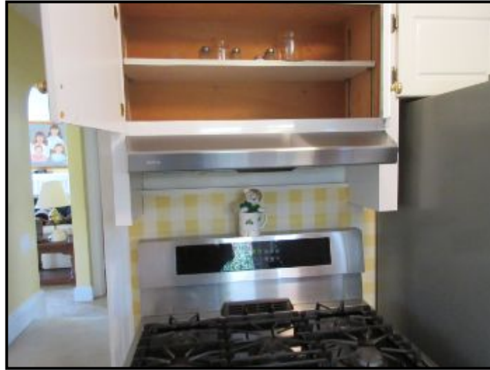
Exterior vented fan is recommended where gas appliances are in place.
