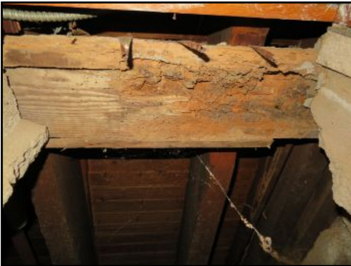
Termite damage and activity noted at crawlspace accessway.
