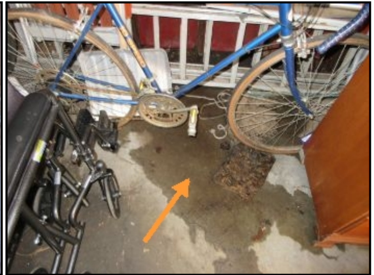
Standing water observed near east wall from snow melting alongside of garage.
