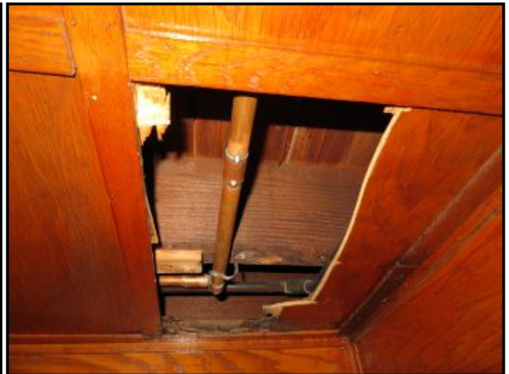
Access to utilities above basement ceiling is limited.
