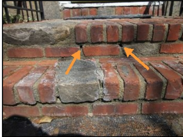
Some repointing needed.
