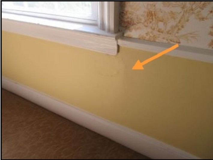
Signs of past water penetration/damage at dining room window below window.
