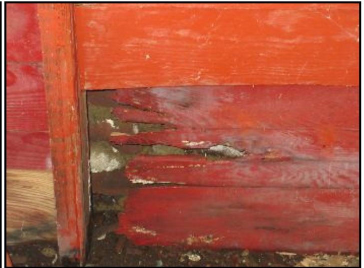
Extensive decay of wall boards and studs noted.
