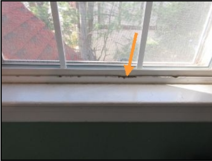
Newer vinyl window in west bedroom room appears to have been gnawed away at sill frame.
