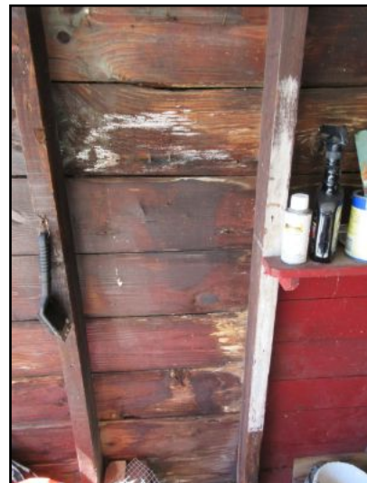
Extensive decay of wall boards noted.
