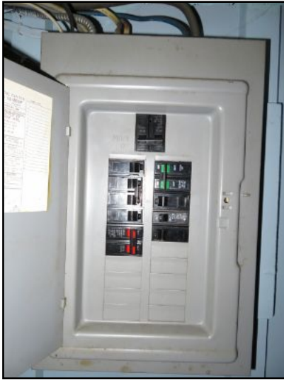
Main Panel in Basement laundry room.
