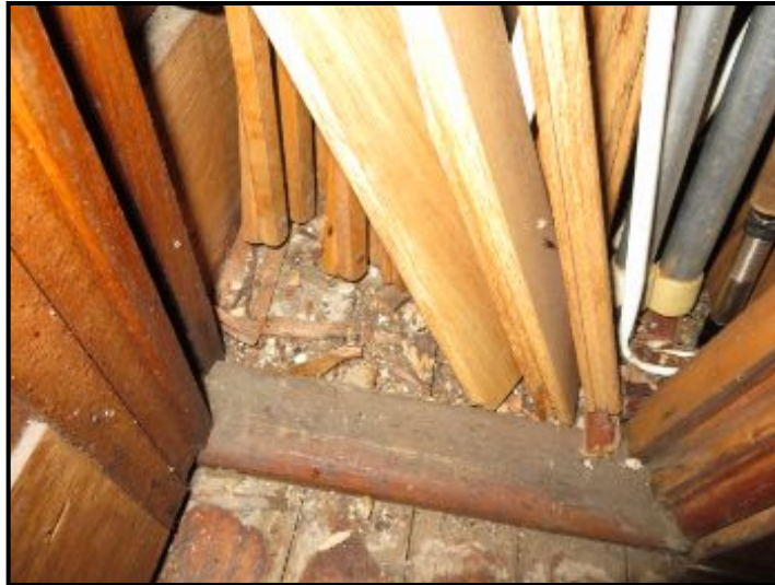
Evidence of past water penetration observed.
