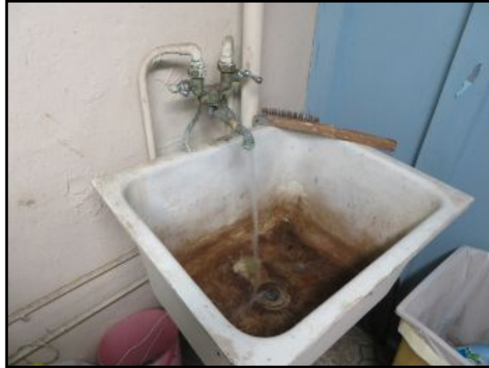
Slop sink in laundry room
