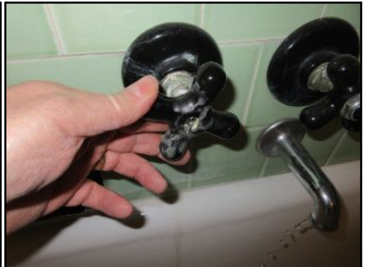
Tub hot water valve handle stripped; could not test hot water at tub.
