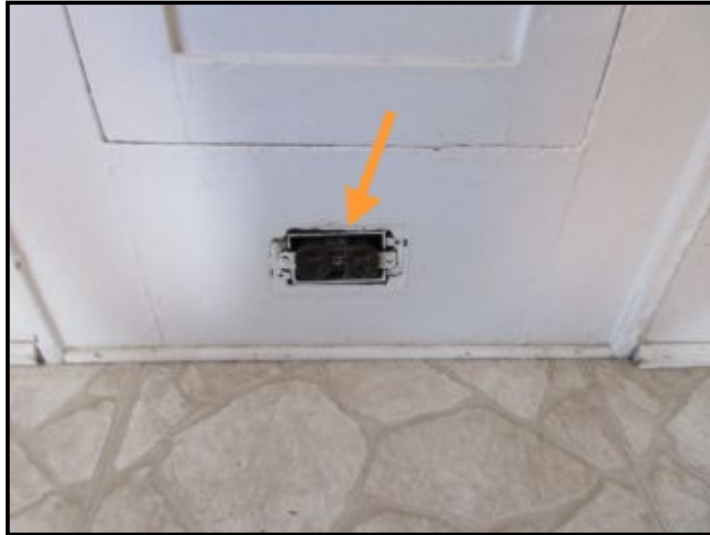
Cover plate missing. Provide missing receptacle and switch cover plates.
