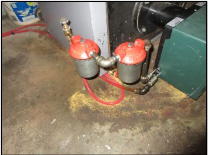
Oil shut-off valve and filters noted at burner.
