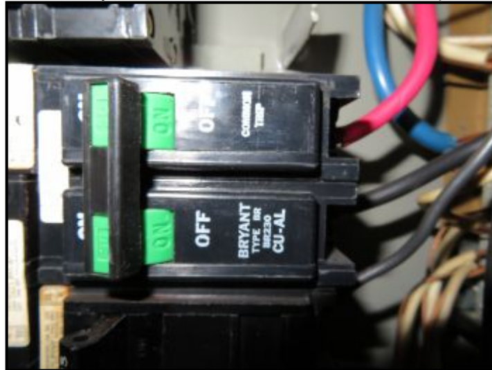
Sub Panel Supply: 30 amp breaker supplies sub panel located in boiler room.
