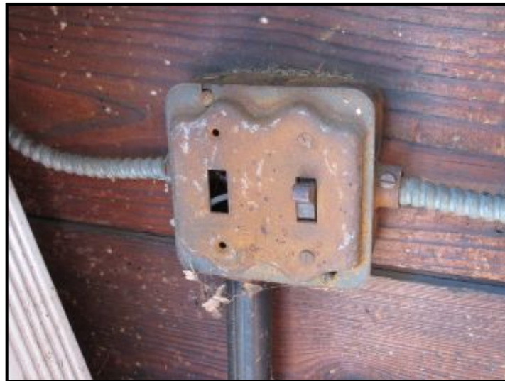
Light switch missing/inoperable.
