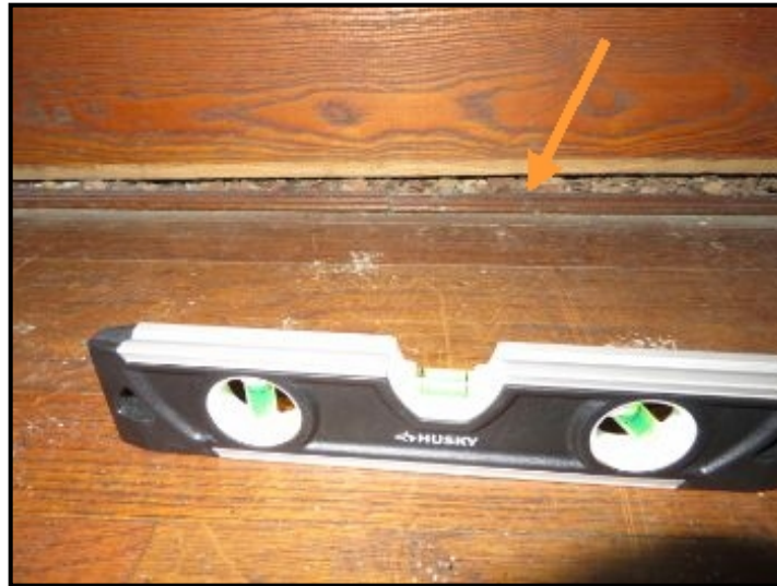
Basement hardwood floor depression; signs of deterioration at south exterior wall.
