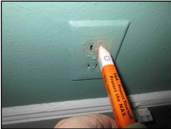
Power noted at 2 prong outlets.
