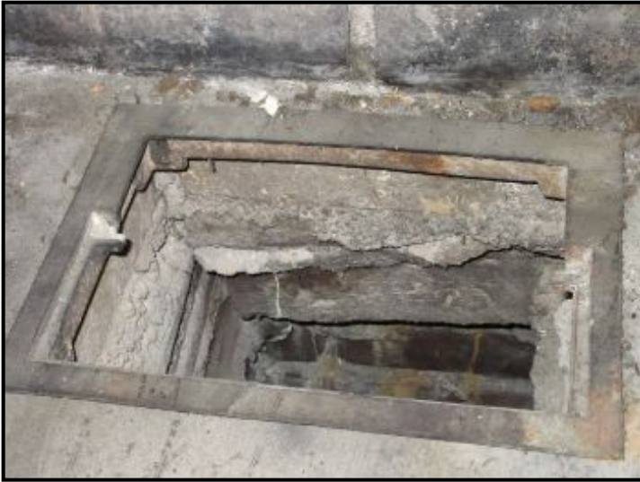
Proper ash dump door was missing. Suggest replacement.
