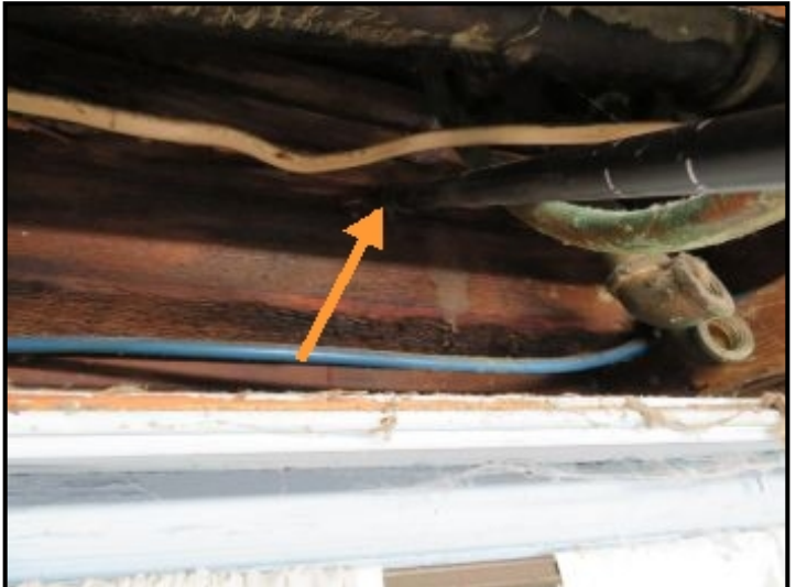
Extensive termite damage noted at joists and sill plate in laundry and crawlspace along east foundation wall.
