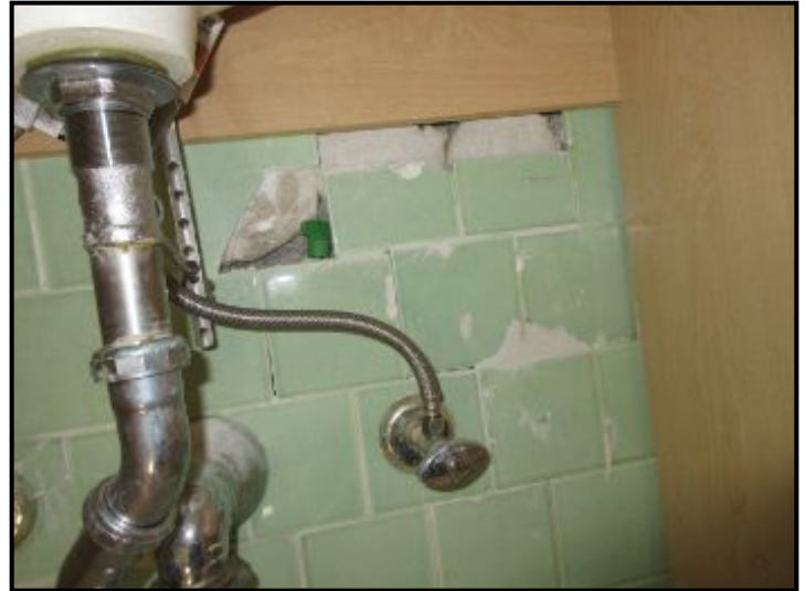
Wall tile damaged/missing below sink; suggest repair(s).
