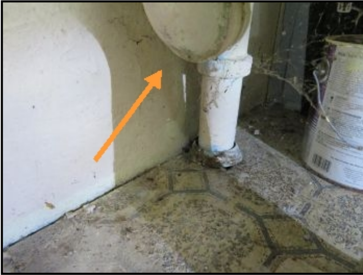
Visible leaking under the slop sink. Source of existing leak(s) could not be determined; suggest Plumber to evaluate and repair.
