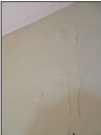
Sitting room wall damage believed to be from past water/plumbing leak.
