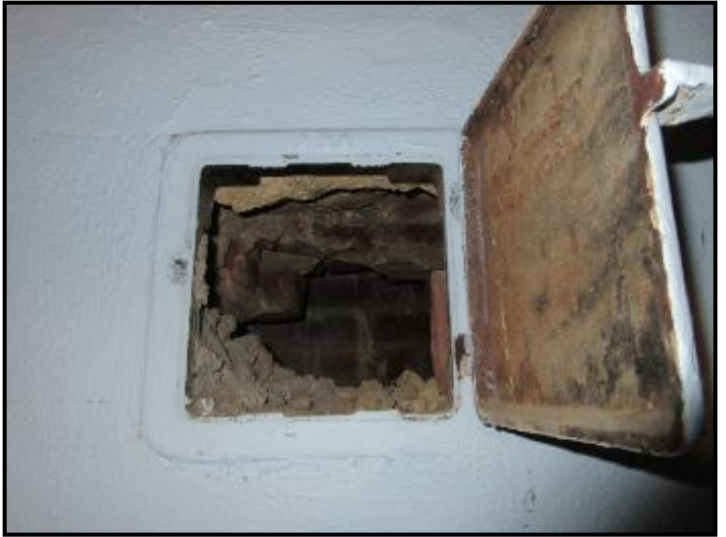
Fireplace clean-out door in boiler room.
