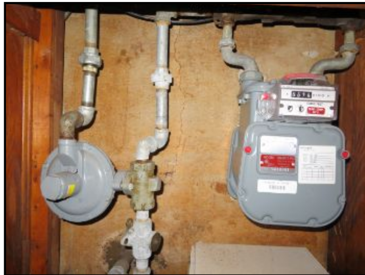
Public Gas Service: Meter, shutoff valve and vented regulator noted in basement. Gas supply presently used for cooking only.
