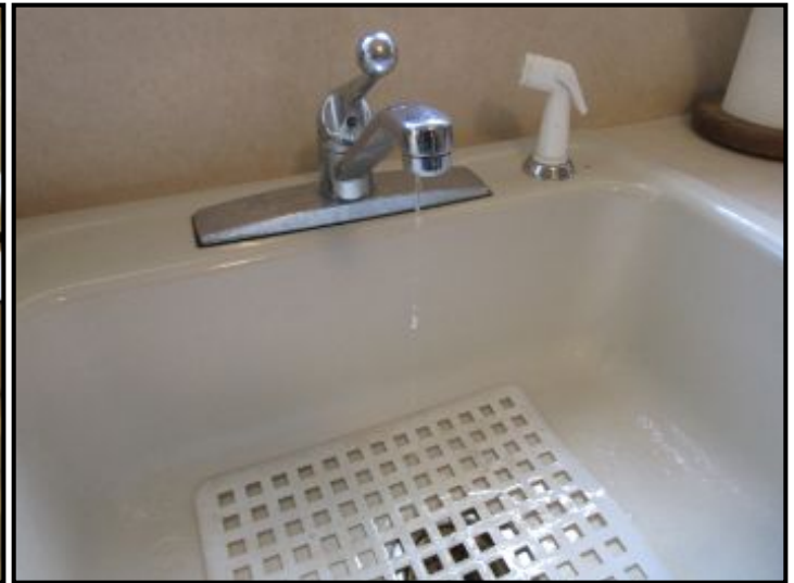
Kitchen faucet spout leaked. Recommend repair or replacement.
