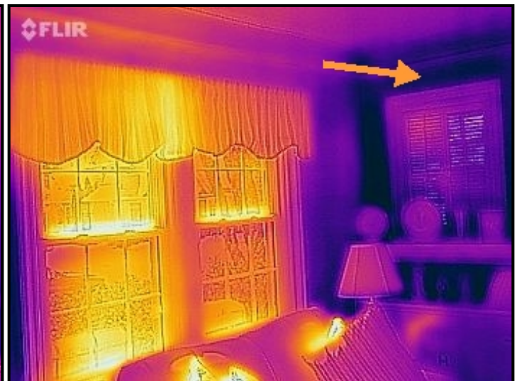
Darker (cooler) area at living room west wall around window indicates a lack of insulation and window infiltration. Suggest updating original windows, adding insulation to wall and window frame.
