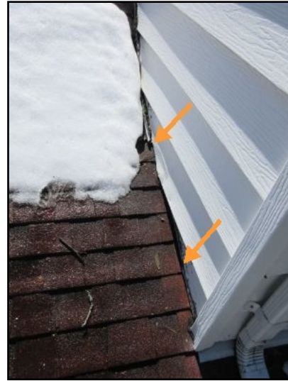
J-channel missing at east side of lower part of dormer.
