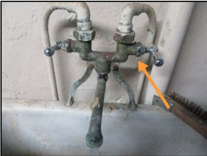
Slop Sink faucet leaks at handle; recommend faucet repair or replacement.
