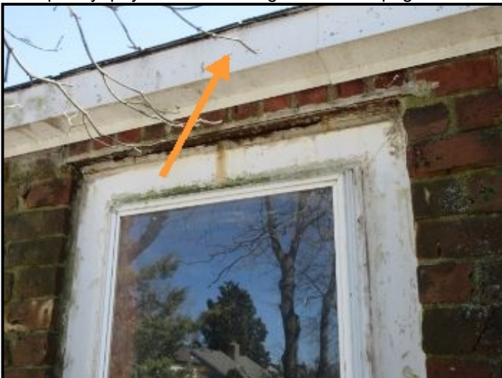
Garage roof gutters and downspouts missing. Recommend adding these to direct water away from the foundation and prevent water intrusion.
