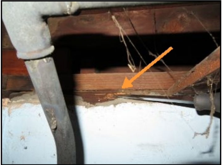
Extensive termite damage noted at sill plate in laundry along east foundation wall.
