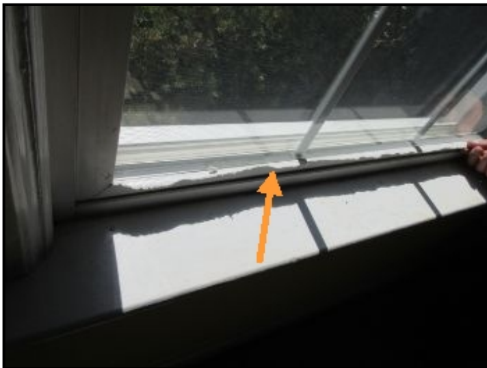
Newer vinyl window in dining room appears to have been gnawed away at bottom of sash.
