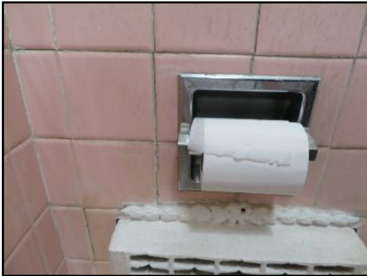
Wall tile grout missing.
