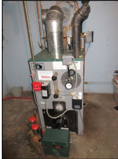
Peerless Oil-fired Cast Iron Forced Hot Water Boiler with integral Tankless Domestic Water Heater.
