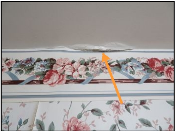
Defects noted at ceiling/walls suspected to be caused by past water/plumbing leaks.
