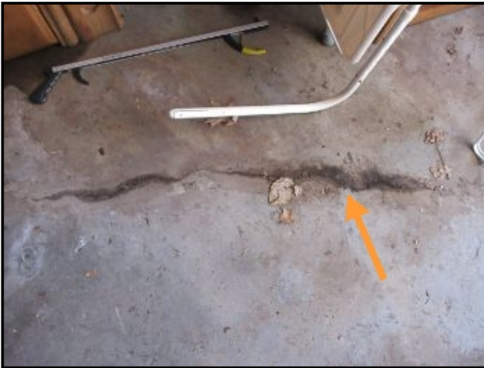
Water seepage up through floor crack noted.
