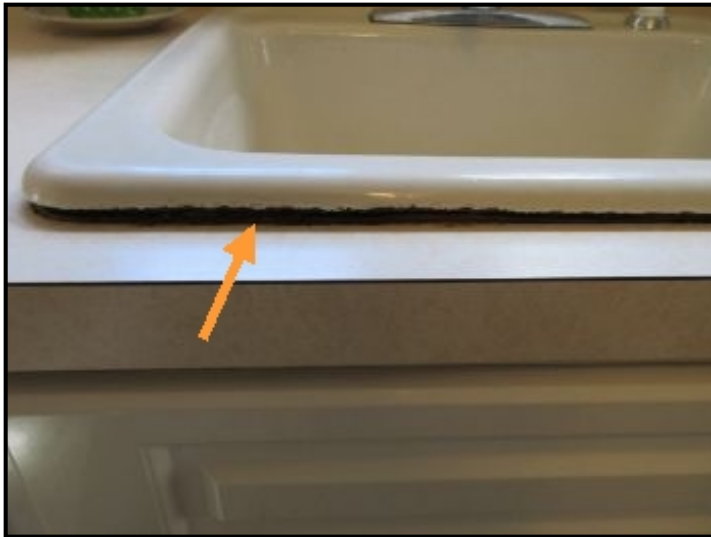
Rust noted at ceramic sink base.
