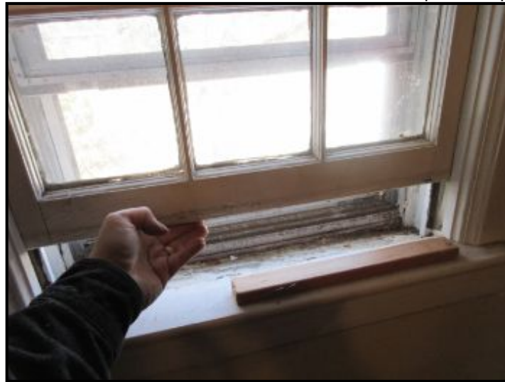
Broken sash wire/cord observed on window frame. This is a "Safety Concern". Sash wire/cord holds window in open position. Suggest repairs/replacement as needed to ensure safety.
