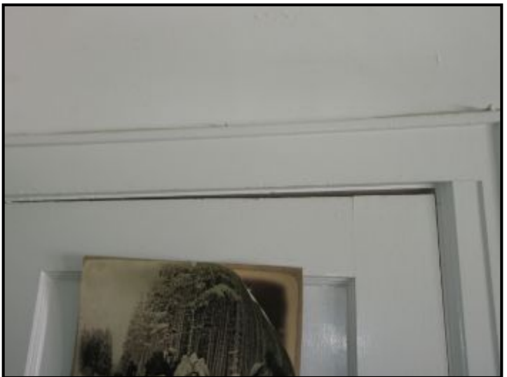
Bedroom door binds against frame; Does not close properly.
