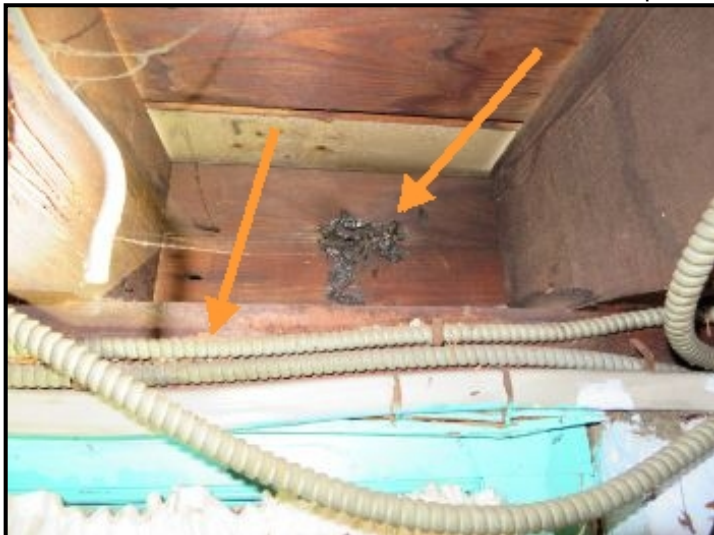
Termite damage noted at band joist and sill plate located in boiler room at south foundation wall.
