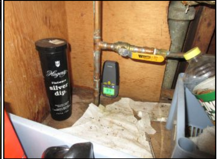
LEAK: Stains at sink cabinet floor, presumably from past leak(s) or spilled products.
