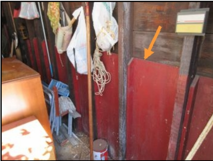
Sections of the wall boards covered over. Although termite activity was not observed here, wood to soil contact at east wall is an invitation to termites. Refer to NPMA-33 report form for treatment recommendation.
