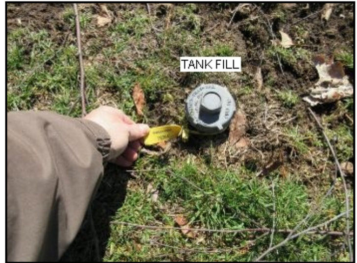
Oil tank Buried underground at the front exterior of the house.
