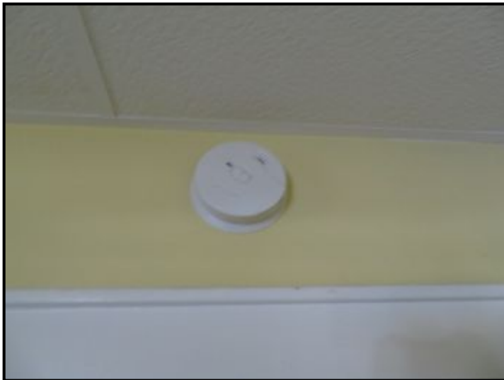
LIFE SAFETY: Maintain functioning Smoke and Carbon Monoxide detectors at each level of the home for Life Safety. Detectors are generally reliable for up to 5 yrs.
