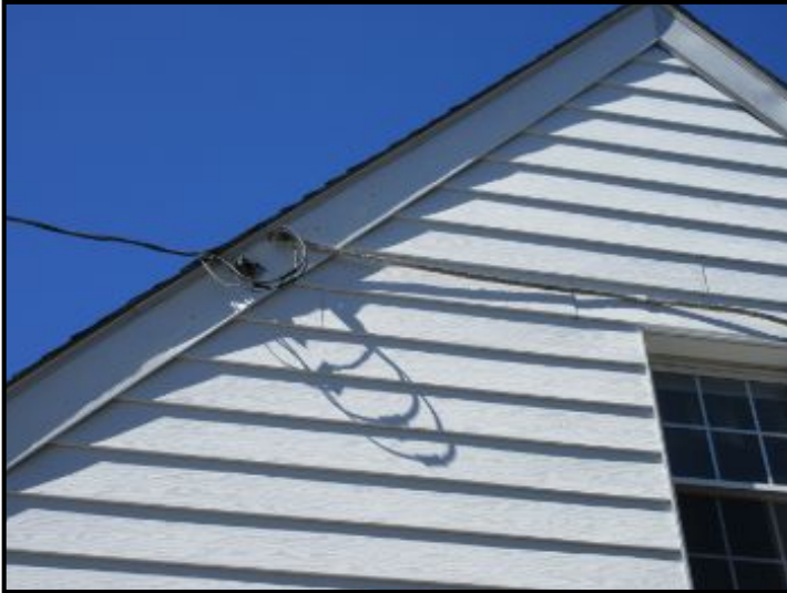
Overhead service drop; 120/240 volts.
