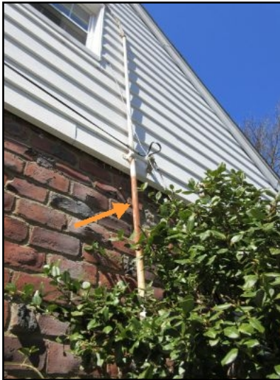
Vegetation contacting electric service meter. Recommend trimming back vegetation.
