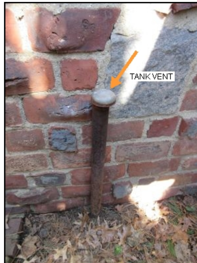
Oil tank Buried underground at the front exterior of the house.
