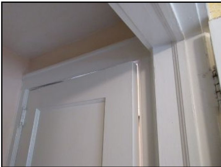
Coat closet door binds against frame; Does not close properly.
