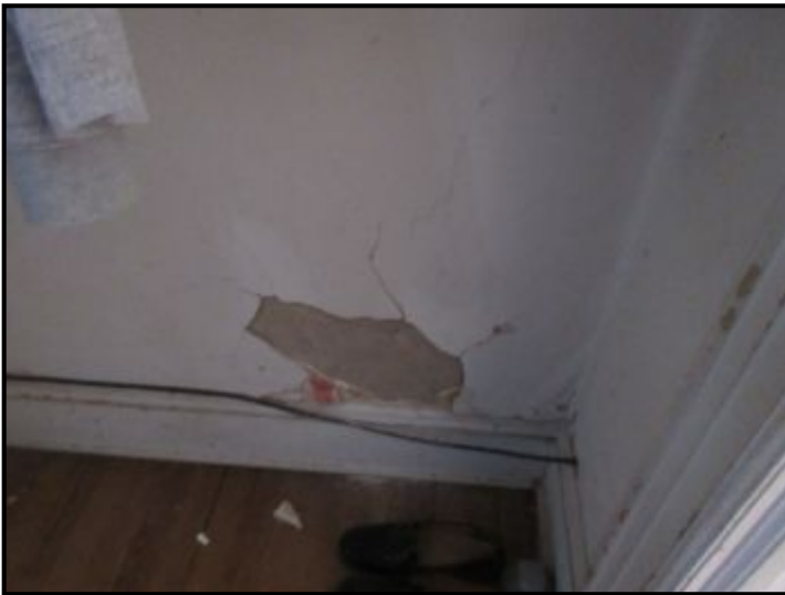
Cosmetic damage in west bedroom closet caused by structural settlement and subsequent neglect.
