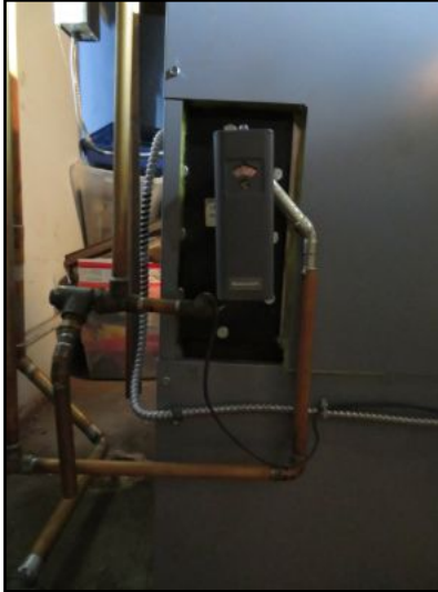
Tankless coil, integral with heating system.
