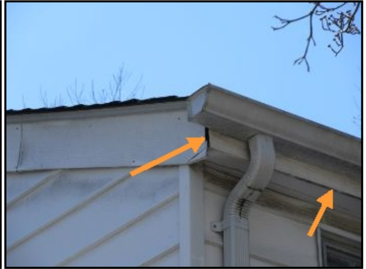
Some defects observed at fascia and soffit aluminum cladding. Suggest repairs to prevent water intrusion.
