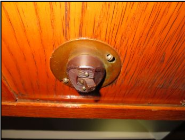
Oil Burner: Remote Emergency Shut-off switch was functional.
