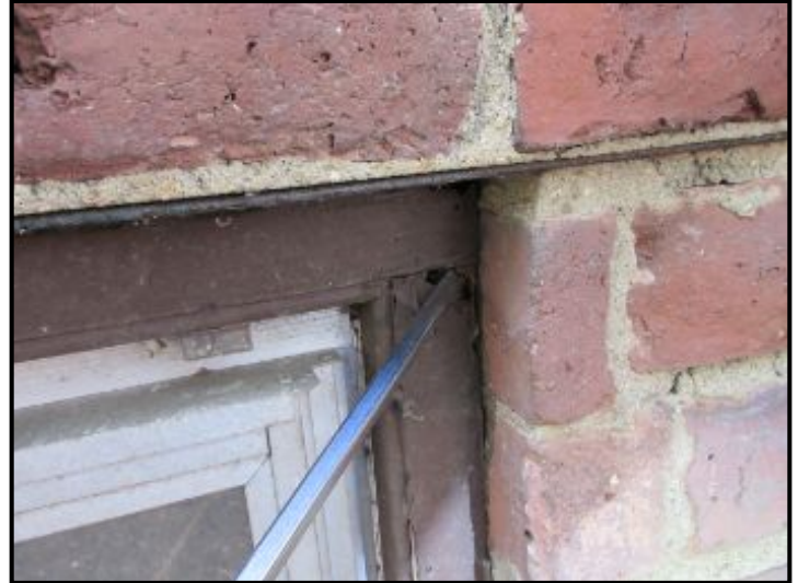
Deterioration of wooden frames noted.
