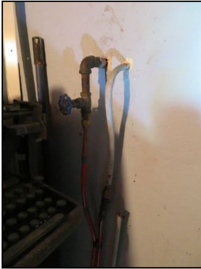
Oil lines to underground fuel storage tank.
