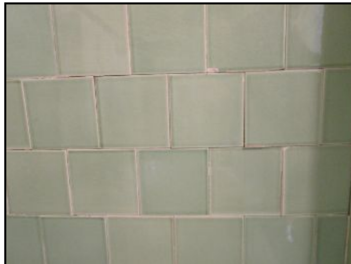
Wall tile grout missing.
