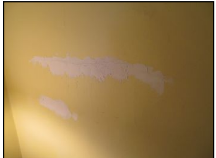
Unfinished wall repairs observed at stairway walls.
