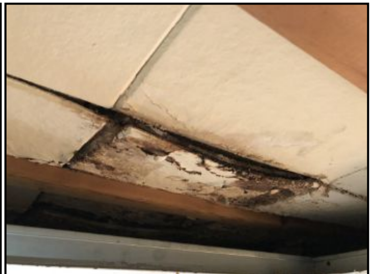
Conditions above hung ceiling in Sitting room show evidence of past plumbing leak. Mold-Like bio-growth observed. Recommend professional testing, evaluation and possible abatement of mold.
