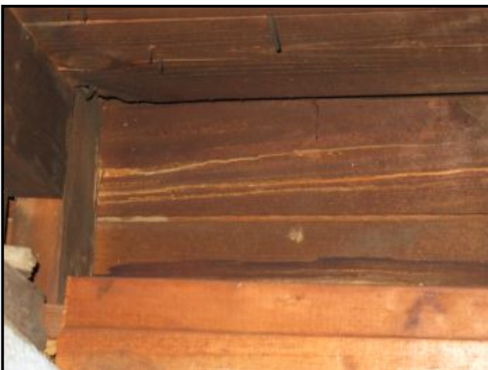
Termite damage noted at band joist, sill plate and vertical studs located in boiler room at north foundation wall. Refer to NPMA-33 report.
