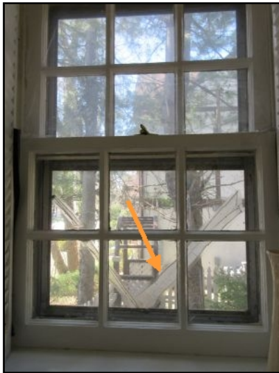
Cracked outer glass pane noted; tape repaired. Recommend proper repair.
