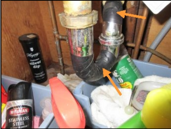
Electric tape used for plumbing repair.
