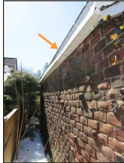
Garage roof gutters and downspouts missing. Recommend adding these to direct water away from the foundation and prevent water intrusion.
