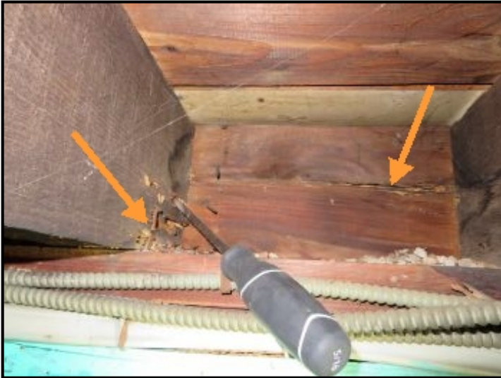
Termite damage noted at joist and sill plate located in boiler room at south foundation wall. Refer to NPMA-33 report.
