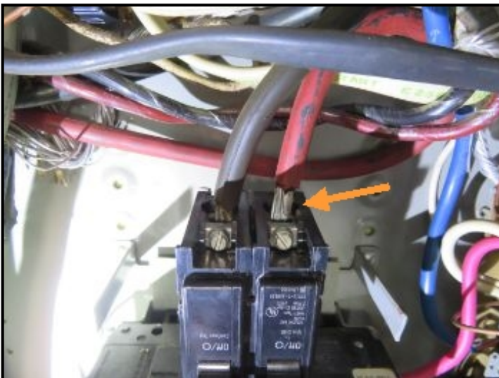
Aluminum non-metallic sheathed cable noted.
