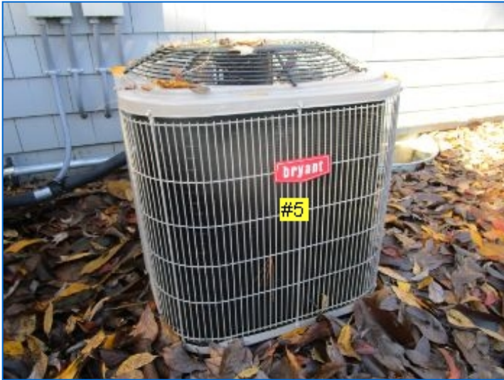
AC#5 Condenser; corresponding ducted air handler located in the Basement.
