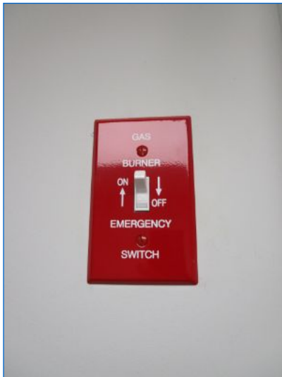
Gas Burner: Remote Emergency Shut-off switch noted.
