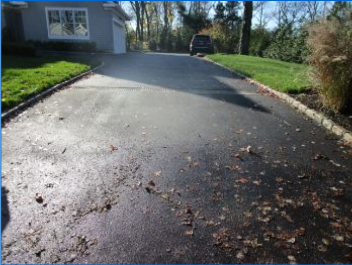
Asphalt driveway appeared new. We recommend sealing within one year to extend life and maintain appearance.
