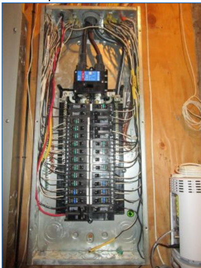
Main panel interiors checked.
