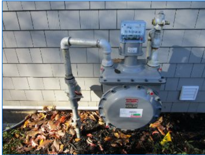
Public Gas Service: Meter w/shutoff valve and vented regulator Outside.
