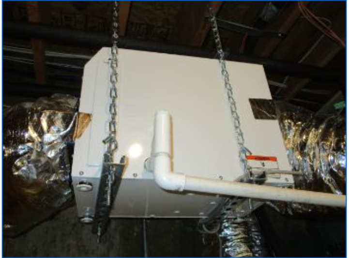
The basement HVAC#1 system was equipped with an operable ducted dehumidifier. Refer to related comment.
