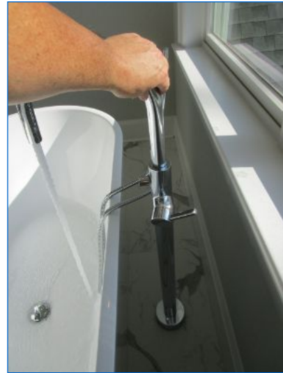
Free-standing floor mounted tub filler was not securely installed at the floor mount. Recommend evaluation and correction by a qualified contractor.
