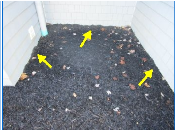
Soil in contact with, and/or in close proximity to siding. This can provide entrance of moisture or insects to siding. The Inspector recommends lowering soil level to 6" below siding.
