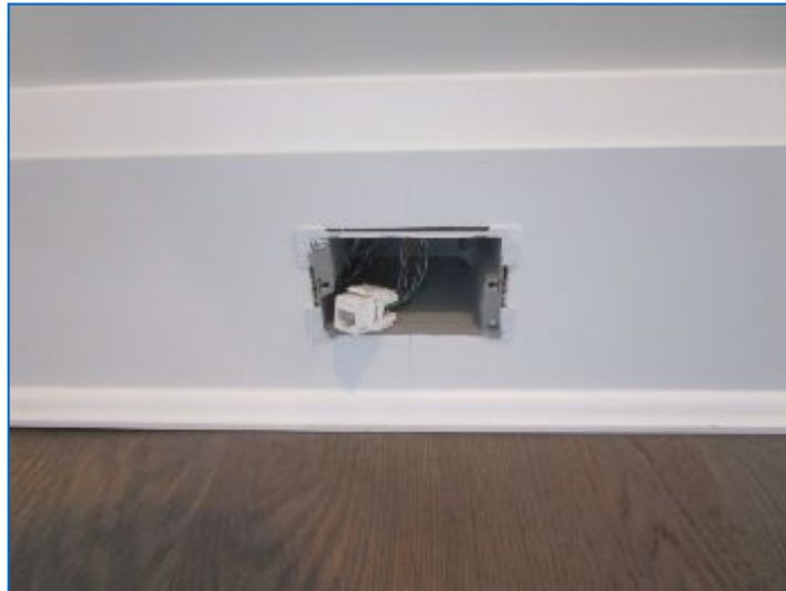
Incomplete data/telecom jack installation noted. Recommend completion and/or finishes prior to close.
