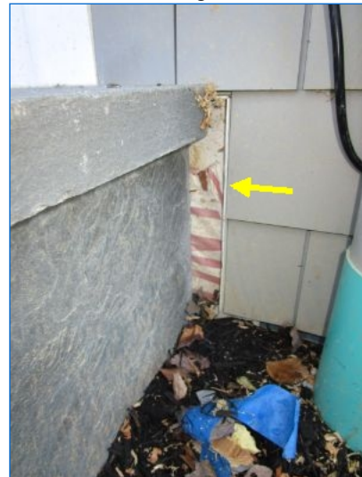
Cedar siding fell short of the steps at the side entrance. Recommend correction by contractor.
