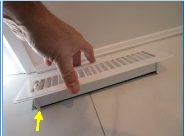
HVAC register not installed; didn't fit floor opening. Recommend completion.
