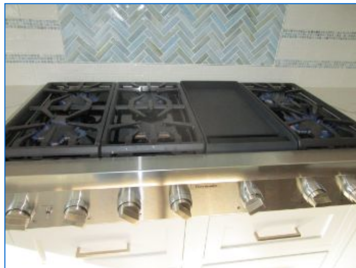
Gas-fired cooktop was operable at time of inspection.
