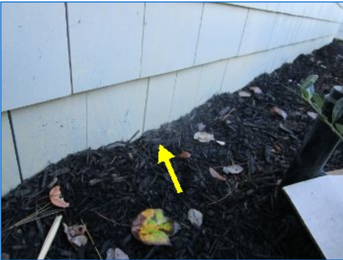
Soil in contact with, and/or in close proximity to siding. This can provide entrance of moisture or insects to siding. The Inspector recommends lowering soil level to 6" below siding.
