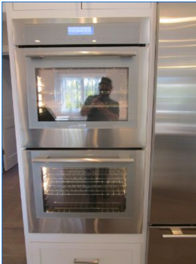
Electric powered built-in double oven; operable. New built-in oven may require initial setup prior to operating elements. Suggest having Seller demonstrate bake/broil modes prior to close.
