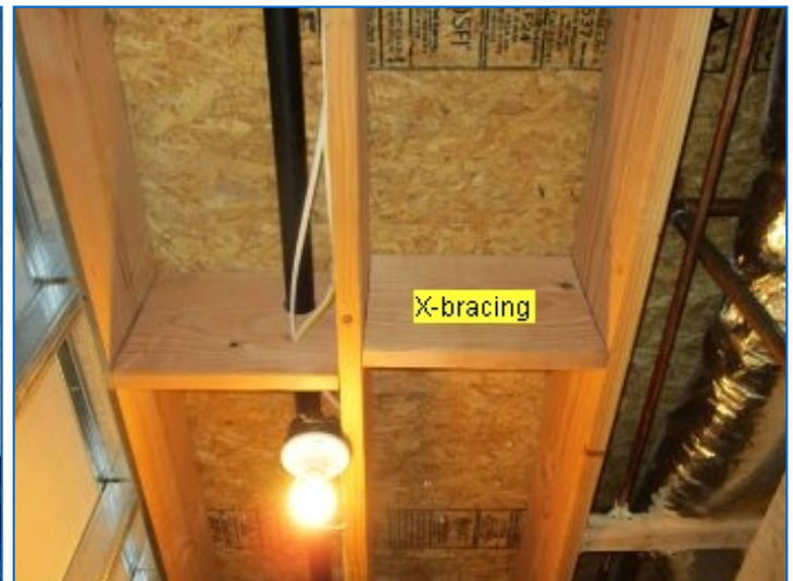
Floor Main Structure: Steel girders supported by steel lally columns, 2x12 Joists 16" O.C. (w/cross braces), Oriented-strand floor boards.
