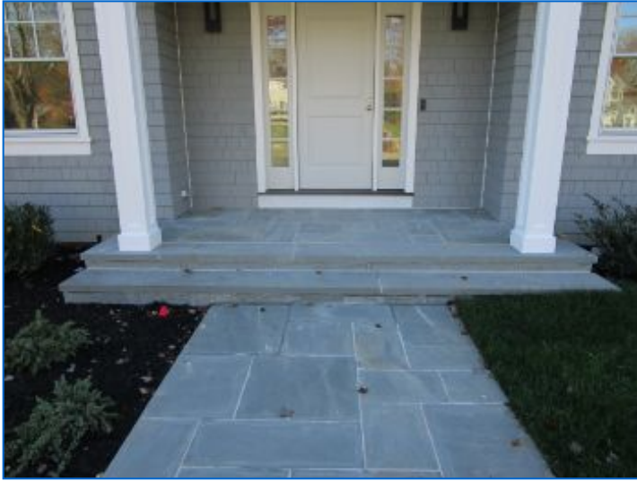
Masonry Steps and Landings noted at Front and side entrances. No system safety or function concerns noted at time of inspection.
