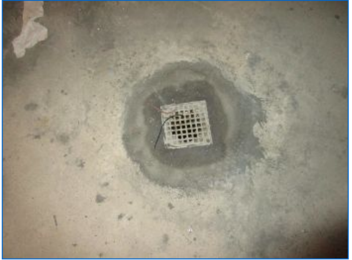
Floor drain observed in boiler room but not tested. Suggest testing for proper operation.
