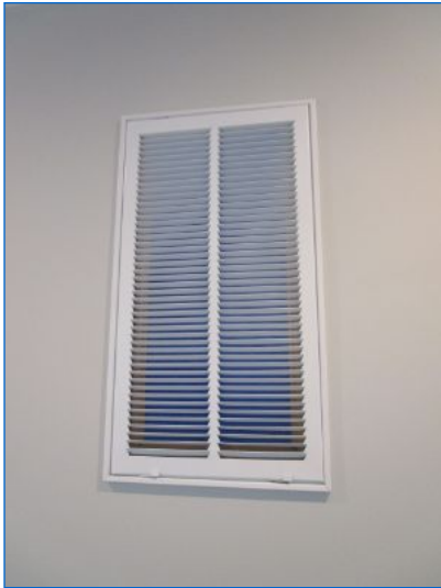
Disposable filters located in filter-grilles at walls in Hallway (1st floor). Two zones noted
