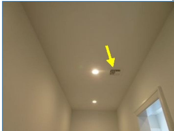
South-side walk-in closet had an HVAC supply register.
