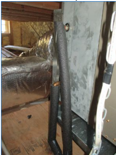
Duct mounted heating coil at HVAC#2.
