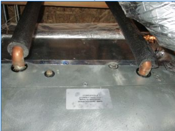
Duct mounted heating coil at HVAC#1.
