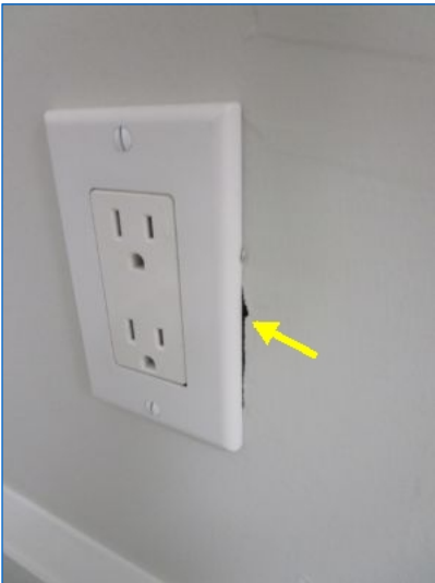
NE corner room: Cosmetic defect noted at outlet.
