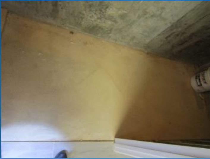
No evidence of moisture intrusion was observed at the visible portions of the concrete floor slab at the time of inspection.
