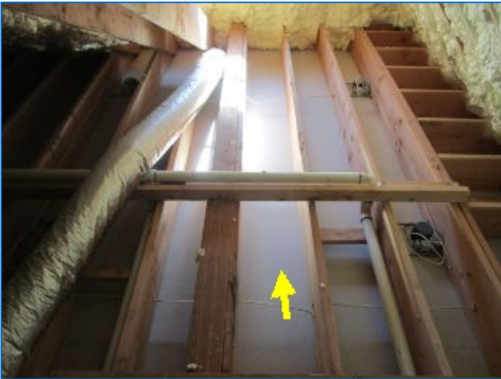
Some floor areas had no floor boards. Suggest adding floor boards for safe access to these areas.
