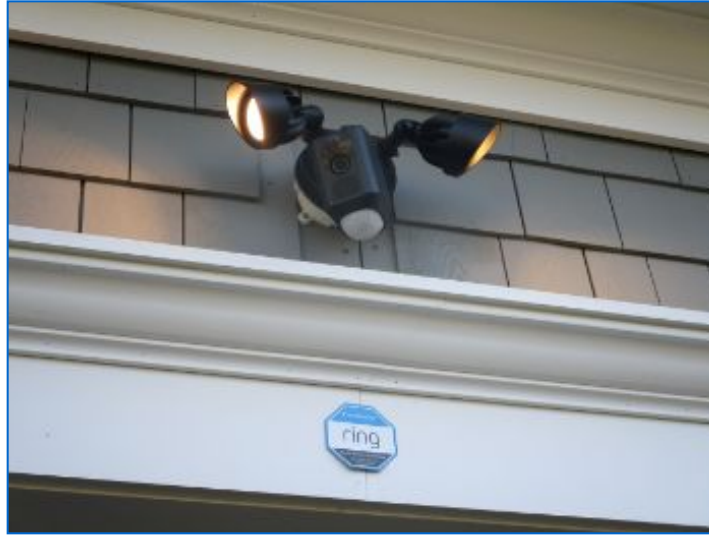
Adjust exterior lighting for dawn-to-dusk operation.
