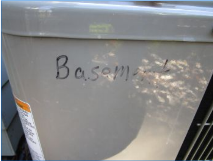
AC#1 Condenser; corresponding ducted air handler located in the Basement.
