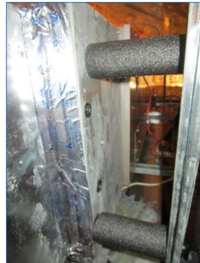
Duct mounted heating coil at HVAC#3.
