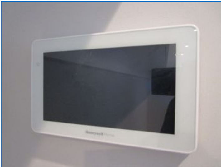
Graphic Touch Pad for integrated control system located at side entrance.
