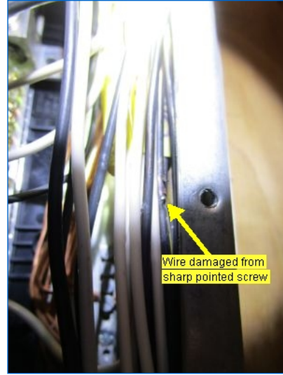
Sharp-pointed metal screws hold panel cover in place. These are a potential hazard as they can puncture wire insulation and electrify panel box, becoming a shock or electrocution hazard. These screws should be replaced with approved, flat-tipped screws. Repair existing damaged wire insulation!
