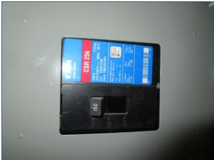
Main Panel #1 Main Disconnect: 150 amp main breaker serves Part of the property.
