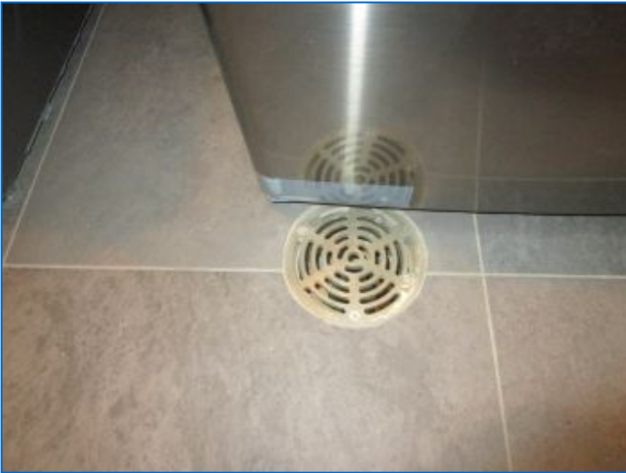
Floor drain noted; not tested. Suggest testing for proper operation.
