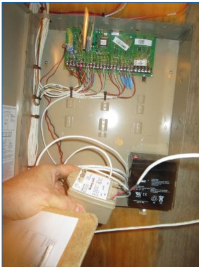
Control panel for the integrated control located in Basement. No available outlet near panel.
