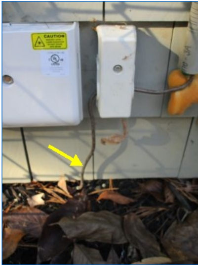
Ground conductor to ground rod noted at service entrance per current standard.
