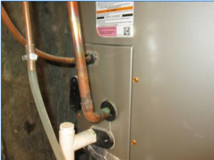
Cooling coil section of HVAC#1.
