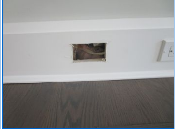
Incomplete data/telecom jack installation noted. Recommend completion and/or finishes prior to close.
