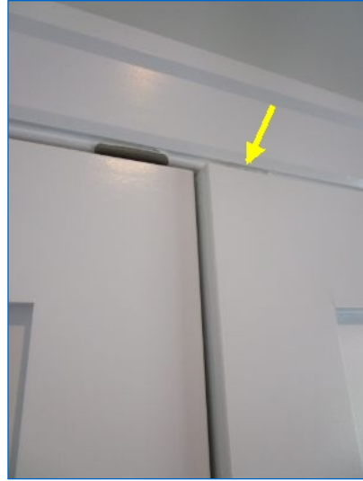
Door ball catch didn't latch properly . Recommend by a qualified contractor.
