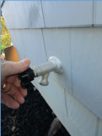
Hose bib at Front was Not active at time of inspection; possibly turned off from inside (winterized) or possible repair needed. Suggest having seller activate and test prior to close.
