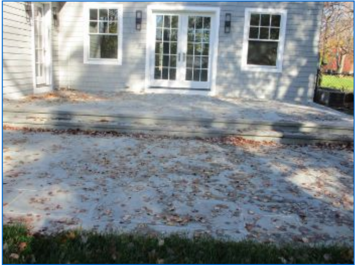
No system safety or function concerns at the visible portions of the patio at time of inspection.
