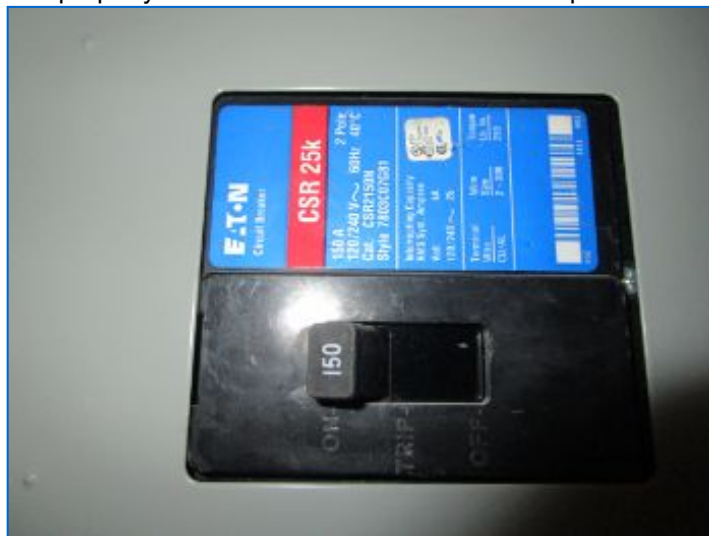
Main Panel #2 Main Disconnect: 150 amp main breaker serves Part of the property.
