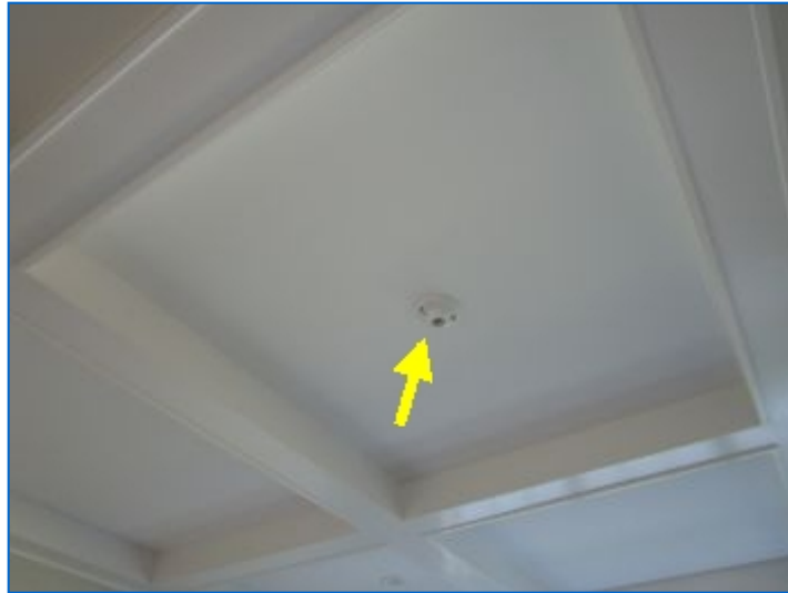
Light fixture bulb missing. Add bulb to check circuit.
