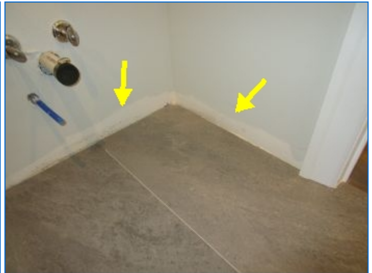
Some base molding was missing. Suggest completion.
