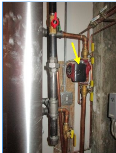
One pump dedicated to water heater storage tank.
