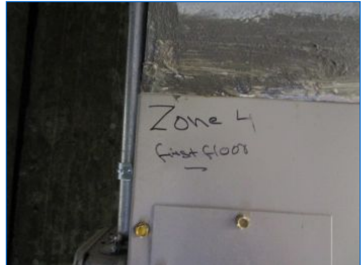
HVAC#5 ducted Air Handler located in the Basement to serves the 1st floor.
