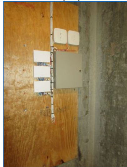
Control panel for the integrated control located in Basement. The Inspector recommends conferring with the seller for system and service contact information for customization and completion of installation.
