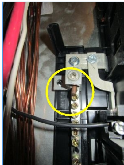
Main Panel #2: Proper Neutral Bus Grounding was not observed. Recommend licensed electrician to ensure proper system grounding per current standard.
