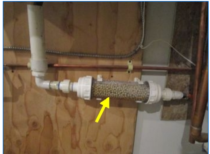
Condensate neutralizer noted. This vessel is installed in the condensate drain from a condensing boiler, water heater or furnace (before it enters the sewer). It's filled with media which raises the pH level of the condensate, making it safe to discharge into the sewage or septic system.
