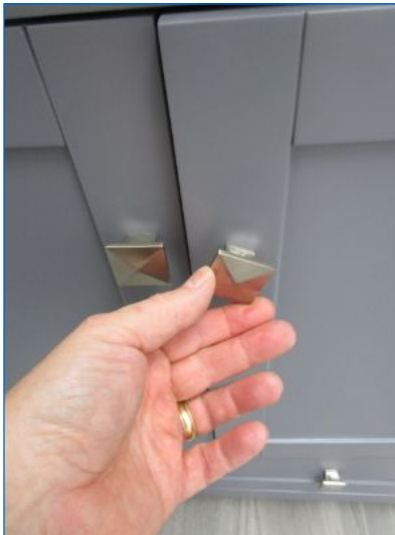
Vanity door knob was loose.
