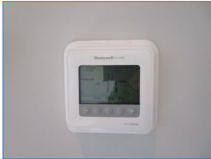
Digital Programmable type thermostat noted in Master bedroom; for Heating & Cooling.
