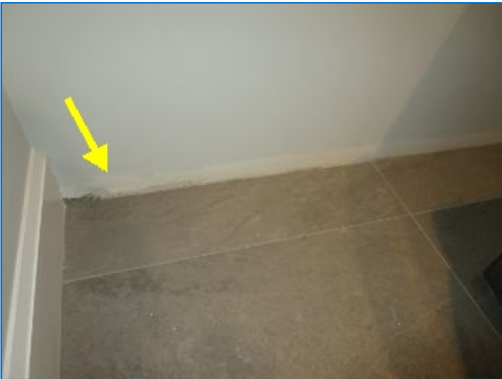
Some base molding was missing. Suggest completion.
