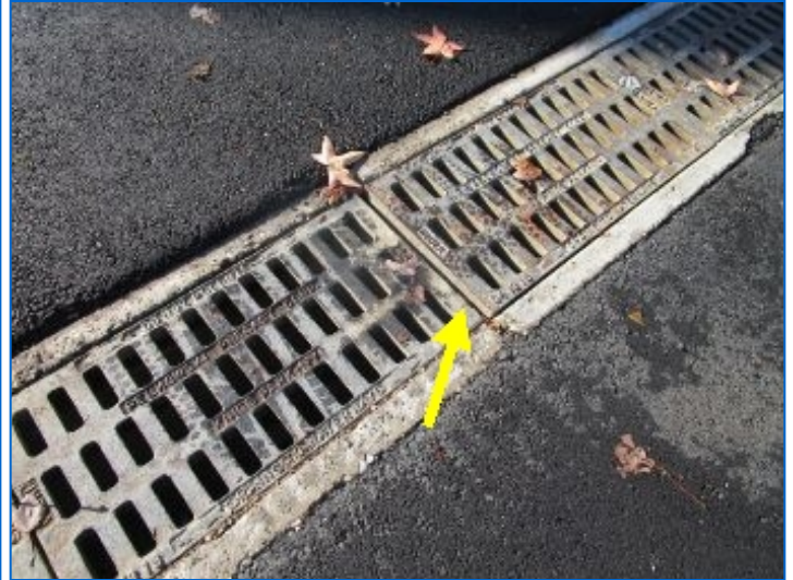
Uneven grate noted at trench drain.
