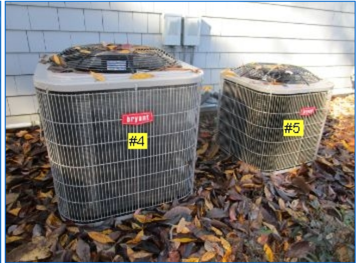
Multiple (5) Central HVAC split-systems, each with outdoor Condenser for cooling and indoor ducted Air Handler. Refer to Heating section for additional information.
