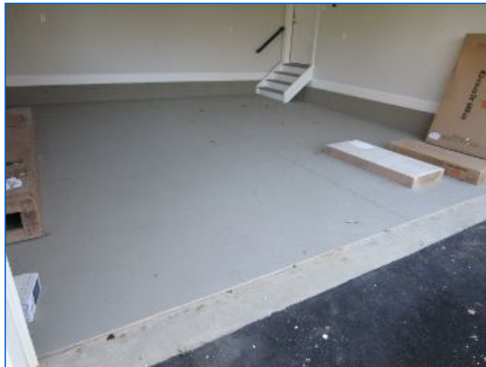
Painted concrete floor noted. The Inspector observed no deficiencies in the condition of the garage floor.
