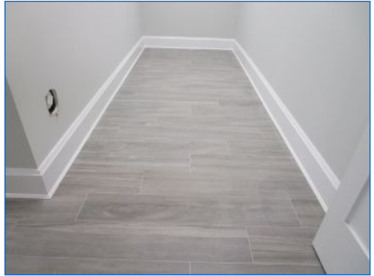
Storage room: No outlets noted in this area.
