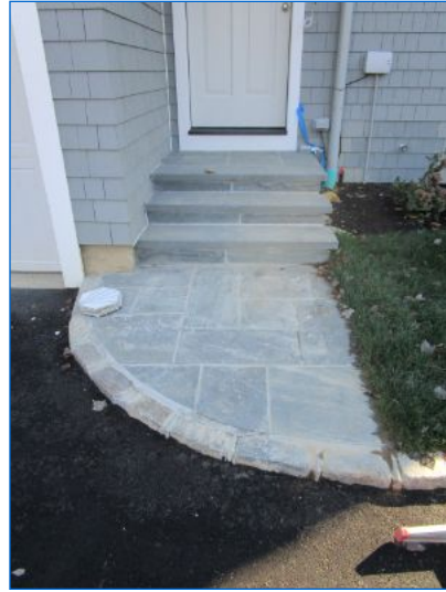
Masonry Steps and Landings noted at Front and side entrances. No system safety or function concerns noted at time of inspection.
