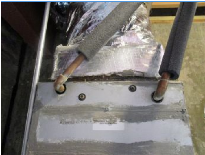
Duct mounted heating coil at HVAC#5.
