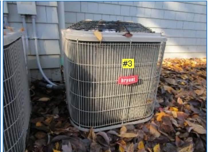
AC#3 Condenser; corresponding ducted air handler located in the Attic.
