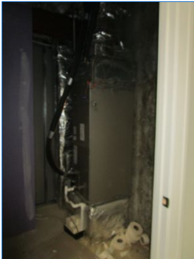
HVAC#5 ducted Air Handler located in the Basement closet appeared to serve the 1st floor.
