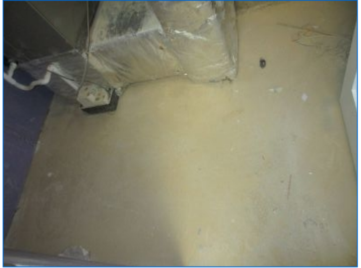
No unusual cracks observed at the visible portions of the concrete floor slab at the time of inspection - In normal condition.
