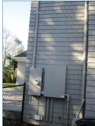
Overhead electrical service drop and riser showed no system safety or function concerns at time of inspection.
