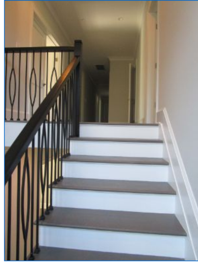
Stairs to 2nd floor. Stairway showed no system safety or function concerns at time of inspection.
