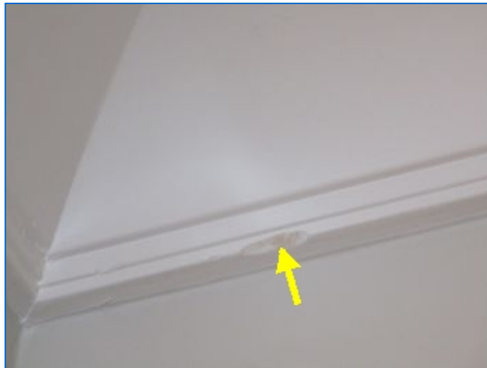
1st floor Hallway Storage Room: Nick noted in crown molding.
