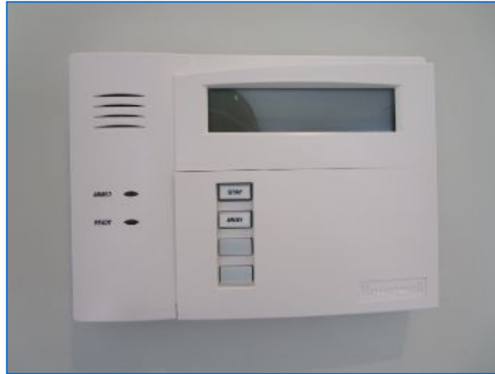
Key pad for the security system was located in Master bedroom.
