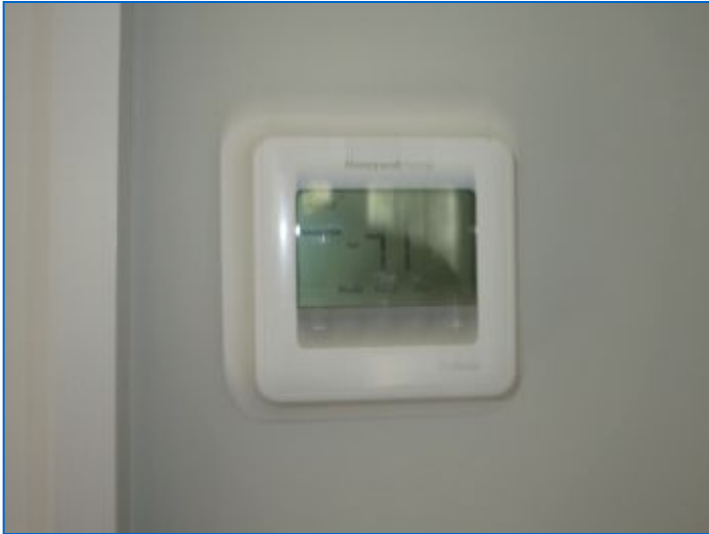
Digital Programmable type thermostat noted in Family room; for Heating & Cooling.
