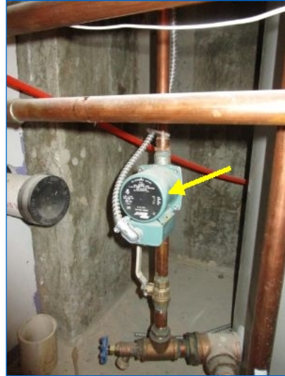
House HW recirculating pump noted.
