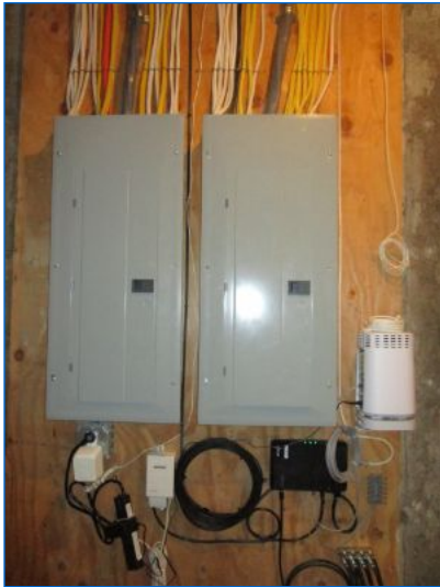
Two Main Panels located in Basement Boiler Room.
