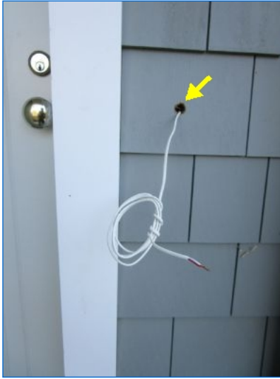
Side doorbell was not installed at time of inspection.
