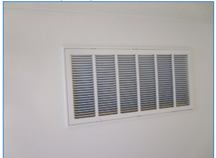
Disposable filter located in filter-grille at ceiling in Hallway (2nd floor).
