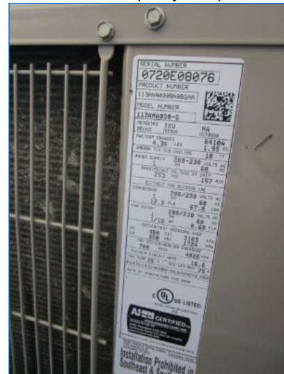
AC#4 Bryant Condenser data-plate/serial no. indicated a cooling capacity of 2.5 tons, and a manufacture date of 2/2020, (0.5 yr old).
