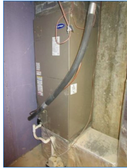
HVAC#4 ducted Air Handler located in the Basement Storage Room serves the 1st floor.
