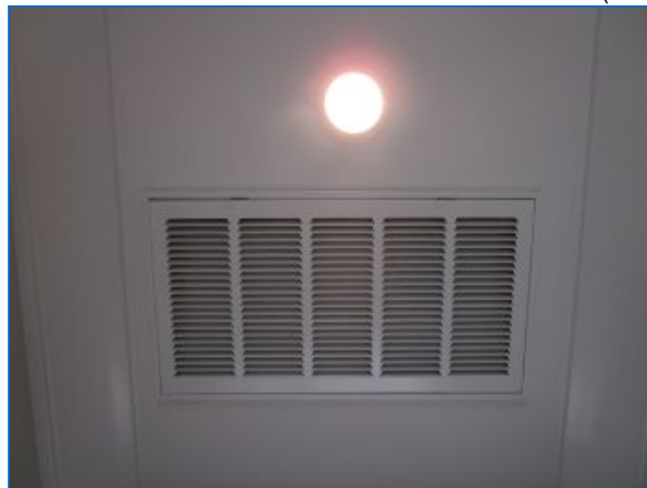
Disposable filter located in filter-grille at ceiling in Master bedroom hallway.
