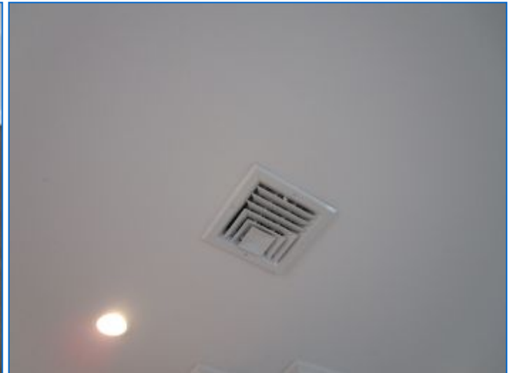
Ductwork with floor/ceiling supply registers & return air grilles distribute Heating & Cooling.
