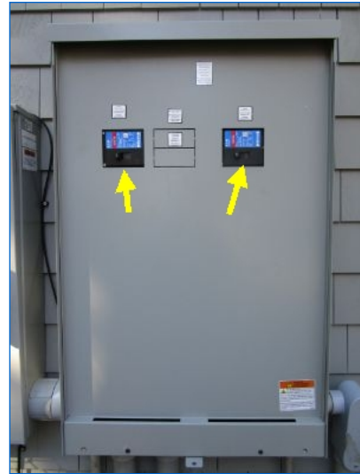
Exterior service entrance panel houses disconnects (200 amps each) for the two main panels located in the basement. This panel design also for housing transfer gear for the backup generator. Refer to related comment.
