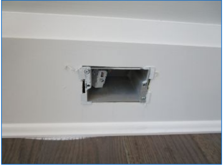
Incomplete data/telecom jack installation noted. Recommend completion and/or finishes prior to close.
