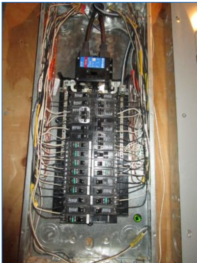
Main panel interiors checked.
