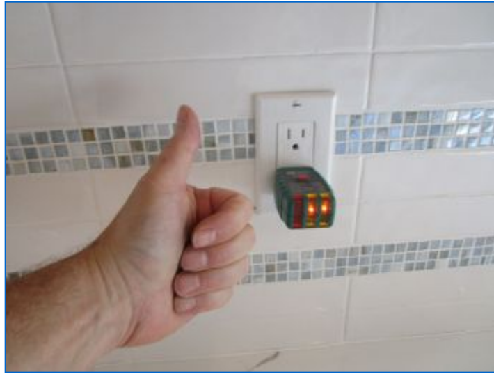
GFCI protected receptacles in place and operational.
