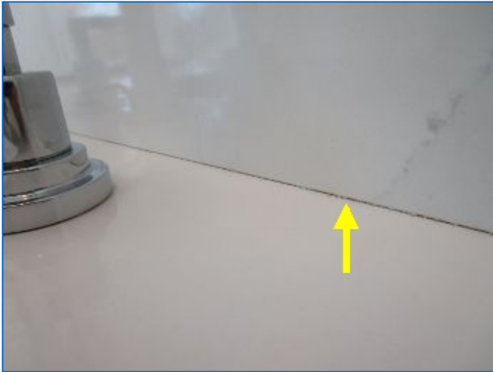
Vanity backsplash not adequately sealed.
