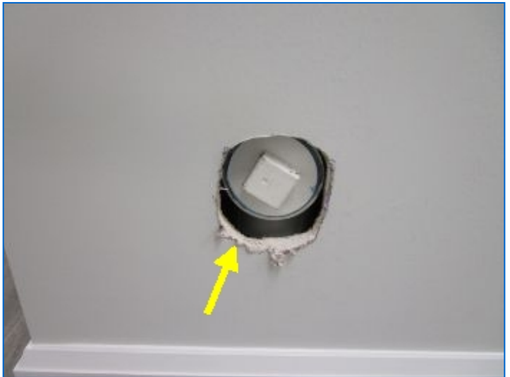
Storage Room: Access cover missing at plumbing clean-out plug.
