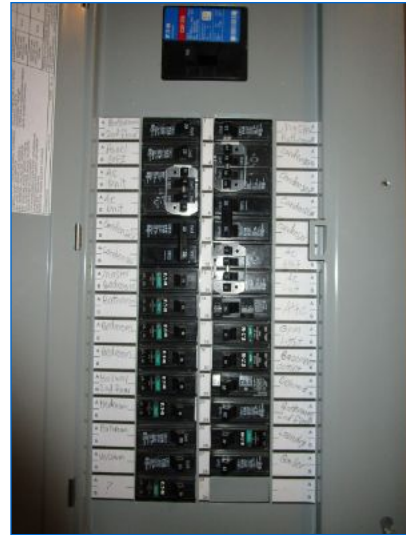
Main Panel #1 Breakers: 30 full-size circuit breaker spaces; 1 spare breaker space(s) noted.
