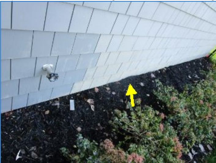
Soil in contact with, and/or in close proximity to siding. This can provide entrance of moisture or insects to siding. The Inspector recommends lowering soil level to 6" below siding.
