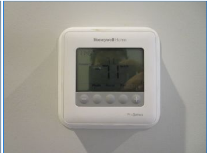
Digital Programmable type thermostat noted in Hallway (2nd floor); for Heating & Cooling.
