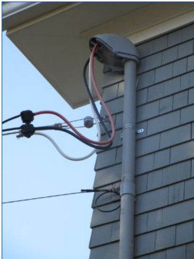
Overhead service drop; 120/240 volts. Overhead electrical service drop and riser showed no system safety or function concerns at time of inspection.
