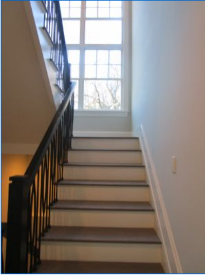
Stairs to 2nd floor. Stairway showed no system safety or function concerns at time of inspection.
