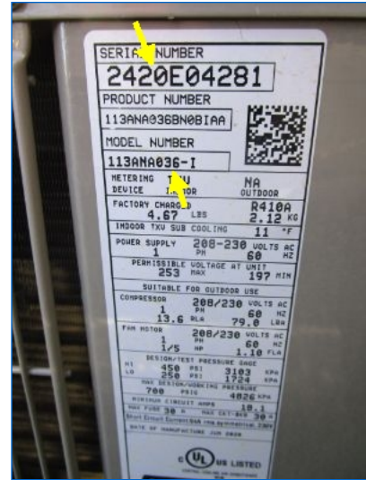
AC#2 Bryant Condenser data-plate/serial no. indicated a cooling capacity of 3 tons, and a manufacture date of 6/2020, (0.5 yr old).
