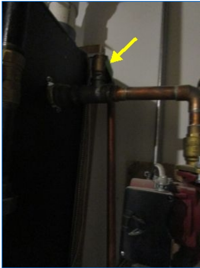
TPR (Temperature Pressure Relief) valve and discharge pipe installation showed no deficiencies.
