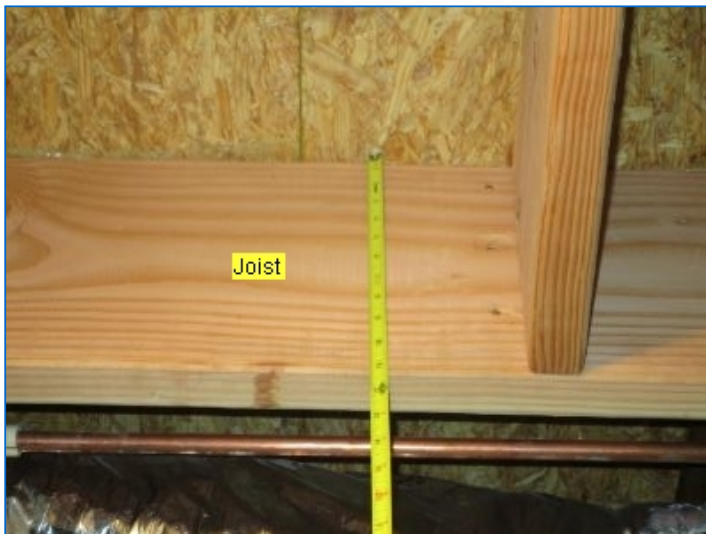
Floor Main Structure: Steel girders supported by steel lally columns, 2x12 Joists 16" O.C. (w/cross braces), Oriented-strand floor boards.
