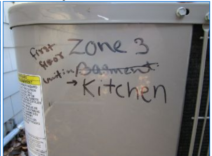
AC#4 Condenser; corresponding ducted air handler located in the Basement.
