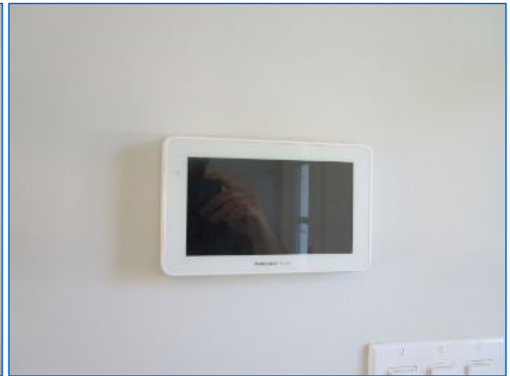
Graphic Touch Pad for integrated control system located in Entryway.
