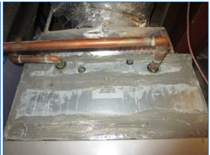
Duct mounted heating coil at HVAC#4.
