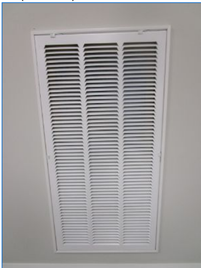
Disposable filter located in filter-grille at wall in Basement.
