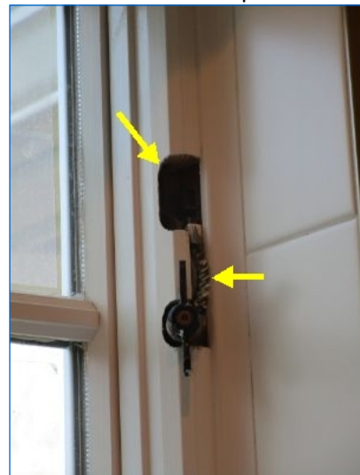
Casement window crank mechanism cover was missing. Recommend correction.
