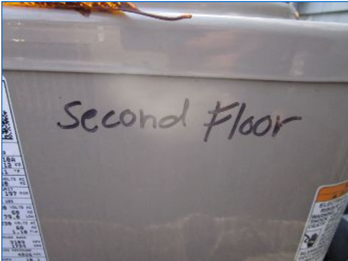
AC#2 Condenser; corresponding ducted air handler located in the Attic.
