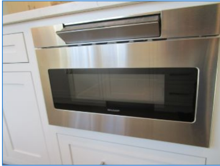
Microwave was operable at time of inspection.
