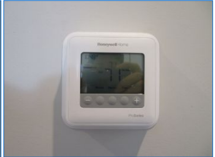
Digital Programmable type thermostat noted in Hallway (1st floor); for Heating & Cooling.
