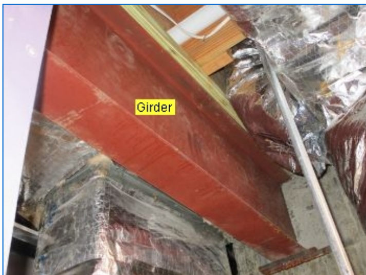
Floor Main Structure: Steel girders supported by steel lally columns, 2x12 Joists 16" O.C. (w/cross braces), Oriented-strand floor boards.
