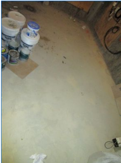
No unusual cracks observed at the visible portions of the concrete floor slab at the time of inspection - In normal condition.
