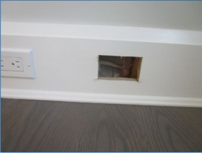
Incomplete data/telecom jack installation noted. Recommend completion and/or finishes prior to close.
