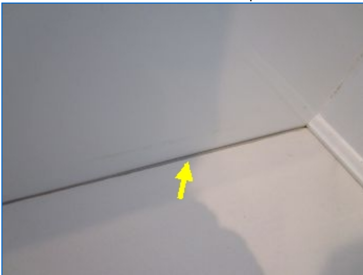
Exterior base grout was cracked/gapped at Tub floor joint. Recommend grout repair to prevent water entry that can cause damage to floor boards/ceiling below.
