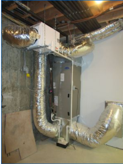
HVAC#1 ducted Air Handler located in the Basement Boiler Room serves the Basement.
