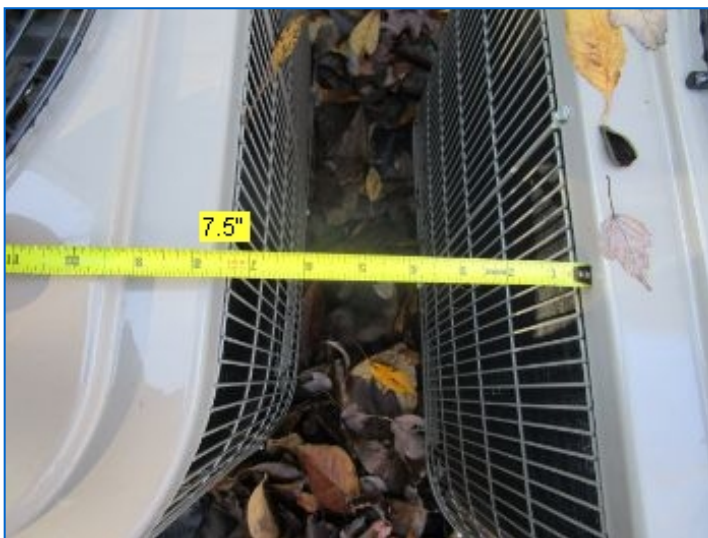
Outdoor condenser air flow appeared restrictive based on the distance between units. This conditions can negatively affect system performances by as much as 10% when both units are operating. Suggest checking manufacturer's clearance requirements.
