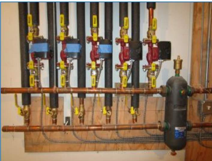
Distribution Piping: 5-zone heating system noted.
