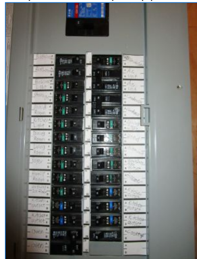
Main Panel #2 Breakers: 30 full-size circuit breaker spaces; 1 spare breaker space(s) noted.
