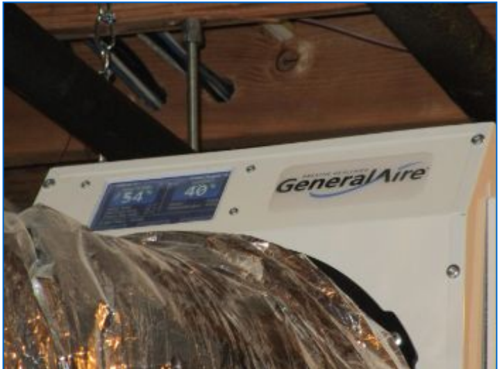
The basement HVAC#1 system was equipped with an operable ducted dehumidifier. Refer to related comment.
