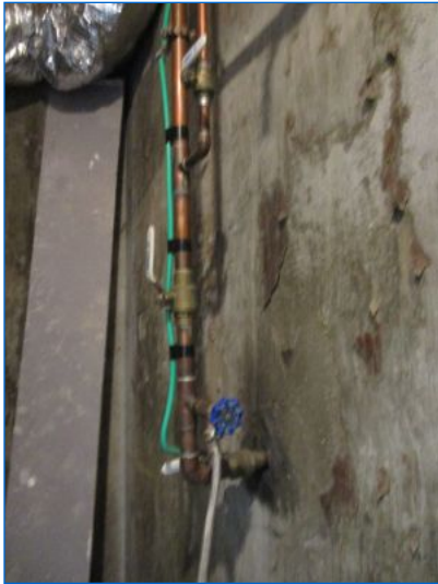
Water Service Entrance: 1" Copper line with shutoff valve/s. Meter external to the structure.
