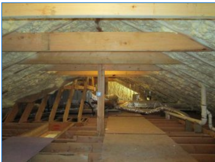
Roof Main Structure: 2x12 Rafters 16" O.C. w/collar-ties, Double laminated veneer lumber (LVL) Ridge beams, Plywood roof boards.
