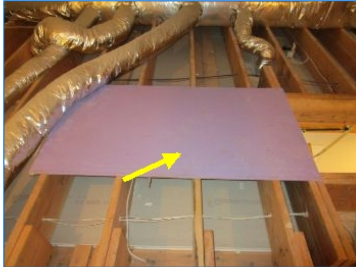
Drywall cover meant for pull-down ladder opening only.
