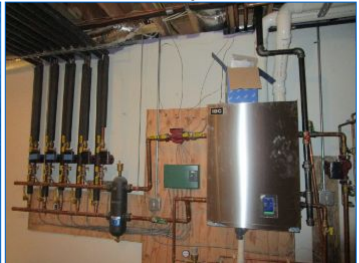
Heating Equipment located in Basement was operable at time of inspection.
