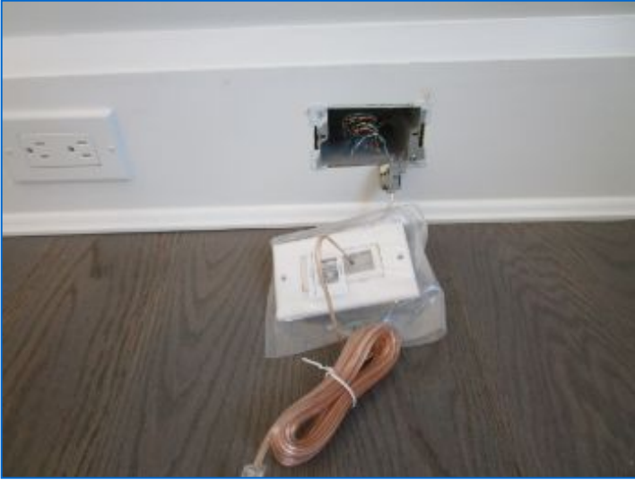
Incomplete data/telecom jack installation noted. Recommend completion and/or finishes prior to close.
