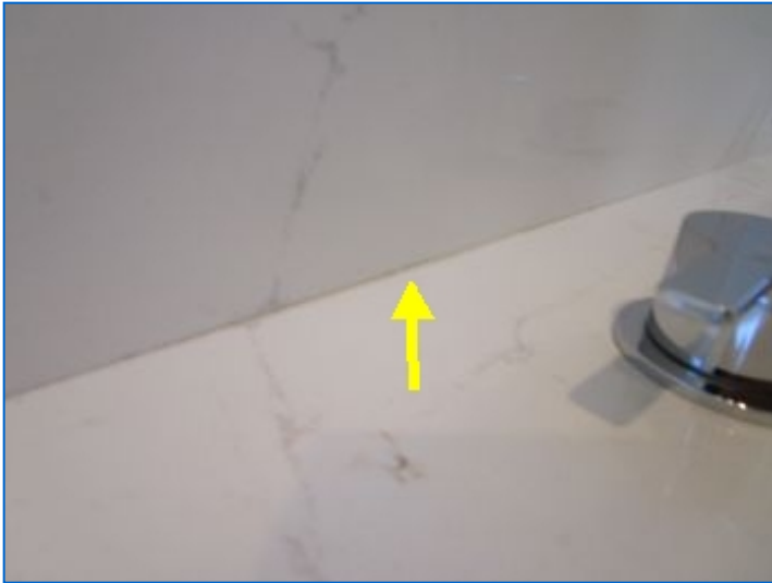
Vanity backsplash not adequately sealed.
