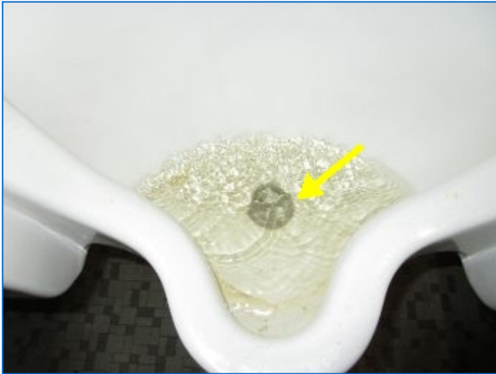
Urinal drain strainer was missing.
