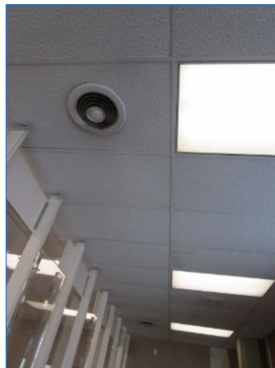
Tellers: HVAC supply registers noted.
