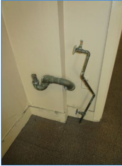
Interior Area-3, Teller Admin: CW supply and drain for water fountain noted at west side.
