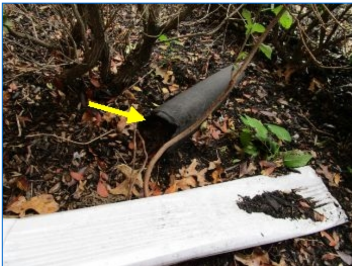
Former downspout connection apparently to underground drywall was not in use; perhaps clogged.
