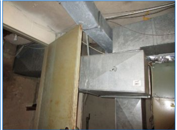
Ductwork appeared in serviceable condition. Recommend replacing supply and return registers/grilles as standard for cosmetic purposes.
