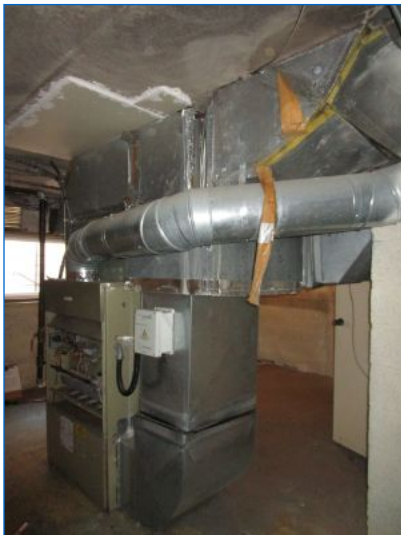
Heating system was originally found in the OFF position at the thermostat. The Inspector returned the thermostat to the original OFF position. This lack of heat could jeopardize plumbing systems in the building during winter.
