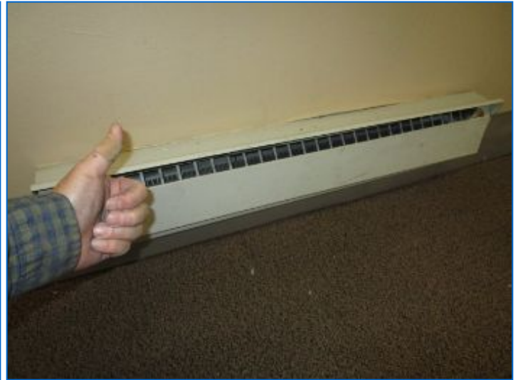
Bank Admin: Electric Baseboard (1) operable.
