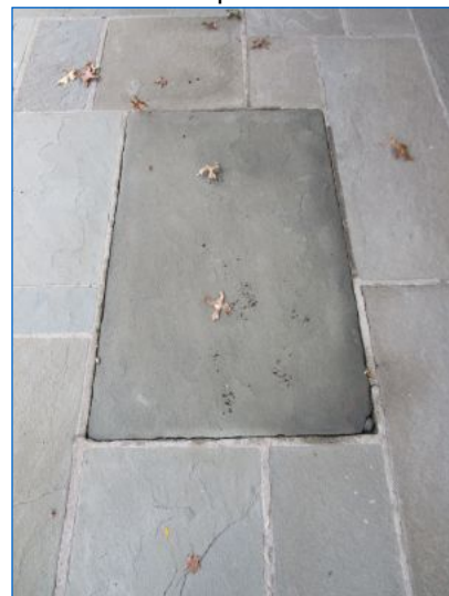
Cracked mortar noted around a bluestone flag.
