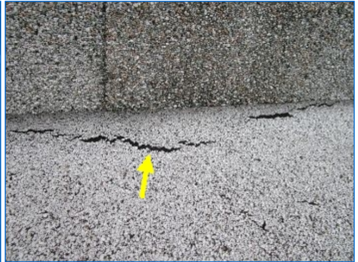
Conditions that can result in roof leaks noted.
