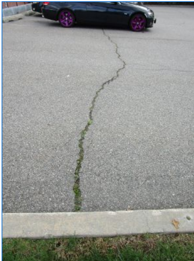
Moderate cracks in parking area and driveway. Monitor cracks for the development of trip hazards and have cracks repaired by a qualified contractor.
