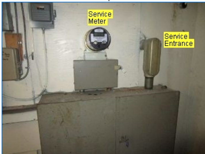
Capacity rating for overall electric service was not available at time of inspection; main disconnect cabinet was locked by utility company. Recommend consulting with PSEGLI for service capacity information as needed.
