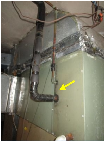
Cooling Coil integrated into ducted forced air furnace located in Basement.
