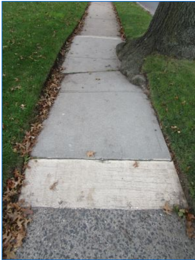
Sidewalk flag/s heaved/cracked by tree roots; monitor for trip hazards. Repair as necessary.
