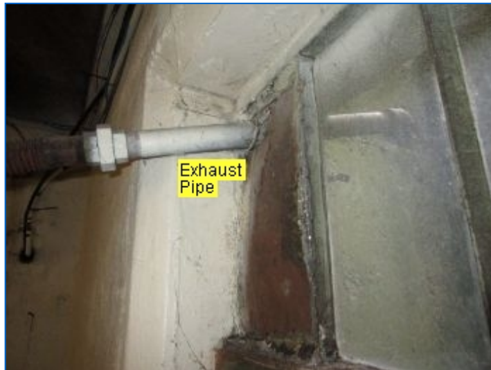
Old defunct engine generator with 30 amp disconnect; no fuel source observed. Recommend removal.
