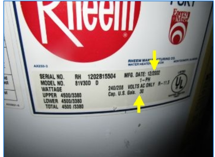
Rheem 30 gallon capacity unit. Water Heater data-plate/serial no. indicated a manufacture date of 12/2002 (18 yrs old).
