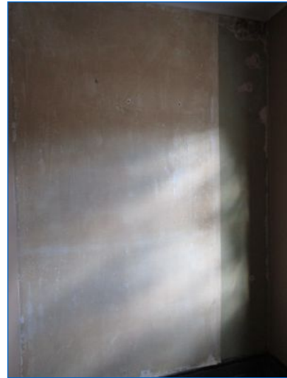
East vestibule walls. Cosmetic updates and repairs needed throughout.
