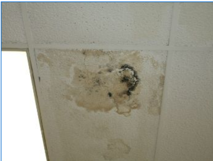
Signs of a roof leak.
