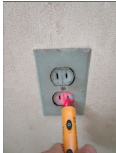
Teller Admin: (2) receptacles were the outdated, ungrounded 2-prong electrical type. Recommend having an electrician update these to meet generally-accepted current standards (grounded 3-prong outlets).
