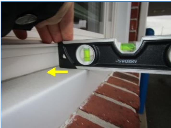
Few aluminum cladded window sills were improperly sloped toward caulked joint where water intrusion can occur, making it critical that caulking is maintained here. Maintenance: Recommend periodic inspection to update caulking around windows to prevent water entry.
