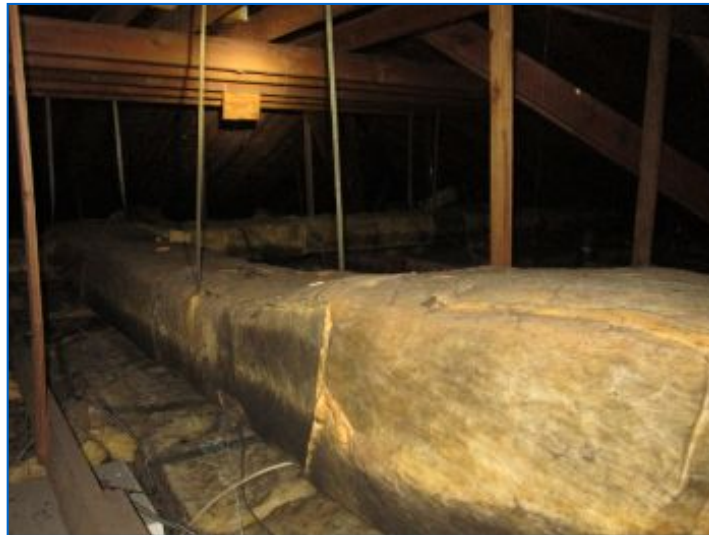
Insulated ductwork noted above hung ceiling.
