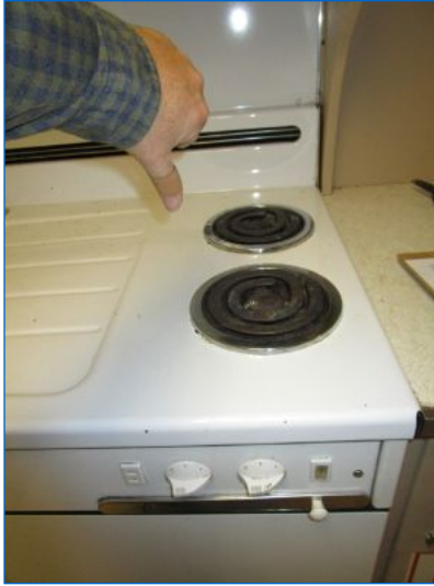
Cafeteria Pantry: Kitchenette was inoperable.
