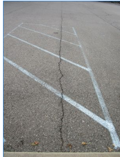
Moderate cracks in parking area. Seal and/or repair cracks to prevent water entry leading to freeze-thaw damage.
