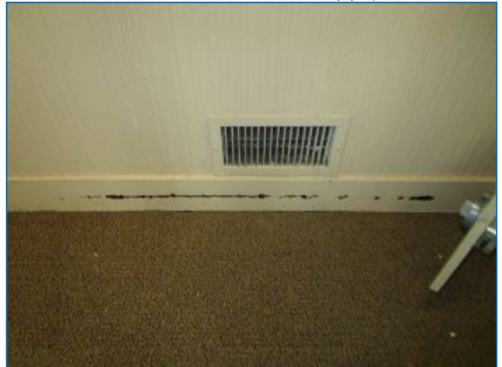
Tellers: HVAC supply registers at east exterior wall not connected to an HVAC system; open-ended at basement ceiling.
