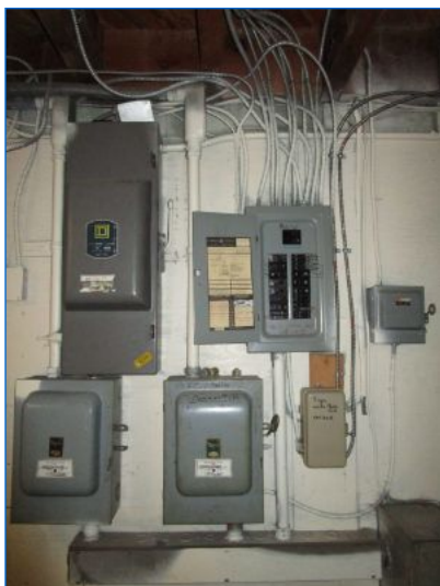
Older switch gear in Utility Room appeared serviceable at time of inspection.
