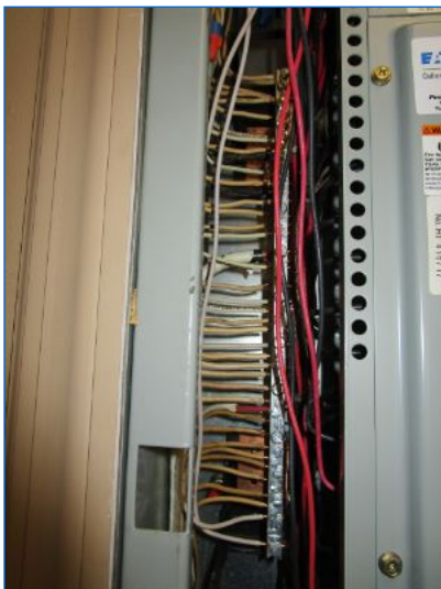
Main Panel #1: Neutral bus grounding could not be confirmed at time of inspection. Recommend having a licensed electrician evaluate to ensure there's proper system grounding per current standard.
