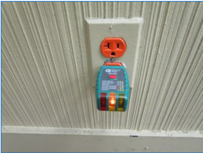
Orange receptacles generally indicate the circuit is backed up by emergency power. Open Ground receptacle noted.
