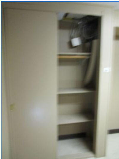
Cafeteria: Former telecom closet.
