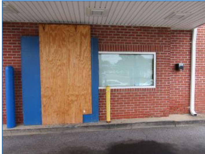
Opening in wall covered with plywood.
