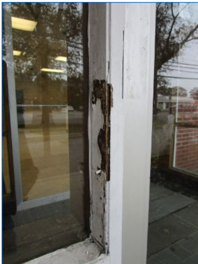
Front vestibule frame/trim had peeling paint; signs of wood deterioration noted. Suggest scrape or strip and repaint to prolong life.
