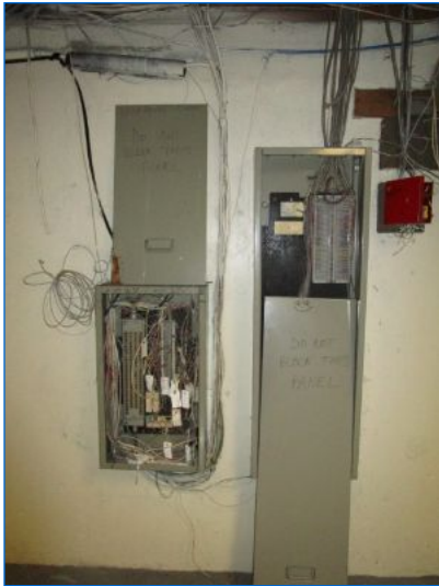
General Area: Old abandoned telecom equipment noted.
