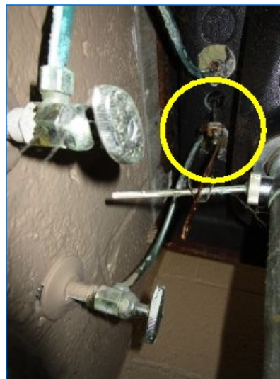
Visible leaking under the sink. Source of existing leak could not be determined; Recommend qualified plumber evaluate and repair.
