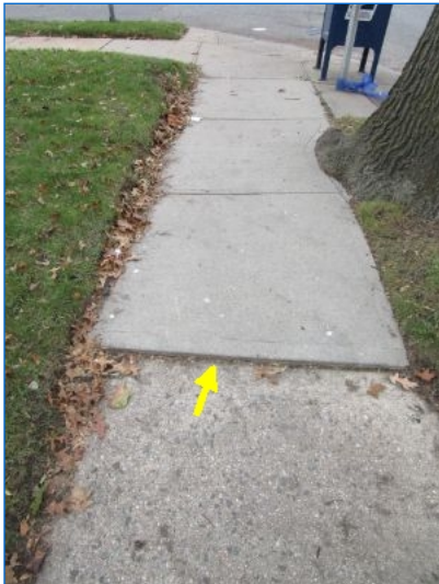
Sidewalk flag/s heaved by tree roots; trip hazards noted. Repair as necessary.
