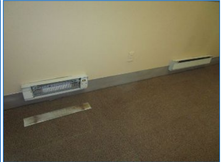
Bank Admin: Heat distribution types included Electric Baseboard.
