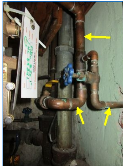
Water supply pipe observed included: Copper.
