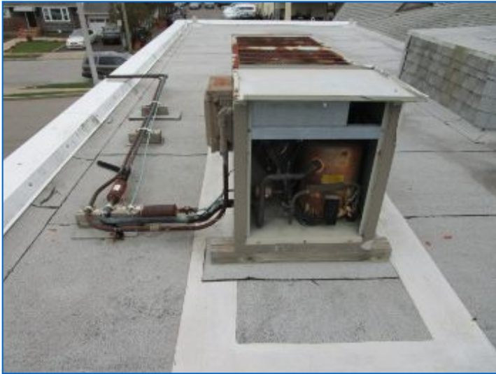
Central HVAC: split-system with outdoor Condenser for cooling and indoor ducted Forced Air Unit. Refer to Heating section for additional information.
