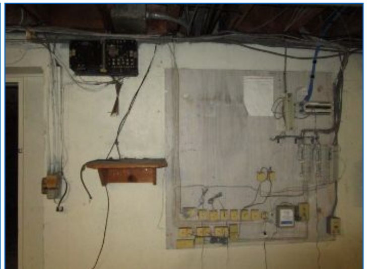
General Area: Old abandoned telecom equipment and circuits noted.
