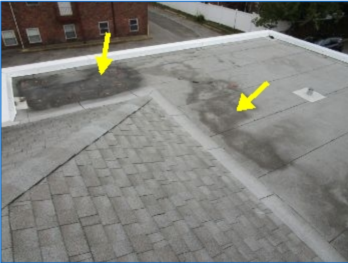
Signs of past ponding at front flat roof area. Maintain seal at seams to prevent roof leaks.
