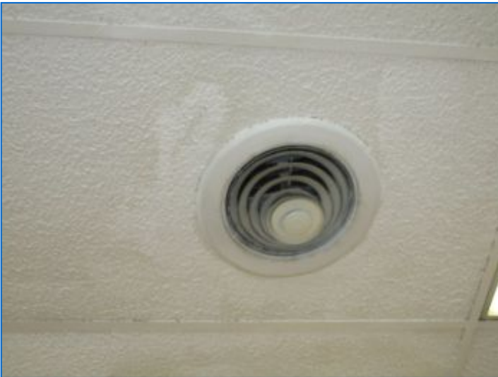
Ductwork with supply & return air registers for distribution of Heating & Cooling noted at main level.
