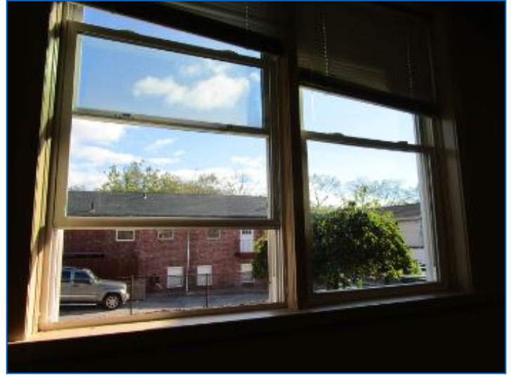
All screens were missing or not installed at the time of inspection. Confer with Seller.
