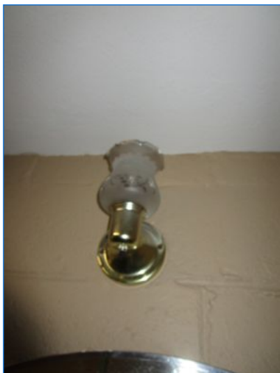
Light fixture or bulb apparently inoperable. Change bulb and check.
