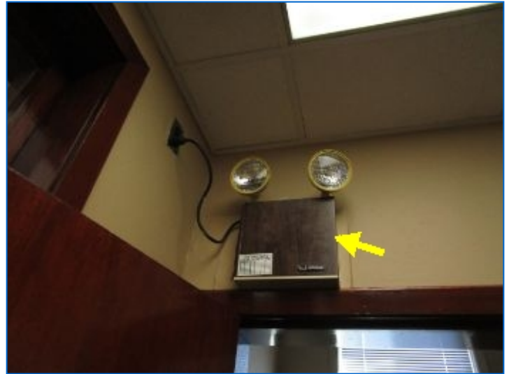
Vault Area Hallway: Emergency lighting and exit signs were present, although all were not tested at time of inspection.
