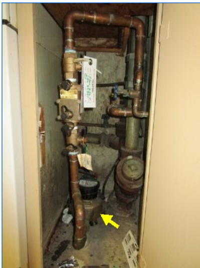
Public water service entrance located in Basement Cafeteria Pantry. Water Service Entrance: 3/4" Copper line with Meter and shutoff valve/s.
