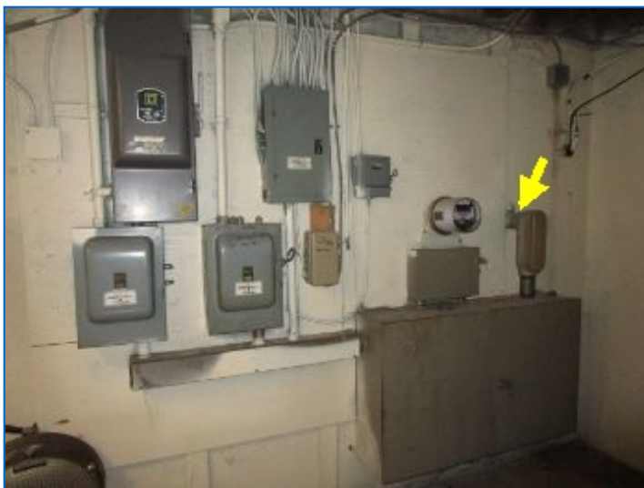
Underground electrical service showed no signs of system safety or function concerns at time of inspection.
