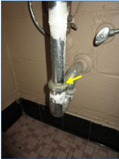
Lavatory drain connection leaked. Recommend repair by a qualified contractor.
