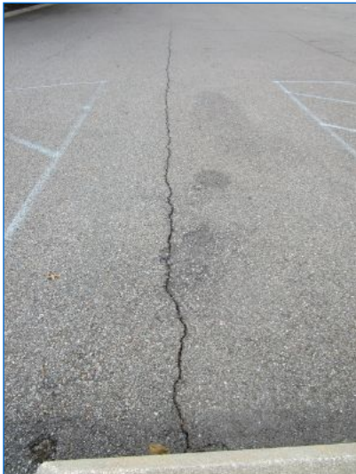
Moderate cracks in parking area. Seal and/or repair cracks to prevent water entry leading to freeze-thaw damage.
