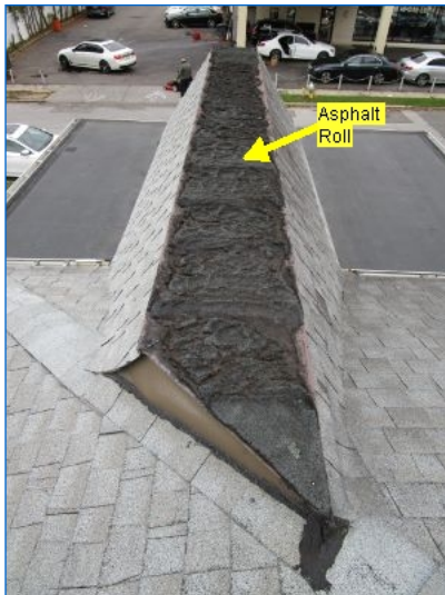
Roof over bank pneumatic tube conveyor consisted of architectural shingles, metal cap flashing and asphalt roll roofing. Asphalt roll roofing was deteriorated exposing the underlying cap flashing; conditions that potentially leak noted here.
