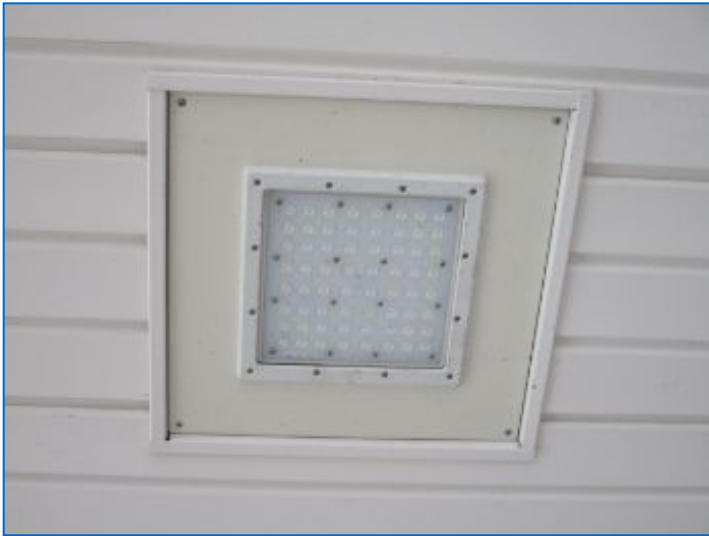
LED lighting noted at front and west soffits; exterior lighting controlled by remote timer schedule.
