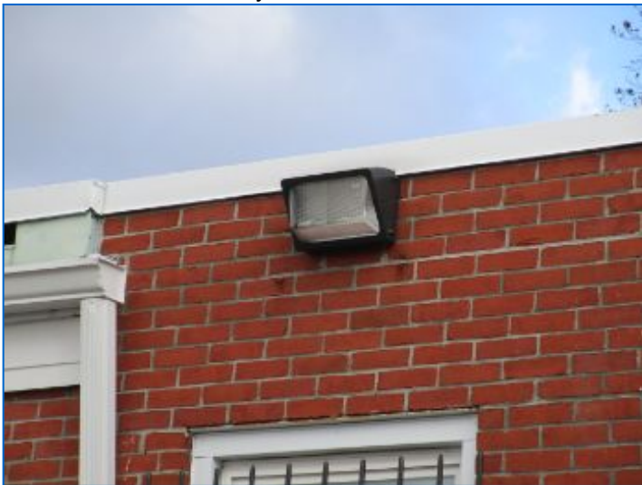
Exterior lighting controlled by remote timer schedule; not tested. Recommend testing prior to close.
