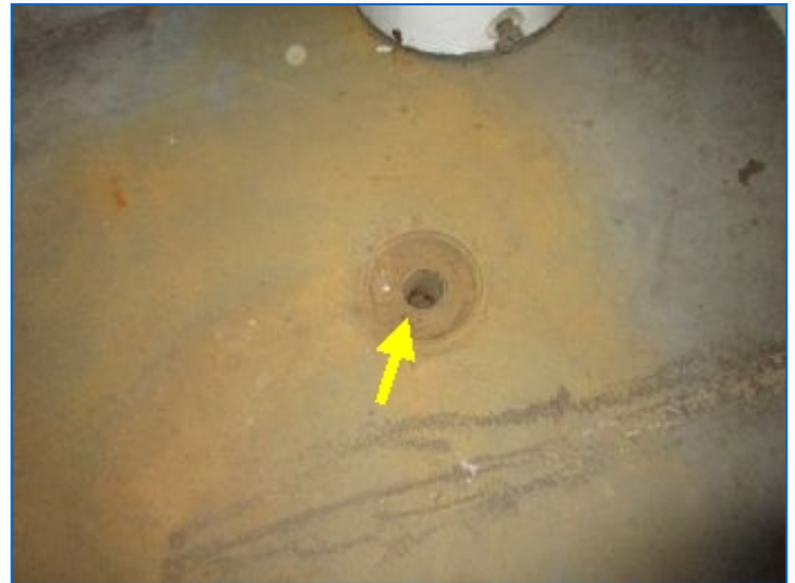
Open floor drain observed, suggest installing a grate or cover for safety. Floor drain observed but not tested. Suggest testing for proper operation.
