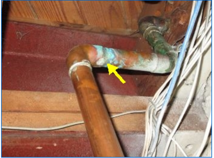
General Area (East-side): Active leaks observed at water supply pipe at time of inspection. Recommend repair by a Qualified Plumber.
