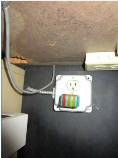
Tellers: Random Outlet Test - No Power at receptacle at time of inspection. Suggest seller locate or restore source of power prior to close.
