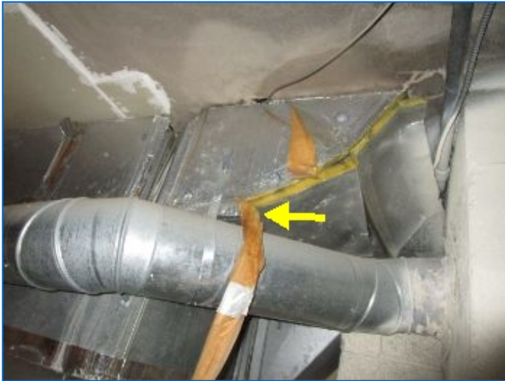
Some insulation tape had detached the duct insulation. Recommend corrective repairs by a qualified contractor.
