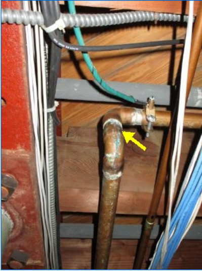
General Area (East-side): Active leaks observed at water supply pipe at time of inspection. Recommend repair by a Qualified Plumber.
