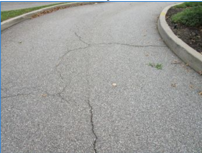
Moderate cracks in parking area and driveway. Seal and/or repair cracks to prevent water entry leading to freeze-thaw damage.
