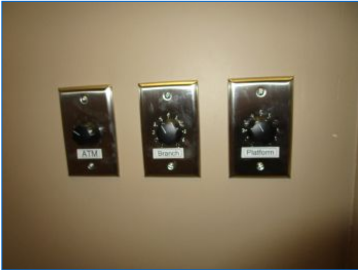
ATM room: Unknown switches noted.
