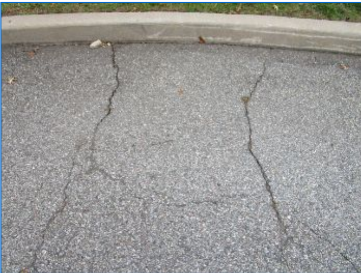
Moderate cracks in driveway. Seal and/or repair cracks to prevent water entry leading to freeze-thaw damage.
