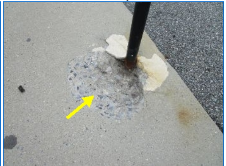
Concrete was chipped at handicap ramp handrail post; mainly a cosmetic concern.
