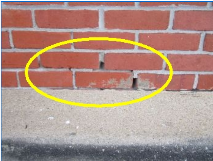
Maintenance: Mortar joint deterioration noted at west side. Repointing of deteriorated mortar is recommended to prevent further deterioration from frost weathering.
