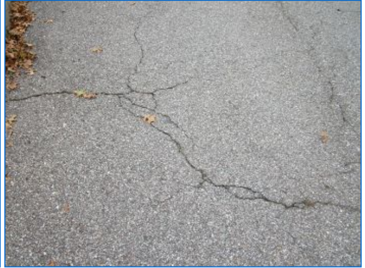
Moderate cracks in driveway. Monitor cracks for the development of trip hazards and have cracks repaired by a qualified contractor.
