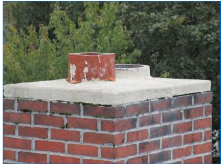
The chimney stacks appeared to have Unlined Flues. While this may have been acceptable at the time of construction, flue liners are a fire safety feature. The Inspector generally recommends installing chimney liner for active chimney flue. Refer to Chimney Liner in Glossary.
