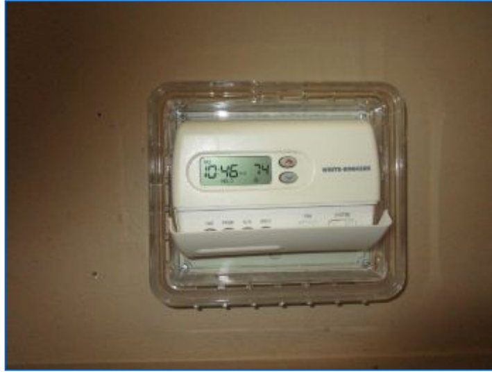
Digital Programmable type thermostat noted in Interior Area 1; for Heating & Cooling.
