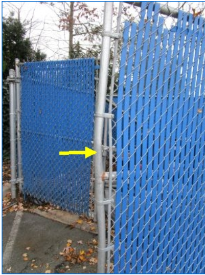
Parking lot storage area: Gate end was bent.
