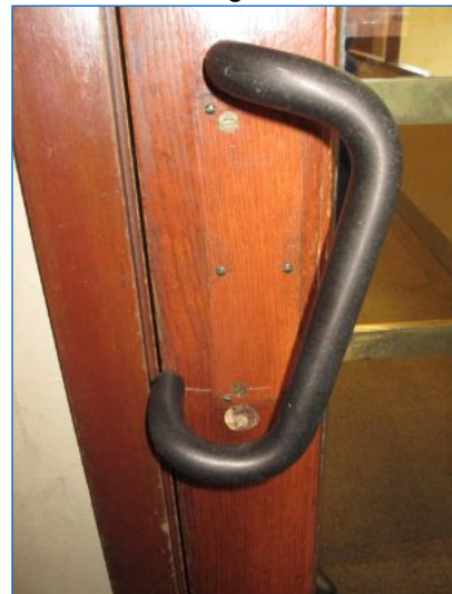
East vestibule; inside door handle was loose. Suggest repair.
