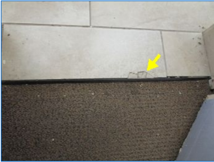
Hall/Stairway Area: Cracked tile noted at threshold.
