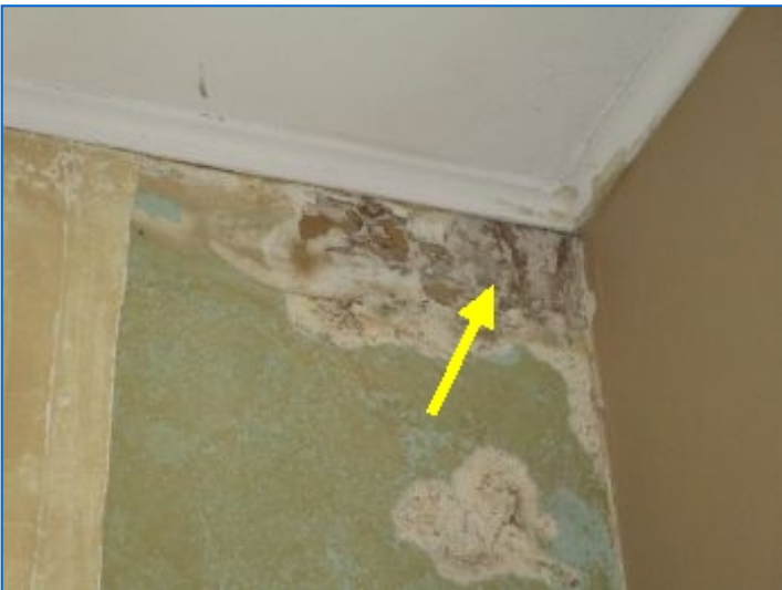
East vestibule; Signs of a past roof leak noted at exterior wall tested dry at time of inspection.
