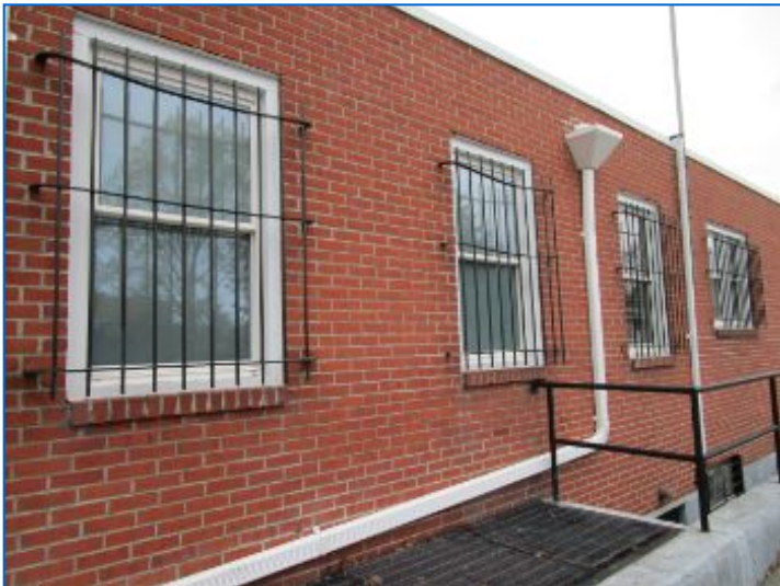
Steel burglar bars mounted to brick wall at 4 rear windows.
