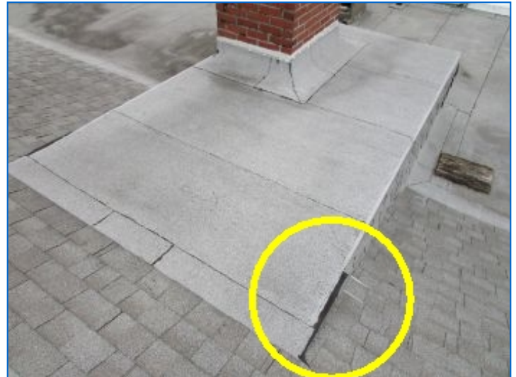
Vicinity of roof leak noted where moisture was observed inside building. Refer to related comments. Recommend evaluation and corrective repair by a qualified roofing contractor.
