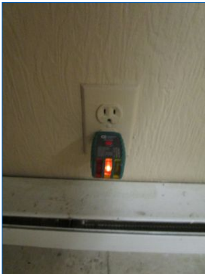
Cafeteria: Random Outlet Test - Ungrounded receptacle noted.
