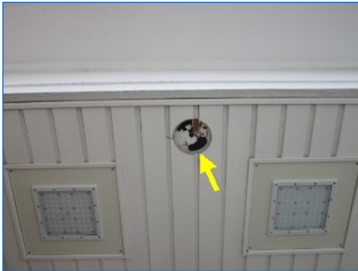
Soffit mounted component removed at front.
