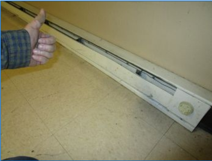
Cafeteria: Heat distribution type included Electric Baseboard.
