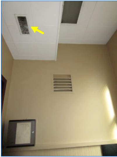
East Viewing Room HVAC supply noted.
