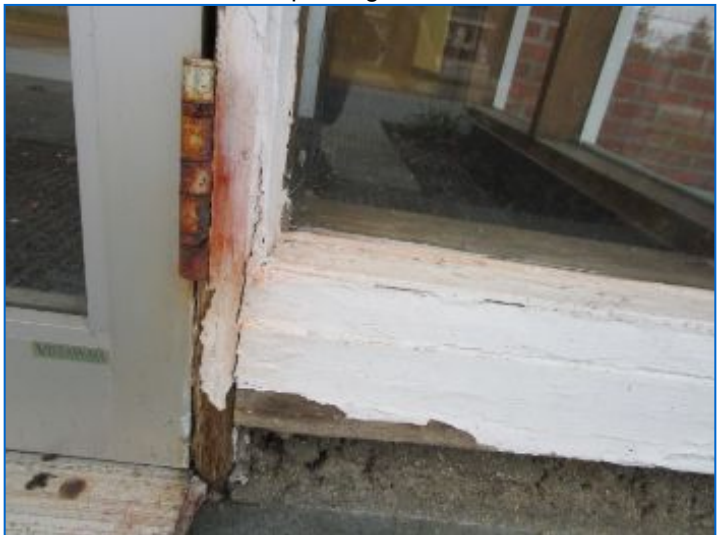
Front vestibule frame/trim had peeling paint; signs of wood deterioration noted. Suggest scrape or strip and repaint to prolong life.
