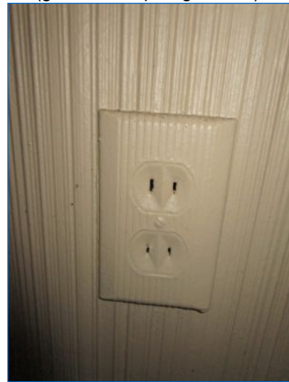
ATM room: Receptacle outdated, ungrounded 2-prong electrical outlets. Recommend having an electrician update these to meet generally-accepted current standards (grounded 3-prong outlets).
