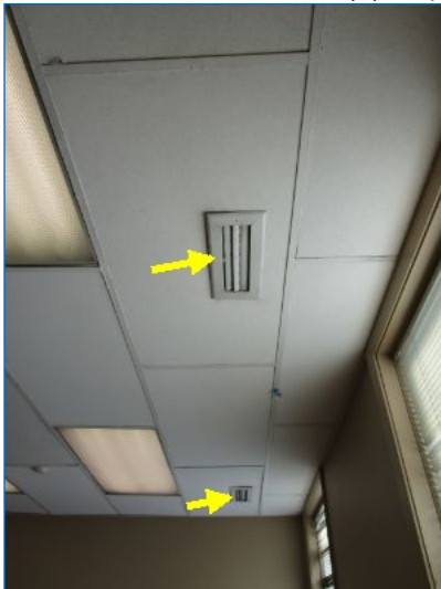
Teller Admin: HVAC supply registers noted.
