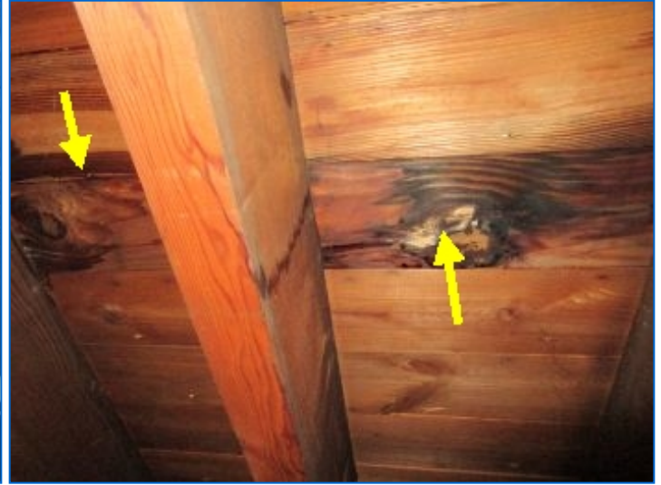
Signs of a roof leak noted above area of wet ceiling tile.
