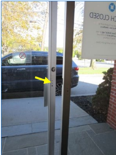
Front door push bar missing. Door did not close completely. Recommend corrective repairs by a qualified contractor.
