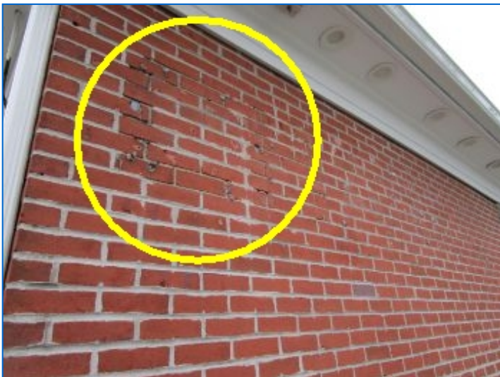
Cosmetic damage noted at front from past signage mounting.
