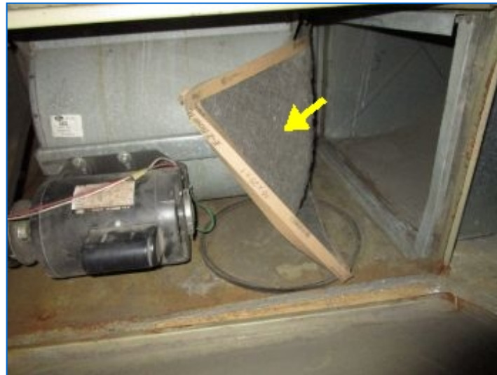
Disposable filter located inside return duct at air handler intake. Air filter was very dirty/clogged and collapsed. Replace with new fiberglass disposable filter; sign of poor maintenance.
