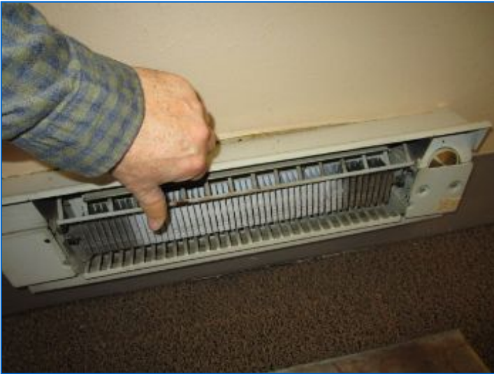
Bank Admin: Electric Baseboard (1) inoperable.
