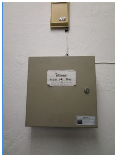
Apparently defunct security system panel noted in Bank Vault.
