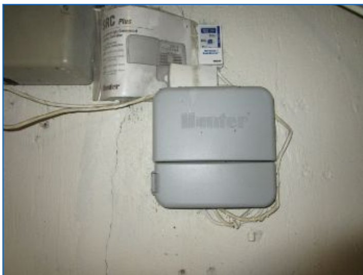
Control panel for sprinkler system located in Basement.
