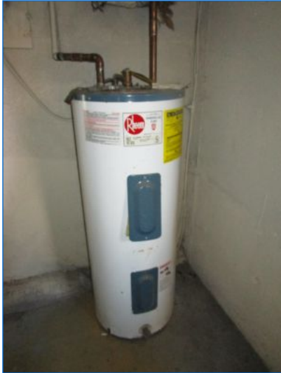
Electric Powered Water Heater located in Basement was partially operable, i.e., produced minimal minimal warm water for a short period of time.
