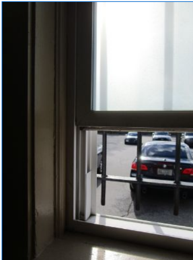
All screens were missing or not installed at the time of inspection. Confer with Seller.
