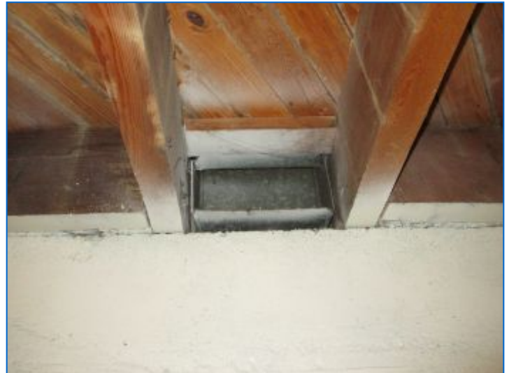
HVAC supply registers at east exterior wall not connected to an HVAC system; open-ended at basement ceiling (typical of 4).
