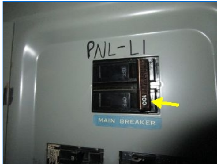
Main Panel #2 Disconnect: 100 amp main breaker serves Part of the property.
