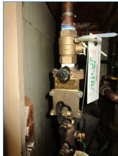
Backflow preventer (whole house) in place per current plumbing standard.
