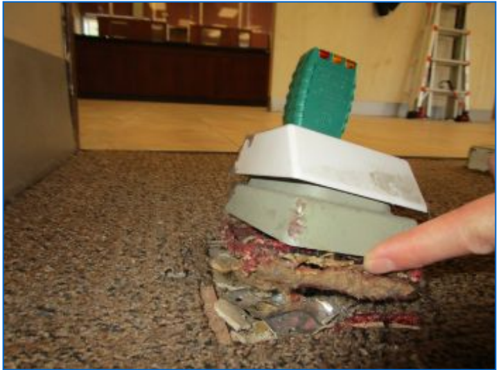
Loosely installed active receptacle noted at floor. Recommend repair by a licensed qualified electrician.
