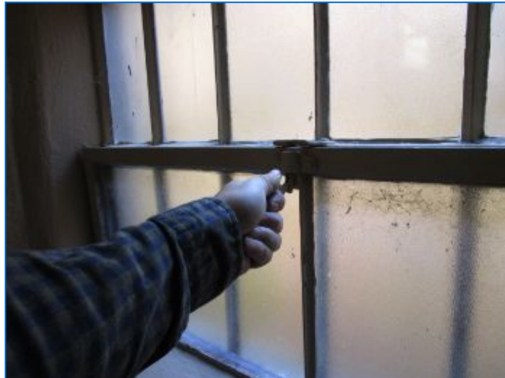
Bathroom window did not open when tested due to frozen latches from lack of use and/or paint layers. Recommend windows be serviced for proper operation prior to close.
