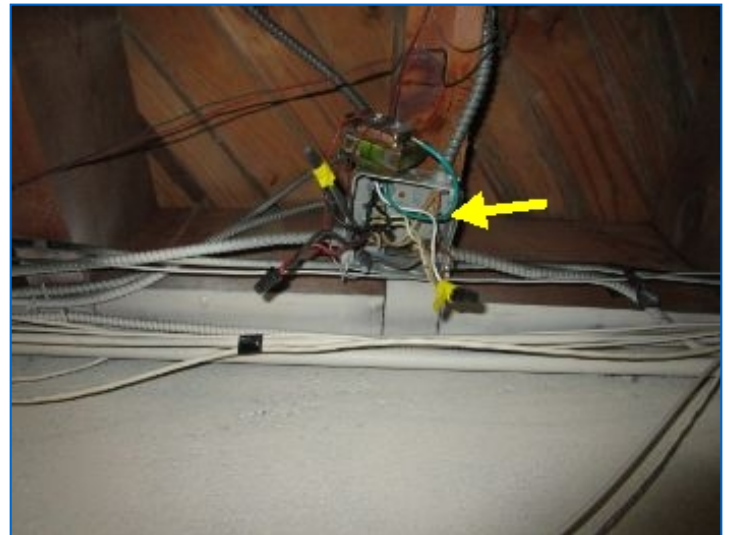
Open junction box observed. This condition is a shock/electrocution hazard. Approved cover plates should be installed by a qualified electrical contractor to prevent direct contact with energized electrical components.
