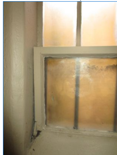
Bathroom window did not open when tested due to frozen latches from lack of use and/or paint layers. Recommend windows be serviced for proper operation prior to close.
