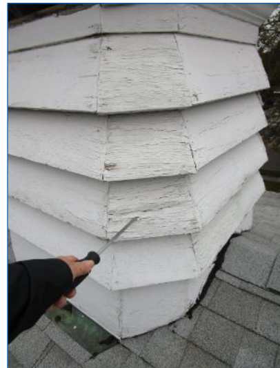
Cupola upper trim piece was missing; potential for wildlife nesting (none noted at time of inspection). Wood softening noted at some louvers of cupola; early signs of deterioration.
