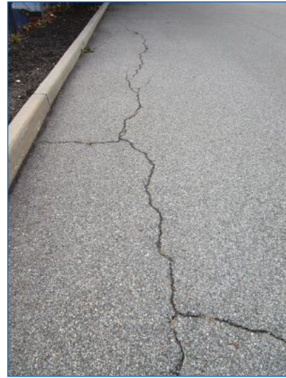
Moderate cracks in driveway. Seal and/or repair cracks to prevent water entry leading to freeze-thaw damage.
