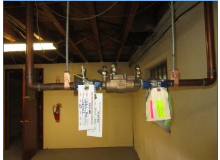
General Area: Backflow preventer noted for sprinkler system/garden hose.
