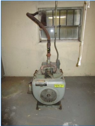
Old defunct engine generator with 30 amp disconnect; no fuel source observed. Recommend removal.
