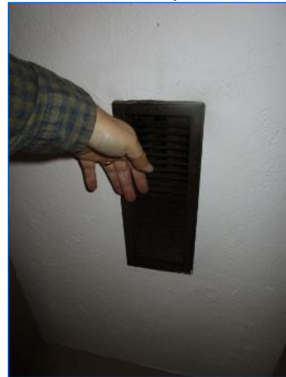
Ceiling register appeared as a supply outlet. No exhaust grille noted.
