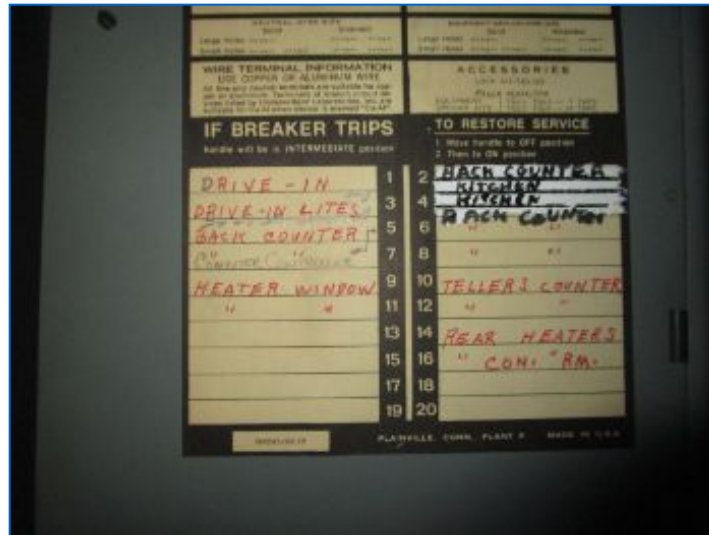
Main Panel #2 Circuit Index noted.
