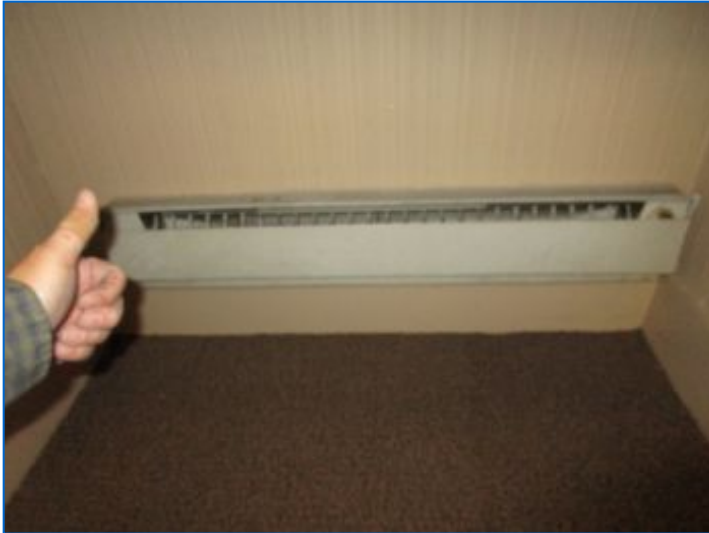
South Viewing Room: Heat distribution types included Electric Baseboard (operable).
