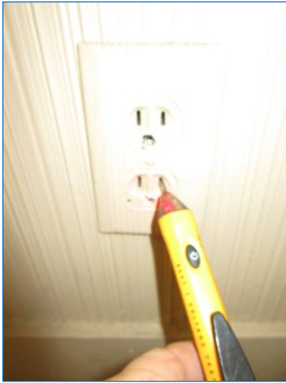
Receptacles were painted over; Active. Recommend replacements by a licensed electrician.
