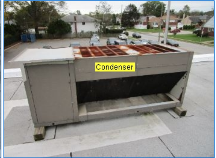
A/C Condenser; corresponding ducted forced air unit located in the Basement.
