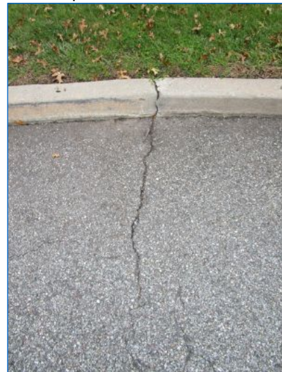
Moderate cracks in driveway. Monitor cracks for the development of trip hazards and have cracks repaired by a qualified contractor.
