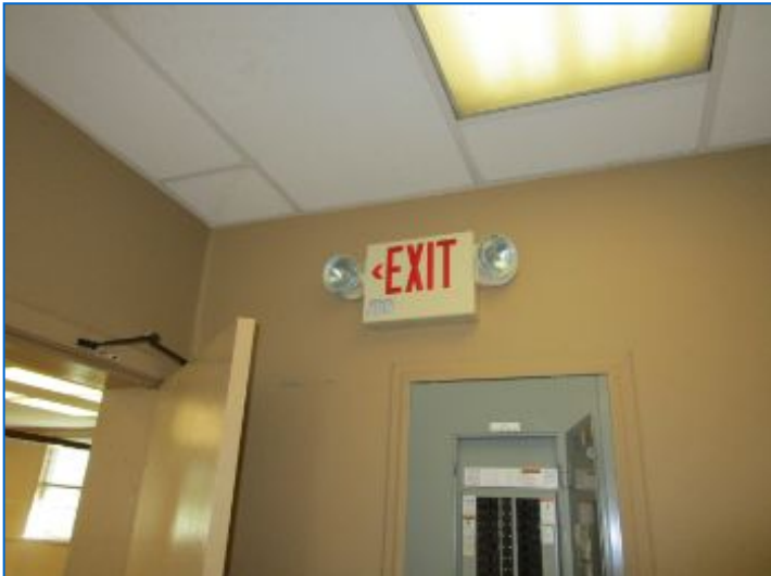
Emergency lighting and exit signs were present, although all were not tested at time of inspection.
