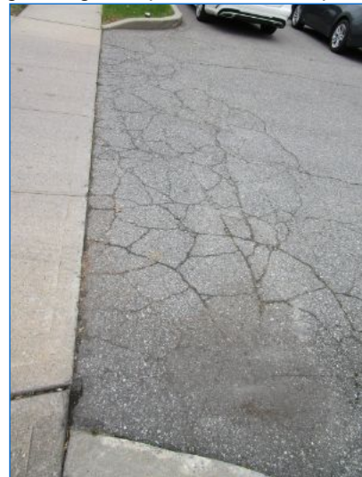
Moderate alligator cracking noted which is a load associated structural failure. The failure can be due to weakness in the surface, base or sub grade; a surface or base that is too thin; poor drainage or the combination of all three. It often starts in the wheel path as longitudinal cracking and ends up as alligator cracking after severe distress. The Fix: Because a structural failure is taking place the only possible solution to alligating is to perform a full-depth patch.
