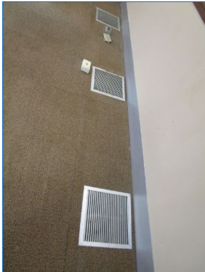
Floor return grilles noted.
