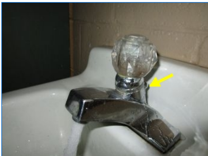
Lavatory faucet leaks from handle; Recommend faucet repair or replacement.
