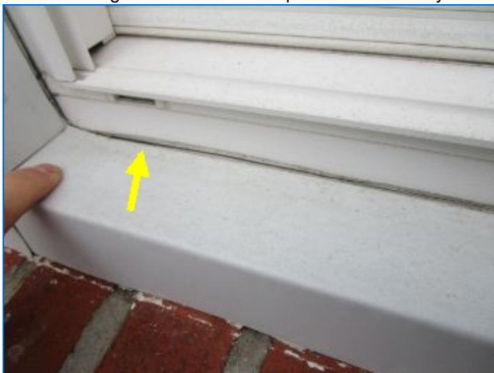
MAINTENANCE: Recommend updating caulking at window frames as needed to prevent water intrusion.
