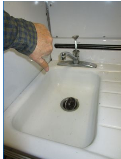
Cafeteria Pantry: Kitchenette was inoperable.
