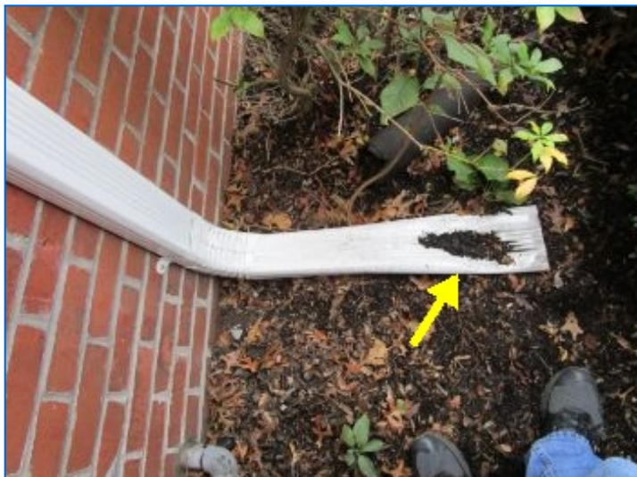
Crushed downspout extension noted at east side. Recommend extending downspouts 4 ft minimum where possible to divert run-off away from the structure to prevent water seepage through the foundation.
