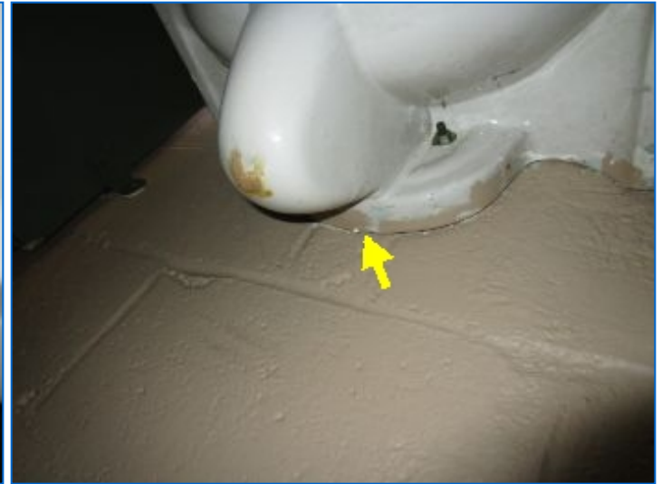
Visible drip leak under the urinal. Source of existing leak could not be determined; Recommend qualified plumber evaluate and repair.
