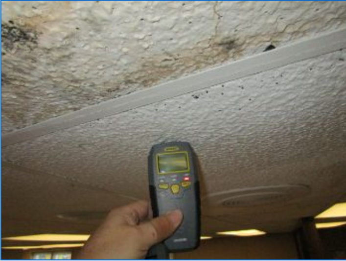
Signs of a roof leak. Moisture detected with signs of mold observed at two ceiling tiles at noted roof leak.
