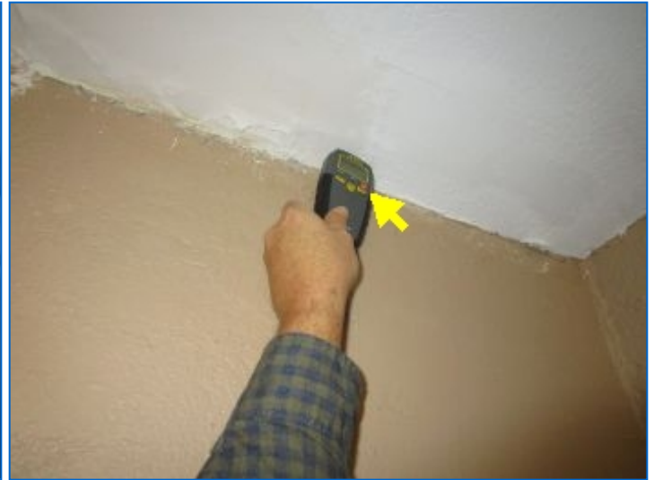
Moisture damage noted at ceiling along west wall; active moisture intrusion - wet condition noted. Refer to related comments in Grounds- Grading section. Recommend corrective repair by a licensed qualified contractor.
