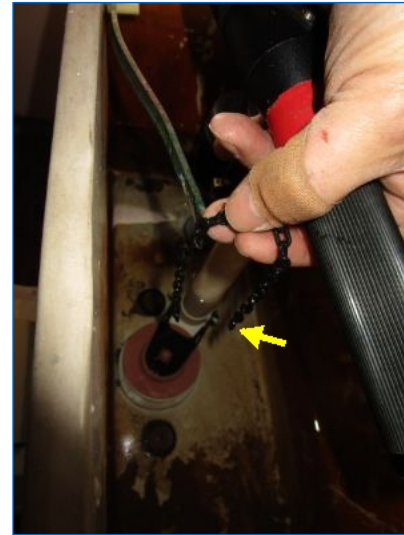
A toilet flapper chain was broken/disconnected; pulled chain to flush. Recommend repair.
