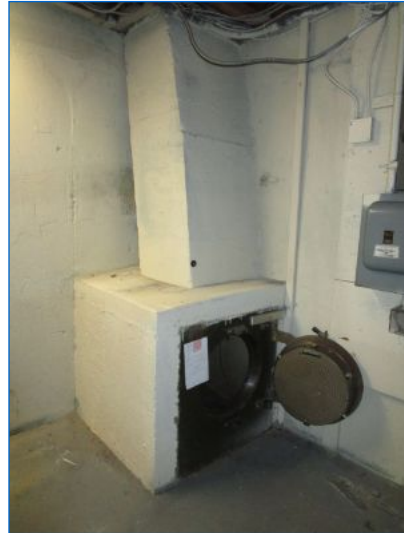
Safe in Utility room.
