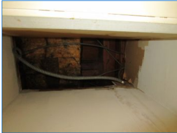
Bank Admin: Closet ceiling was open to attic.
