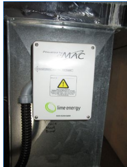
Unidentified and questionable component mounted to HVAC system return duct.
