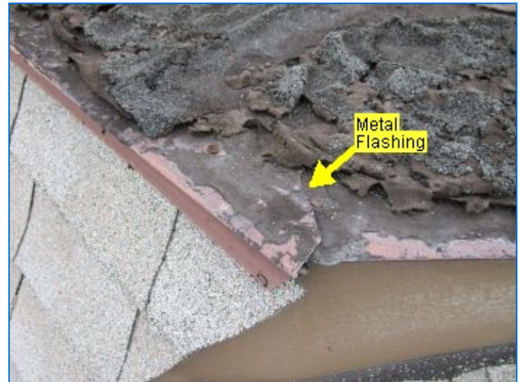
Roof over bank pneumatic tube conveyor consisted of architectural shingles, metal cap flashing and asphalt roll roofing. Asphalt roll roofing was deteriorated exposing the underlying cap flashing; conditions that potentially leak noted here.
