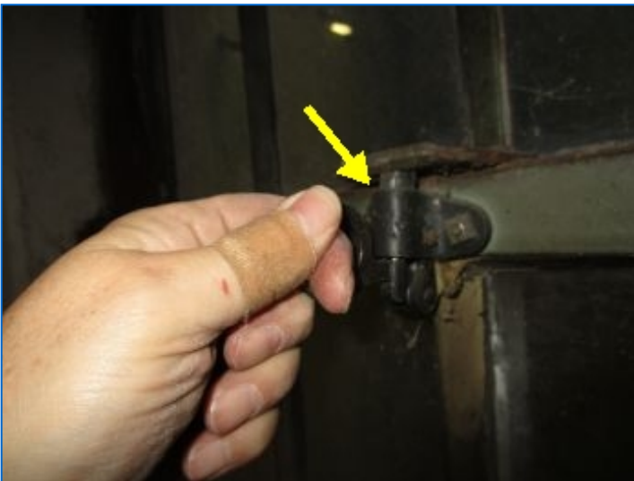
No basement windows opened when tested due to frozen latches from lack of use and/or paint layers. Recommend windows be serviced for proper operation prior to close.
