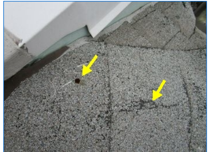
Some exposed nail heads noted on roofing material. Recommend sealing all fastener heads. Miscellaneous minor damage and cracked shingles noted. Suggest review and repairs by a qualified contractor.
