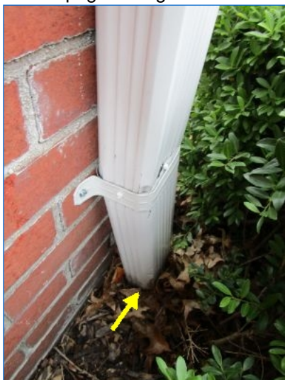
Downspout at East side drains to underground drainage system/drywell; Recommend lowering soil level to prevent dirt/debris from entering and clogging drainage system.
