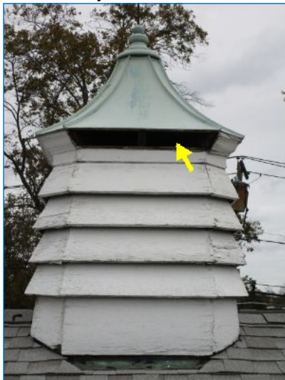
Cupola upper trim piece was missing; potential for wildlife nesting (none noted at time of inspection). Wood softening noted at some louvers of cupola; early signs of deterioration.
