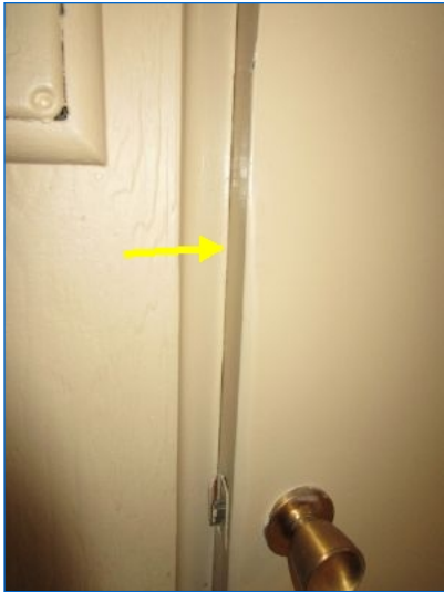
Cafeteria: Doors hit frame; didn't close properly. Suggest adjustment, repair or replacement if necessary.
