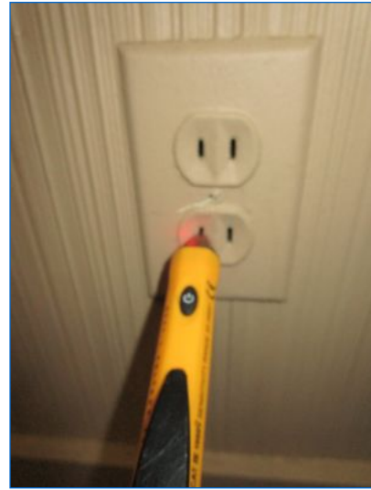
Several receptacles are the outdated, ungrounded 2-prong electrical outlets. Recommend having an electrician update these to meet generally-accepted current standards (grounded 3-prong outlets).
