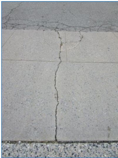
Moderate crack in concrete driveway. Repair or replace damaged areas as necessary to prevent trip hazards. Seal or repair cracks to prevent water entry that will cause further freeze-thaw damage.
