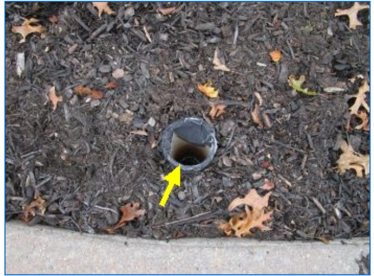
Apparent drain connection to underground drywell at NE planting bed was left unprotected from organic debris entering and causing clogging. Recommend adding screen or cap to protect.
