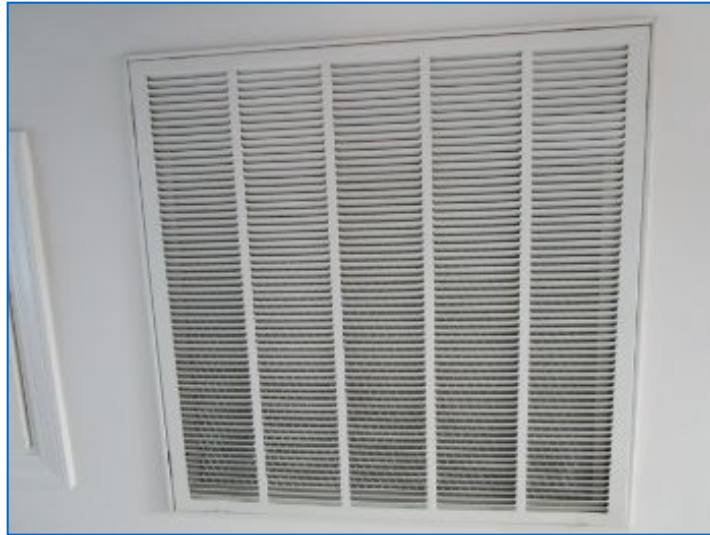
AC#1&2 Combined: Disposable filter located in filter-grille at Hallway (2nd floor) ceiling.
