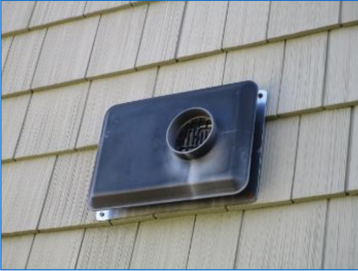
Combination inlet and exhaust boiler vent noted at South wall.
