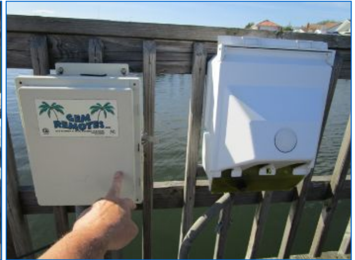
Boat lift control panel and marine sub panel at dock gangway.
