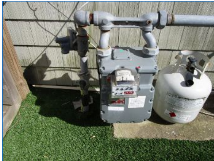
Public Gas Service: Outside meter w/shutoff valve and vented regulator noted.
