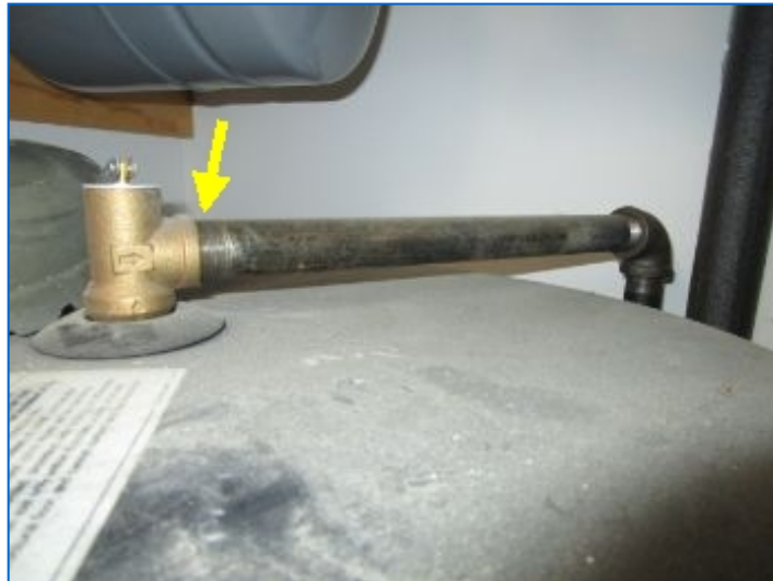
Temperature Pressure Relief (TPR) valve and discharge pipe showed no deficiencies.
