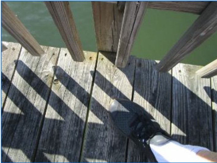
Several plank fasteners had failed at dock gangway, resulting in loose planks. Recommend corrective repairs.
