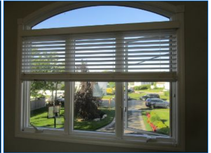
Screens missing or not installed at the time of inspection.
