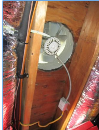
Thermostatically controlled Power Ventilator was operable. Recommended Temperature setting is 85 deg F.
