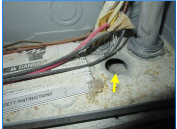
Unused Conduit Knockout should be blanked off to prevent mice from entering the panel box.
