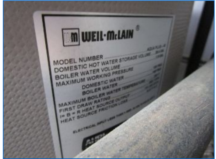
Weil McLain 39 gallon capacity unit. Water Heater Storage Tank data plate/serial no. indicates a manufacture date of 4/2014, (6 yrs old).
