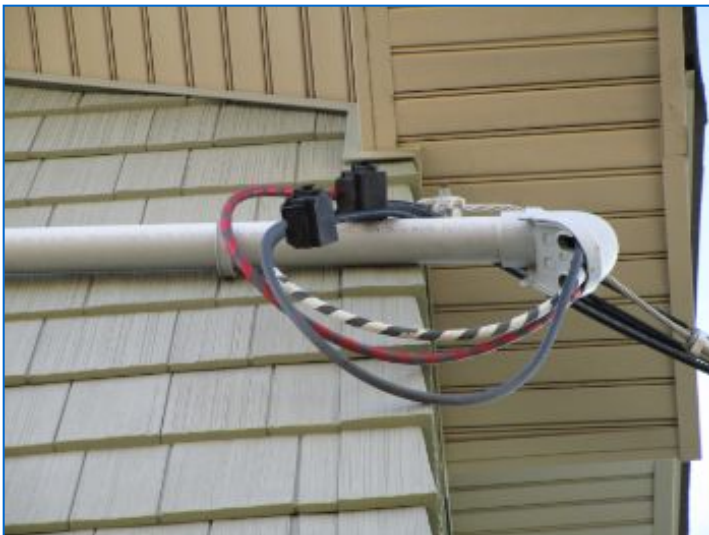
Overhead electrical service drop and riser showed no system safety or function concerns at time of inspection.
