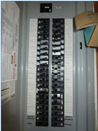
Main Panel Breakers: 40 full-size circuit breaker spaces; 0 spare breaker space/s noted; 1 breaker/s in the Off/Tripped position.
