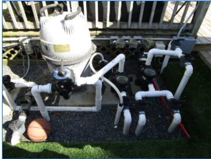
Pool filter was operational at the time of the inspection.
