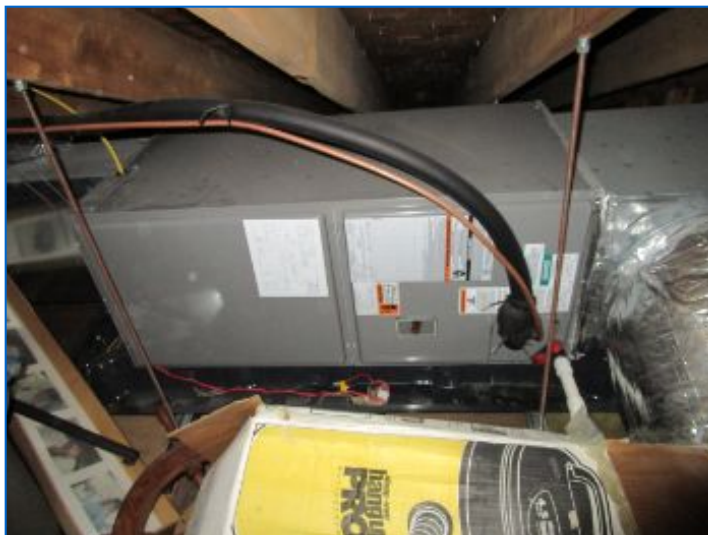
Ducted Air Handler (AC#2) located in Attic.
