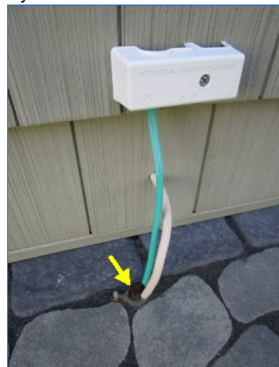
Ground conductor to ground rod noted at service entrance per current standard.
