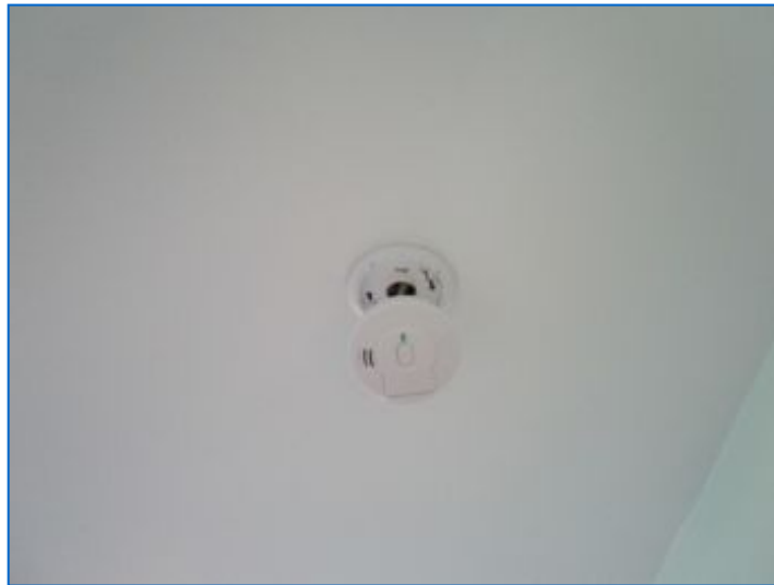
Smoke detector was not properly secured.
