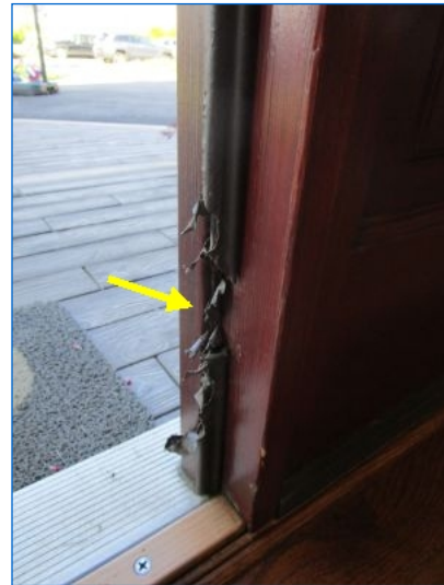
Weatherstripping damaged at front door. Suggest repair.
