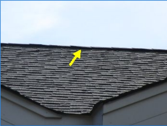
Ridge exhaust venting noted for attic ventilation.
