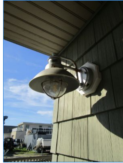
Light fixture or bulb/s apparently inoperable. Change bulb/s and check.
