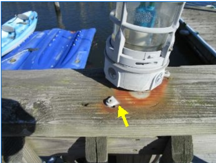
Surface mounted light fixture had a broken mount.
