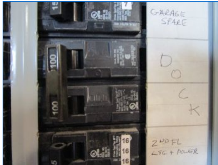
Sub Panel Disconnect: 100 amp main breaker located in the Main Panel.
