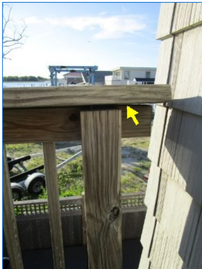
Top rail of guardrail had separated from the post.
