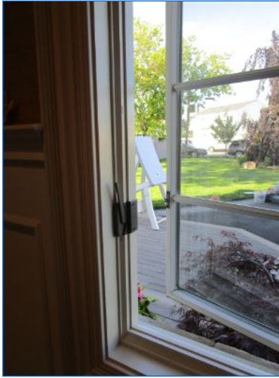
Screens missing or not installed at the time of inspection (check attic).
