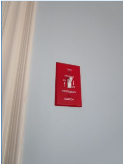
Gas Burner: Remote Emergency Shut-off switch noted.
