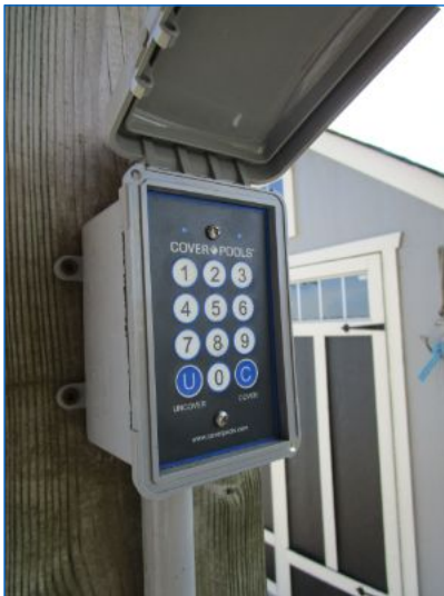
Automatic pool cover control pad noted.
