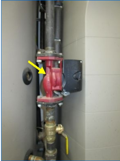
One pump is dedicated to water heater storage tank.
