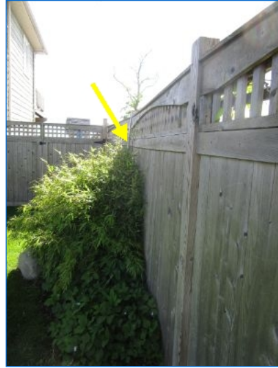
Fence was leaning in one post area.
