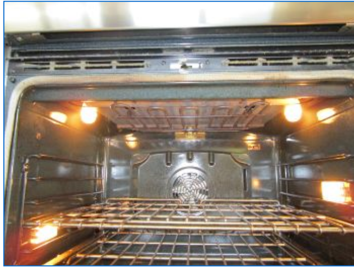
Electric powered built-in oven; appeared operable at time of inspection.
