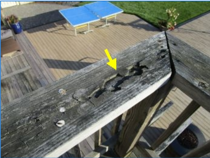
The top rail of the guardrail exhibited moderate deterioration and localized decay. Suggest replacing damaged wood.
