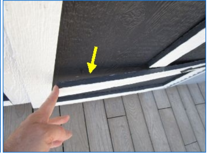
Loose/detached plank noted at shed door.
