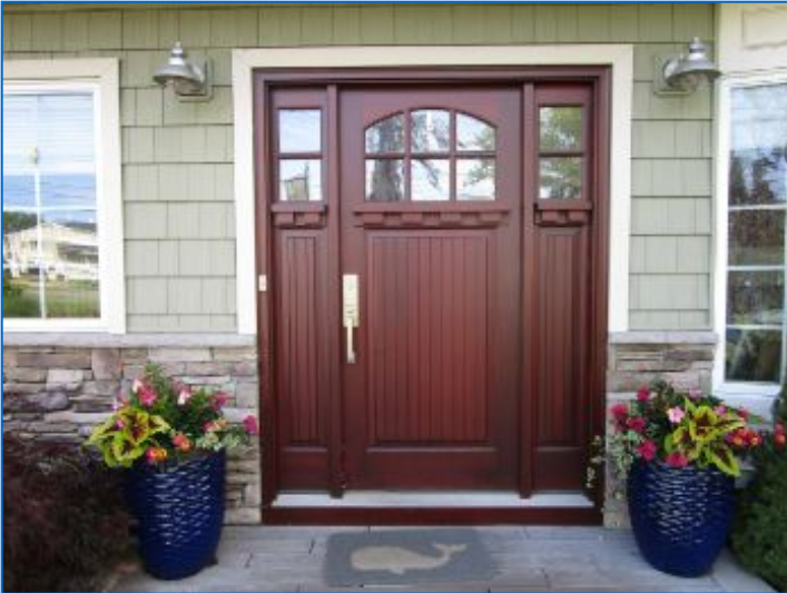
Front doorbell operated normally when tested.
