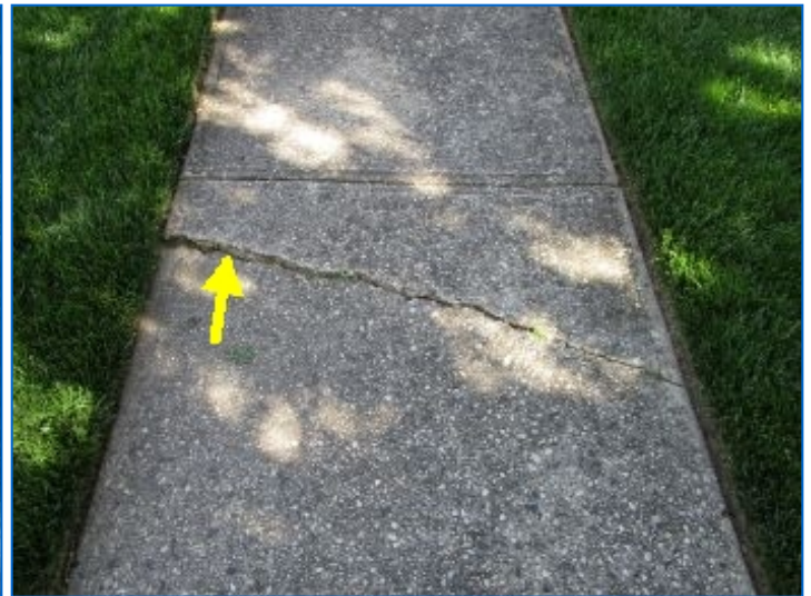
Potential Trip Hazards noted at sidewalk; repair as necessary.
