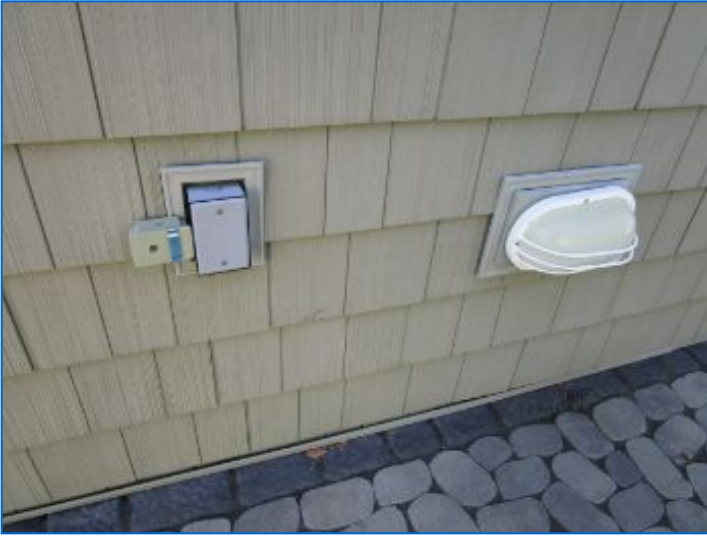
Some exterior lighting controlled by dusk/dawn sensors.
