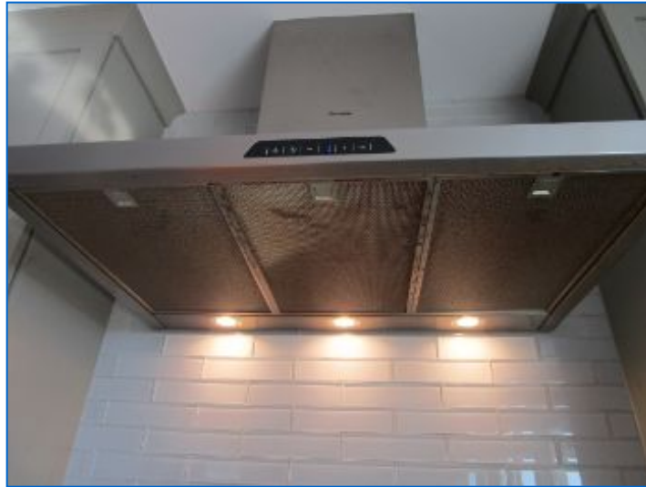
Exterior vented type hood fan with grease filter and light was operable.
