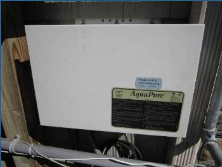
AquaPure Salt Chlorine Generator noted.
