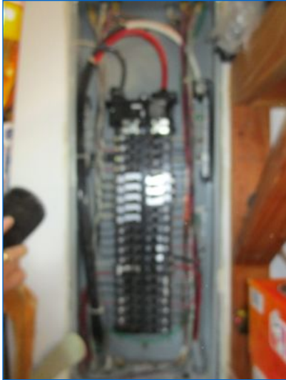
Main panel interior checked.
