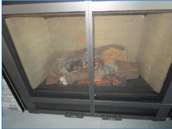
Gas-burning fireplace in the Living room was operable.
