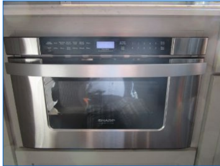
Drawer type microwave was operable at time of inspection.
