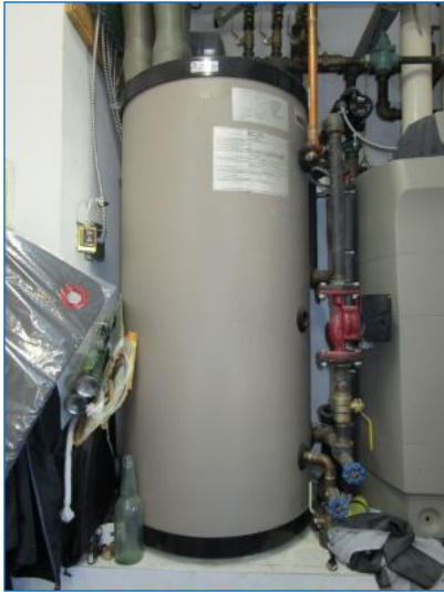
HW Storage Tank, integral with heating system (indirect-fired) was operable.
