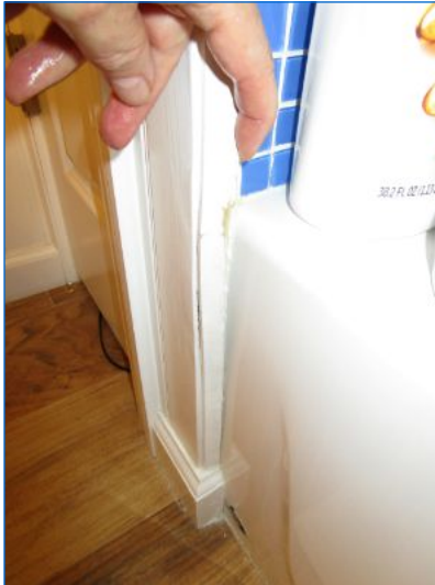
Wood at tub molding was moisture damaged; recommend repair.
