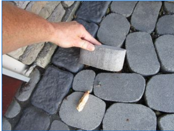
Loose unfitted pavingstone noted at front in non-mortared area where the house trap was buried.
