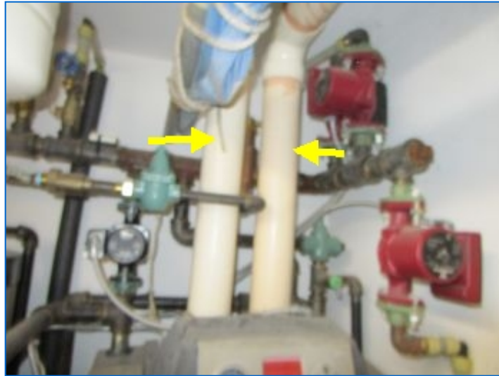
Visible portions of the vent pipes appeared functional.
