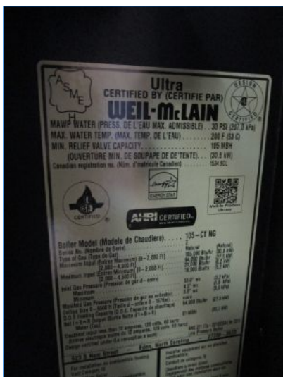
Boiler data plate indicated an input heating capacity of 105,000 Btu/hr.
