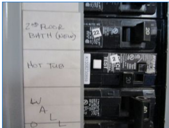
Main Panel 20 amp breaker labeled "Hot Tub" was in the Off/Tripped position.
