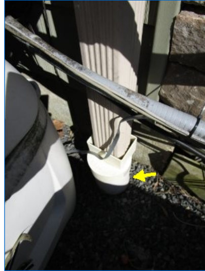
Downspout connected to underground drainage system; drywell/s.
