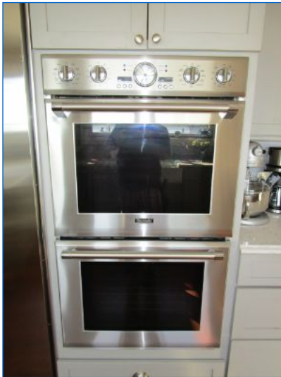
Electric powered built-in oven; appeared operable at time of inspection.
