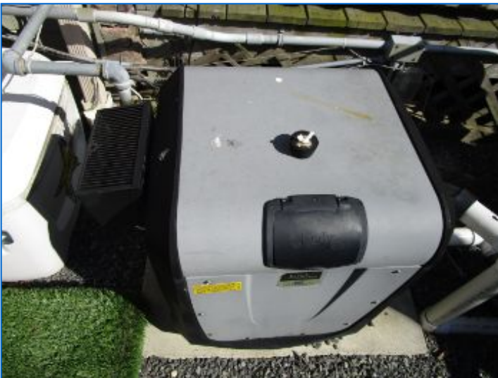
Jandy Pool Heater (gas-fired) was off at time of inspection. Suggest seller demonstrate operation at final inspection.
