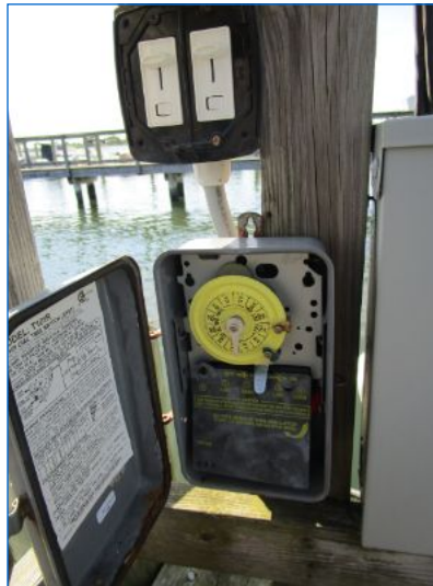
Dock lighting timer/switches at NW corner of bulkhead
