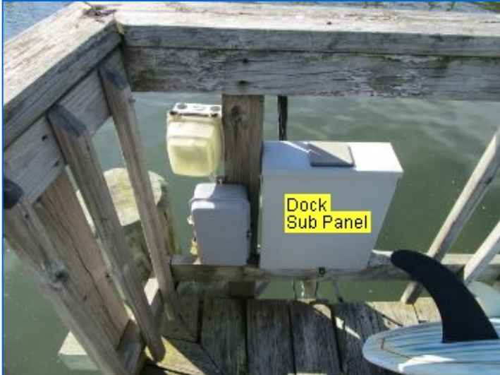
Dock sub panel and lighting timer/switches noted at NW corner of bulkhead.
