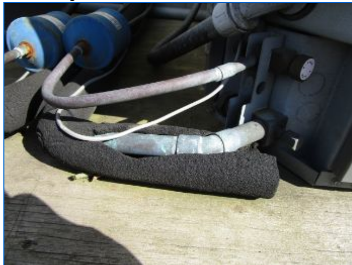
AC#1 section of outdoor refrigerant pipe insulation to outdoor condenser was Deteriorated/Missing. Recommend repairing defective insulation for the larger suction line.
