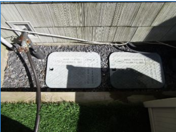
Property is equipped with an underground sprinkler system.
