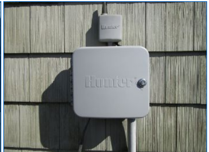
Control panel for sprinkler system located at the north exterior.
