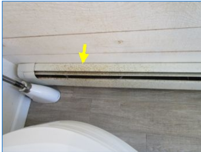
Baseboard enclosure had rusted finish.
