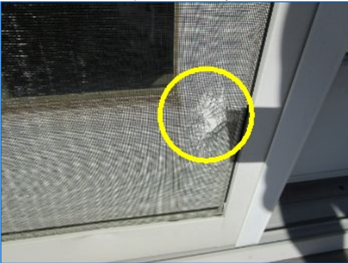
Sliding door screen was damaged at rear sliding door to den. Suggest repair.
