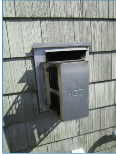
Gas fireplace direct vent noted at North exterior wall.
