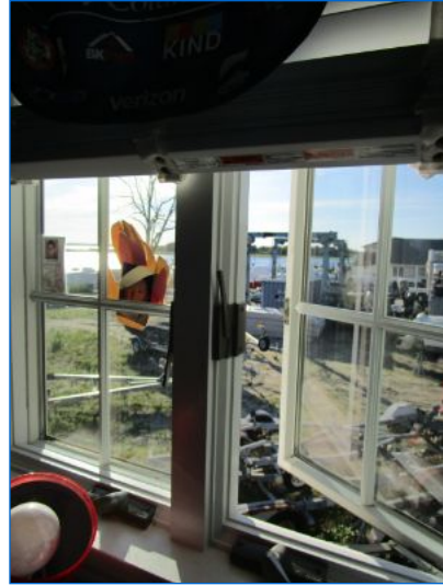
Screens missing or not installed at the time of inspection.
