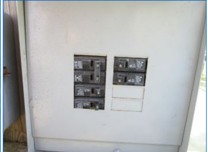
Dock Sub Panel located at NW corner of bulkhead. Sub Panel Disconnect: 100 amp main breaker located in the Main Panel. Sub Panel Breakers: 8 full-size circuit breaker spaces; 2 spare breaker space/s noted; 0 breaker/s in the Off/Tripped position.
