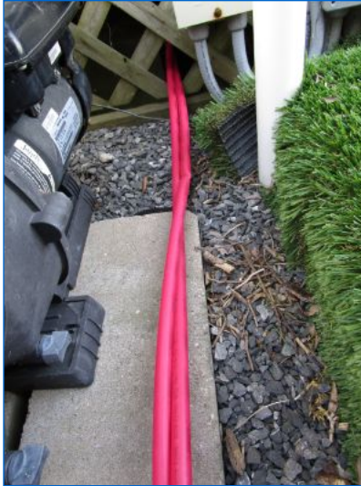
Unused PEX tubing coming from under the deck.
