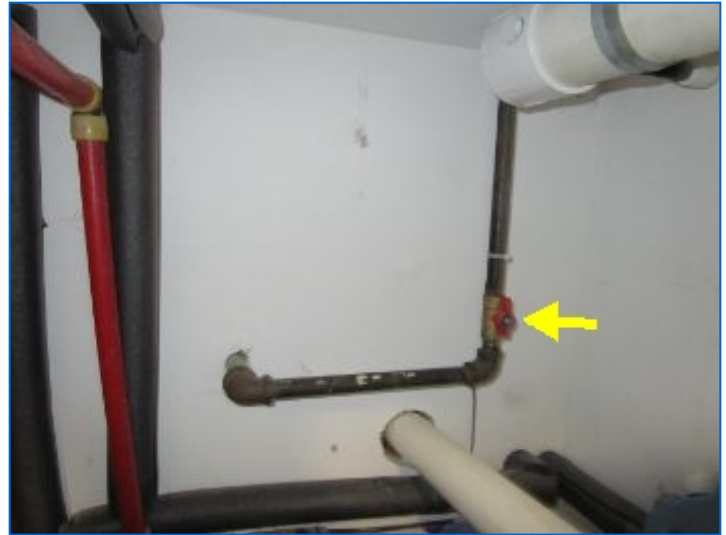
Gas shut-off valve noted at burner.
