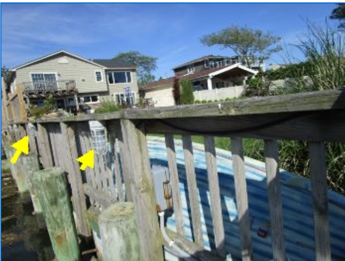
Bulkhead light fixtures appeared operable. Not all bulbs worked. Change bulb/s and check.
