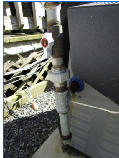
Gas shut-off valve and proper drip leg noted at burner.
