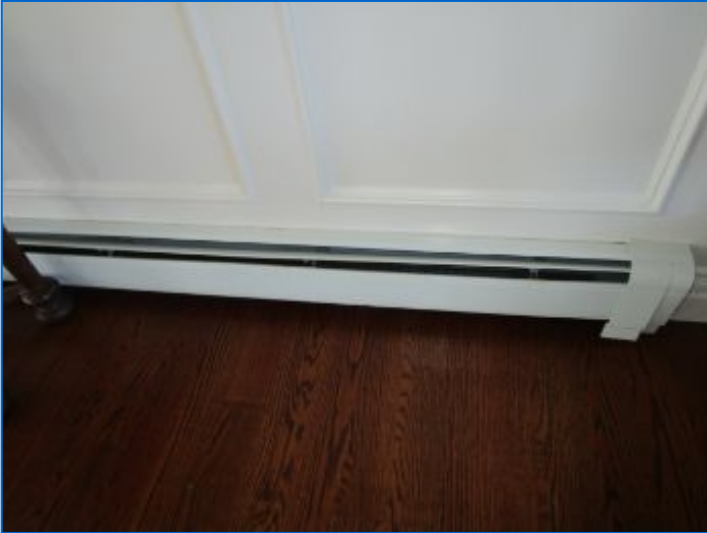
Heat distribution type/s included Baseboard.
