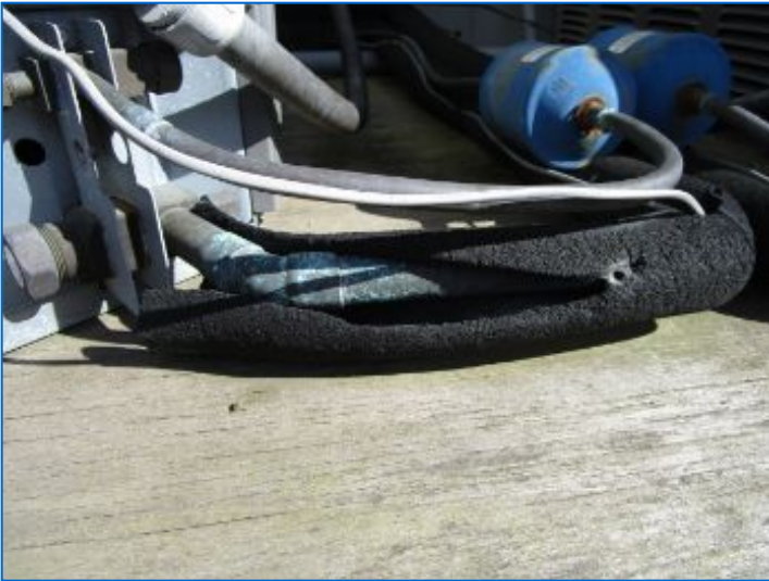
AC#2 section of outdoor refrigerant pipe insulation to outdoor condenser was Deteriorated/Missing. Recommend repairing defective insulation for the larger suction line.
