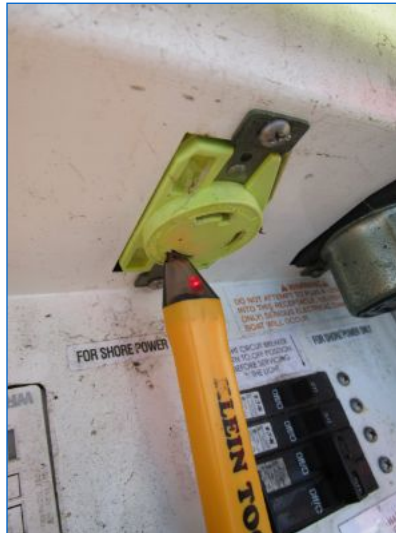
Marine sub panel at dock gangway was powered at time of inspection.
