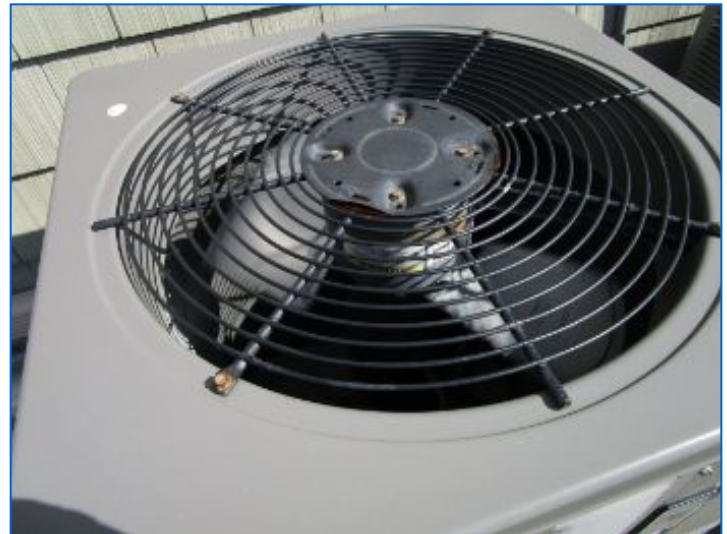
A/C systems operated and appeared functional at the time of inspection.
