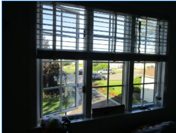
Screen missing or not installed at the time of inspection.
