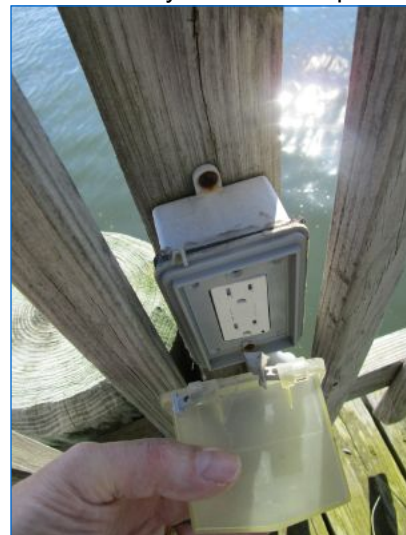
Exterior receptacle weatherproof cover was defective at non-WR GFCI receptacle.
