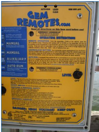
Boat lift control panel appeared functional at time of inspection.
