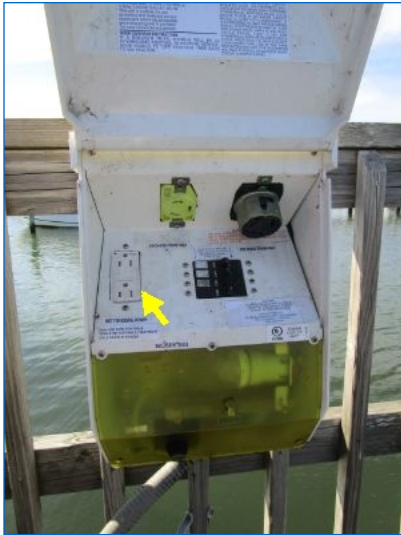
Marine sub panel at dock gangway. GFCI receptacle did not appear to have power when tested; possibly due to oxidation.
