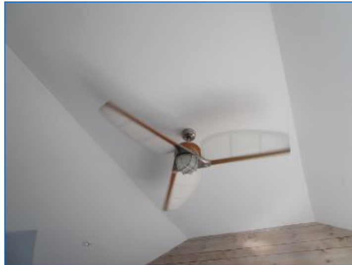
Ceiling fan operated normally when tested at time of inspection.
