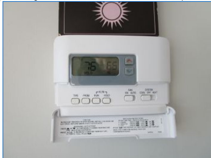
Digital Programmable type thermostat noted in Master bedroom; for Heating only.
