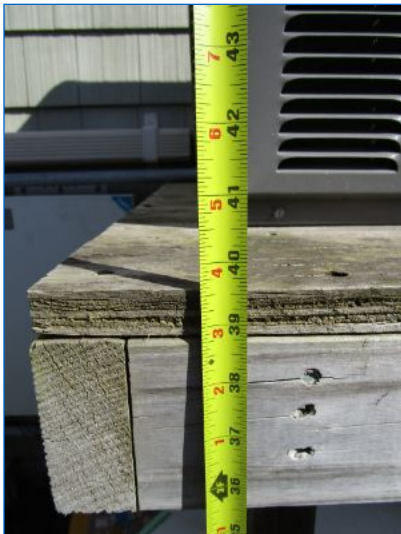
Coastal Areas: The most effective flood-resistant design for outdoor HVAC equipment is to strap or bolt the equipment onto a platform above the Design Flood Elevation (DFE).
