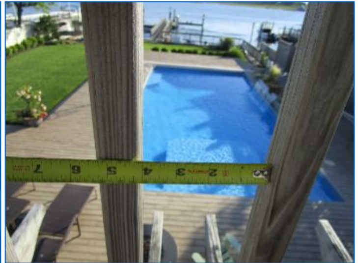
Spaces between deck guardrail balusters were too wide. Safe building practices dictate that a 4 inch sphere may not pass through the handrail at any point. This condition is hazardous to small children. Recommend that this condition be updated to meet generally-accepted modern safety standards by a qualified contractor.
