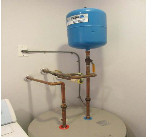
IMG_0292.JPG Water heater supply shutoff valve and expansion tank noted.
