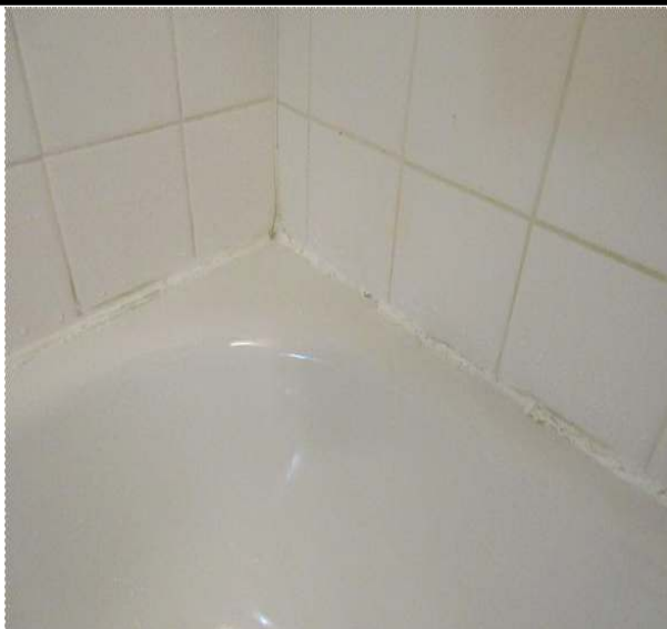
IMG_0282a.JPG Full Bathroom: Shoddy (but functional) silicone caulking job at tub perimeter.
