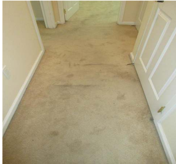
IMG_0302.JPG Hallway carpet is loose; trip hazard.
