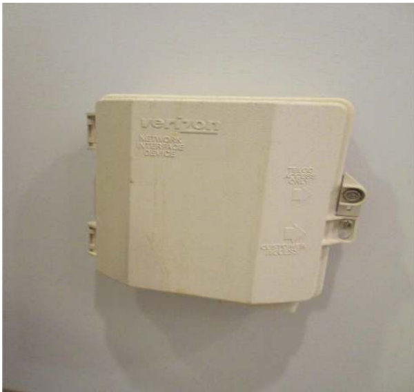
IMG_0284.JPG Verizon cable connection noted in the laundry/utility room.
