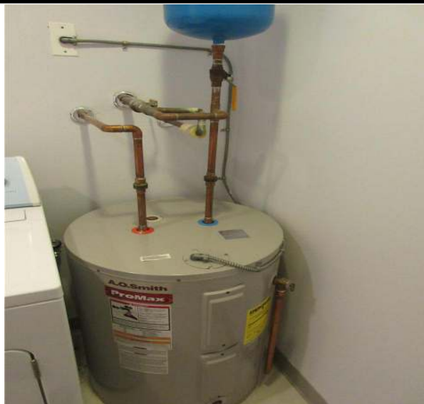
IMG_0288.JPG Electric A.O Smith electric water heater.
