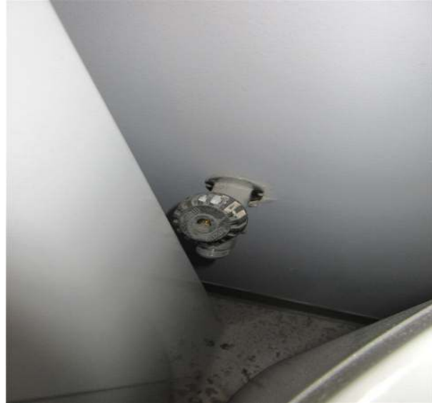
IMG_0293.JPG Hose bibb at wall behind clothes dryer.
