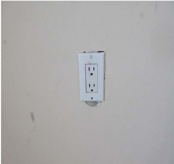
IMG_0301.JPG Cosmetic damage around wall outlet in living room.l
