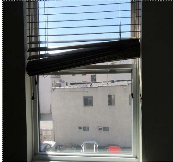
IMG_0271a.JPG Living room window blinds appear defective.
