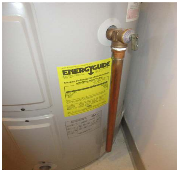
IMG_0291.JPG Water heater has the required relief valve with extension pipe.
