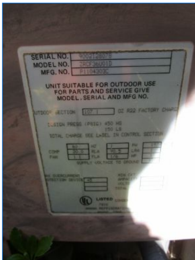
AC#1 Amana Condensing Unit data plate/serial no. indicates a cooling capacity of 3 tons, and a manufacture date of 2/1990, (29 yrs old).
