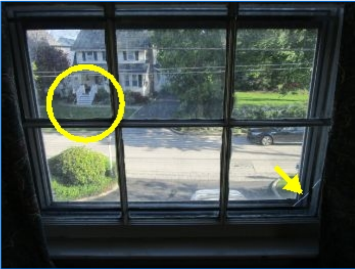
A window in the Office had cracked panes. Repair to prevent injury.
