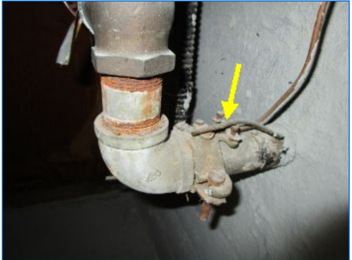
System Grounding: Ground wire connection noted at inlet-side of meter only; ground missing at outlet-side of meter. Suggest having licensed electrician ensure that plumbing system grounding is adequate.
