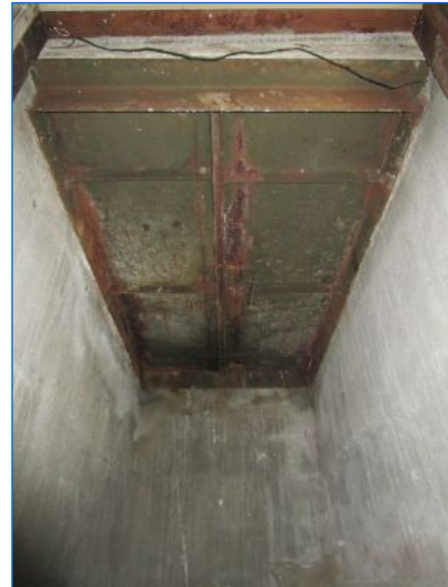
Basement extension under garage with steel access doors above. Doors showed signs of rust but appeared operable.
