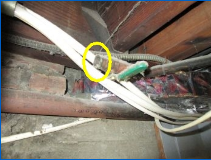
Uncapped supply valve noted in basement. All water pipes not supplying a fixture must be properly terminated/capped to prevent possible water damage and or personal injury from scald burns if valve is accidentally operated.
