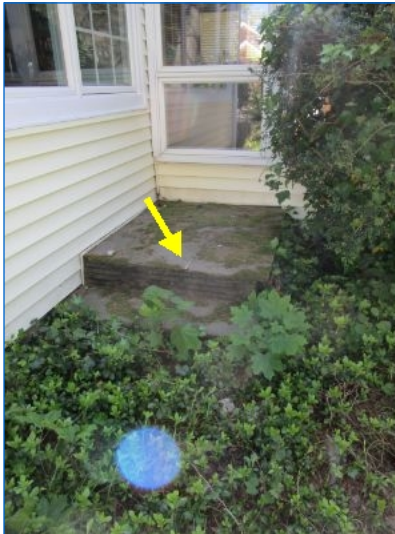
Abandoned steps noted at rear; confer with seller.
