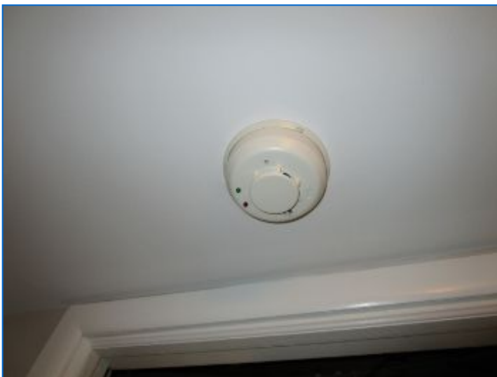
Smoke/Carbon Monoxide Detector noted in vicinity of furnace room. Maintain functioning Smoke/Carbon Monoxide detectors as recommended. Detectors are generally reliable for up to 5 yrs.
