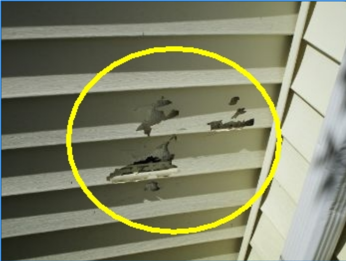
Cosmetic damage/s noted at Front siding by an unknown cause. Repair and seal all openings in siding to prevent water intrusion into the structure.
