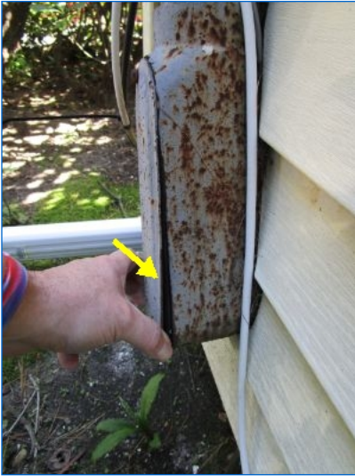
Cover at LB conduit body was note secured/sealed; recommend repair.
