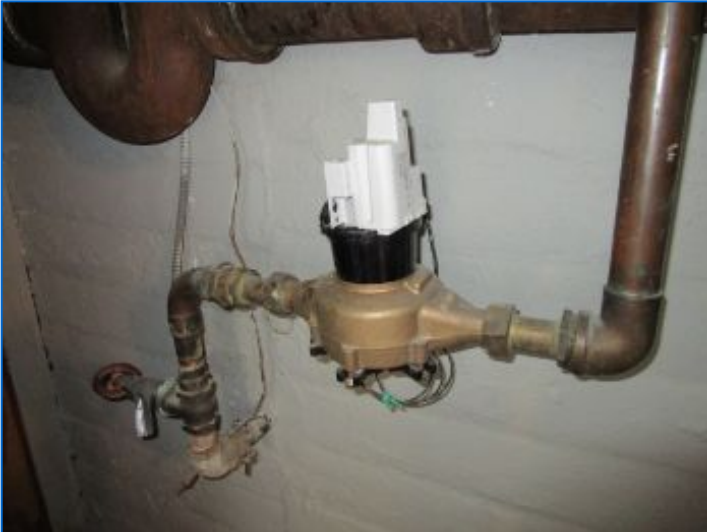
Water Service Entrance: 1" Galvanized line entering with meter and shutoff valve/s.
