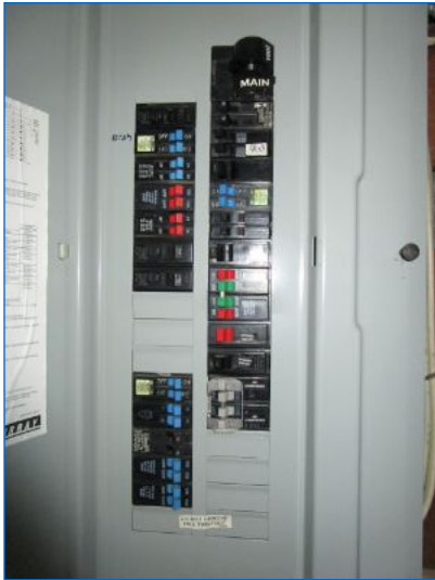
Main Panel Breakers: 32 circuit breaker spaces; 8 spare breaker space(s) noted.
