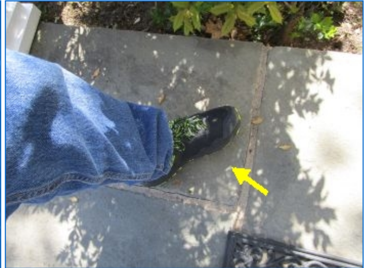
Deteriorated/cracked mortar at two Bluestone tiles at front steps/landing; loosening tiles noted. Recommend repairs to eliminate potential trip/fall hazard.
