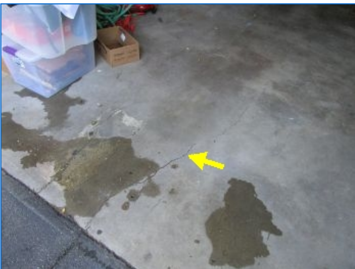
The garage floor had common settlement type cracks. These cracks are not a structural concern.
