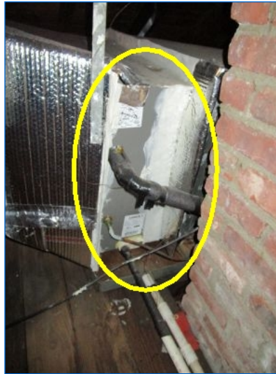
AC#2 Cooling coil (Lennox) integrated into ducted forced air furnace located in Attic (installed in conjunction with AC#2 condenser).
