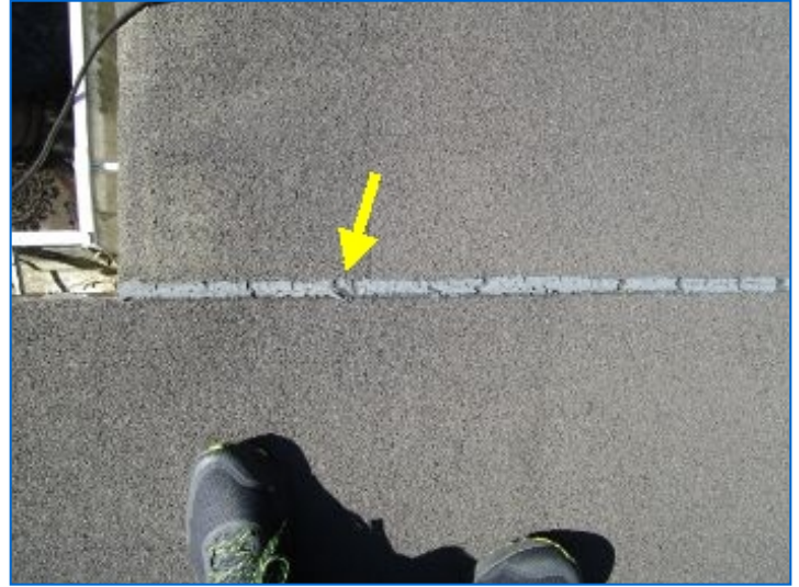
Mastic sealant along roof seam appeared to be in need of maintenance. Recommend hiring a qualified licensed roofing contractor to review and provide the necessary maintenance. Inspecting and re-sealing seams in roofing is a part of routine maintenance to prevent water entry.
