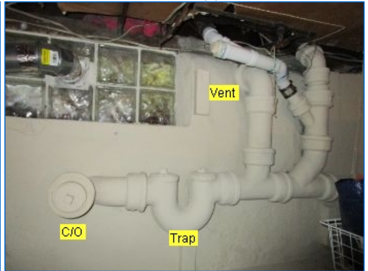
Waste Pipe Exit #1 located at the Southwest side of the house/basement includes whole-house trap w/vent and clean-out fitting..
