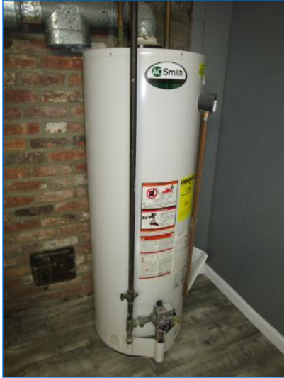
Gas, direct-fired water heater was operable.
