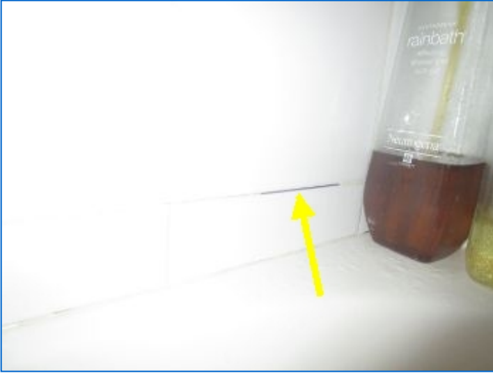
Wall tiles in tub area have damaged/missing grout; suggest re-grouting or adding grout where needed to prevent water damage.
