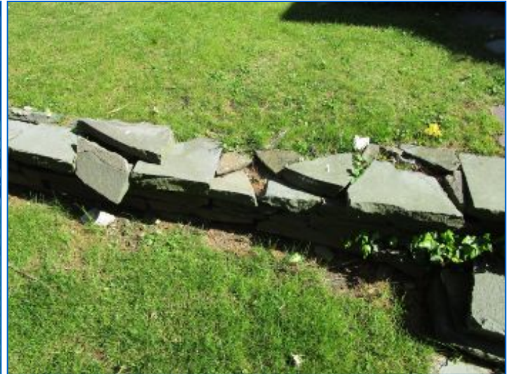
Loose stones creating trip hazards; Recommend review by a qualified professional for repair as necessary.
