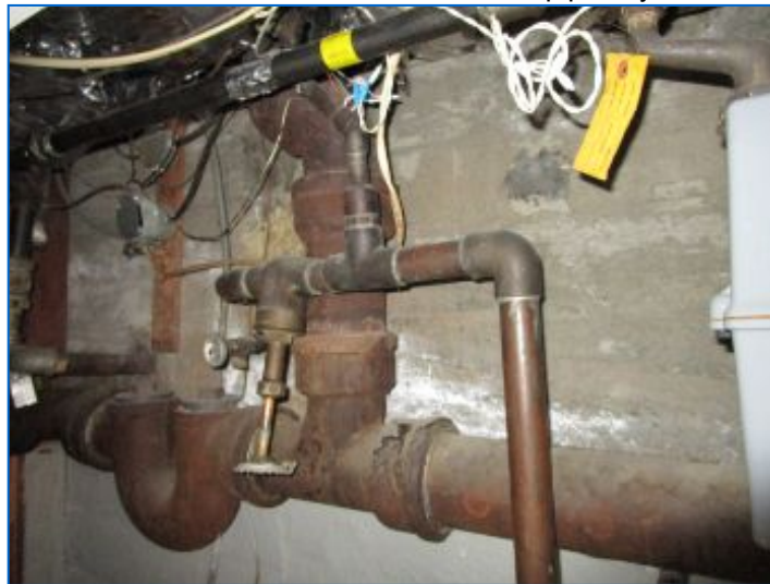
Waste Pipe Exit #2 located at the Southeast side of the house/basement includes whole-house trap w/vent and clean-out fitting..
