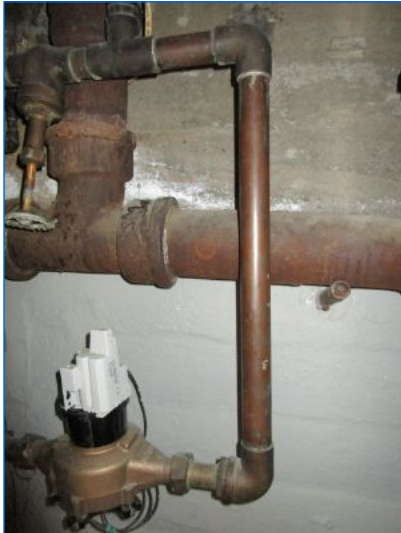
System Grounding: Ground wire connection noted at inlet-side of meter only; ground missing at outlet-side of meter. Suggest having licensed electrician ensure that plumbing system grounding is adequate.
