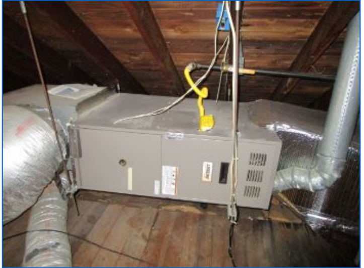
HVAC#2 Forced Air Furnace located in the Attic serves the 2nd floor was operable at time of inspection.
