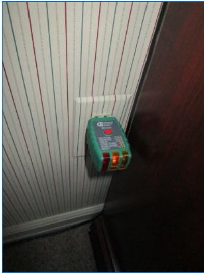
Open ground receptacle noted.
