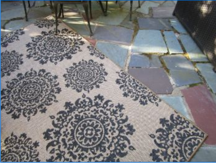
Some cracking of mortar joints; some loosening of slates under carpet noted; Repair to avoid potential trip hazard.
