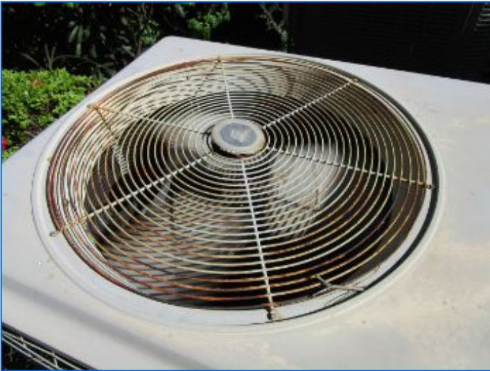
A/C systems 1 & 2 operated and appeared functional at the time of inspection, however the overall performance of the home air conditioning system may not be sufficient during warmer outdoor conditions due to the noted deficiencies.
