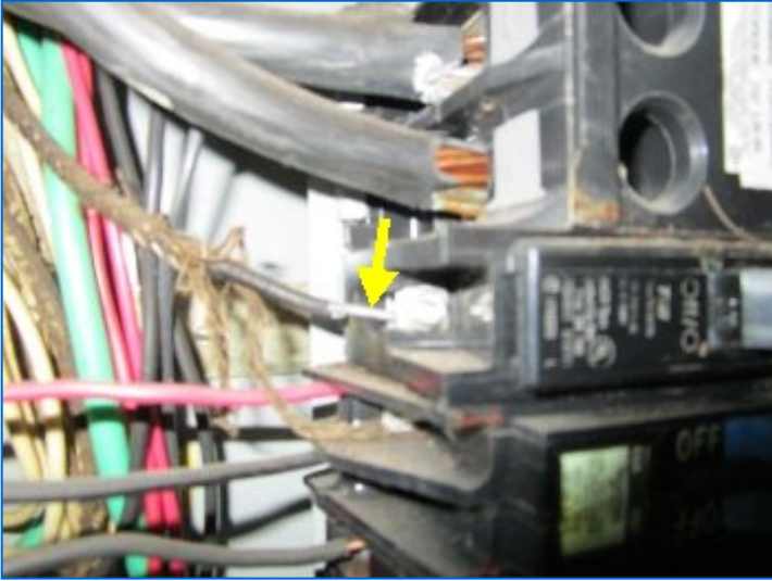
Aluminum wiring present — Recommend review and maintenance be performed by a licensed electrician prior to close.
