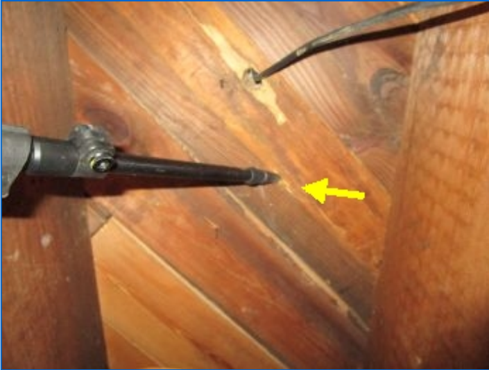
Damage noted from past termite activity at exposed floor boards above ceiling in southwest room of basement. Refer to NPMA-33 Report.
