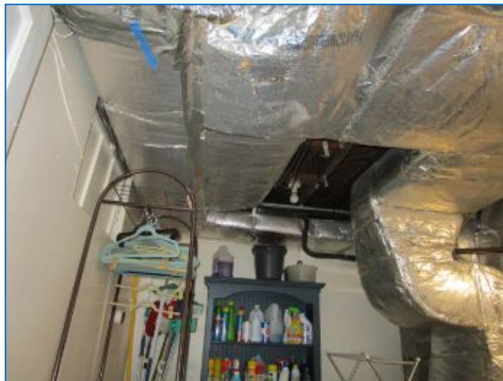
HVAC ductwork was well insulated.
