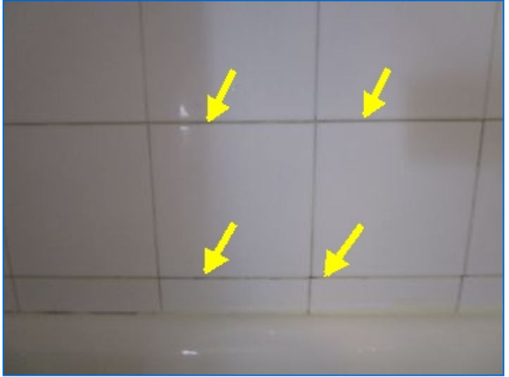
Wall tiles in tub area have damaged/missing grout; suggest re-grouting or adding grout where needed to prevent water damage.
