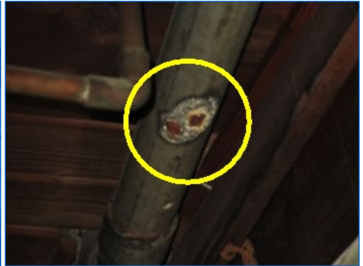
Galvanized DWV pipe corroded through. Recommend evaluation and repair of defective length/s of galvanized pipes by a licensed qualified plumber.
