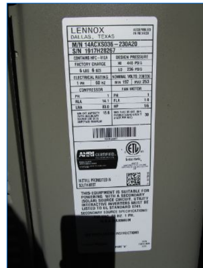
AC#2 Lennox Condensing Unit data plate/serial no. indicates a cooling capacity of 3 tons, and a manufacture date of 8/2017, (2 yrs old).
