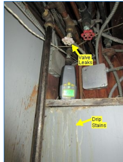
Deposits observed at water valve/s is a sign of leakage and possible valve body corrosion. Suggest evaluation and repair by a qualified plumber.
