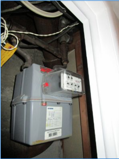
Public Gas Service: Meter w/shutoff valve and vented regulator in Basement.
