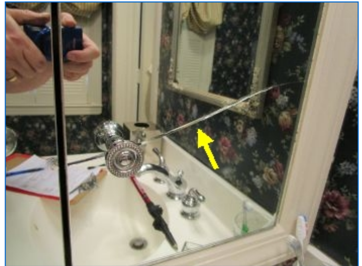
Cabinet mirror was cracked; recommend repair to prevent injury.
