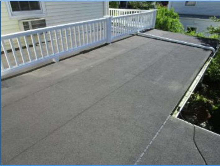
Flat asphalt roof covering showed conditions consistent with 10+ yr old roll roofing.
