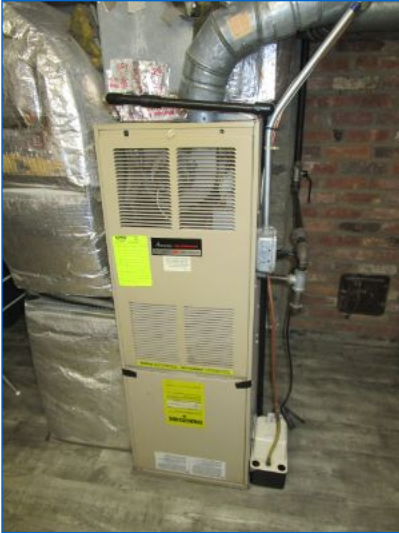
HVAC#1 Forced Air Furnace located in the Basement serves the 1st floor & basement was operable at time of inspection.
