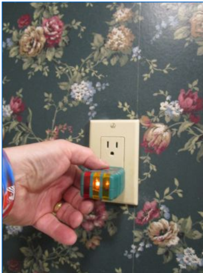
GFCI type receptacle did not trip when tested. Recommend rewiring/replacing GFCI receptacle.
