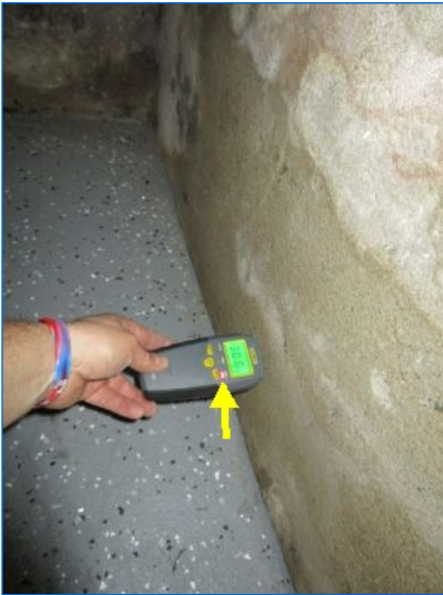
Moisture level tested high at lower part of foundation wall in basement extension under garage.
