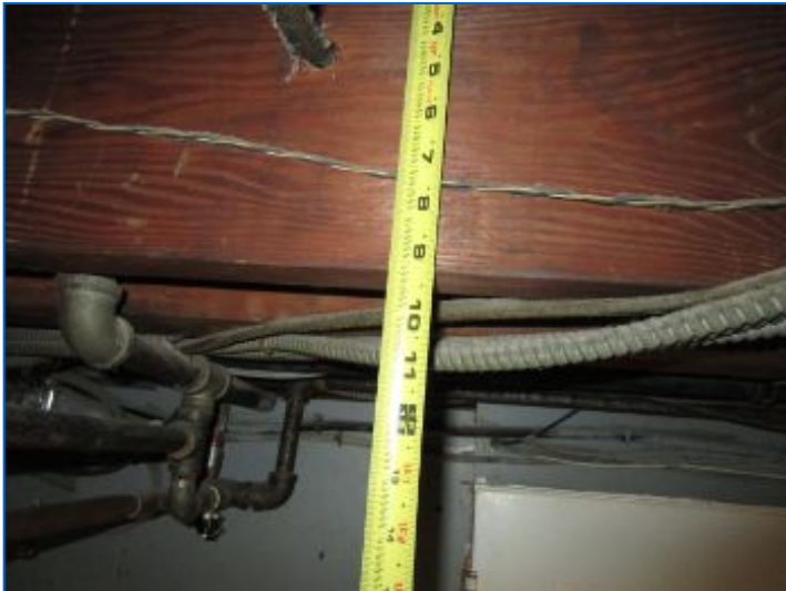
Main Floor Structure: Main beams supported by foundation walls, 2x10 Joists 16" O.C. (w/cross braces), T&G floor boards.
