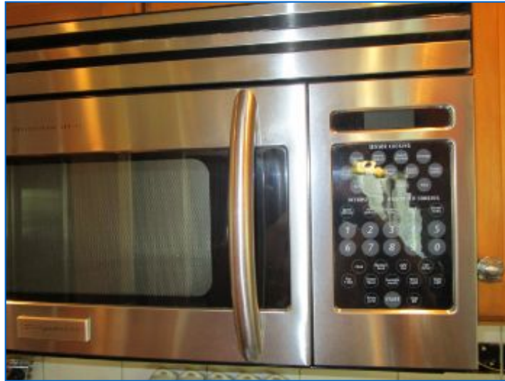
Microwave was operable at time of inspection.
