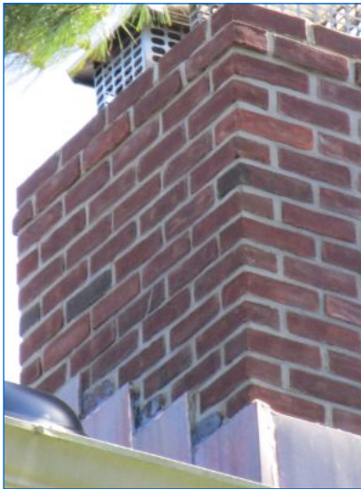
Some areas of the chimney flashing were not visible from inspection level. Suggest roof/chimney contractor inspect further to ensure there's no water intrusion here. From the inspection level, the chimney flashing appeared to be intact and functional.
