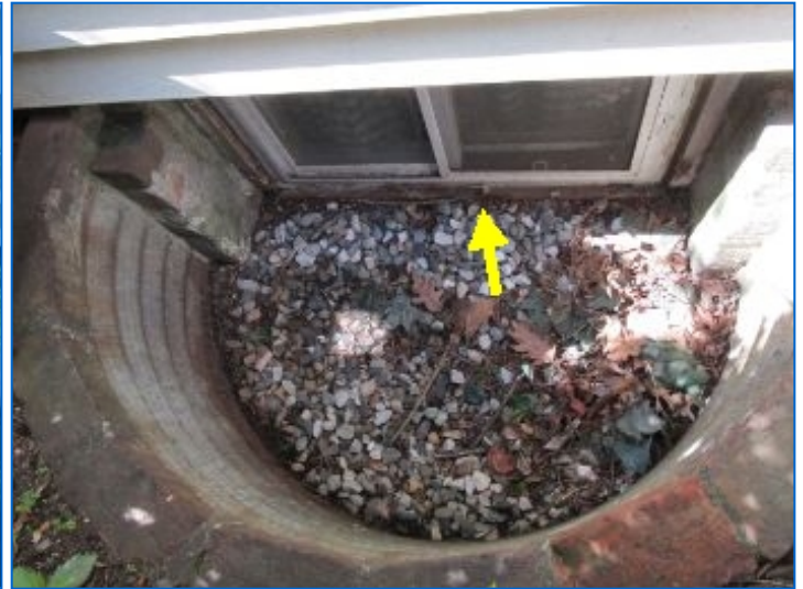
Basement window wood frames in contact with soil showed signs of moisture damage at Front exposure. Recommend regrading soil level to 6 inches below frame; repair and protect wood from further moisture damage.
