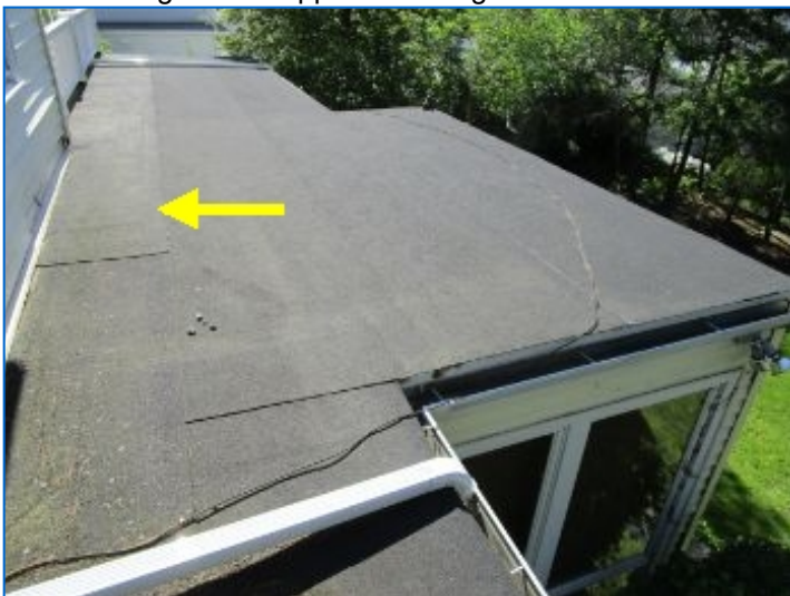
Flat roof, asphalt rolled roof noted (vicinity of Den). Additional layer and/or seam noted here. Refer to Den ceiling section.
