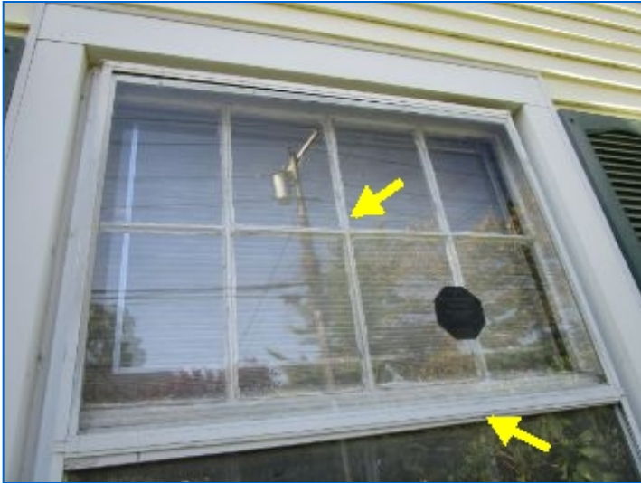
The home had the original Single pane Wood frame windows. Aluminum framed triple-track storm windows noted.
