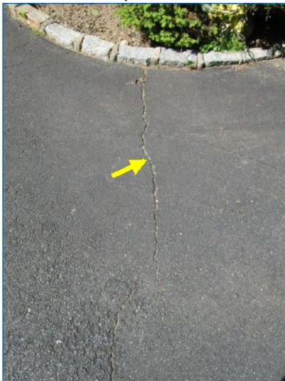
Normal cracks in asphalt driveway. Seal and/or repair cracks to prevent water entry leading to freeze-thaw damage. Monitor existing cracks for expansion.
