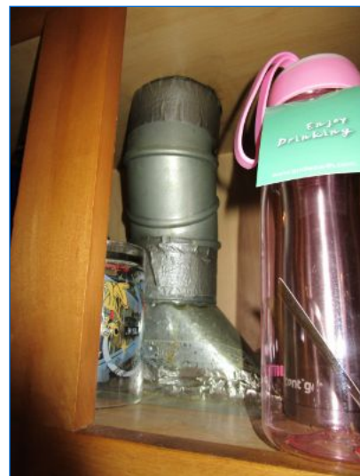
Range hood fan vented to the exterior.
