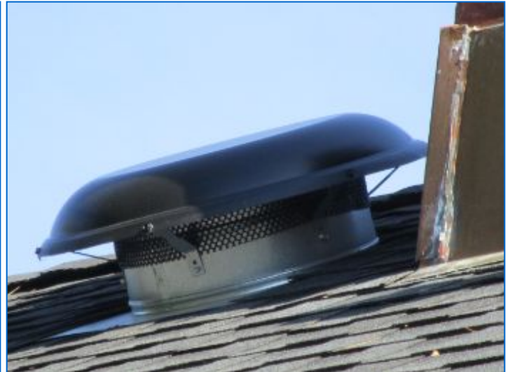
Power Ventilator noted for attic ventilation.
