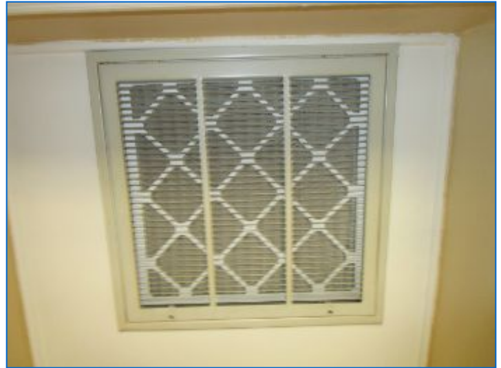
AC#2: Disposale filter located in filter-grille at Hallway (2nd floor) ceiling.
