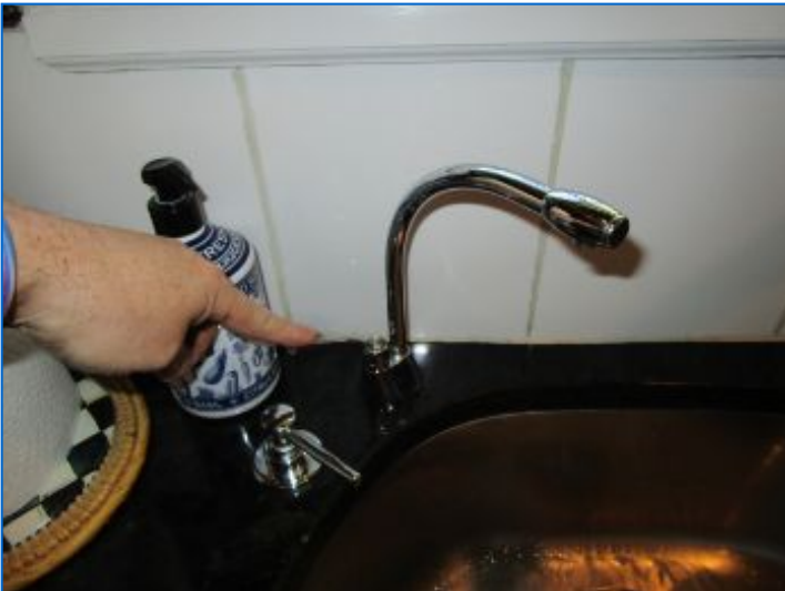
Hot water dispenser was inoperable at time of inspection.
