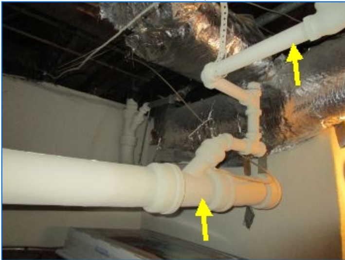
Some DWV pipes were recently painted.
