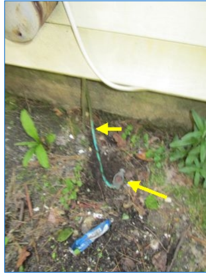
Grounding Rod and cable connection noted at service entrance.
