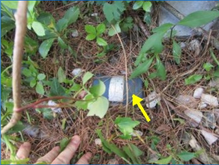
AC#1 refrigerant piping and filter/drier was buried by pine needles/soil. Recommend replacing and raising refrigerant pipe above ground to prevent corrosion that can lead to refrigerant leakage.
