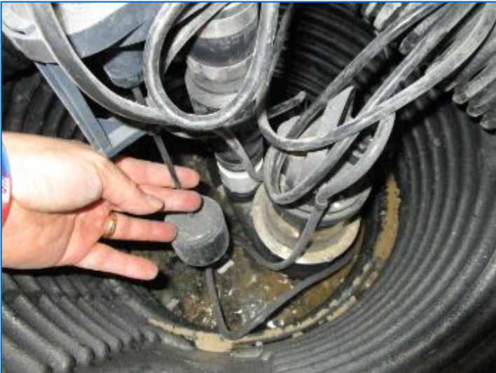
The sump pump responded to the controls at the time of the inspection.
