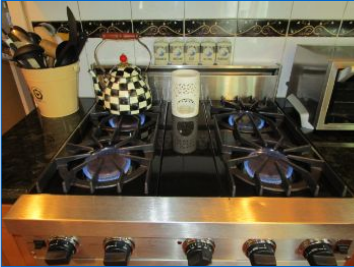
Gas-fired range; operable.
