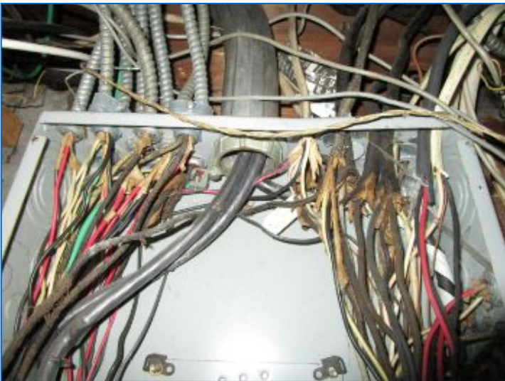
Distribution wiring observed consisted of copper and some aluminum, non-metallic and metallic armored cable.
