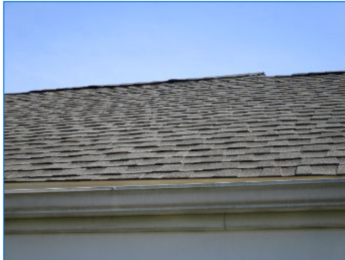
Top asphalt architectural shingle roof covering showed conditions consistent with < 1 yr old shingles. Confer with seller about transferring the installer and manufacturer warranties.
