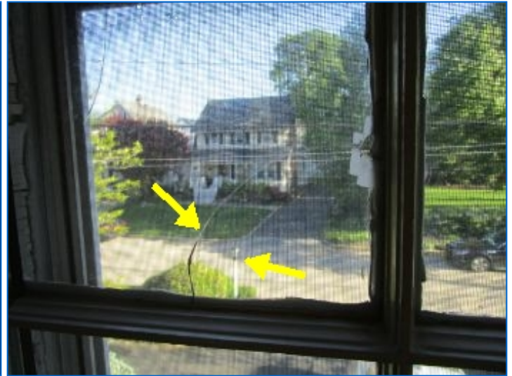
A window in the Office had cracked panes. Repair to prevent injury.
