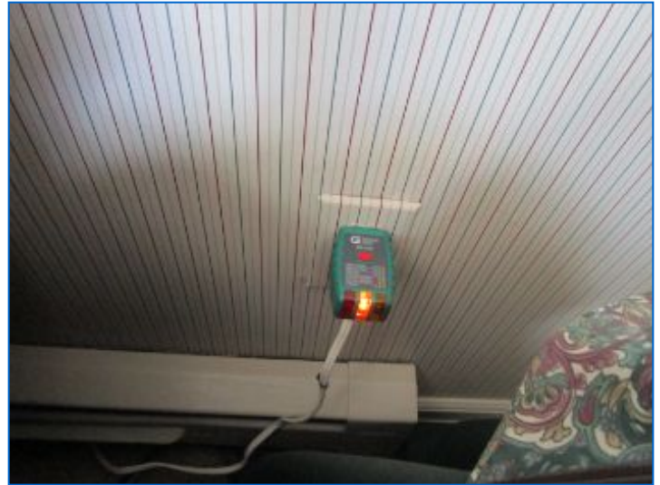
Open ground receptacle noted.
