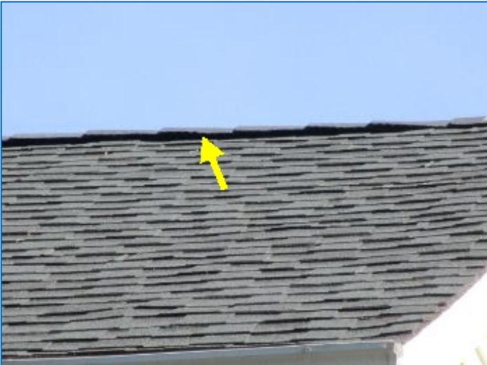
Lower roof ridge exhaust venting noted for attic ventilation.
