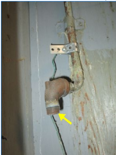
Uncapped supply line noted in basement. All water pipes not supplying a fixture must be properly terminated/capped to prevent possible water damage and or personal injury from scald burns if valve is accidentally operated.
