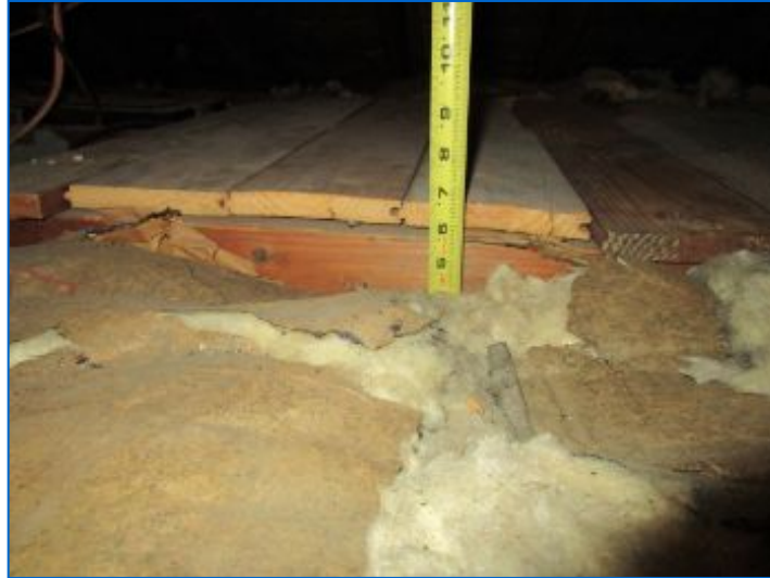
Insulation depth varied 4 - 5 inches (R-15.5 overall). Latest energy conservation standards call for 9-10 inches (R-30). Additional insulation should be installed where possible for enhanced energy efficiency of the home.
