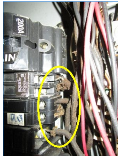
Some older cloth covered power cables are present in the home. Avoid damage to older cloth covered wiring; update when practicable. Suggest having a qualified electrician evaluate and apply corrective measures to avert hazard.
