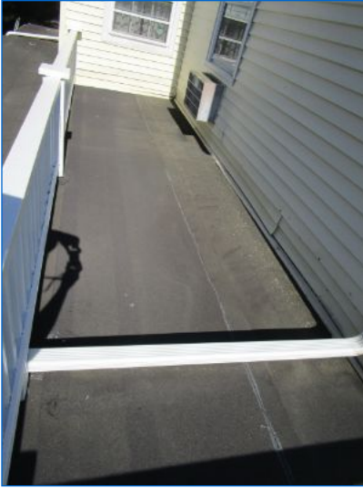
Flat asphalt roof covering showed conditions consistent with 10+ yr old roll roofing.
