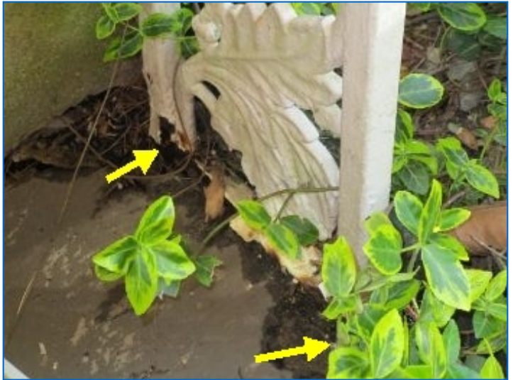
Wrought iron decorative type roof supports showed signs of corrosion where in contact with soil; Recommend removing soil from these areas around supports; repair where necessary; strip and apply a rust inhibitor type coating and repaint.
