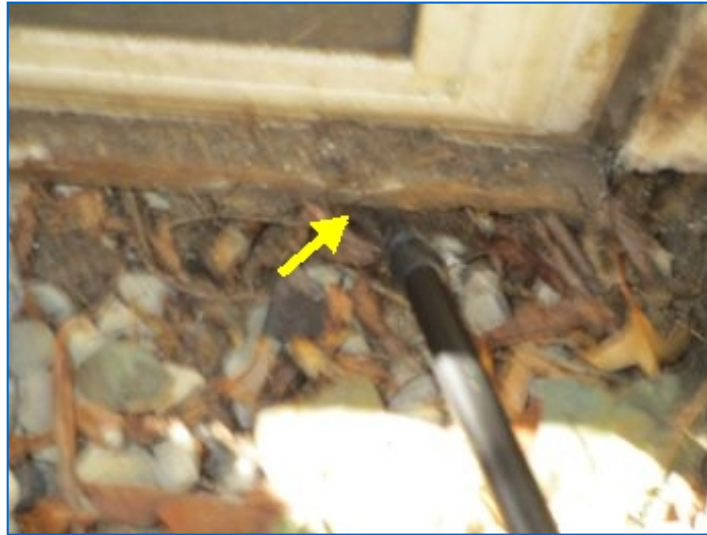
Basement window wood frames in contact with soil showed signs of moisture damage at Front exposure. Recommend regrading soil level to 6 inches below frame; repair and protect wood from further moisture damage.
