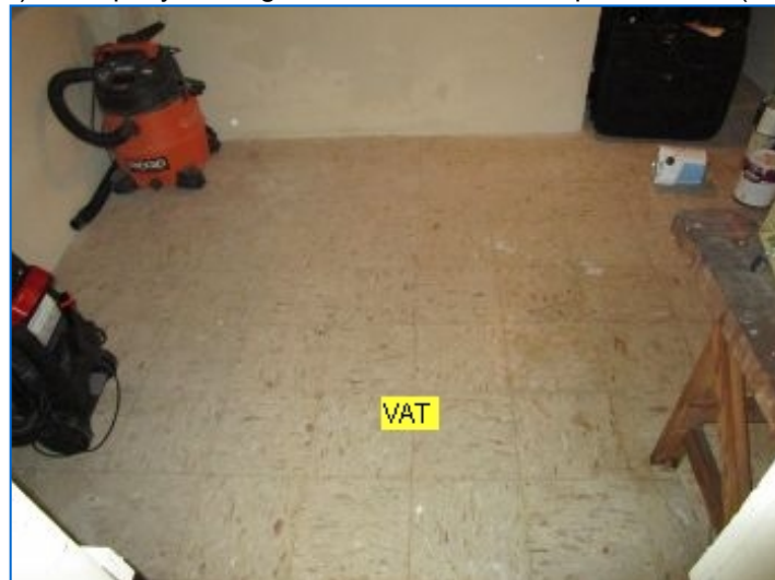
Floor covering consisted of a combination of Laminate, Vinyl Composition Tile (VCT) and Epoxy coating.
