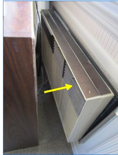
Older through-wall A/C unit (supplemental) in 2nd floor office was inoperable at time of inspection.
