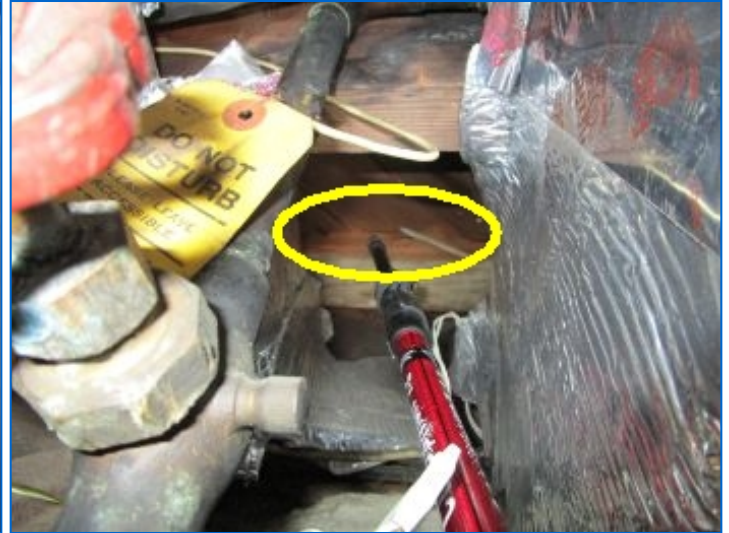
Damage noted from past termite activity at south sill plate in water meter closet. Refer to NPMA-33 Report.
