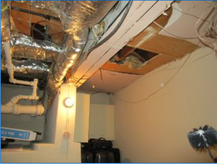
Ceiling conditions in southwest room in basement.
