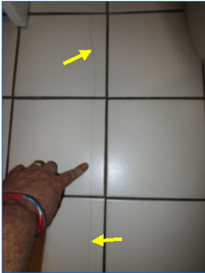
Floor tiles cracked from common structural settlement; suggest tile repair/s.
