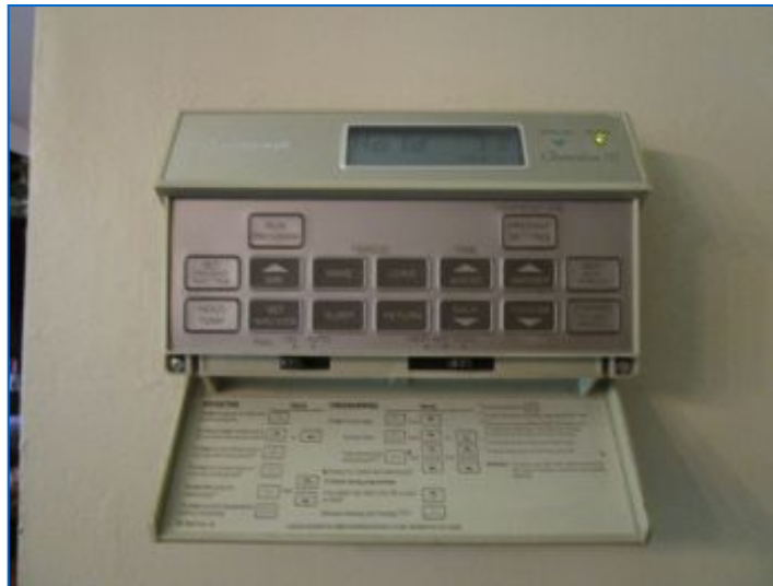
Digital Programmable type thermostat noted in Dining room for AC#1.
