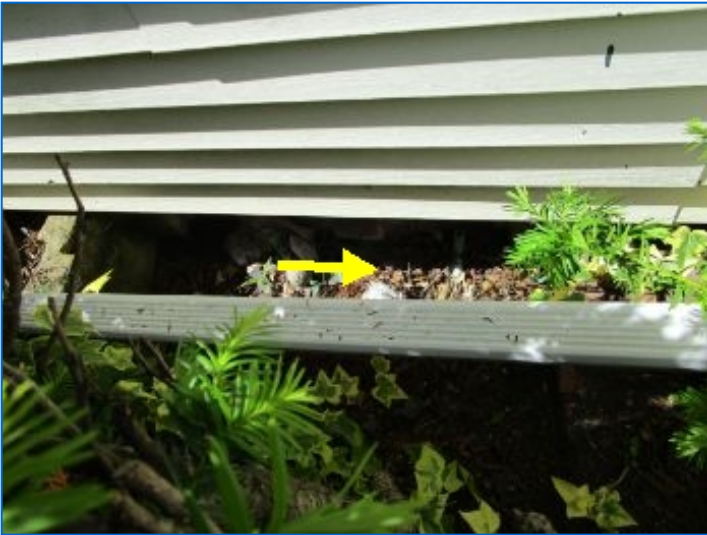
Basement window frames in contact with soil at Front exposure. Recommend regrading soil level to 6 inches below frame; repair and protect wood from further moisture damage.
