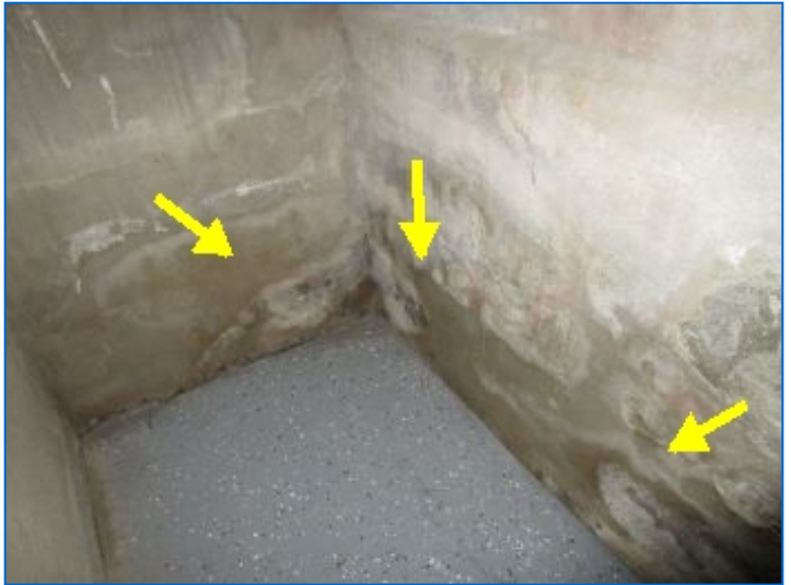
Area where moisture level tested high at lower part of foundation wall in basement extension under garage.
