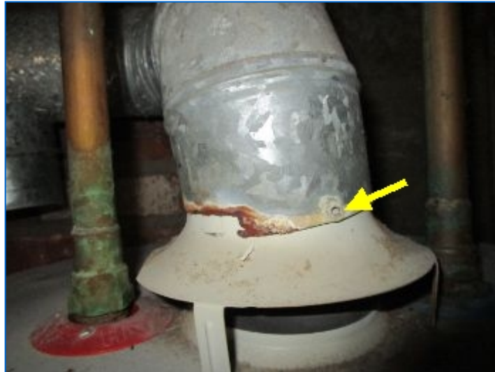
Vent pipe was not properly fastened to water heater vent hood; Recommend repair.
