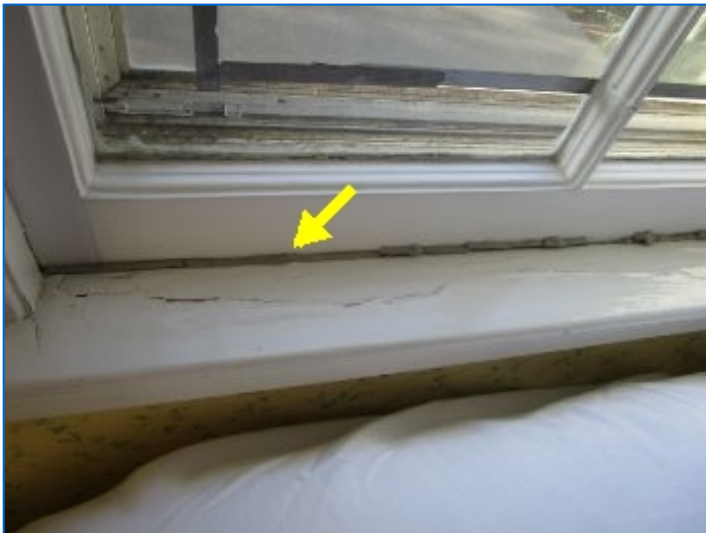
One window was caulked shut; inoperable; recommend bedroom window repair or replacement by a qualified contractor.
