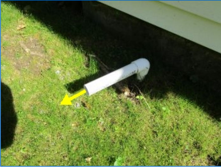
Basement sump pump discharge pipe noted at back yard.
