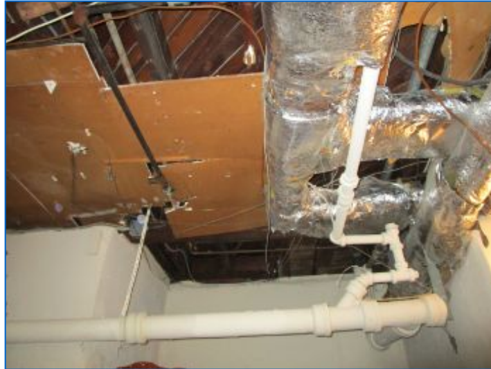
Ceiling conditions in southwest room in basement.
