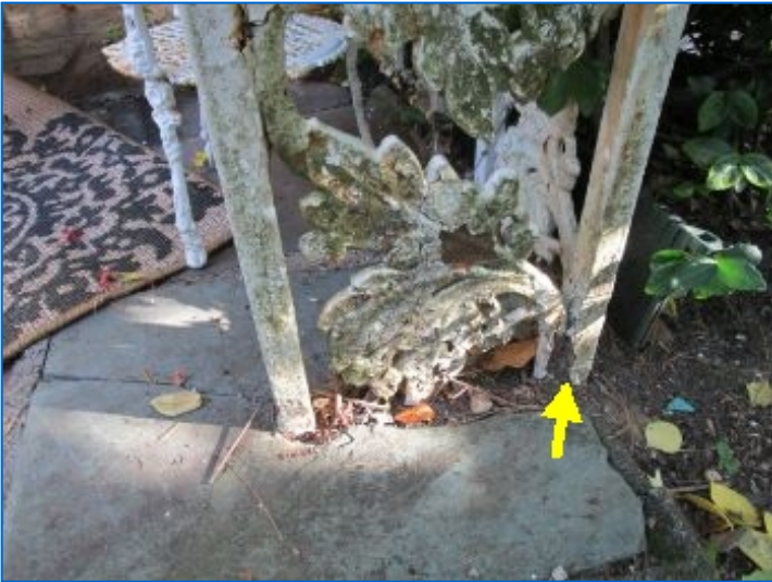
Wrought iron decorative type roof supports showed signs of corrosion where in contact with soil; Recommend removing soil from these areas around supports; repair where necessary; apply a rust inhibitor type coating and repaint.
