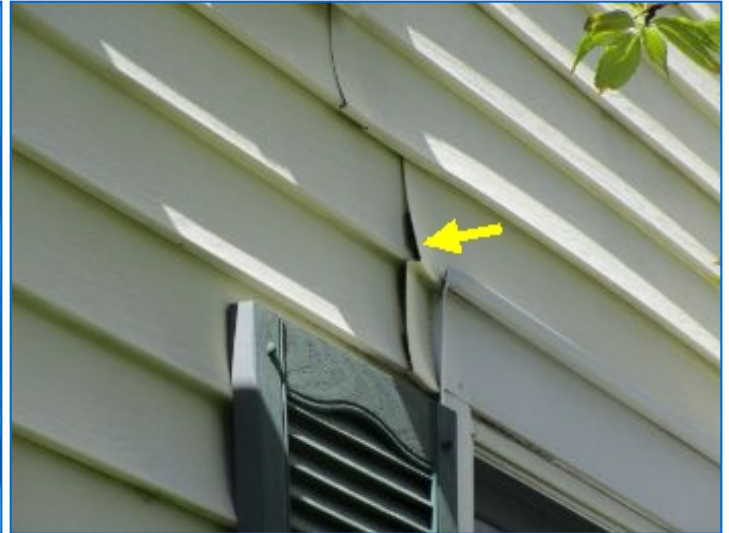
Irregular seam noted at front siding. Repair siding seam to prevent water intrusion into the structure.
