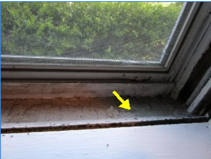
Window sills at original wood frame windows had peeling paint and are in need of maintenance. The Inspector recommends service by a qualified painting contractor.
