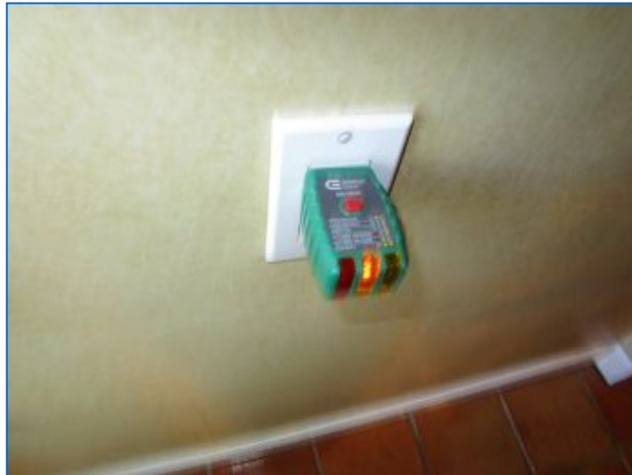
Random Outlet Test: Ungrounded receptacle noted.
