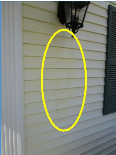
Cosmetic damage/discoloration noted at Front, perhaps caused by cleaning chemical.
