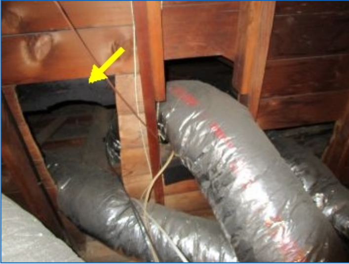
Not all areas of the attic were physically accessible at time of inspection.
