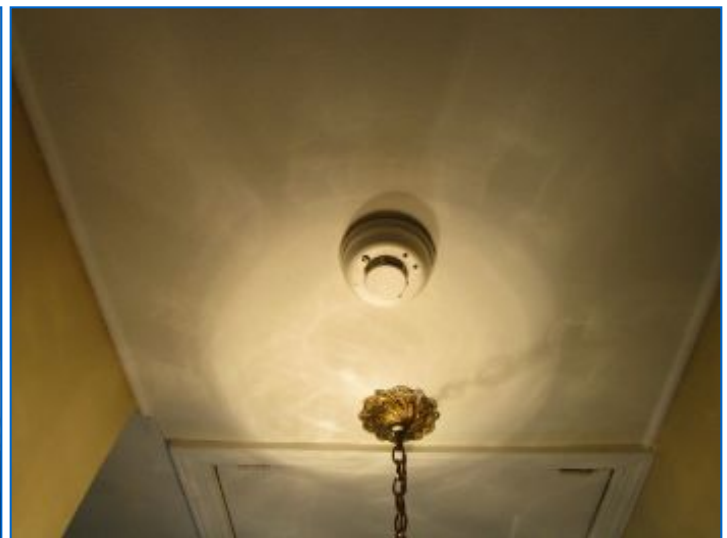
Smoke/Carbon Monoxide Detector noted in Hallway (2nd floor). Maintain functioning Smoke/Carbon Monoxide detectors as prescribed. Detectors are generally reliable for up to 5 yrs.
