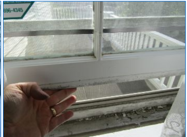
The lower sash of a double-hung window would not stay up when lifted and released; recommend bedroom window repair or replacement by a qualified contractor.
