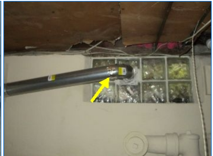
Dryer vented to exterior.
