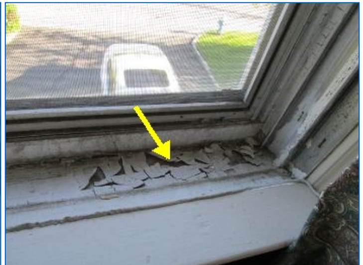
A window jamb in the Office had peeling paint and needed maintenance. The Inspector recommends service by a qualified painting contractor.
