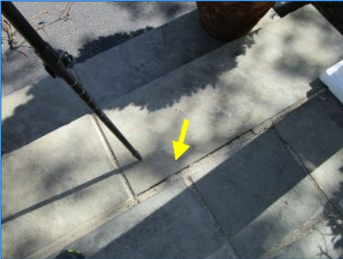
Deteriorated/cracked mortar at two Bluestone tiles at front steps; loosening tiles noted. Recommend repairs to eliminate potential trip/fall hazard.
