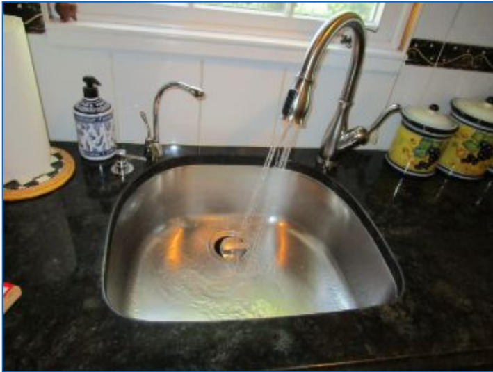
Main faucet operated normally at time of inspection.
