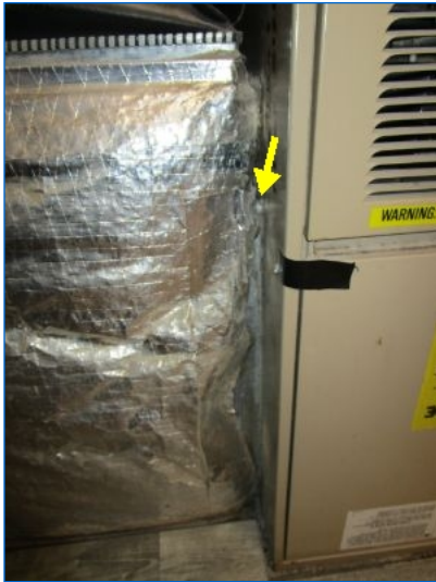
No filter located at HVAC#1 cabinet intake.
