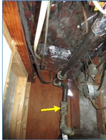
Whole house gas supply shutoff valve at gas meter location.
