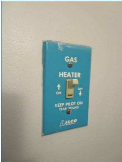
Remote Emergency Shut-off switch noted at basement stairs.
