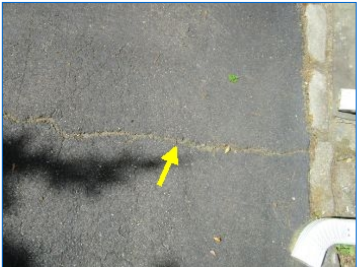
Normal cracks in asphalt driveway. Seal and/or repair cracks to prevent water entry leading to freeze-thaw damage. Monitor existing cracks for expansion.
