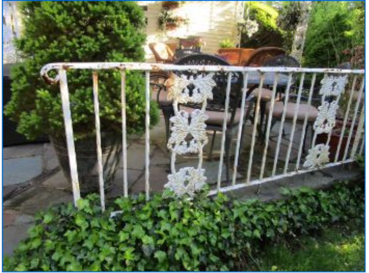
Wrought iron handrail was supportive, however showed signs of corrosion; Recommend stripping; apply a rust inhibitor type coating and repaint.
