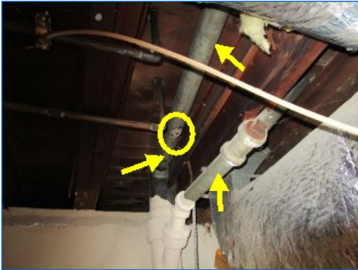
Galvanized DWV pipe noted.
