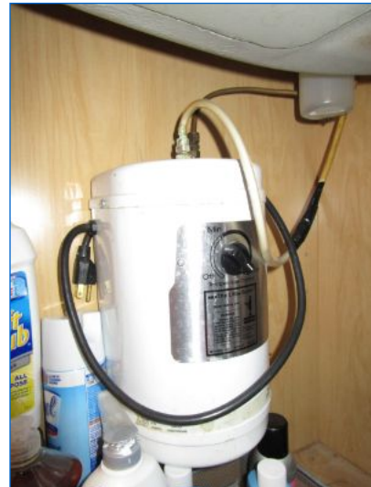
Hot water dispenser was inoperable (unplugged) at time of inspection. Confer with seller.
