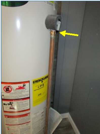
Temperature Pressure Relief (TPR) valve and discharge pipe showed no deficiencies.
