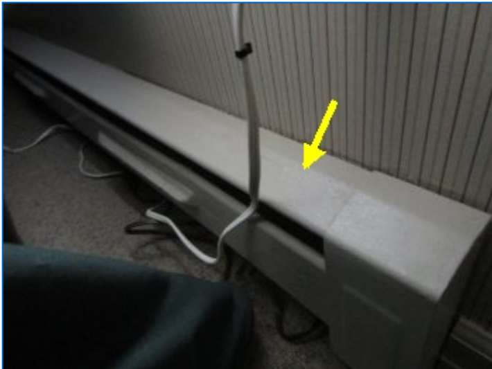
Defunct length of baseboard heating noted in office. Office heating is via ducted HVAC#2 system
