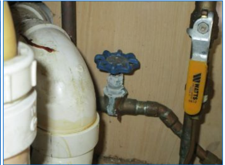
Deposits observed at water valve under sink is a sign of valve body corrosion and past leakage; recommend repair or replacement by a qualified plumber.
