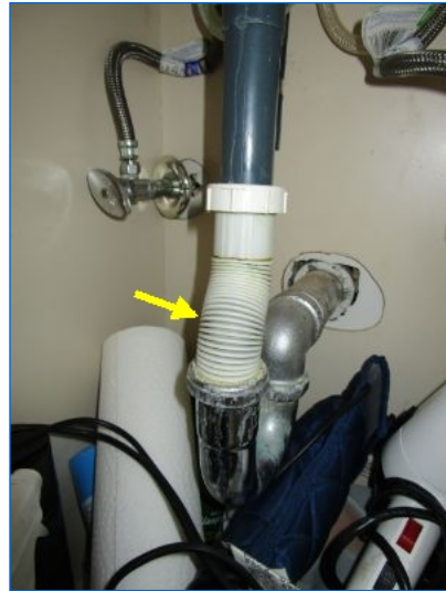
Flex drain connections are not compliant and are subject to frequent clogging. Recommend replacement with proper drain piping by a licensed plumber.
