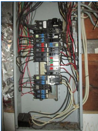
Main panel interior checked.
