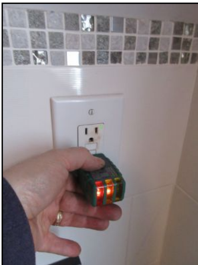
GFCI type receptacle did not trip when tested. Recommend replacing GFCI receptacle.
