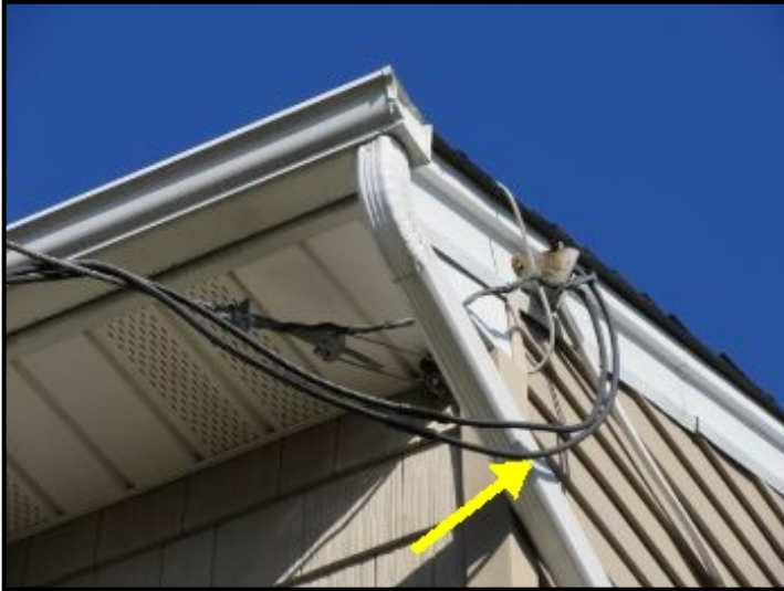
Overhead service drip loop should not be in contact with aluminum downspout. Recommend review by a licensed electrician for corrective repair.
