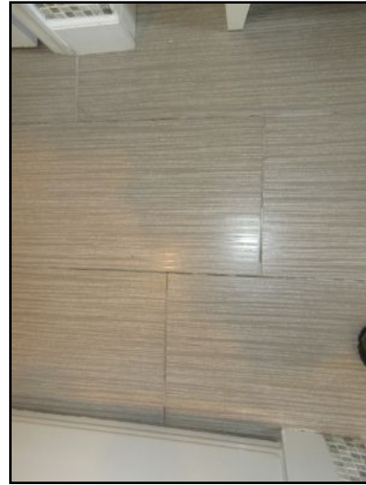
Floor tile grout cracked/missing; suggest grout repair(s).
