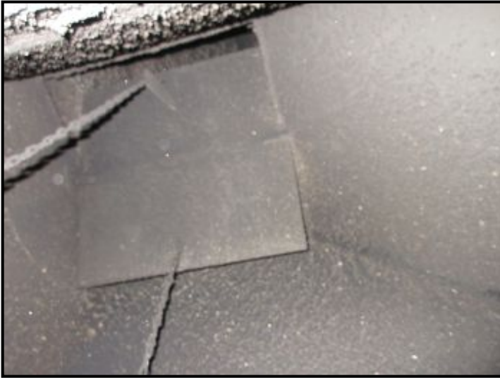
Damper was opened and closed several times.
