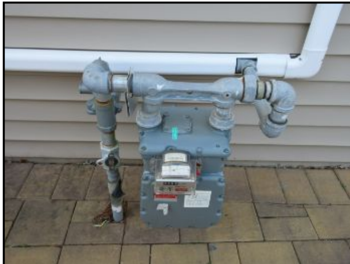
Public Gas Service: Meter, shutoff valve and vented regulator noted outside.
