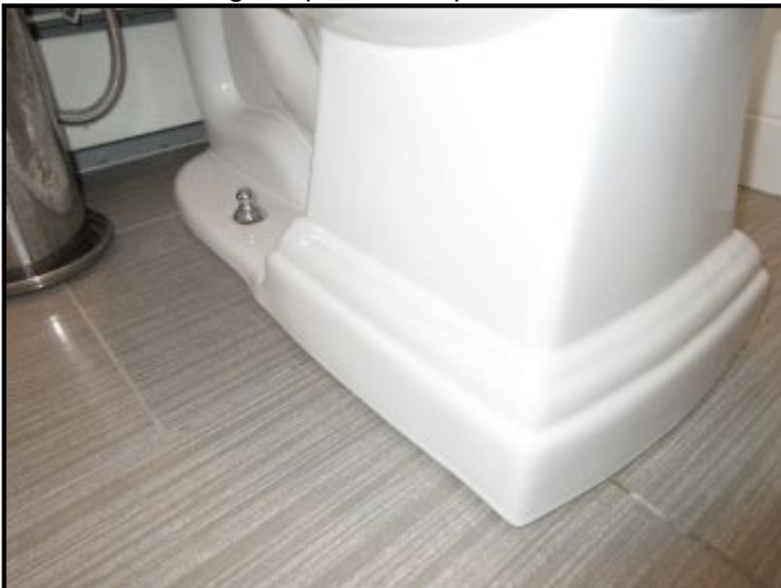
Toilet bowl is loose at floor anchor bolts. The wax ring inside the unit must have a snug, secure fit in order to keep from leaking. Properly resealing and re-securing this unit is suggested to prevent water leakage and damage to the sub-floor area. This type of damage is not always visible or accessible to the inspector at time of inspection.
