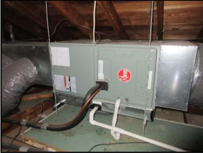
One of two Rheem central air handlers located in the attic. Only the units' fans were tested and found operable. See related A/C test limitation.
