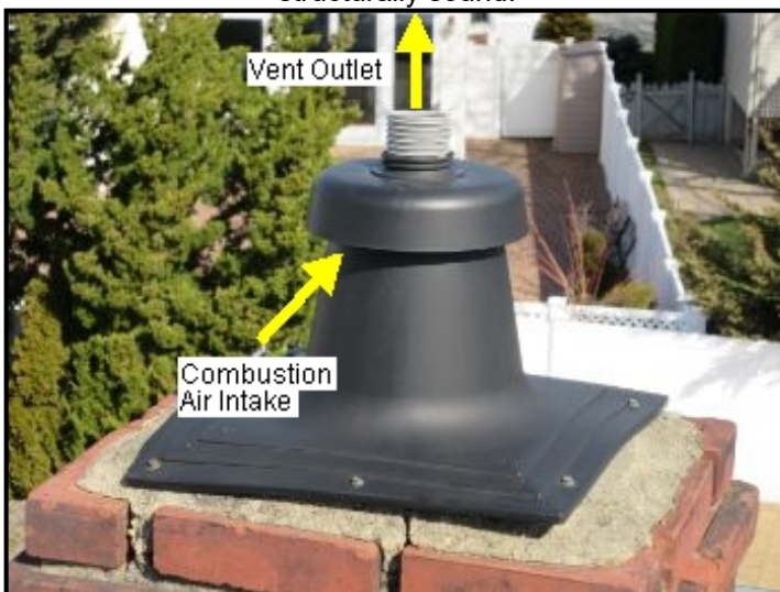
Combustion air intake/outlet (concentric vent termination) for tankless water heater located in basement.
