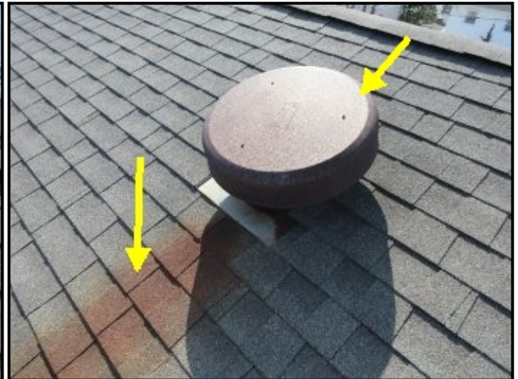
Power roof vent noted for attic ventilation. Rusty vent cover staining roof shingles.
