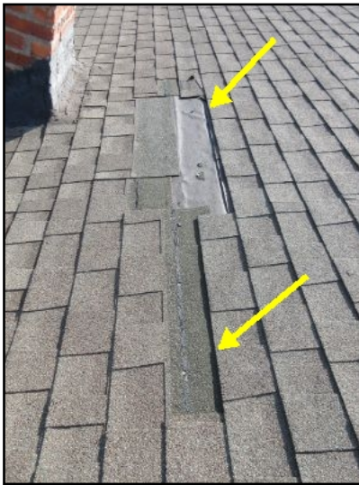
Section of shingles were apparently blow loose and are missing. Suggest priority repair.
