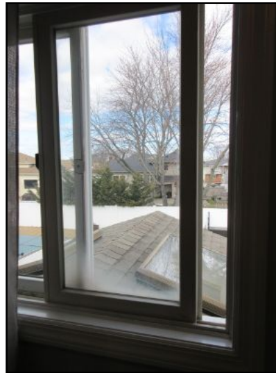
Rear bedroom: Cloudiness/condensation observed in a couple of thermopane double glazed windows in bedrooms. This is an indication of a failed seal. A qualified contractor should review for replacement as needed.
