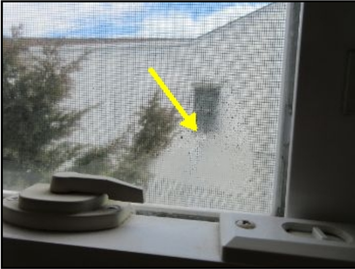
Insulated glass window gas seal may have broken; Repair insulated glass panel, or replace whole sash.
