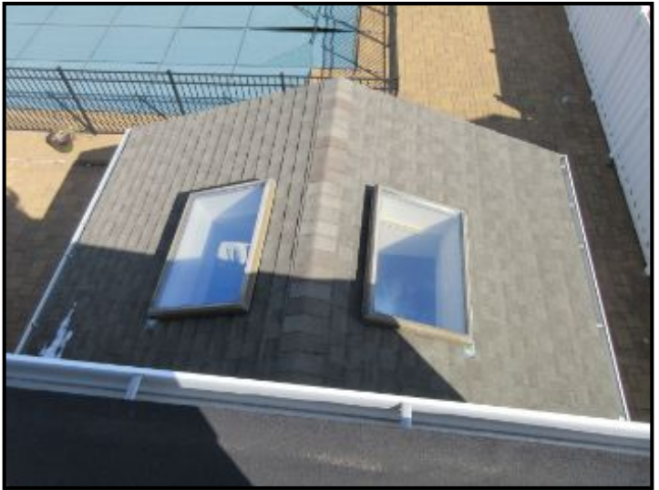
Roof over kitchen addition. Skylights did not display any outward signs of active or past leaks at time of inspection.
