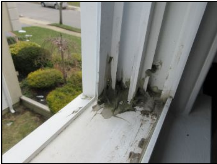
Sloppy caulking repair noted at front corner bedroom.
