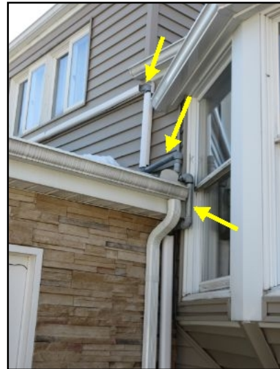
Cosmetic finishes (gas pipe covering) with sections missing.
