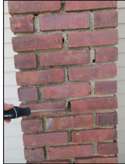
West chimney mortar shows sign of deterioration. Recommend repointing mortar joints where needed to prevent further degradation. The chimney is otherwise structurally sound.
