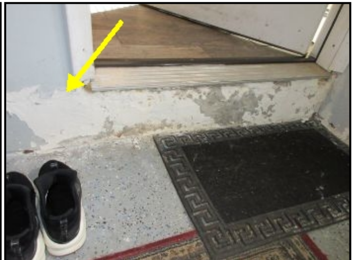
Drywall cover damaged at step riser.
