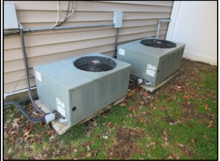
Two Central A/C split-systems, each with outdoor condenser and Ducted indoor air handler.
