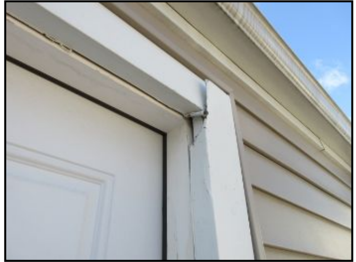
Cosmetic damage noted at garage service door frame trim.
