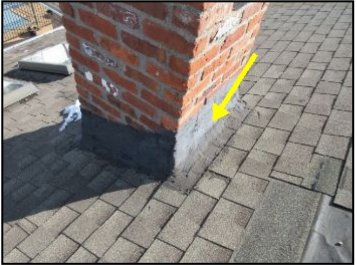
Flashings are mastic covered, recommend periodic re-sealing all through the roof vents and projections as a part of routine maintenance.
