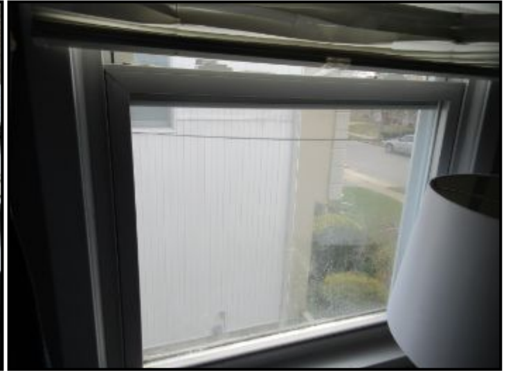
Cloudiness/condensation observed in a couple of thermopane double glazed windows in bedrooms. This is an indication of a failed seal. A qualified contractor should review for replacement as needed.
