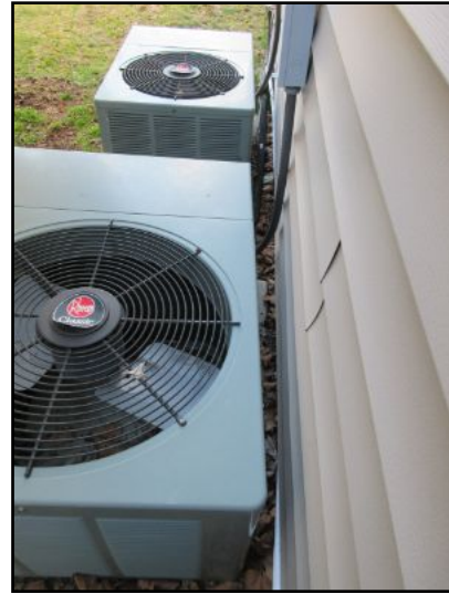
Outdoor condenser air flow appears restrictive based on its distance from the house. This can negatively affect system performance. Suggest checking manufacturer's clearance requirements.
