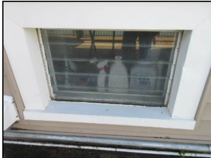
Aluminum framed Louvered windows noted. Recommend updating basement windows to insulated glass vinyl type windows for energy efficiency, maintenance and aesthetic reasons.
