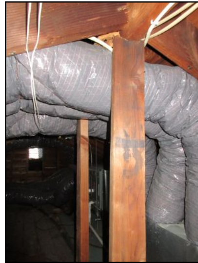
Vertical support of roof ridge beam noted.
