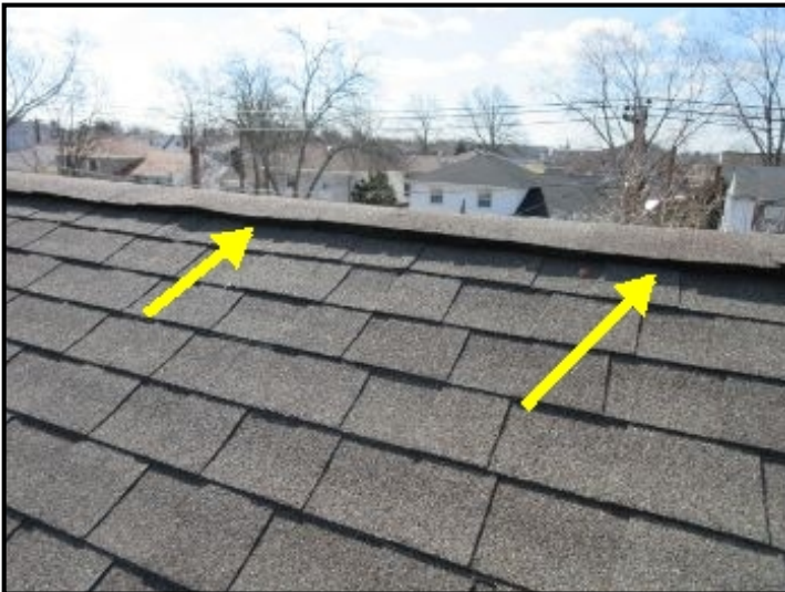
Ridge vent noted for attic ventilation.
