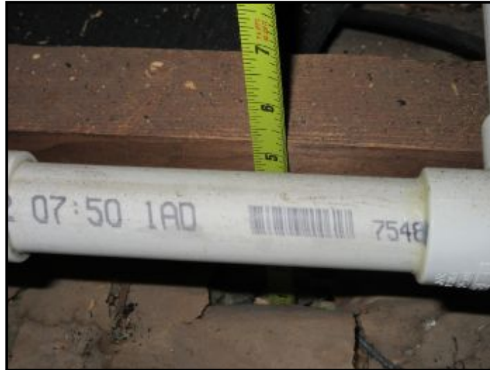
Insulation depth varies 1 - 2 inches (R-5); Poorly insulated; Recommend improvement.
