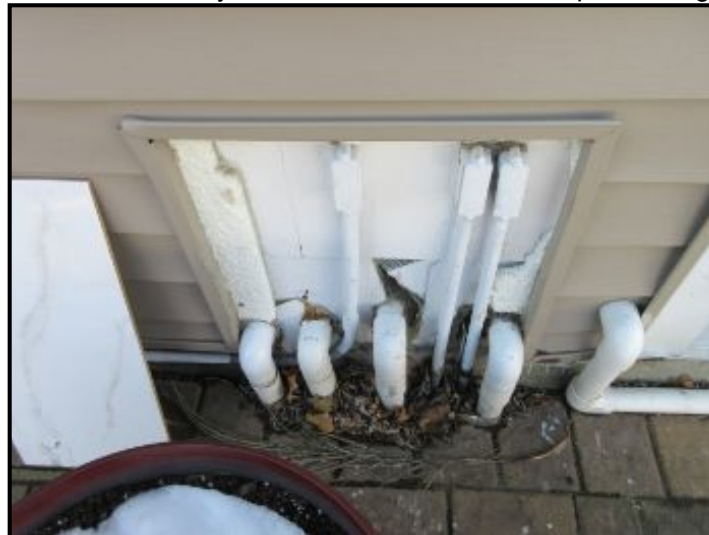
Pool filter pipe cover missing at garage rear exterior wall. Suggest fabricating a water resistance cover for cosmetic purposes.
