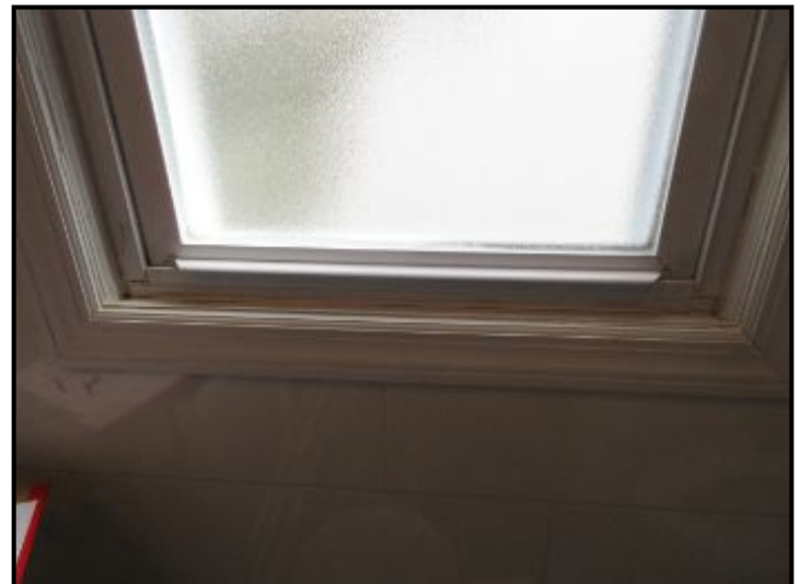
Window sill shows signs of moisture damage. Suggest repairing and refinishing affected wood.
