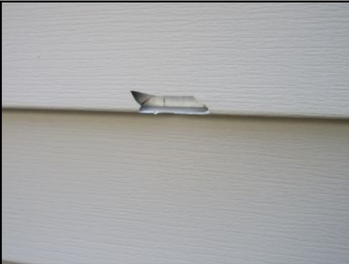
Vinyl siding damage noted at west exposure. Recommend repair or replacement of damaged section to prevent moisture intrusion of the wall assembly.
