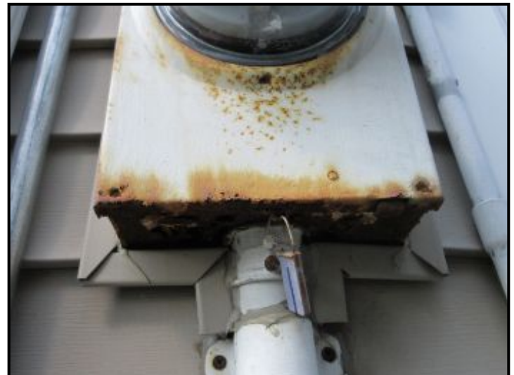
Older meter box badly rusted , caused by water entry. Recommend electrician to update.
