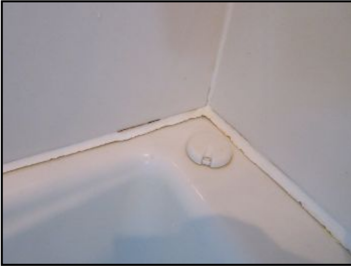
Suggest updating caulk at tub perimeter.
