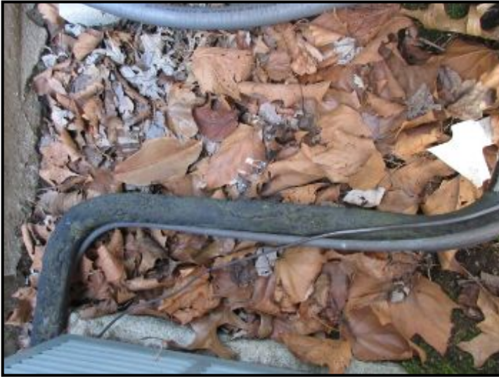
Outdoor refrigerant piping insulation is deteriorated. Recommend replacing outdoor deteriorated insulation.
