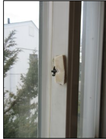
Damaged/missing hardware at Rear bedroom. Repair as needed.
