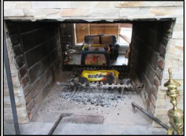
Fireplace ash dump door was operable. Have chimney swept by professional.
