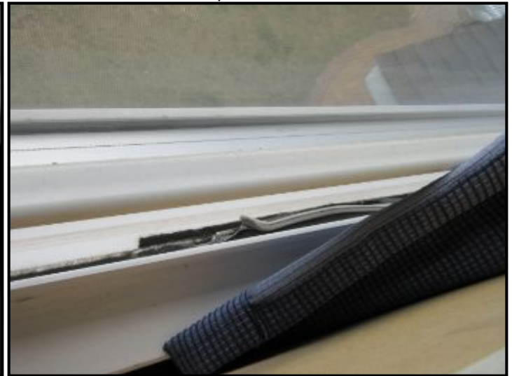
Older (1991 manufactured) thermal windows - weatherstripping deteriorated.
