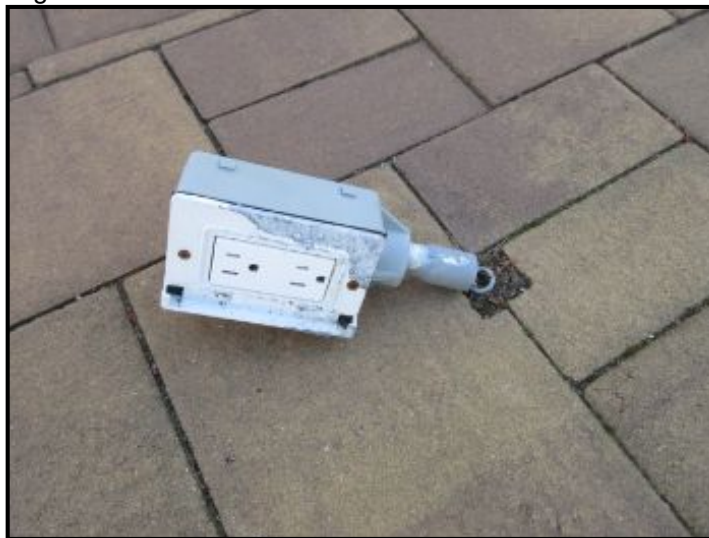
Floor mounted receptacle conduit broken; potential for water entry into conduit. Recommend priority repair.
