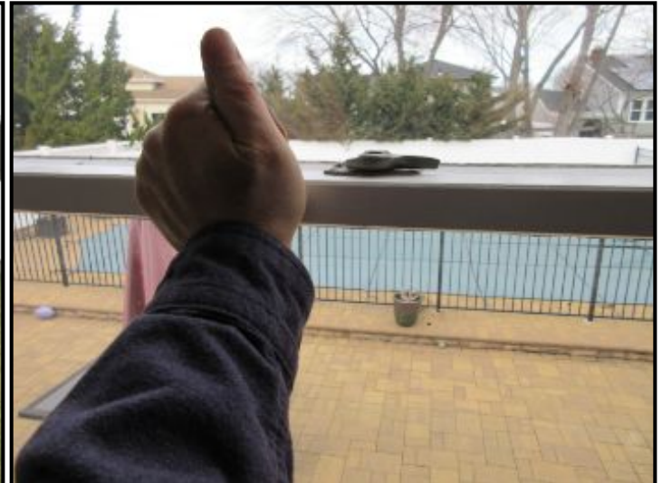
Some living room windows were stuck closed.
