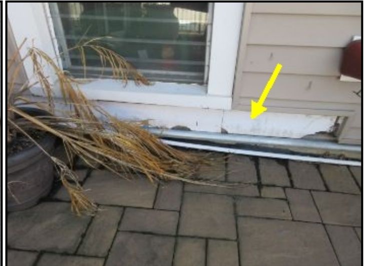
Asbestos cement siding noted beneath vinyl siding. Recommend covering with vinyl siding to prevent water penetrating the structure.
