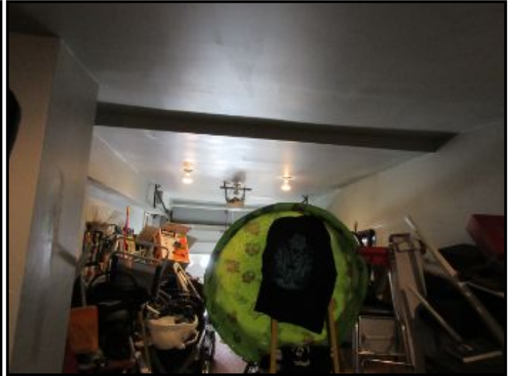
Garage walls and ceiling finished in drywall. Condition was filled with stored items.
