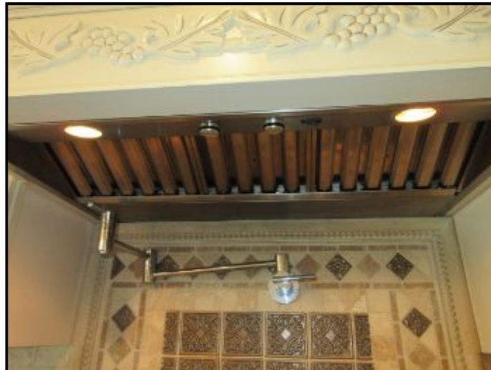
Exterior Vented Fan and light was operable.
