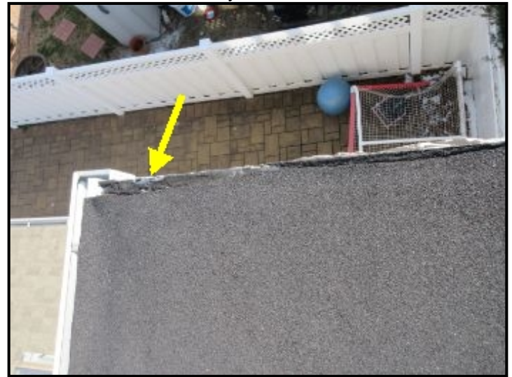
Condition along drip edge at rear bedroom addition roof should be sealed to prevent future water penetration.
