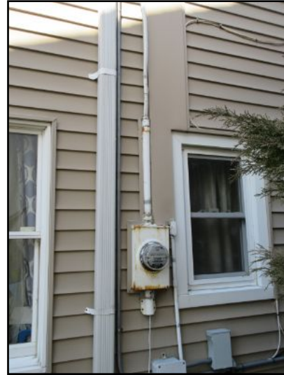
ELECTRICAL Electrical Service Entrance
