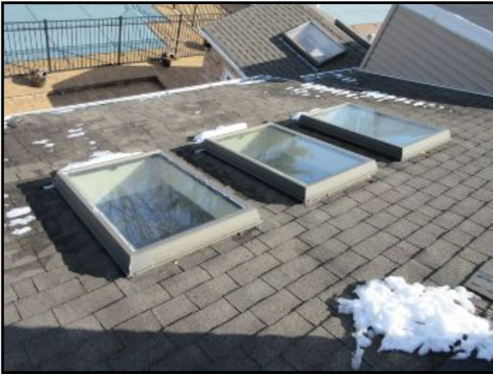
Skylights did not display any outward signs of active or past leaks at time of inspection.
