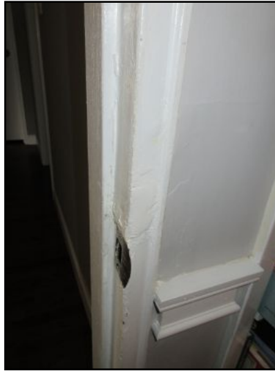
Cosmetic damage noted at front corner bedroom door frame..
