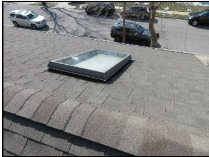
Master bedroom skylights did not display any outward signs of active or past leaks at time of inspection.
