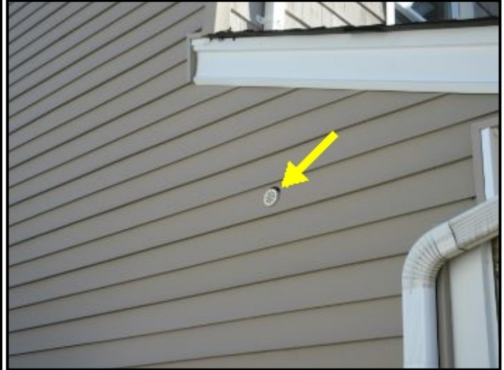
Vent pipe penetration at west exterior. Recommend caulk to seal around penetration to prevent moisture intrusion of the wall assembly.
