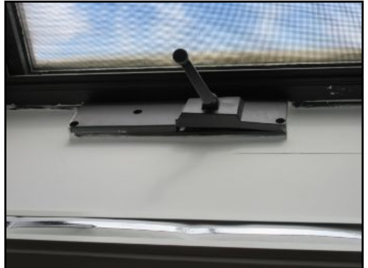
Rear bedroom: Skylight operator was broken and shouldn't be operated. Suggest repairing operator.
