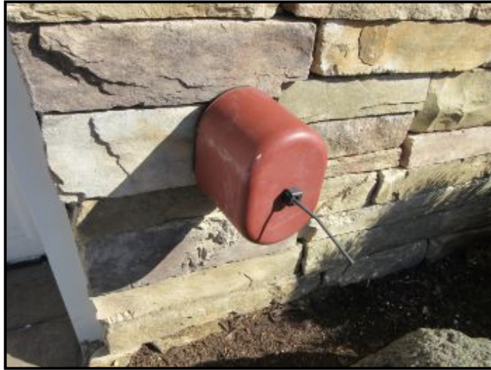
Hose bibbs covered with freeze caps for winterization.
