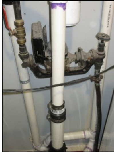
Water Service Entrance: 3/4" Copper, meter, shut-off valves and grounding observed.
