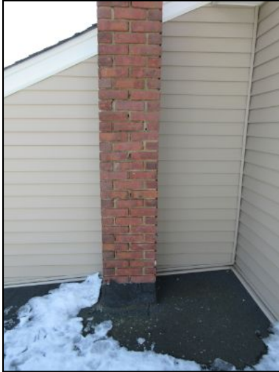
West chimney mortar shows sign of deterioration. Recommend repointing mortar joints where needed to prevent further degradation. The chimney is otherwise structurally sound.
