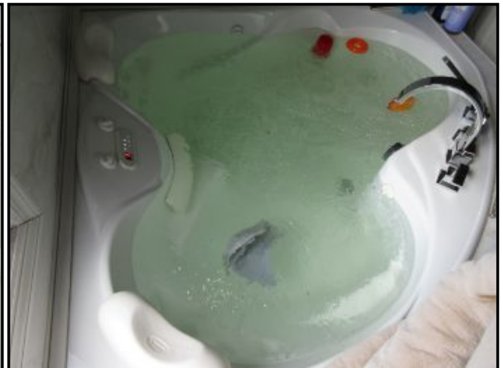
Whirlpool pump was operable.
