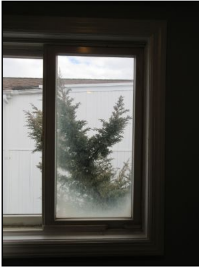
Rear bedroom: Cloudiness/condensation observed in a couple of thermopane double glazed windows in bedrooms. This is an indication of a failed seal. A qualified contractor should review for replacement as needed.
