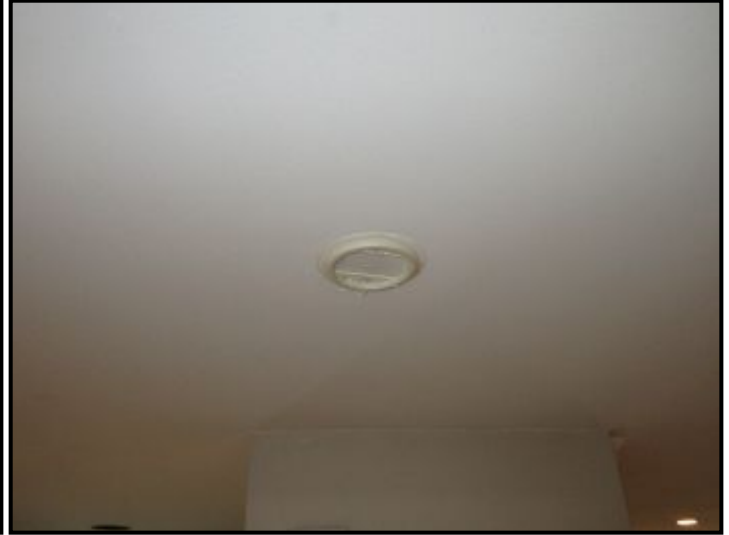
Smoke/Carbon Monoxide detector missing in main hall.
