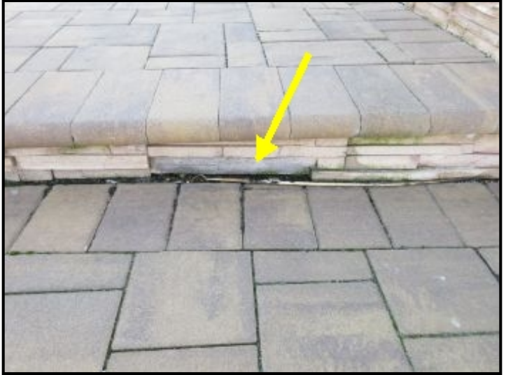
Stone face missing at step riser.
