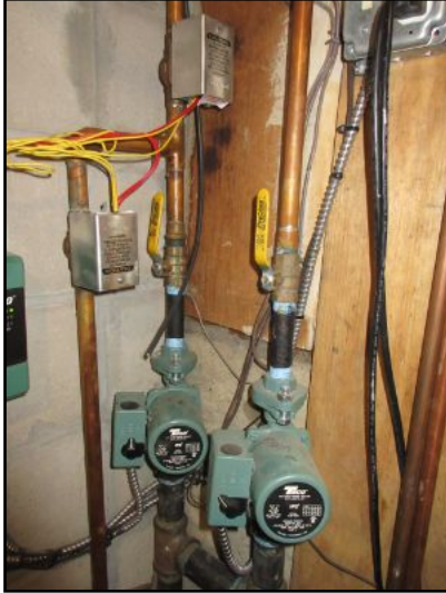
3-zone heating system noted.
