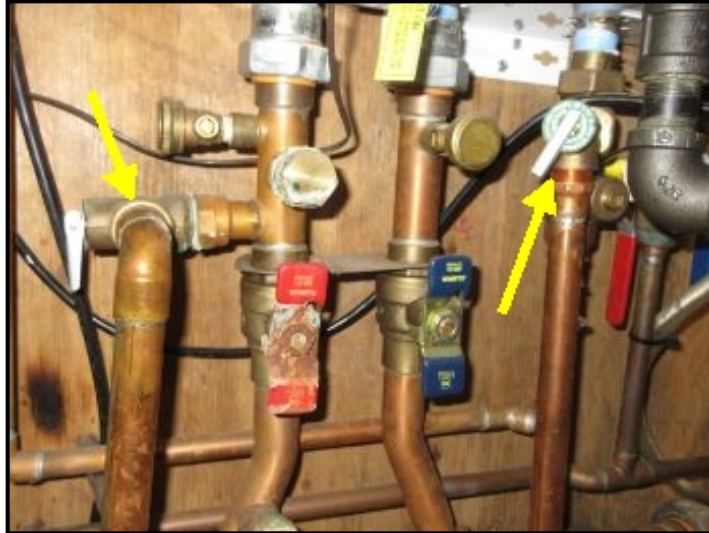
TPR (Temperature Pressure Relief) valves and discharge pipes show no deficiencies.
