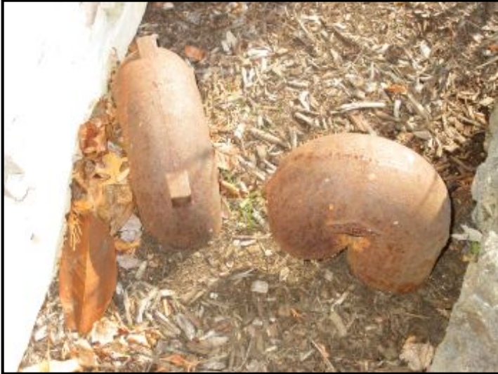
Waste Pipe Exit located at front of house with vent and whole-house trap.
