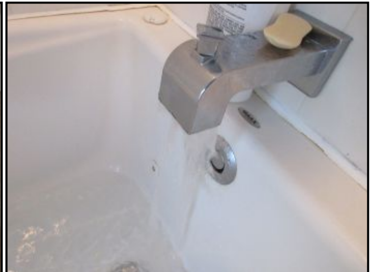
Whirlpool/tub faucet did not supply hot water. Recommend plumber to evaluate. Water pressure/flow is low when running other fixtures in one area.
