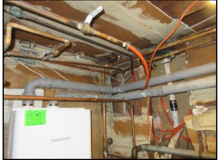
Copper, black iron pipe and PEX-AL-PEX tubing noted.
