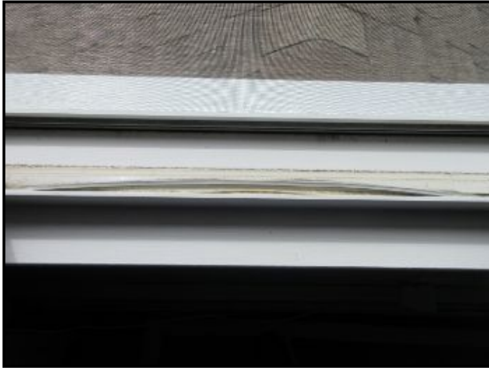
Front bedroom: Older (1991 manufactured) thermal windows - weatherstripping deteriorated.
