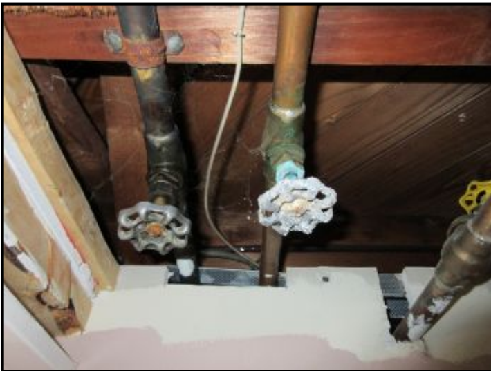
Leaky valve noted in basement. Deposits observed at water valves is a sign of valve body corrosion and past leakage.
