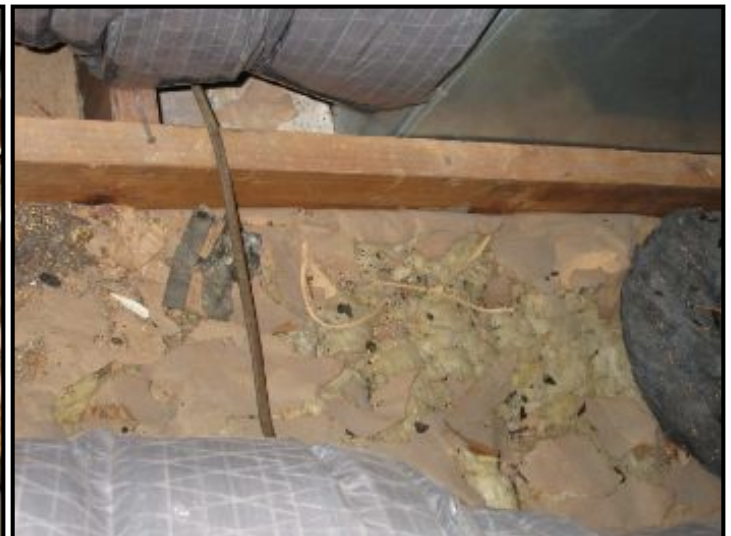
Insulation is missing and damaged in some sections of the attic floor.
