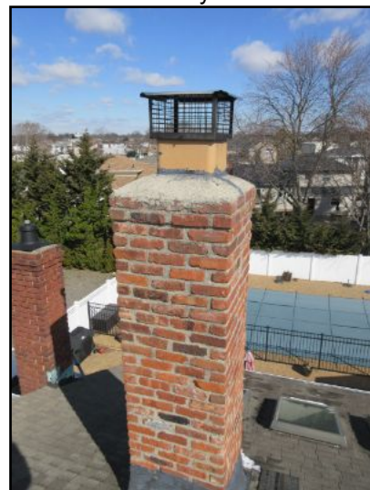
Fireplace chimney showed no major system safety or function concerns noted at time of inspection.
