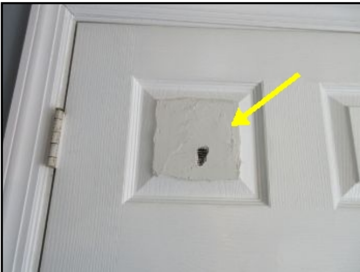
Damage and attempted repair of door.
