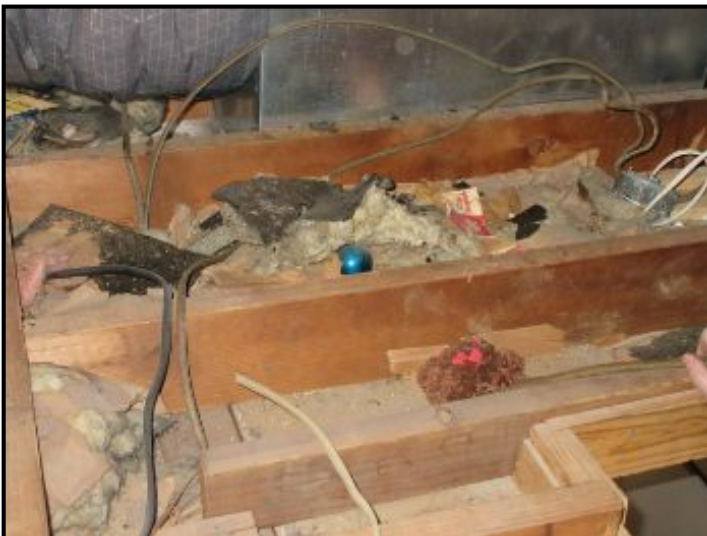
Insulation is missing and damaged in some sections of the attic floor.
