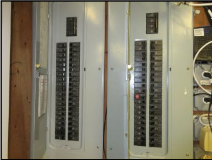
Two 200 amp distribution panels
