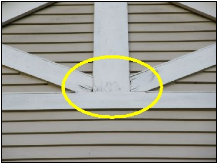
Wooden Gable Pediments show signs of water damage at front of house due to a lack of protection from the elements. Repairs and proper painting is recommended.
