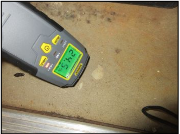
AC-4 Closet floor measured "high" moisture content due to condensate pump suspected to have been overflowing. See related notes. This was the only high moisture level reading taken.
