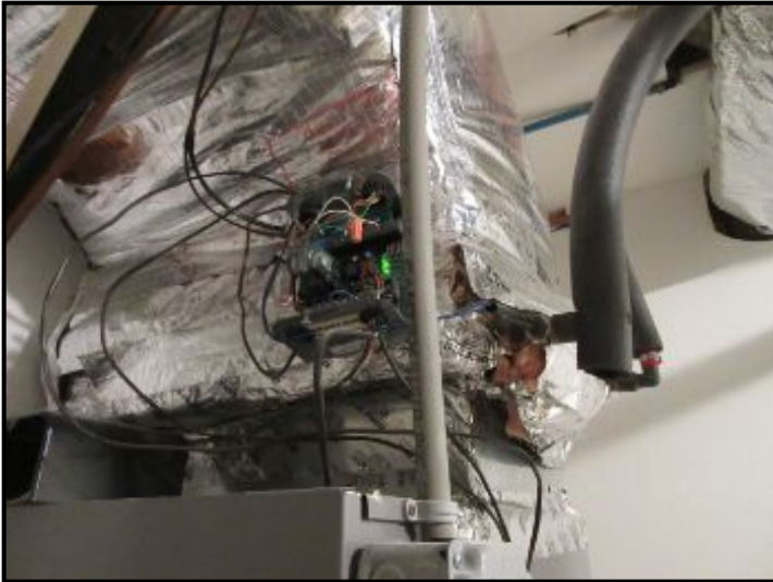
AC-1: Cover removed from HW heating coil controller and left on top of air handler. Suggest having HVAC technician check controller operation, repair as necessary and cover exposed wiring/components.
