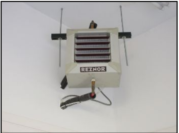
Garage heater on separate zone.
