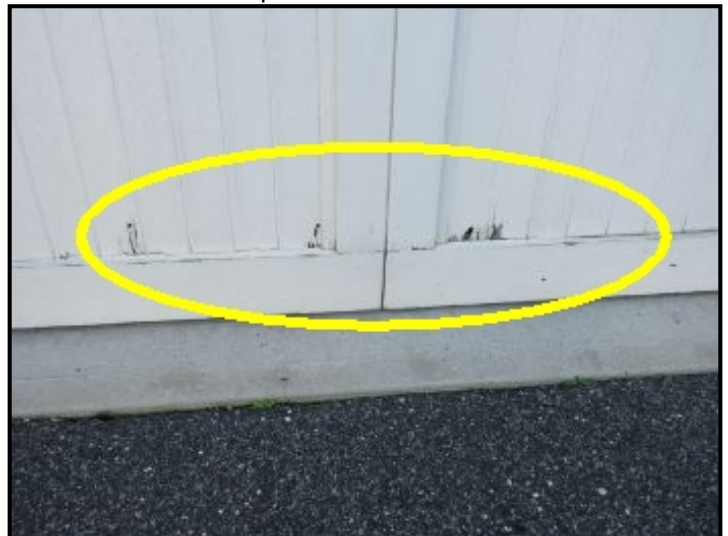
Garage wooden door shows signs of deterioration.
