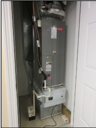
AC-3 air handler located in the basement serves the 1st floor (south-side).
