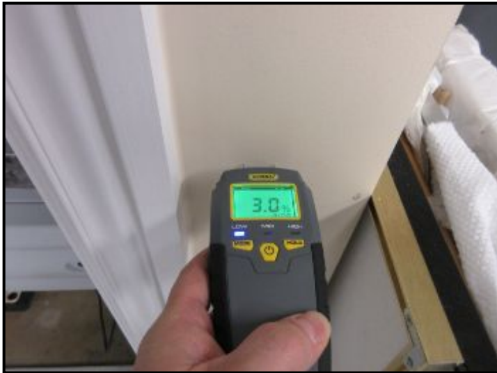
Wall outside AC-4 closet measured "Low" moisture content
