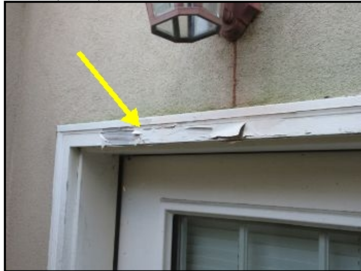
Paint peeling at basement exterior door casing.
