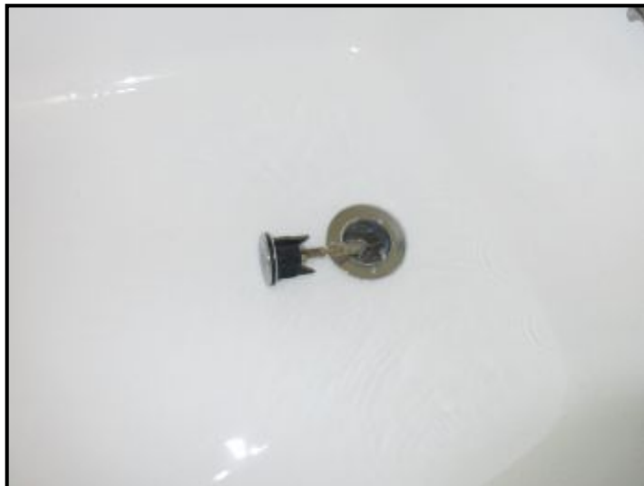
Tub stopper linkage was detached; suggest repair.
