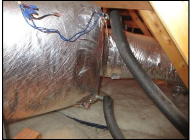
AC-2: HW heating coil.
