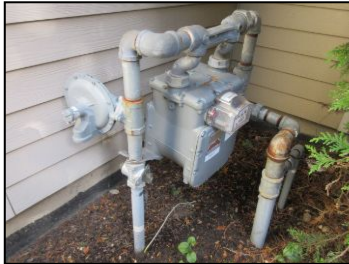
Gas service includes meter, shutoff valve and vented regulator.
