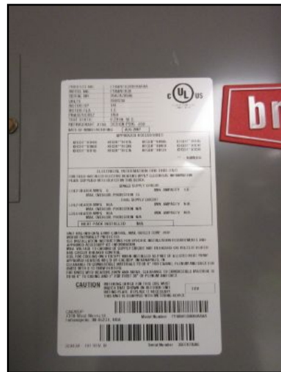
AC-4 split system has a 2.5 ton air handler; matched with AC-4 outdoor condenser.
