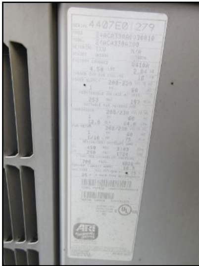
AC-3 split system data plate/serial nos. indicate a cooling capacity of 2.5 tons, and a manufacture date of 11/2007, (10 yrs old).
