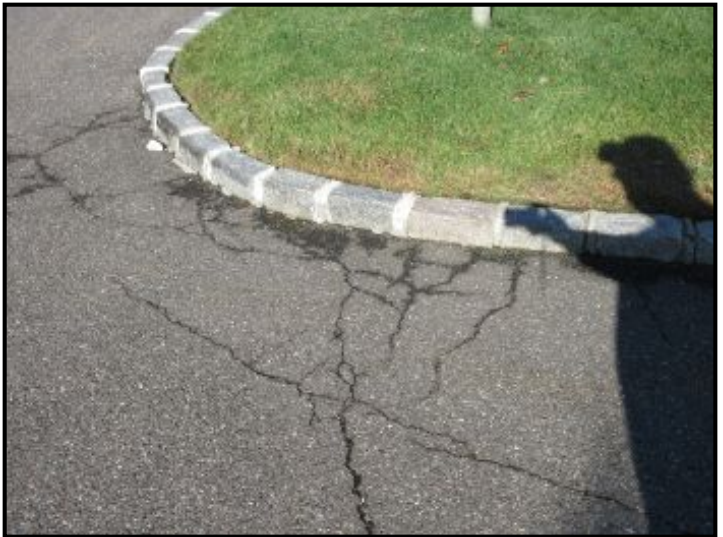
Moderate cracks in asphalt driveway. Suggest maintaining/sealing cracks to prevent wayer entry and freeze/thaw damage.
