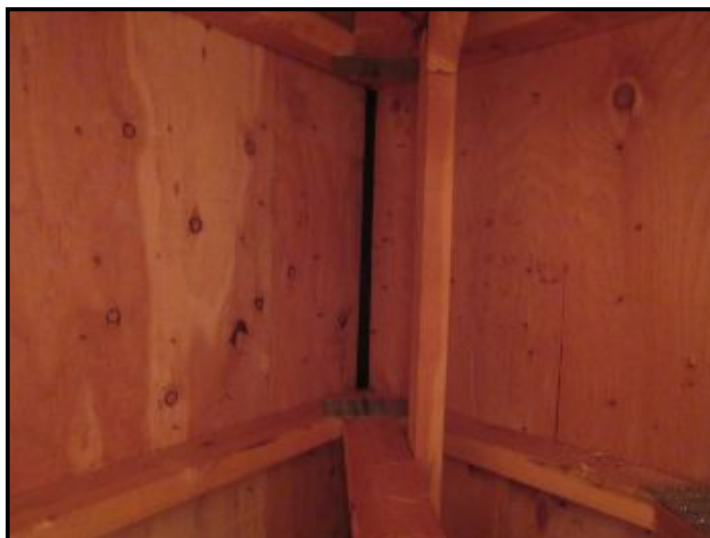
Attic roof ridge outlet vents observed. Under eave soffit inlet vents and fixed roof outlet vents also noted for attic ventilation.
