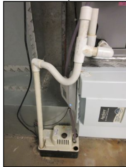
AC-4: condensate pump appeared to have been malfunctioning; pump basin has overflowed, evidenced by floor wetness here. Suggest HVAC technician evaluate and repair/replace the condensate pump.
