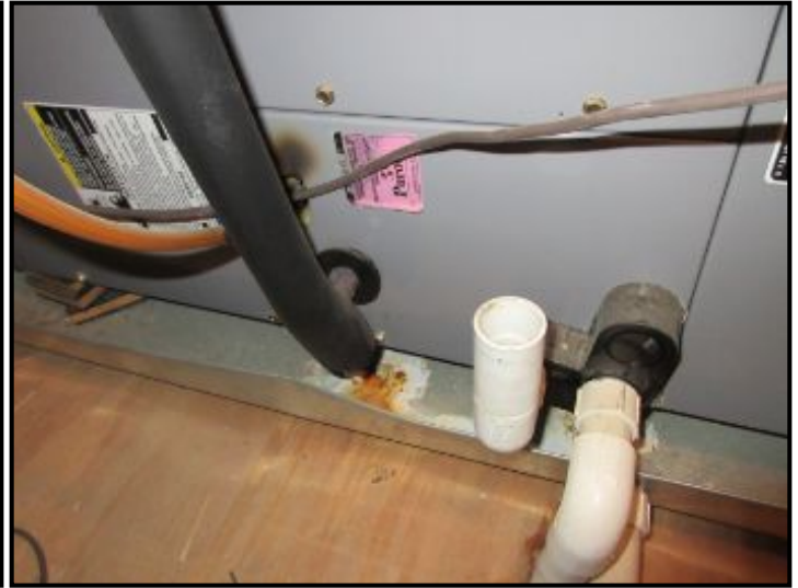
No condensate pumps required for AC-5 and AC-2 attic air handlers (gravity drainage).
