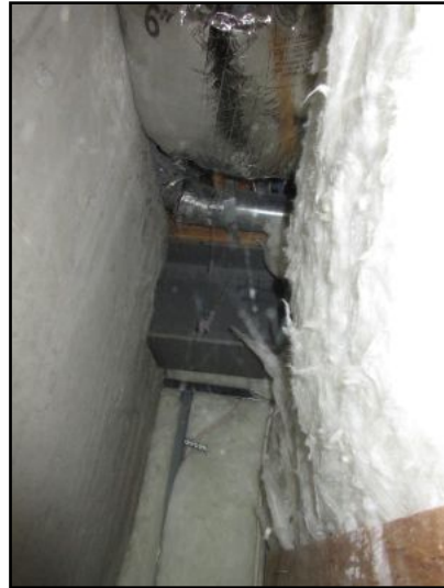
Steel beam noted above at south wall cavity; supports floor joist system.
