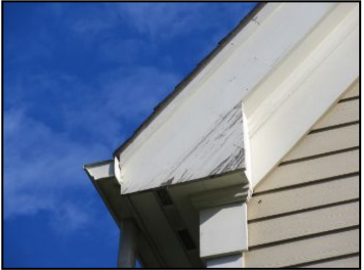
Bargeboards show signs of weathering.
