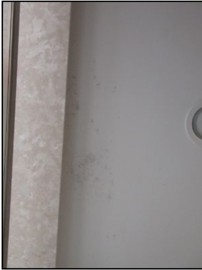
Signs of mildew noted at ceiling above shower.
