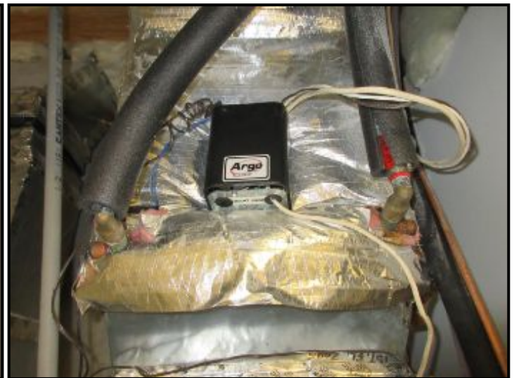
AC-4: HW heating coil and controller.
