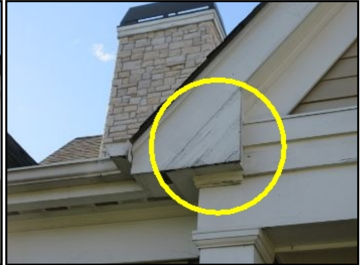
Bargeboards show signs of weathering.
