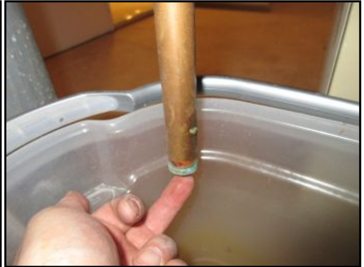
TPR valve (pipe on left) observed to leak into a basin at the floor.
