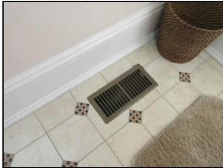
Floor supply grille may be subject to water entry.
