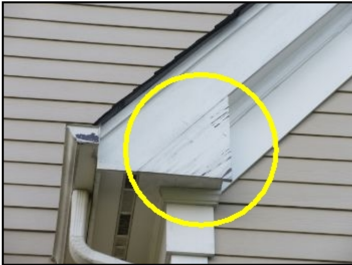
Bargeboards show signs of weathering.
