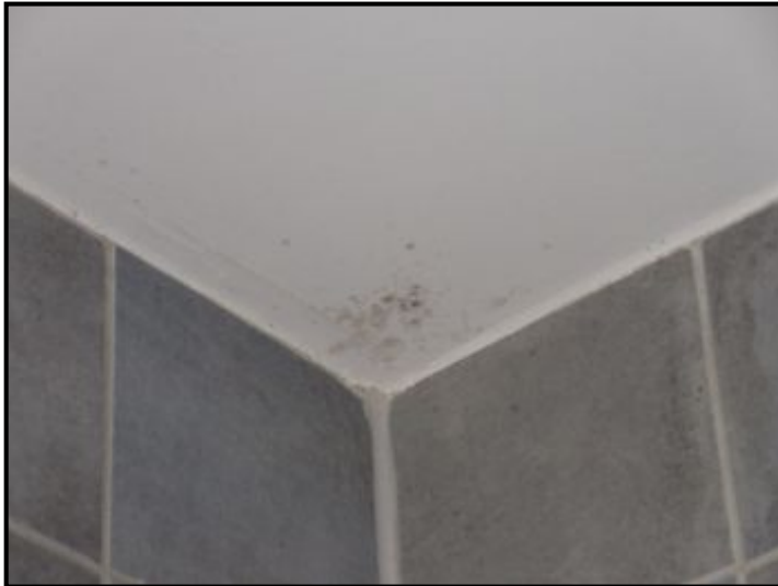
Signs of mildew noted at ceiling above tub.
