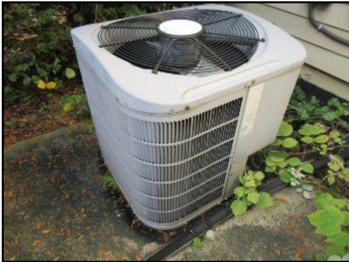
AC-4 condensing unit provides cooling; works in conjunction with the air handler located in the basement and serves the 1st floor (north-side).
