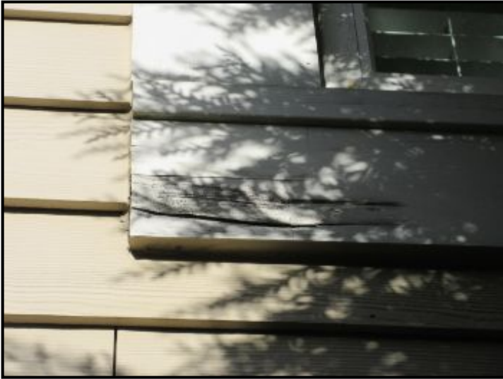
2nd floor window trim shows signs of water damage. Repairs and proper painting is recommended.
