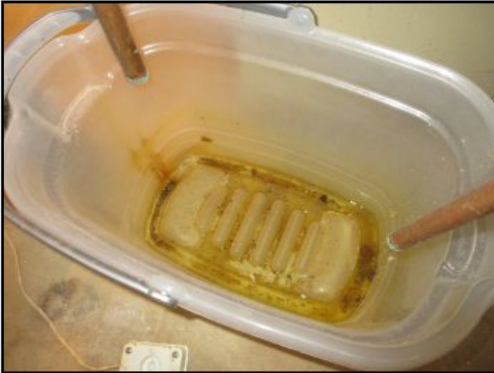
TPR valve (pipe on left) observed to leak into a basin at the floor.
