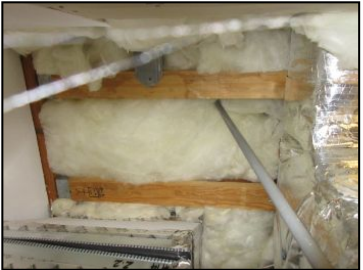
Floor Structure (above AC-4 closet): Engineered Joists - Laminated Veneer Lumber (LVL) or (Microllam) used. 16" O.C. Floor joist cavities are insulated.
