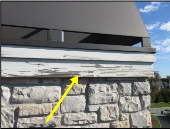
Chimney cap trim in need of paint update.
