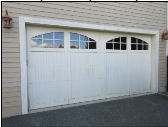
Garage wooden door shows signs of deterioration.
