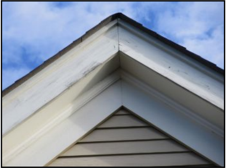
Peak bargeboards and trim in need of paint update.
