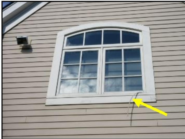
Window bottom weatherstripping had come loose and hanging.
