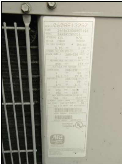
AC-1 condensing unit data plate/serial no. indicates a cooling capacity of 3 tons, and a manufacture date of 11/2007, (10 yrs old).
