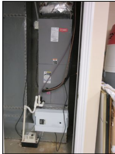
AC-4 air handler located in the basement serves the 1st floor (north-side).
