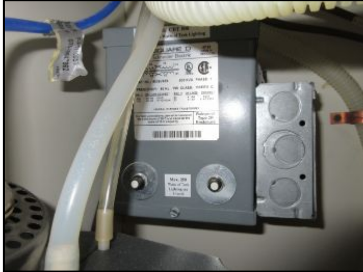
Step down transformer for counter top task lighting.
