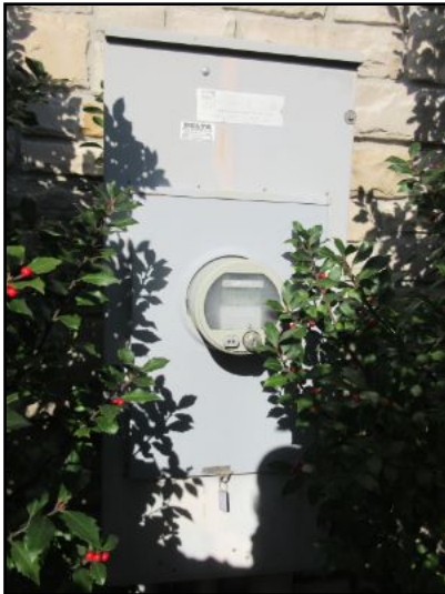
Electrical service meter.
