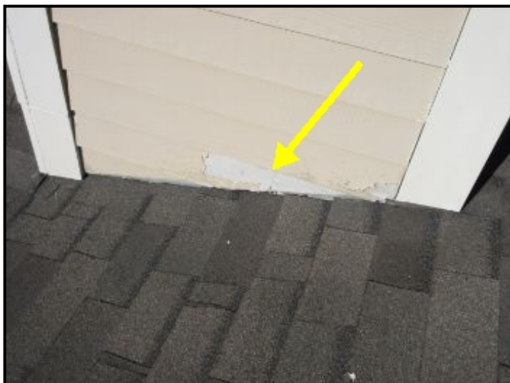
Fiber-cement siding has cosmetic damage at north chimney.
