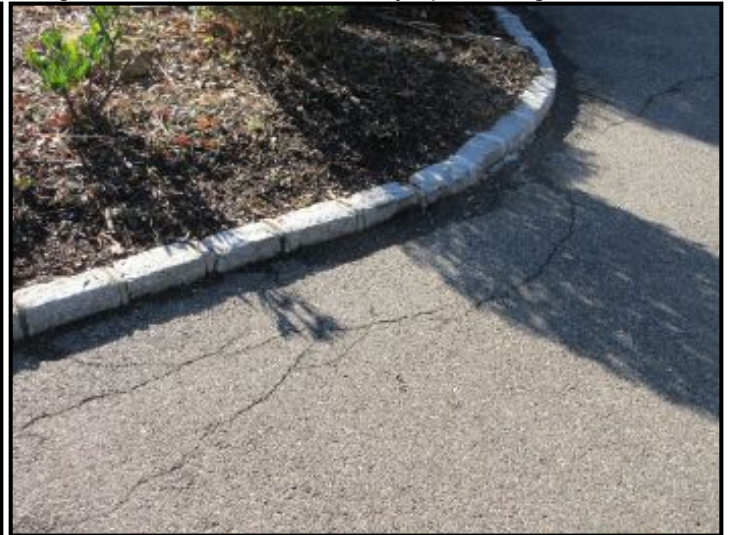
Asphalt driveways require sealing every 3-5 yrs to prevent freeze/thaw damage.
