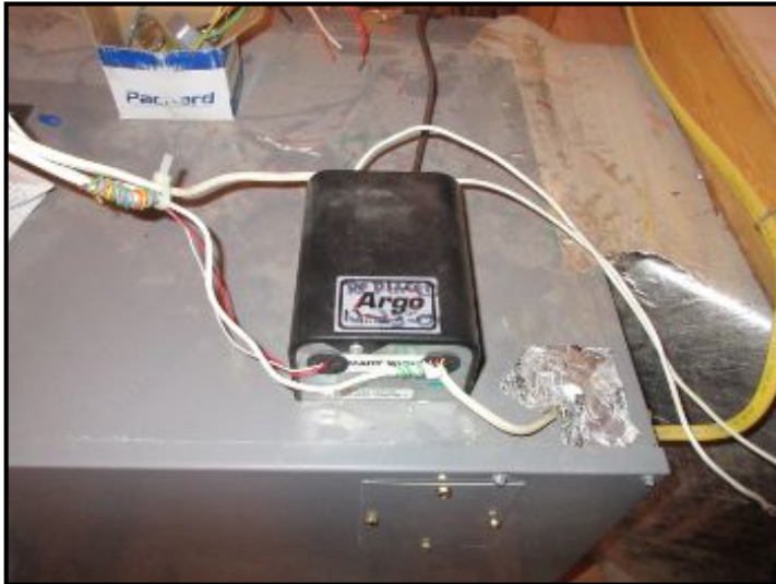
AC-2: HW heating coil controller.
