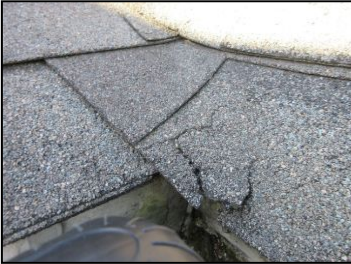
Some cracked shingles noted.
