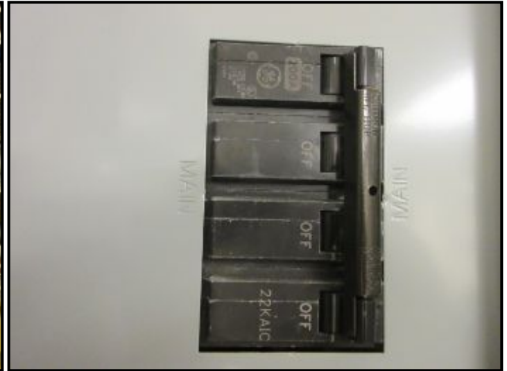
Each panel is fed through its 200 amp main breaker respectively.
