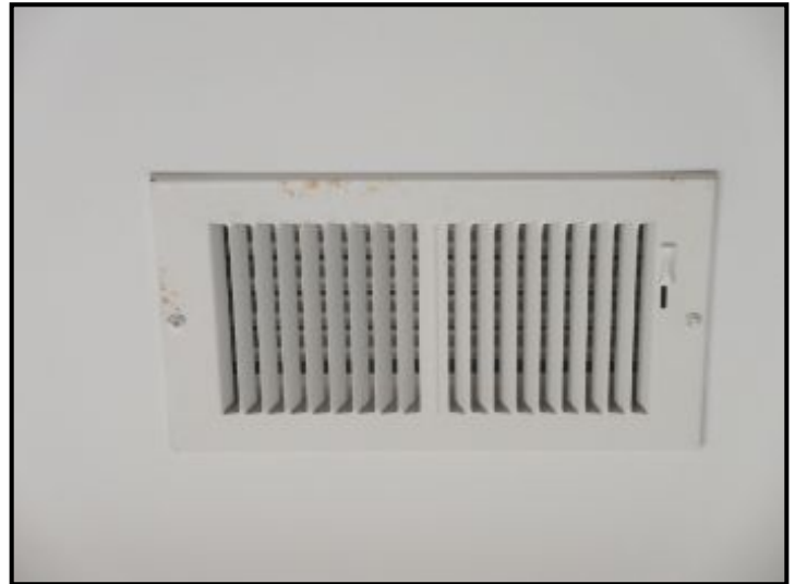
Condensation stains on supply register.
