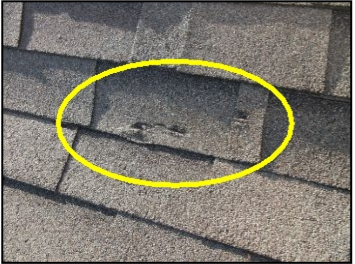
Surface damage noted at roof shingle.
