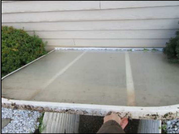
Basement emergency egress with ladder functional (with rain cap) noted at 2 places.
