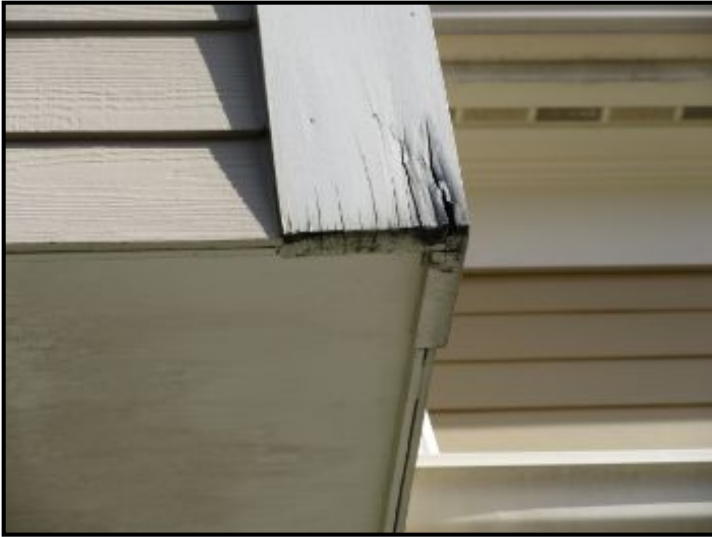
Wood trim show signs of water damage at rear of house due to a lack of protection from the elements. Repairs and proper painting is recommended.
