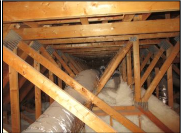
Roof Structure: Built using prefabricated components. Various truss assemblies with gusset connections effectively support the roof structure.
