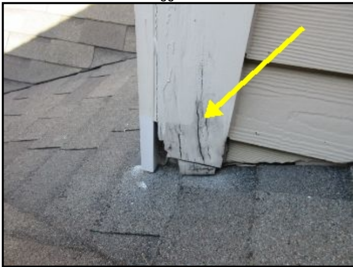
Chimney corner trim shows signs of water damage at base where in contact roofing. A 1" gap is recommended between roofing and wood trim to reduce water absorption and subsequent deterioration of the wood. Repairs and painting suggested.
