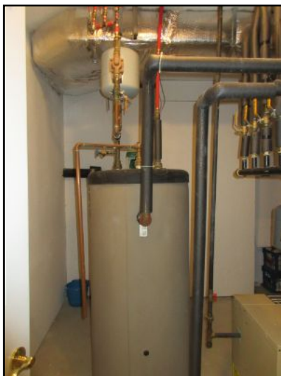
70 gal. domestic HW Storage Tank is integral with heating system in boiler room.
