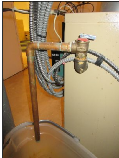
TPR valve leaks into a basin at the floor. This usually means that either the TPR valve, or the expansion tank is defective. Otherwise, the supply water regulator is either missing or it's not adequately reducing the supply water pressure to the boiler system. We recommend a licensed HVAC contractor review and repair as necessary to stop TPR valve leakage.
