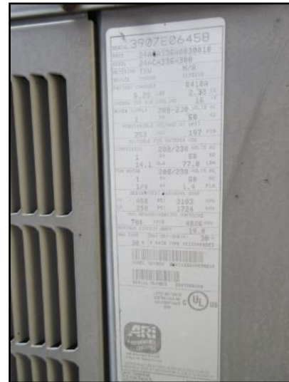
AC-2 split system data plate/serial nos. indicate a cooling capacity of 3 tons, and a manufacture date of 9/2007, (10 yrs old).
