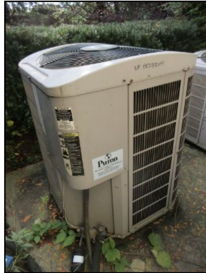
AC-2 condensing unit provides cooling; works in conjunction with the air handler located in the attic and serves the 2nd floor (south-side/bedrooms).
