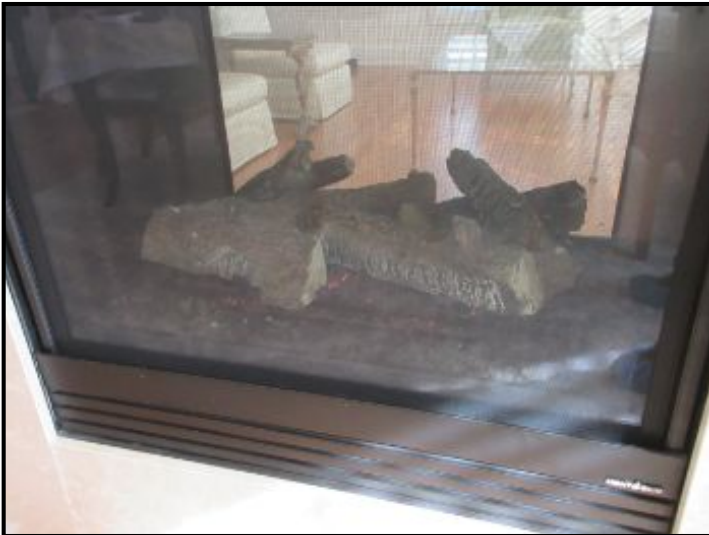
Gas Fireplace was operable and vented. Enclosure intact and complete.
