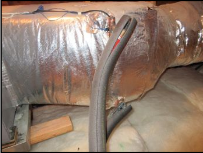
AC-5: HW heating coil.
