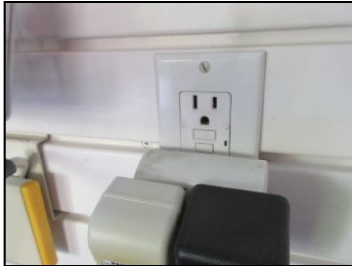
Garage GFCI protection noted.
