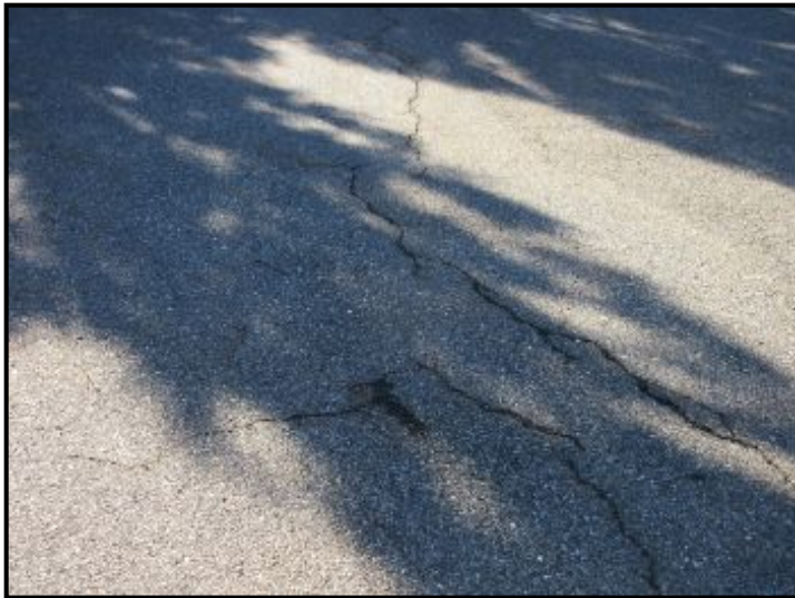
Moderate cracks in asphalt driveway. Suggest maintaining/sealing cracks to prevent wayer entry and freeze/thaw damage.
