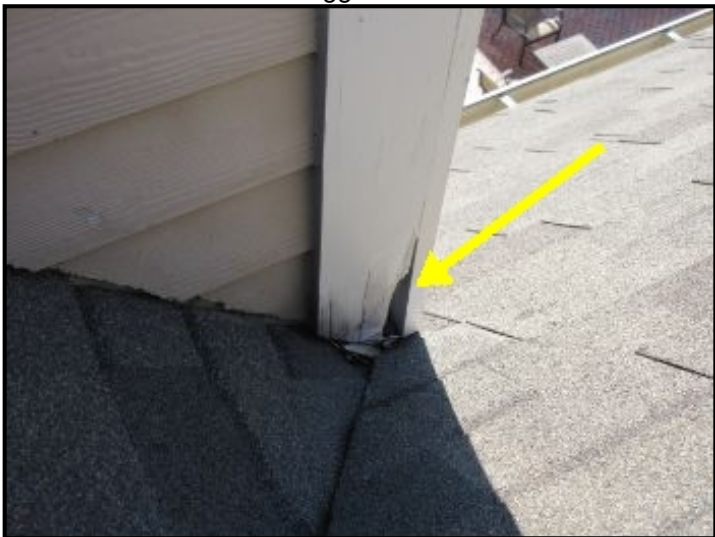
Chimney corner trim shows signs of water damage at base where in contact roofing. A 1" gap is recommended between roofing and wood trim to reduce water absorption and subsequent deterioration of the wood. Repairs and painting suggested.
