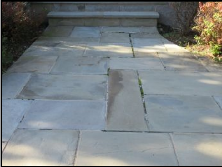
Bluestone walkways: Mortar cracked/missing observed. Suggest repair/replacement of defective mortar joints.
