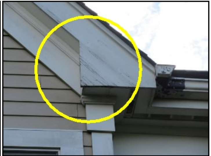
Bargeboards show signs of weathering.
