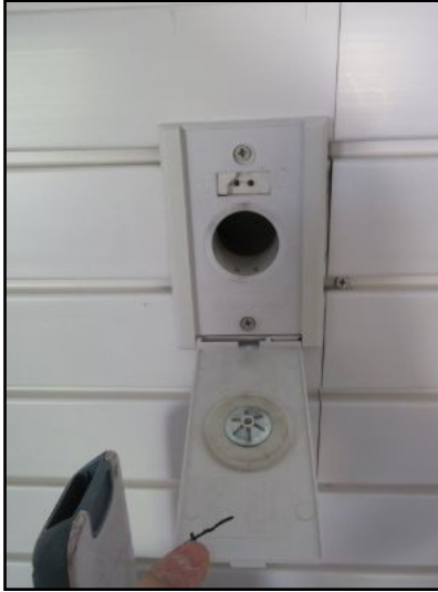
Garage central vacuum hose connection noted.
