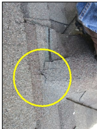
Some cracked shingles noted.
