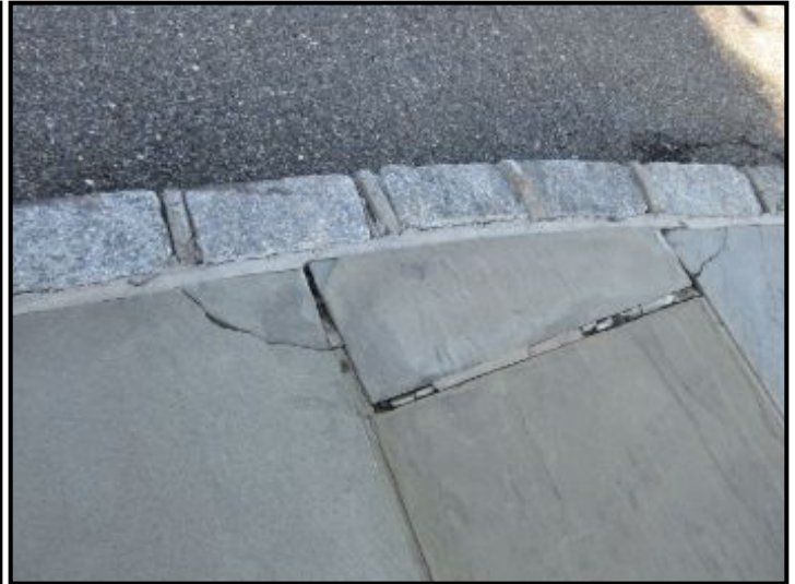
Cracked/missing mortar and cracked flags observed. Suggest mortar repairs and replacing cracked flags.
