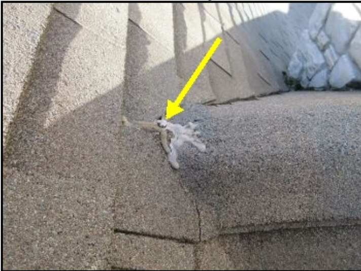
Exposed nails on roofing material. Maintain seal at all fastener heads.
