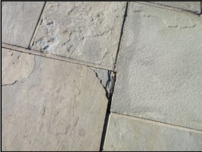
Bluestone walkways: Few cracked flags observed. Suggest repair/replacement of cracked flags.
