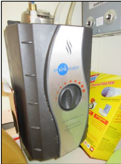
Hot water dispenser was inoperable.
