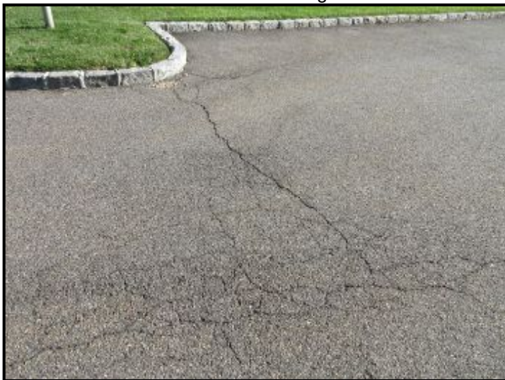
Moderate cracks in asphalt driveway. Suggest maintaining/sealing cracks to prevent wayer entry and freeze/thaw damage.
