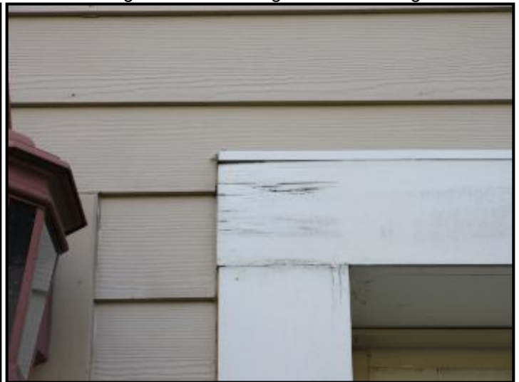
Wood trim at garage door show signs of water damage due to a lack of protection from the elements.
