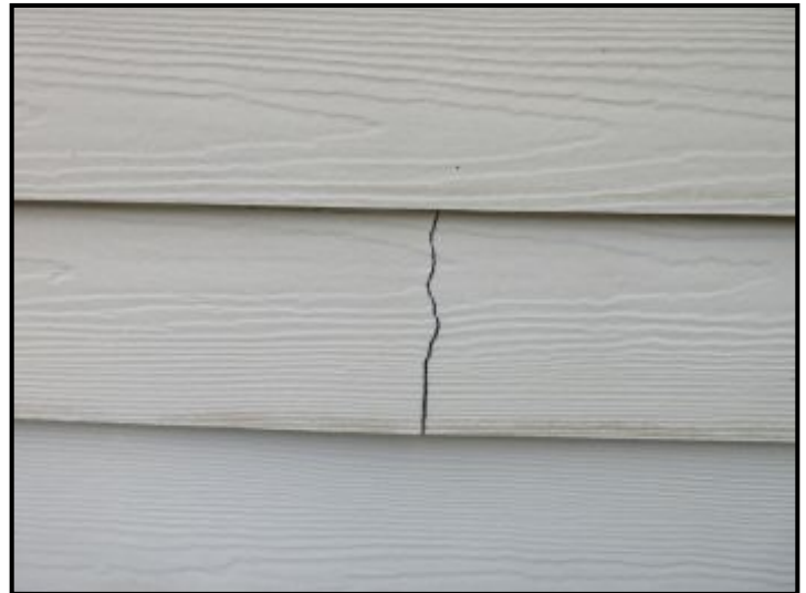
Cracked fiber-cement siding course at rear. Suggest repair.
