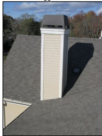
Two chimneys are metal flue pipe enclosed in an architectural chase.
