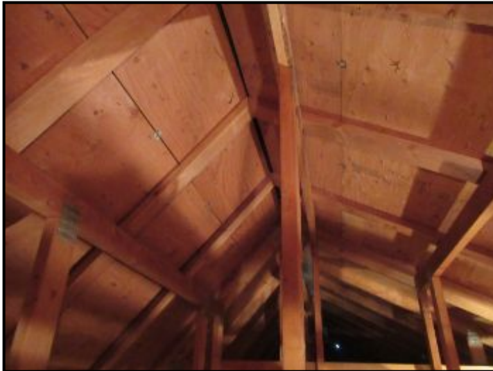
Roof boards appeared dry and unstained.
