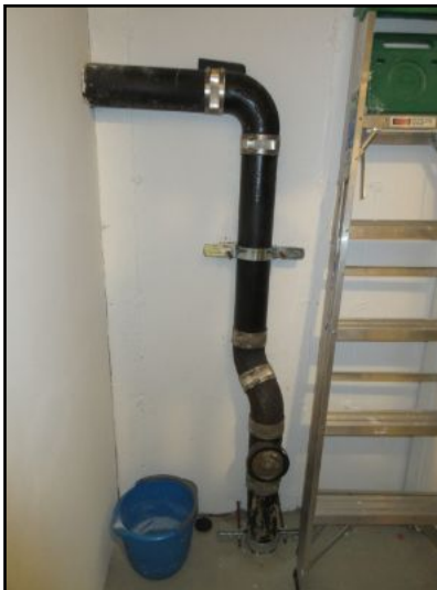
Sanitary waste pipe exit with clean-out located in boiler room.
