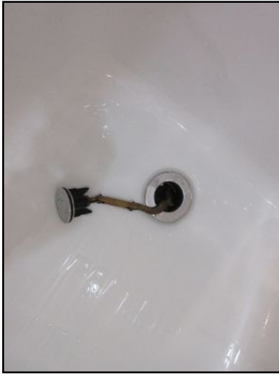
Tub stopper linkage was detached; suggest repair.
