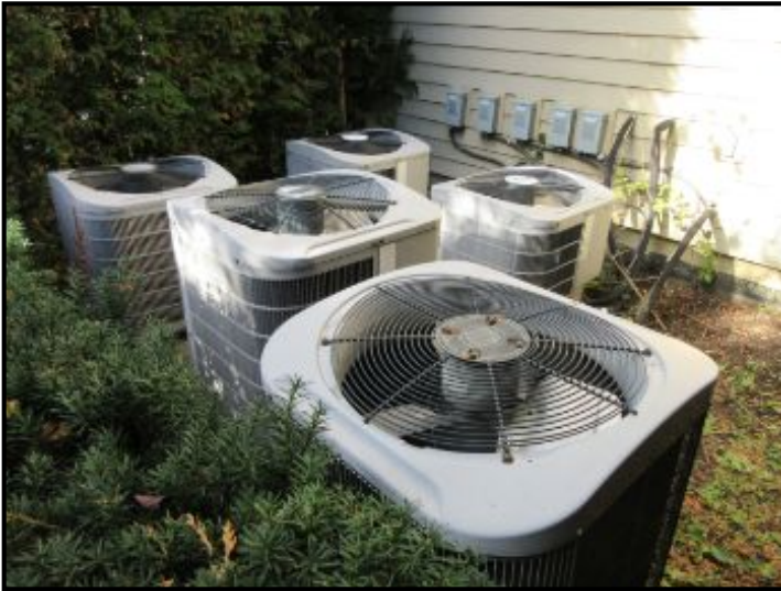
Multiple Central A/C split-systems (AC-1,2,3,4 & 5 clockwise) each with outdoor condenser and indoor ducted air handler.
