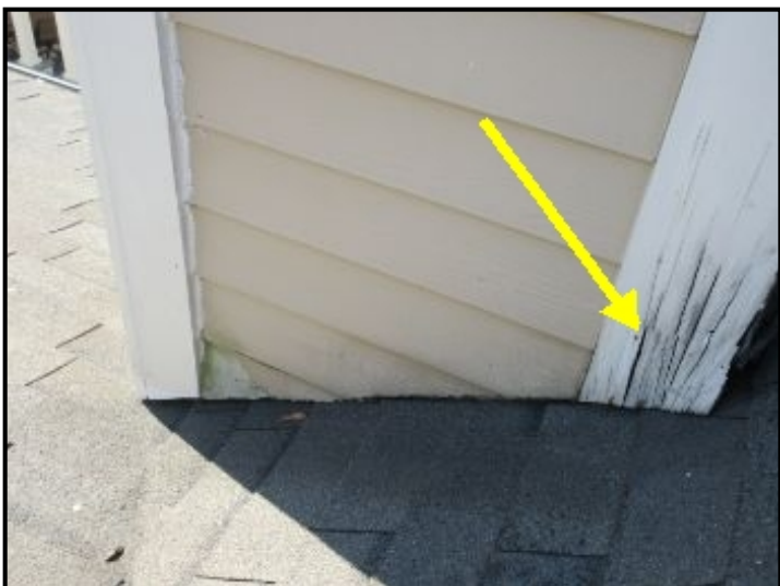
Chimney corner trim shows signs of water damage at base where in contact roofing. A 1" gap is recommended between roofing and wood trim to reduce water absorption and subsequent deterioration of the wood. Repairs and painting suggested.
