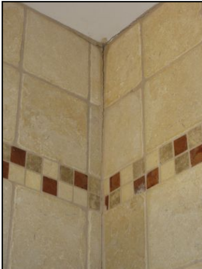
Grout cracked at tub left wall corner joint due to movement. This is common; suggest replacing grout with matching silicone based sealant at corner movement joints.
