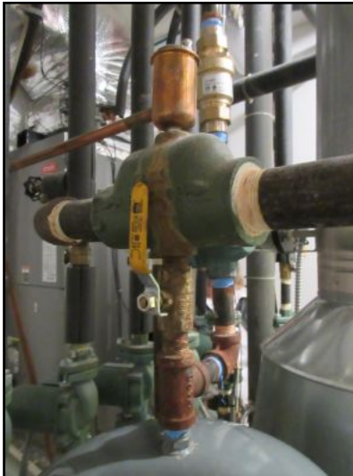
Automatic air vent atop air separator fitting shows signs of leakage, rusting steel pipe surfaces. This may also be caused by the same concerns relative to the TPR valve leak.
