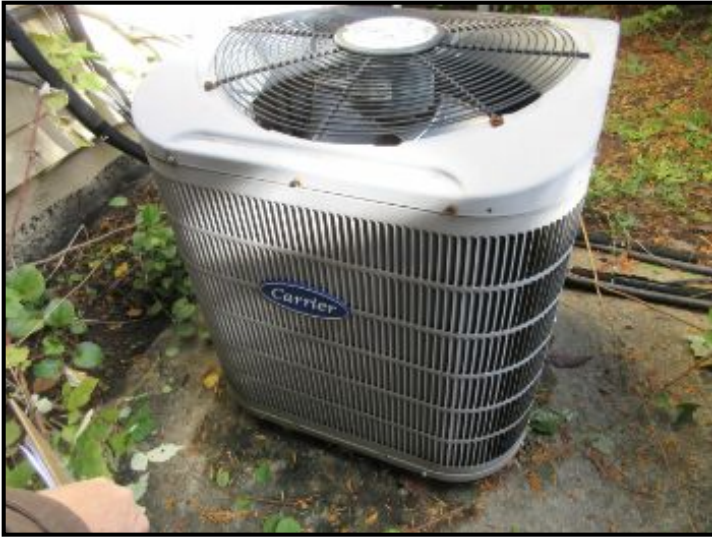
AC-5 condensing unit provides cooling; works in conjunction with the air handler located in the attic and serves the 2nd floor (north-side/bedrooms).
