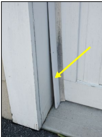
Garage door weather stripping coming loose at left side of larger door.
