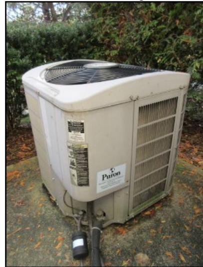
AC-3 condensing unit provides cooling; works in conjunction with the air handler located in the basement and serves the 1st floor (south-side).
