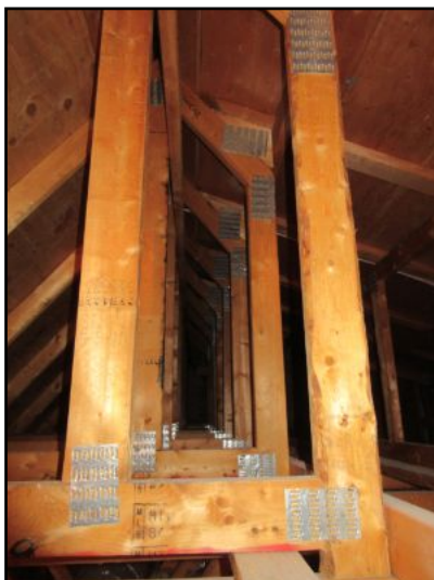
Roof Structure: Built using prefabricated components. Various truss assemblies with gusset connections effectively support the roof structure.
