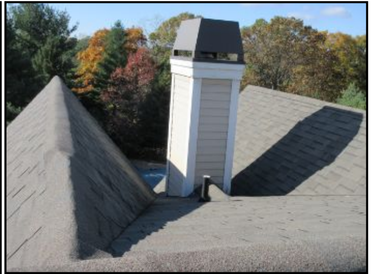
Two chimneys are metal flue pipe enclosed in an architectural chase.
