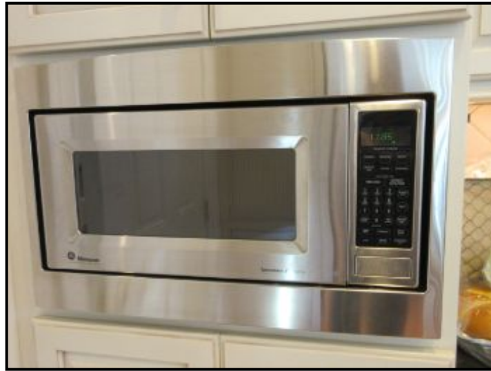
Built-in microwave oven operable.
