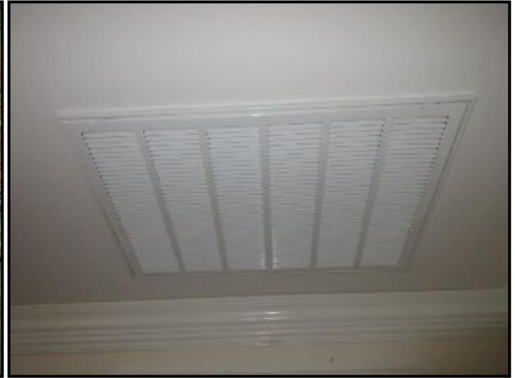
Return air filter/grille believed to be for AC-5 air handler.
