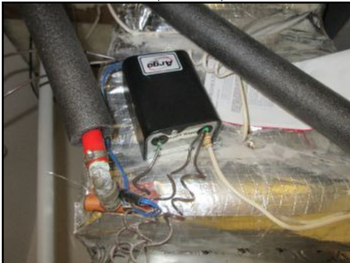
AC-3: HW heating coil and controller.
