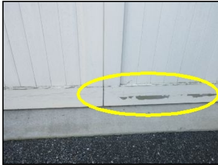
Garage wooden door shows signs of deterioration.
