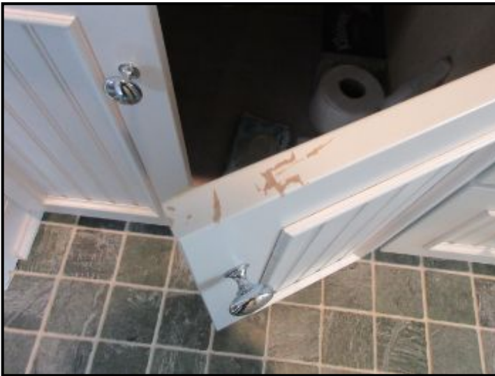
Vanity door finish shows signs of wear.
