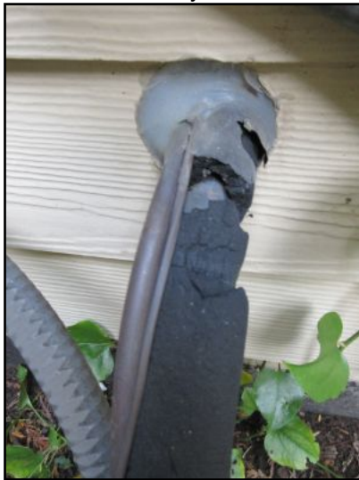
Refrigerant pipe insulation is deteriorated/missing at outdoor condensers. Recommend replacing outdoor deteriorated/missing insulation on the larger suction lines only.
