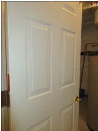
Fire resistant boiler room door in accordance with NFPA requirement.
