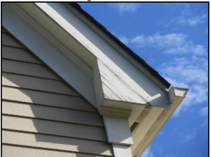
Bargeboards show signs of weathering.
