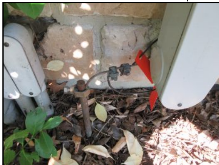
Grounding noted at service entrance.
