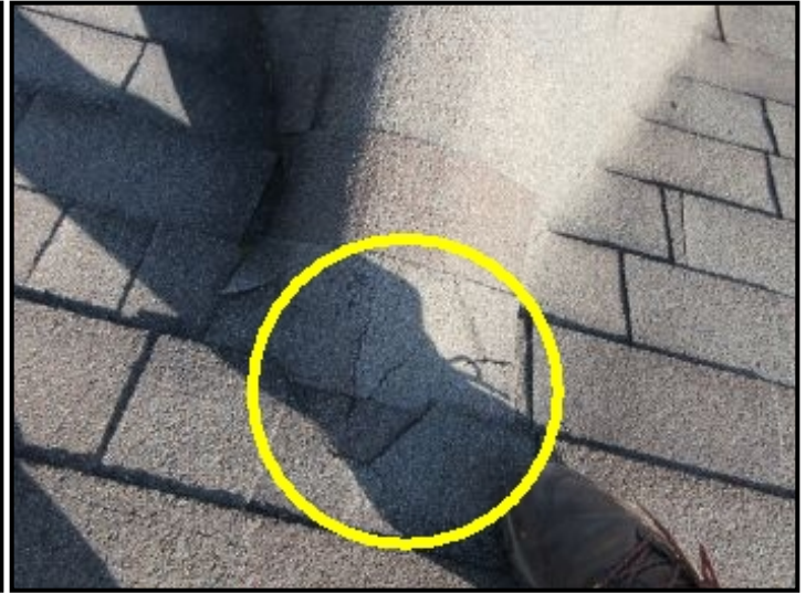
Some cracked shingles noted.
