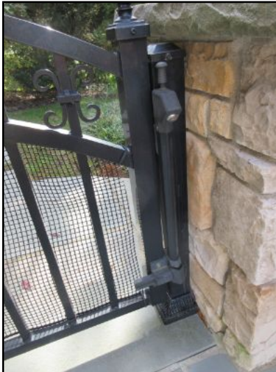
Patio south gate appeared to be locked at time of inspection.
