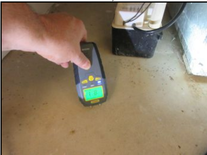
AC-3 air handler closet floor moisture reading was "Low".
