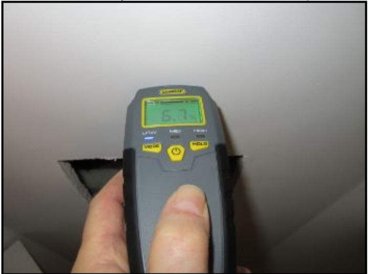
Moisture measurements taken at water service entrance in the basement indicated "Low" moisture levels (left blue light on meter).
