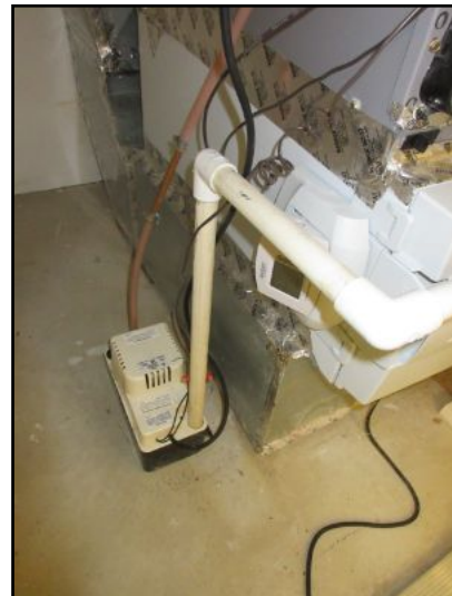
AC-3: condensate pump appeared operational.
