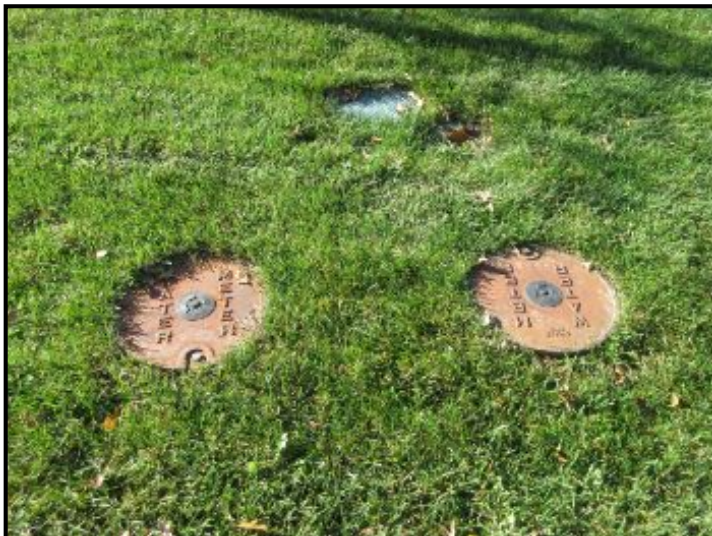
Water meter access at front lawn.
