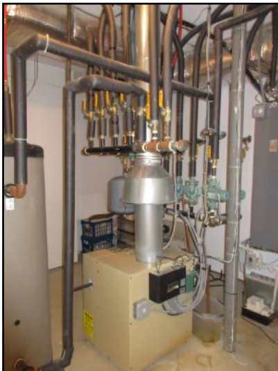
Gas-fired boiler plant with integral domestic HW heating system located in basement.
