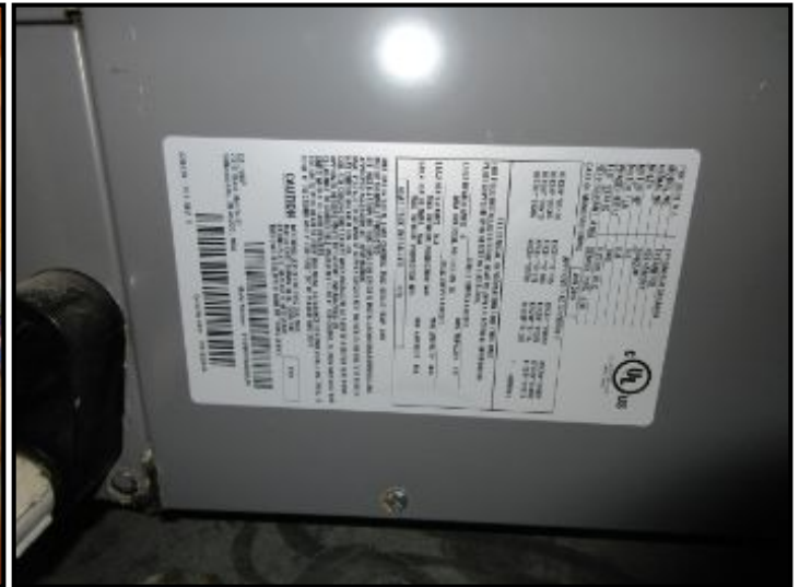
AC-2 split system has a 3 ton air handler; matched with AC-2 outdoor condenser.
