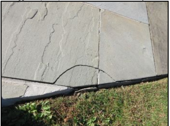
Bluestone walkways: Few cracked flags observed. Suggest replacing cracked flags.
