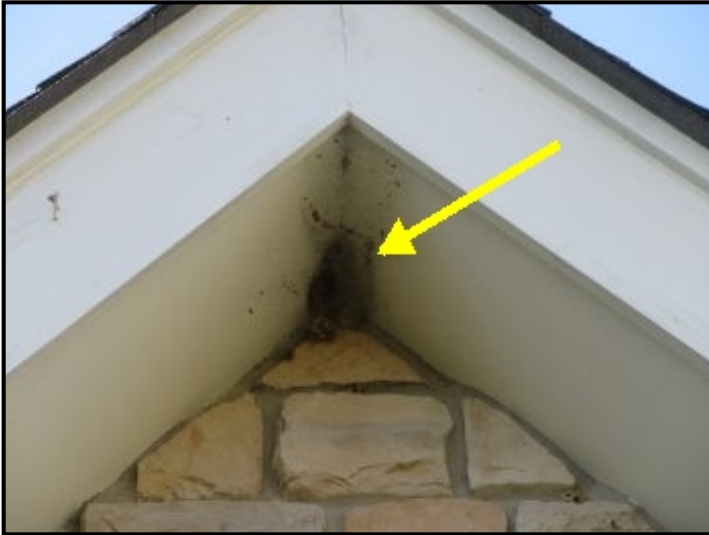
Bee's nest observed at underside of front lower peak.
