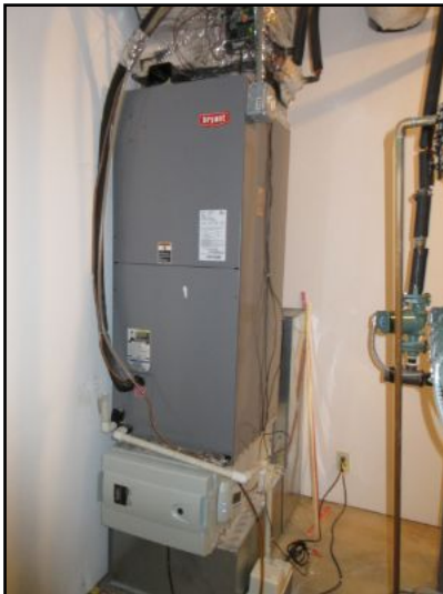
AC-1 air handler located in the boiler room serves the basement.
