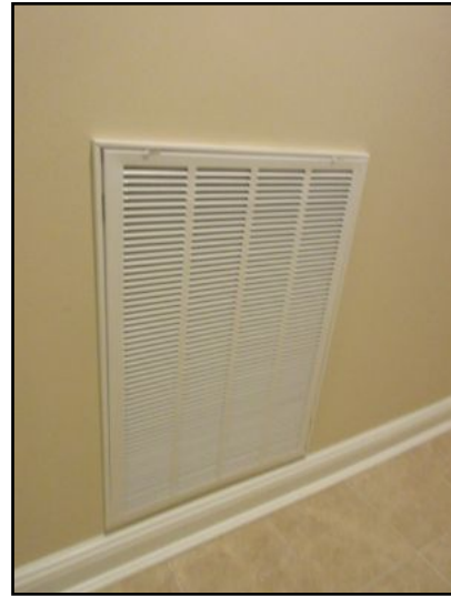
AC-1 filter return grille in basement wall.
