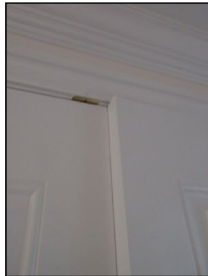
2nd floor double door closet doors bind together upon closing. Suggest door adjustment.
