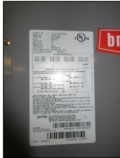
AC-3 split system has a 2.5 ton air handler; matched with AC-3 outdoor condenser.
