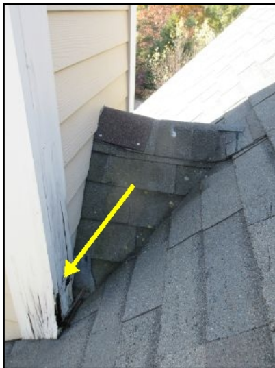
Chimney corner trim shows signs of water damage at base where in contact roofing. A 1" gap is recommended between roofing and wood trim to reduce water absorption and subsequent deterioration of the wood. Repairs and painting suggested.
