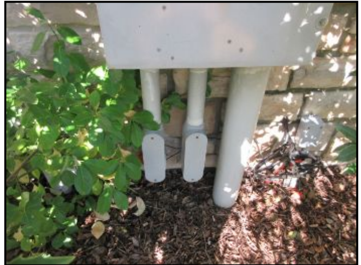
Underground service lateral (120/240 volts) feeds the two panels in basement.
