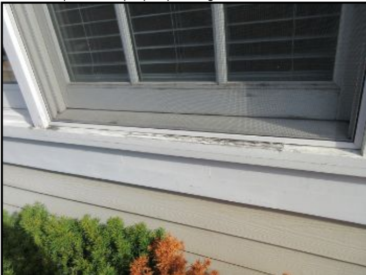
Window sills and trim in need of paint updates.
