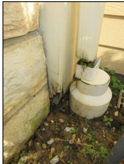
Downspout not connected to dry well inlet causing water damage to wood trim.
