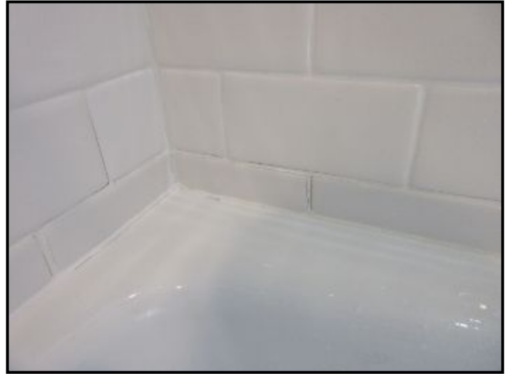
Grout slightly damaged/missing at wall tile at tub corner. Suggest grout repair to prevent water entry.
