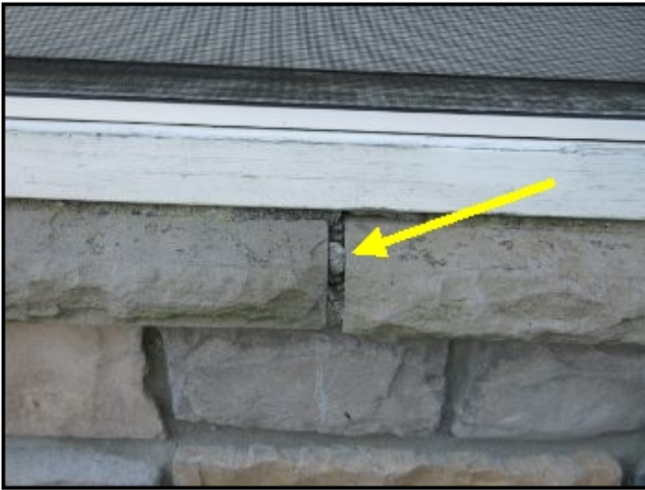
Stone veneer at front has a few gaps in the mortar joints. Suggest filling gaps with matching mortar to prevent water entry and freeze/thaw damage.
