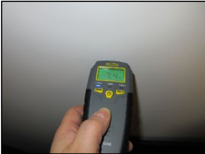
Moisture measurements taken at sample locations in the basement indicated "Low" moisture levels (left blue light on meter).
