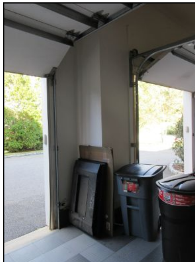
Garage vehicle door openers -- both operable.
