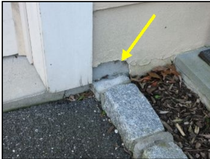
Cosmetic defect at synthetic stucco by garage door.
