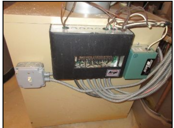
Pump control panel at boiler.
