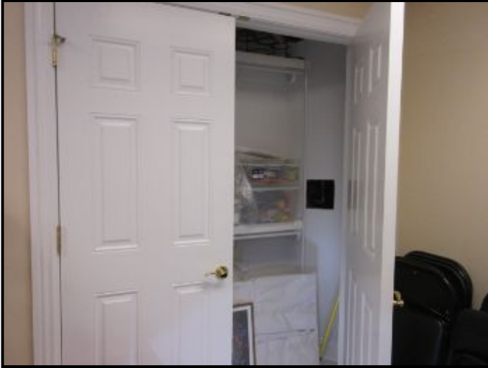
Public water service entrance located in basement storage room closet at front wall.
