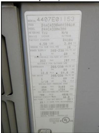
AC-4 split system data plate/serial nos. indicate a cooling capacity of 2.5 tons, and a manufacture date of 11/2007, (10 yrs old).
