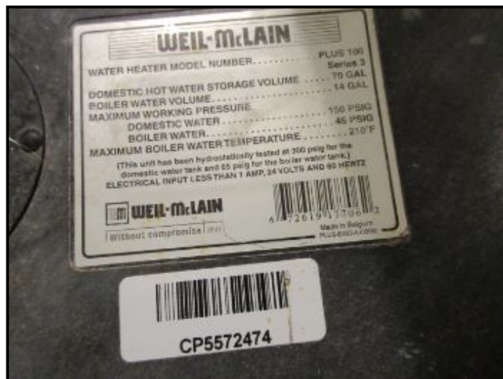
Water Heater was installed with the boiler and is 10 yrs old. Water Heater service life expectancy is normally up to 20 yrs. for this type of unit.
