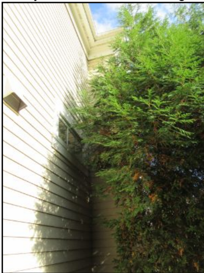
Recommend trimming back vegetation from contact with gutter and roof shingles to prevent damage to the house.
