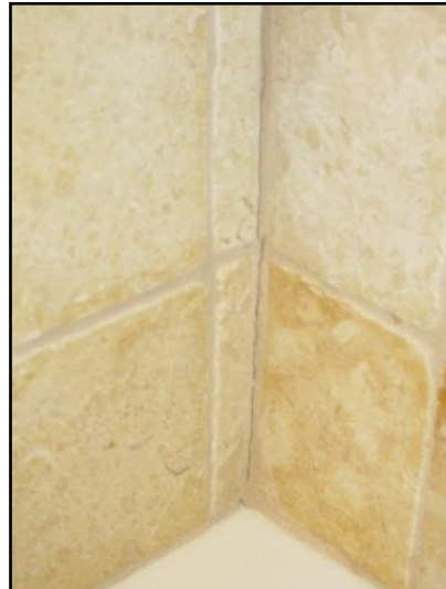
Grout cracked at tub left wall corner joint due to movement. This is common; suggest replacing grout with matching silicone based sealant at corner movement joints.
