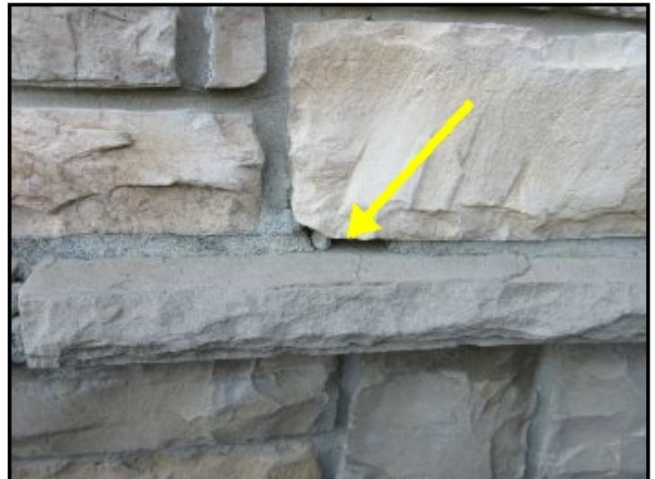
Stone veneer at front has a few gaps in the mortar joints. Suggest filling gaps with matching mortar to prevent water entry and freeze/thaw damage.
